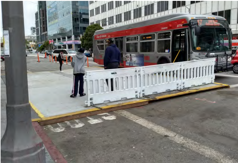
Temporary bus bulbs
