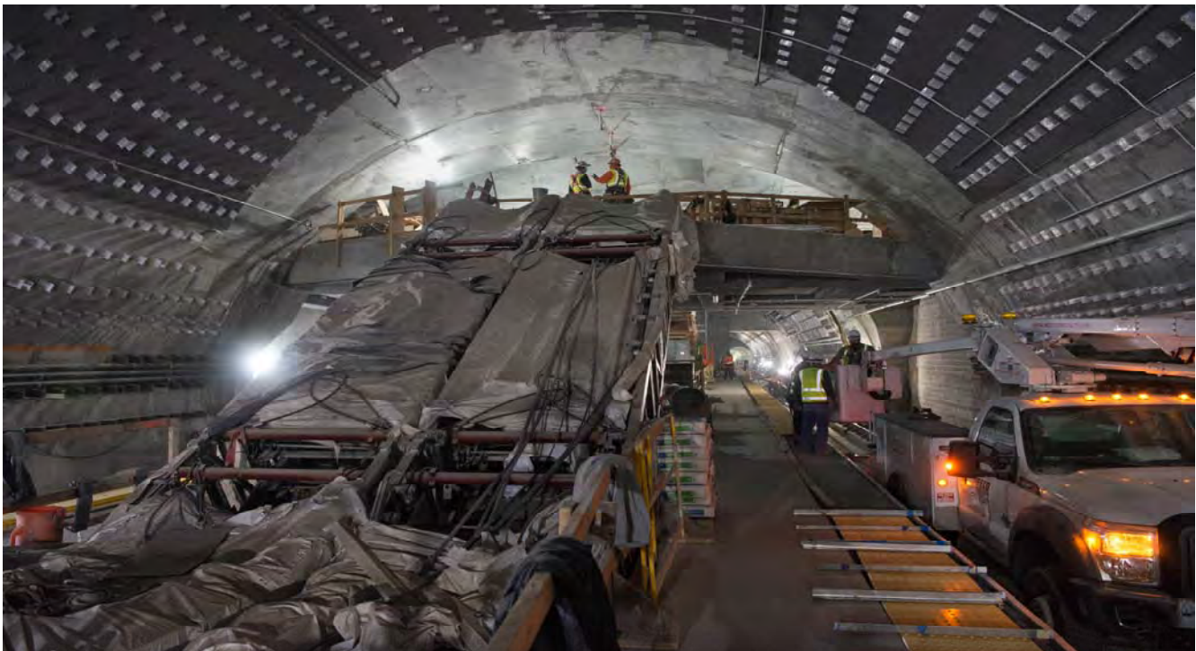
Future escalators remain covered during the installation of steel brackets across the arched ceiling and walls of the Chinatown Station platform cavern.
