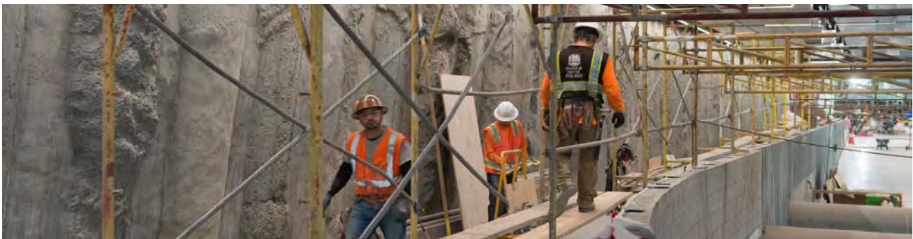
A crew disassembles scaffolding used to install ceiling panels just outside the ramp leading to escalators inside the south concourse for Union Square/Market Street Station.
