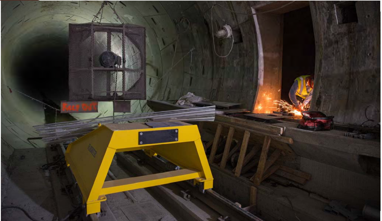
A worker makes alterations to a steel floor panel inside the entrance for one of the tunnel cross-passages, where it meets the current end of the southbound track, north of the Chinatown Station platform.
