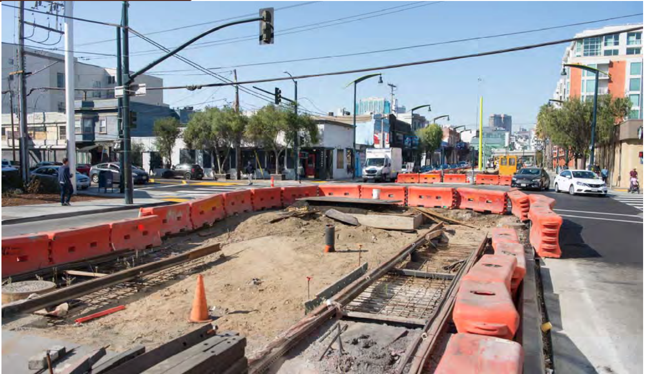
Crews are preparing to extend the dual trackways across the 4th and Brannan intersection.
