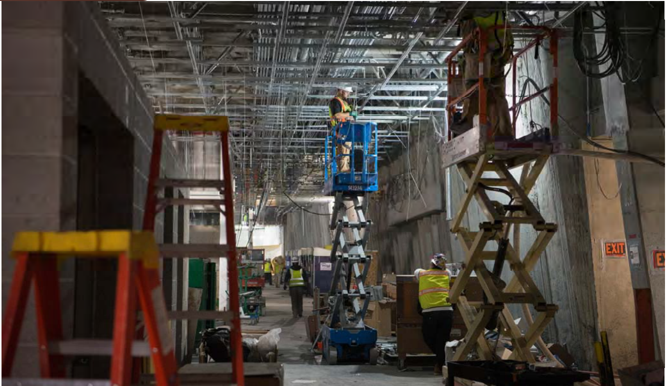
Workers hang wires which will be used to suspend ceiling panels and lighting on the east side of the Union Square/Market Street Station concourse.
