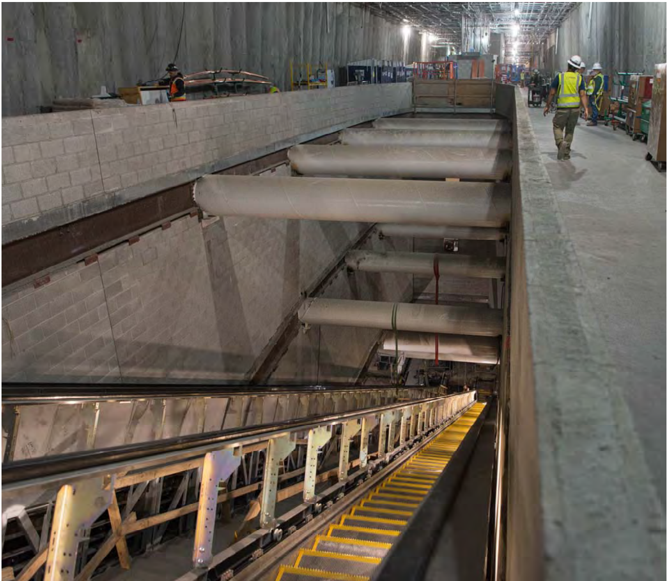
Cylindrical steel struts span across the opening in the north concourse for Union Square/Market Street Station, where recently-installed escalators span far below to the station platform.
