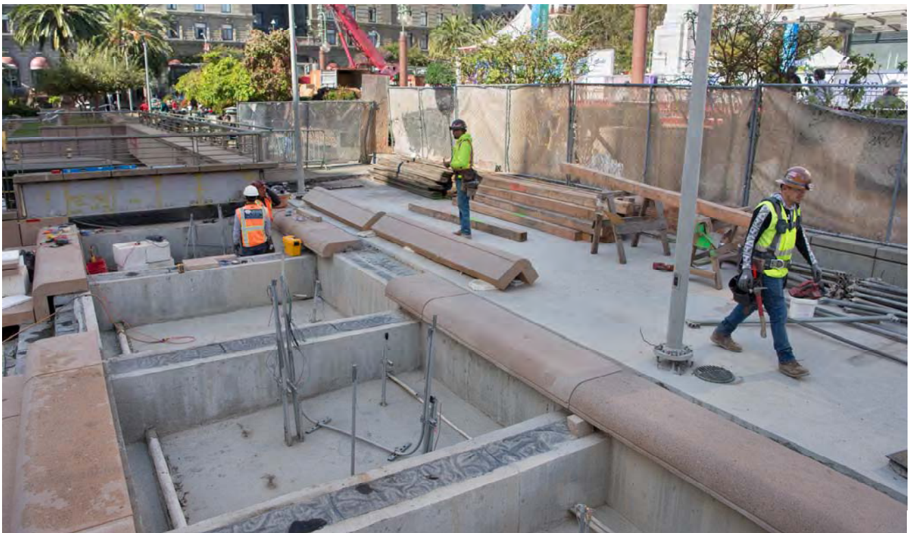
Rounded terrace blocks are being placed as part of the reconstruction of Union Square's southeast corner, adjacent to the new station entrance.
