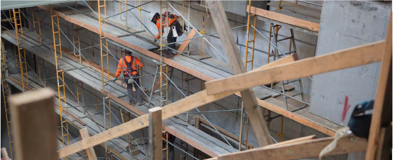
Workers assemble scaffolding along the east side of the Chinatown Station headhouse structure, where waterproofing and shotcrete work have begun.
