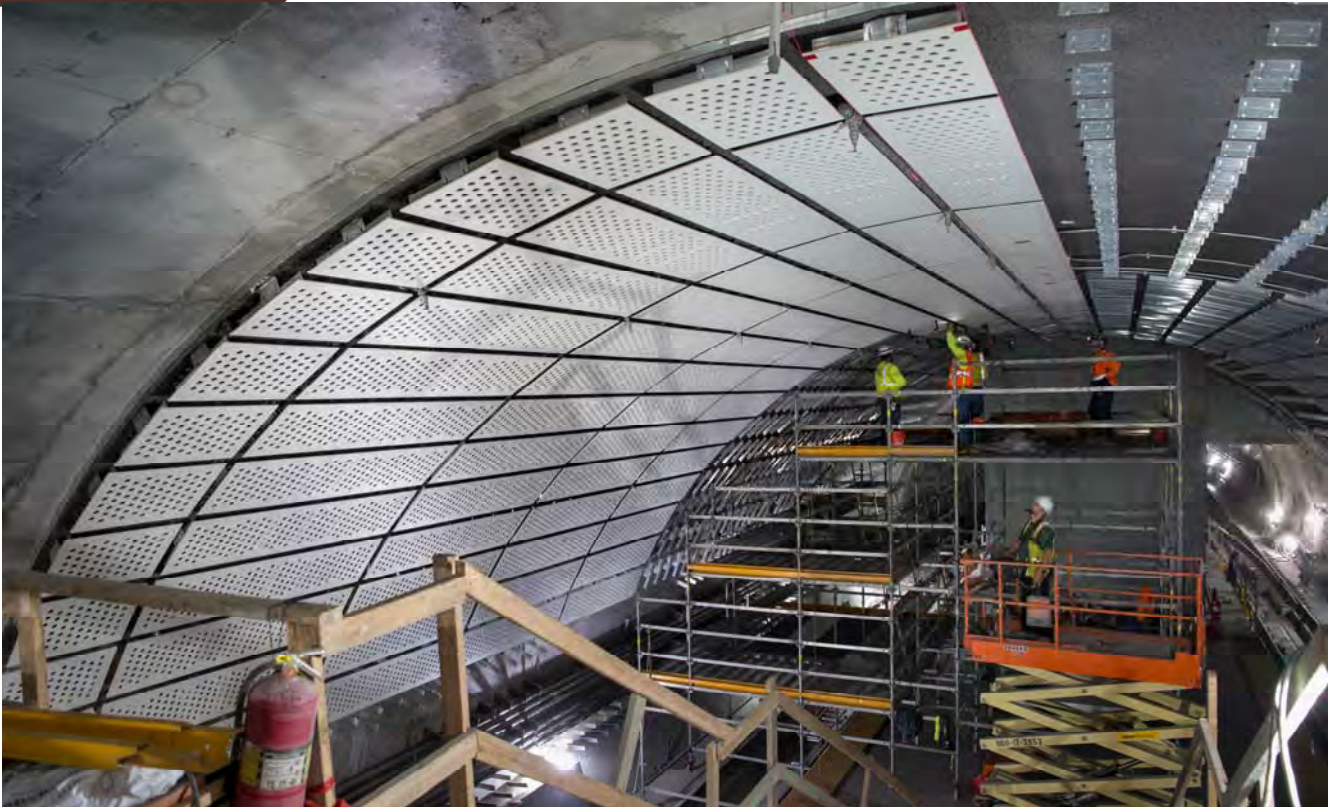
Sound reduction panels are being attached to steel brackets mounted to the arched concrete ceiling of the Chinatown Station platform cavern.
