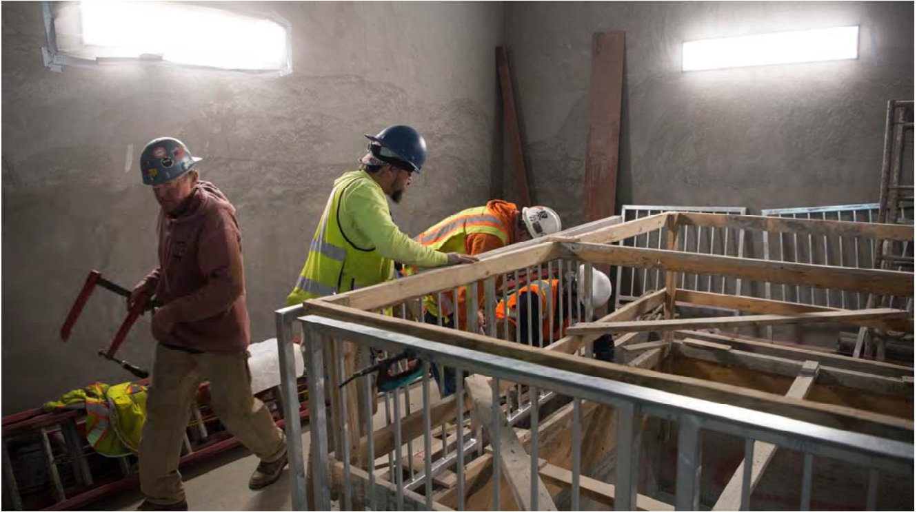
Permanent steel railing is installed around an access shaft at the north end of the Yerba Buena/Moscone Station headhouse's mezzanine level.
