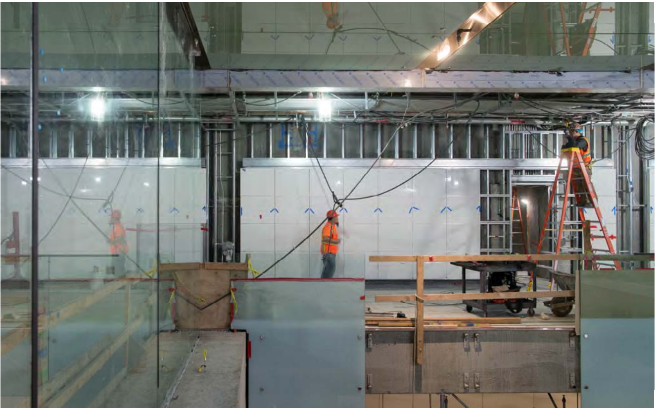
Large glass panels have been installed atop strut beams inside the concourse level of Yerba Buena/Moscone Station as part of the final station interior build-out.
