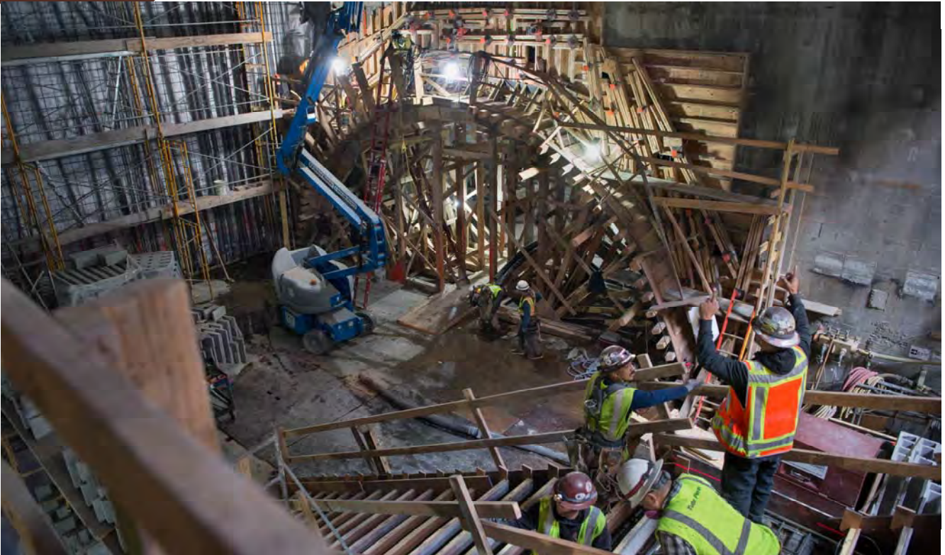
Concrete formwork has been built for the last section of arch construction at the Chinatown Station cross-cut cavern entrance, where future fare gates will be located.
