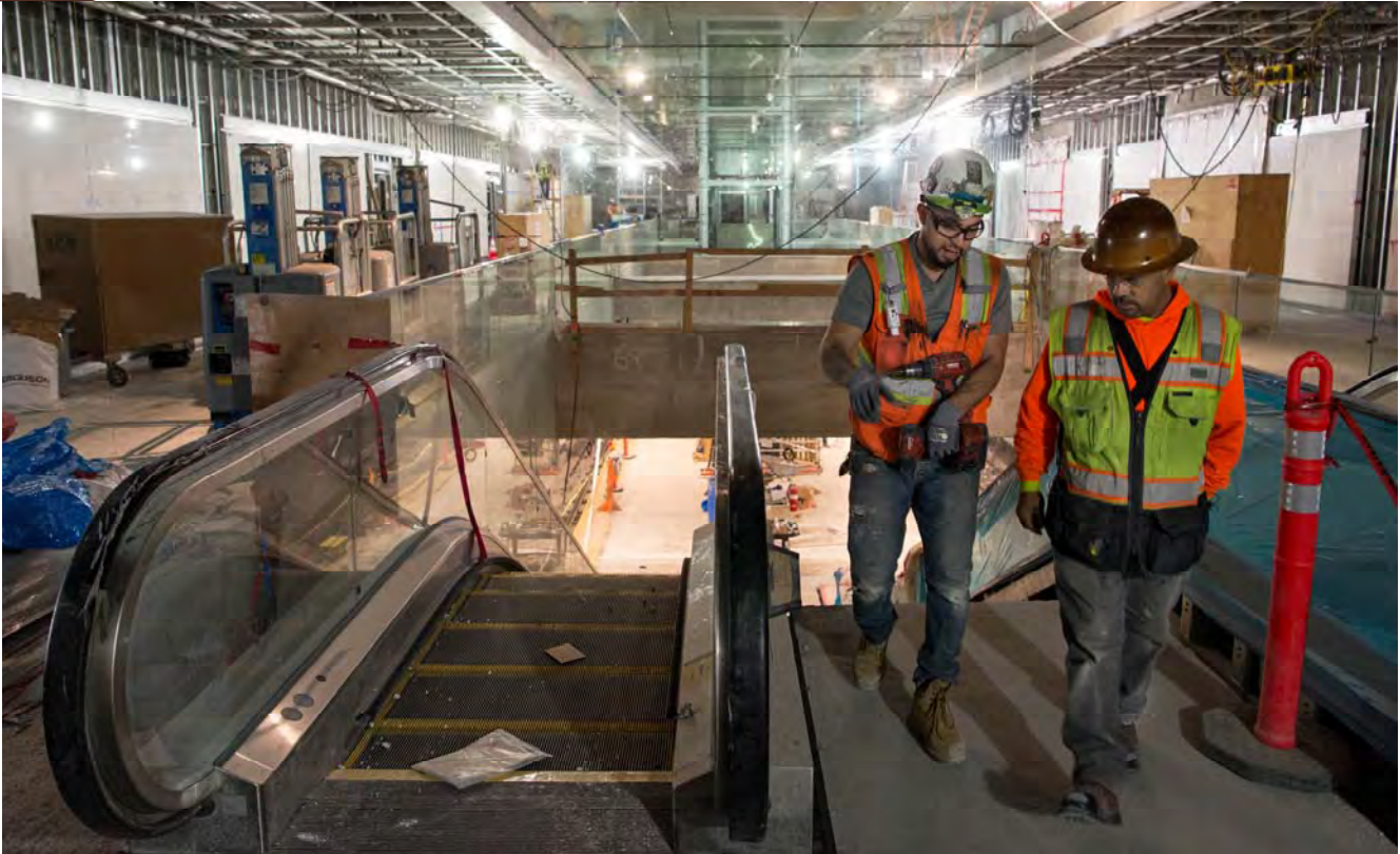
A steel lattice for installing ceiling panels and lighting is one of many interior elements being added to the Yerba Buena/Moscone Station concourse.
