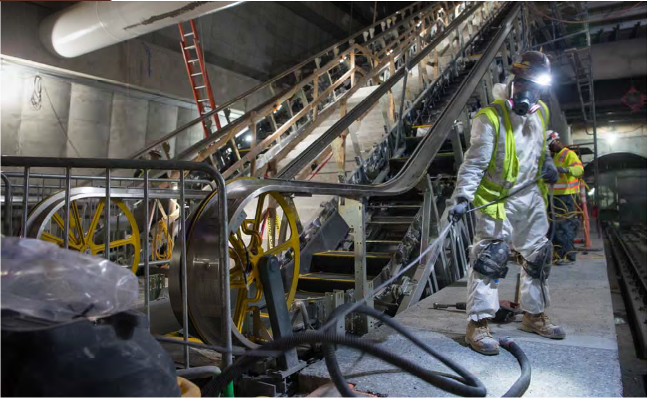
A worker untangles a power cord from a vacuum at the base of the north escalators inside the station during work to prepare the station platform for terrazzo work.
