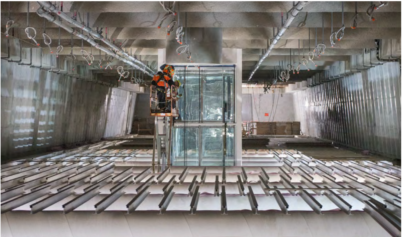
Workers on a scissor lift above the station platform install framed glass panels on the south elevator for Union Square/Market Street Station.
