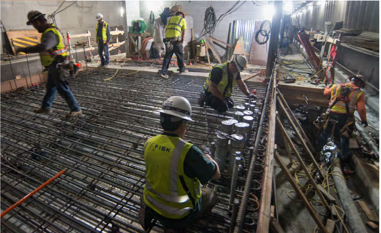
A crew installs rebar for a remaining unbuilt northern section of the Union Square/Market Street Station platform.
