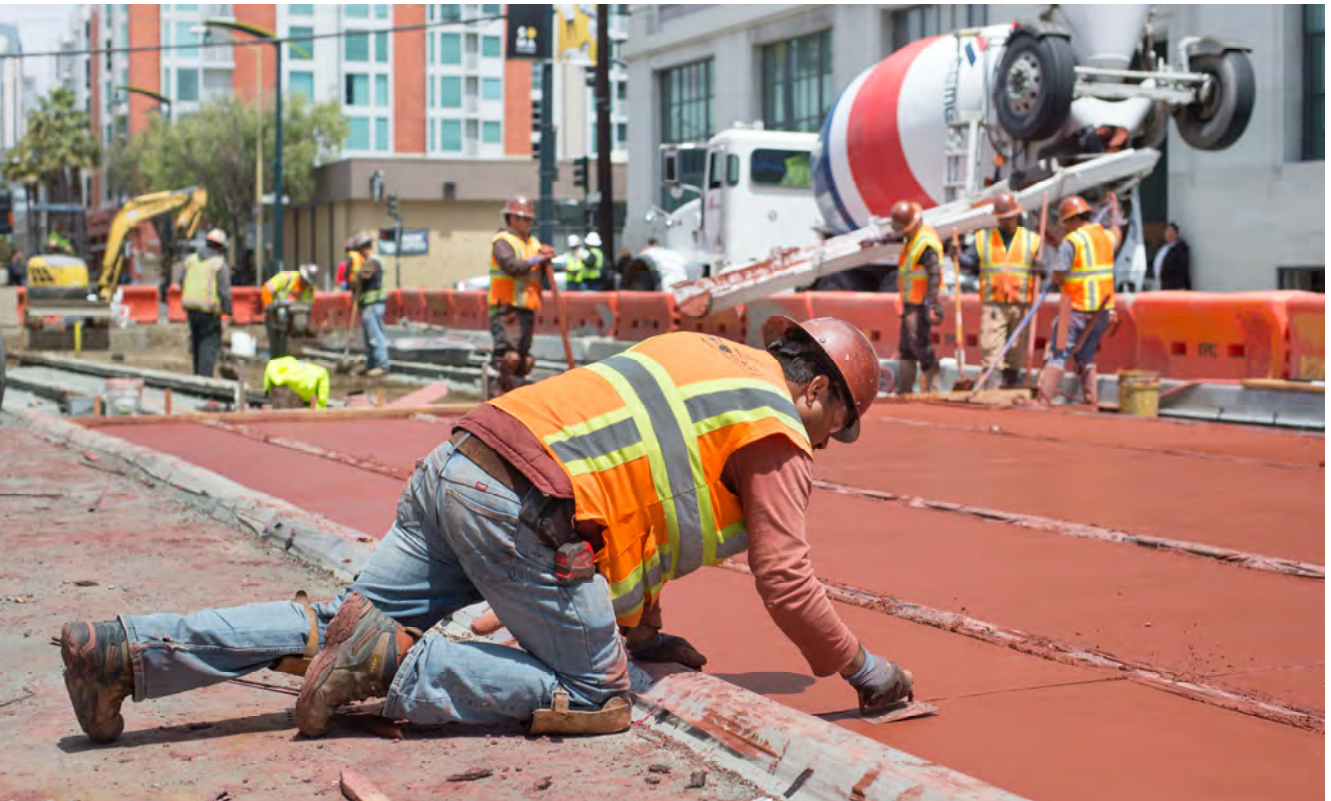
A worker smooths the edges of a recently-poured red-tinted topping slab along the surface alignment south of Brannan Street.
