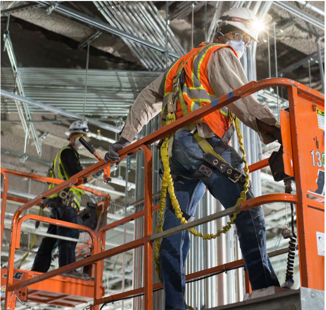
A massive tree of utility conduits sprouts from a utility shed under construction on the concourse level of Union Square/Market Street Station.
