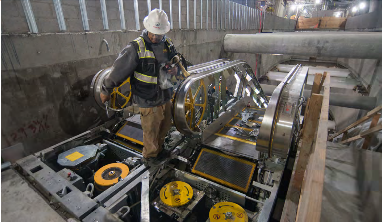
Workers install mechanical elements of the tandem escalators at the south end of the Union Square/Market Street Station's concourse.
