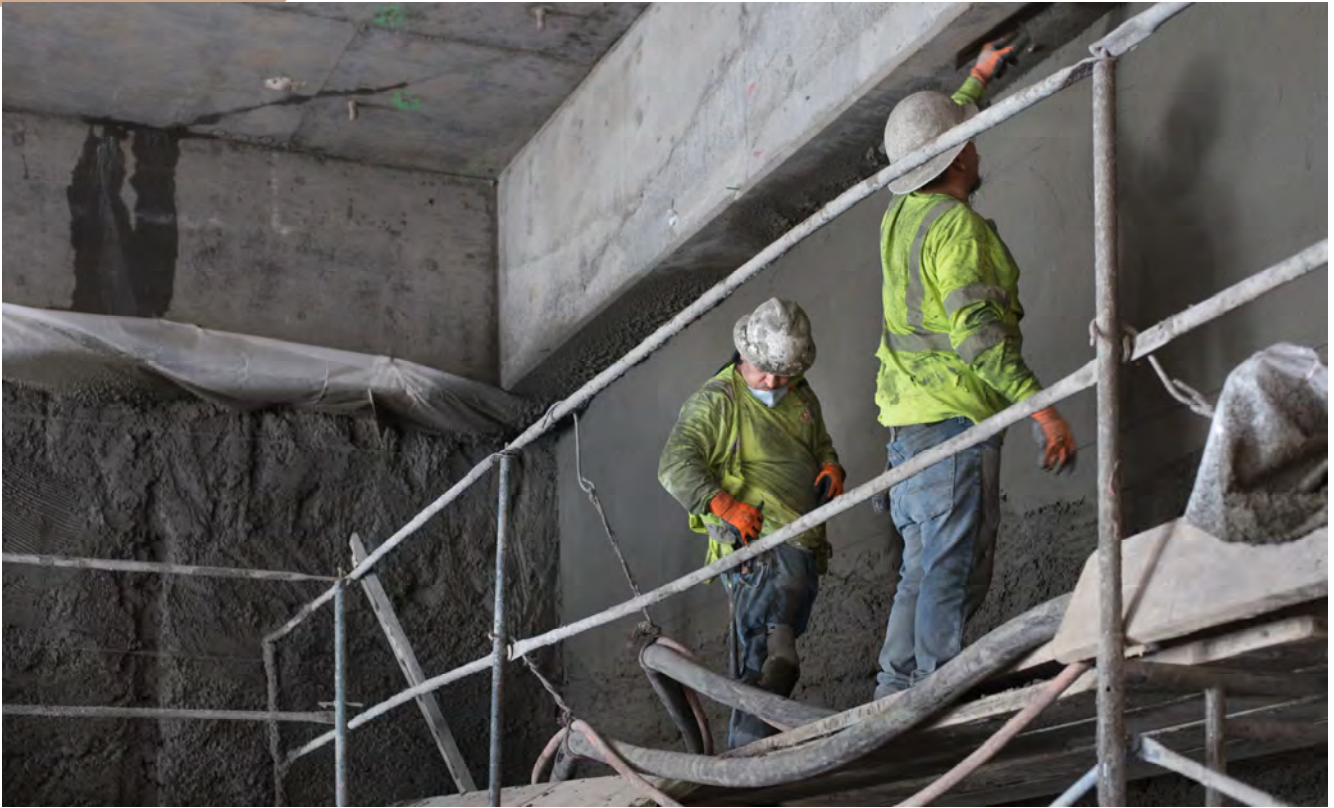
A crew smooths recently applied shotcrete at the southeast corner of the upper mezzanine level for Chinatown Station.
