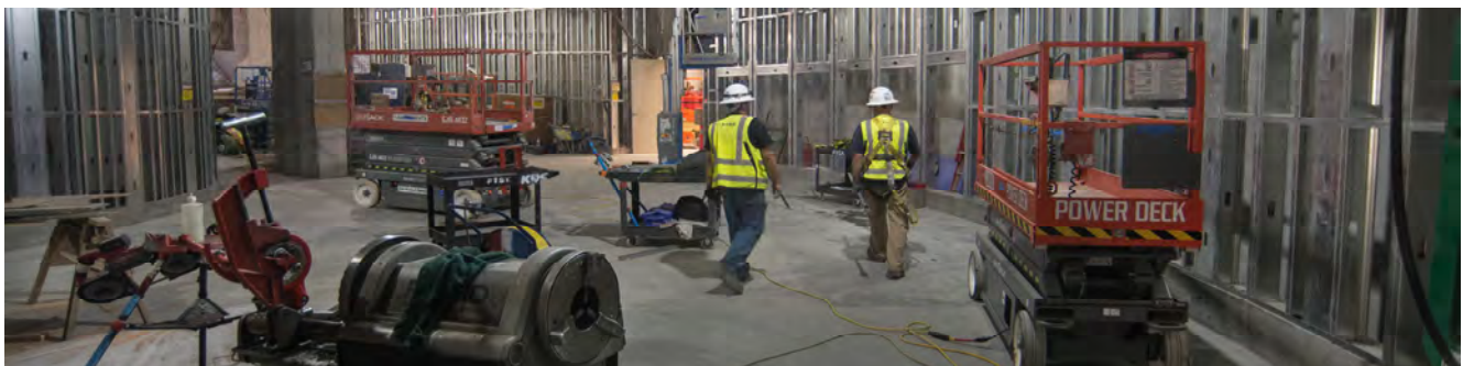
Crews continue to install utility conduits and structural elements inside the north concourse of Union Square/Market Street Station, near the entrance at Union Square.
