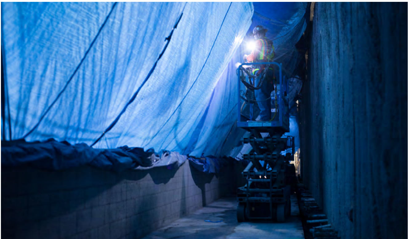
Crews install large tarps to help mask off a section of the south Union Square/Market Street concourse where sound reduction materials are being sprayed.
