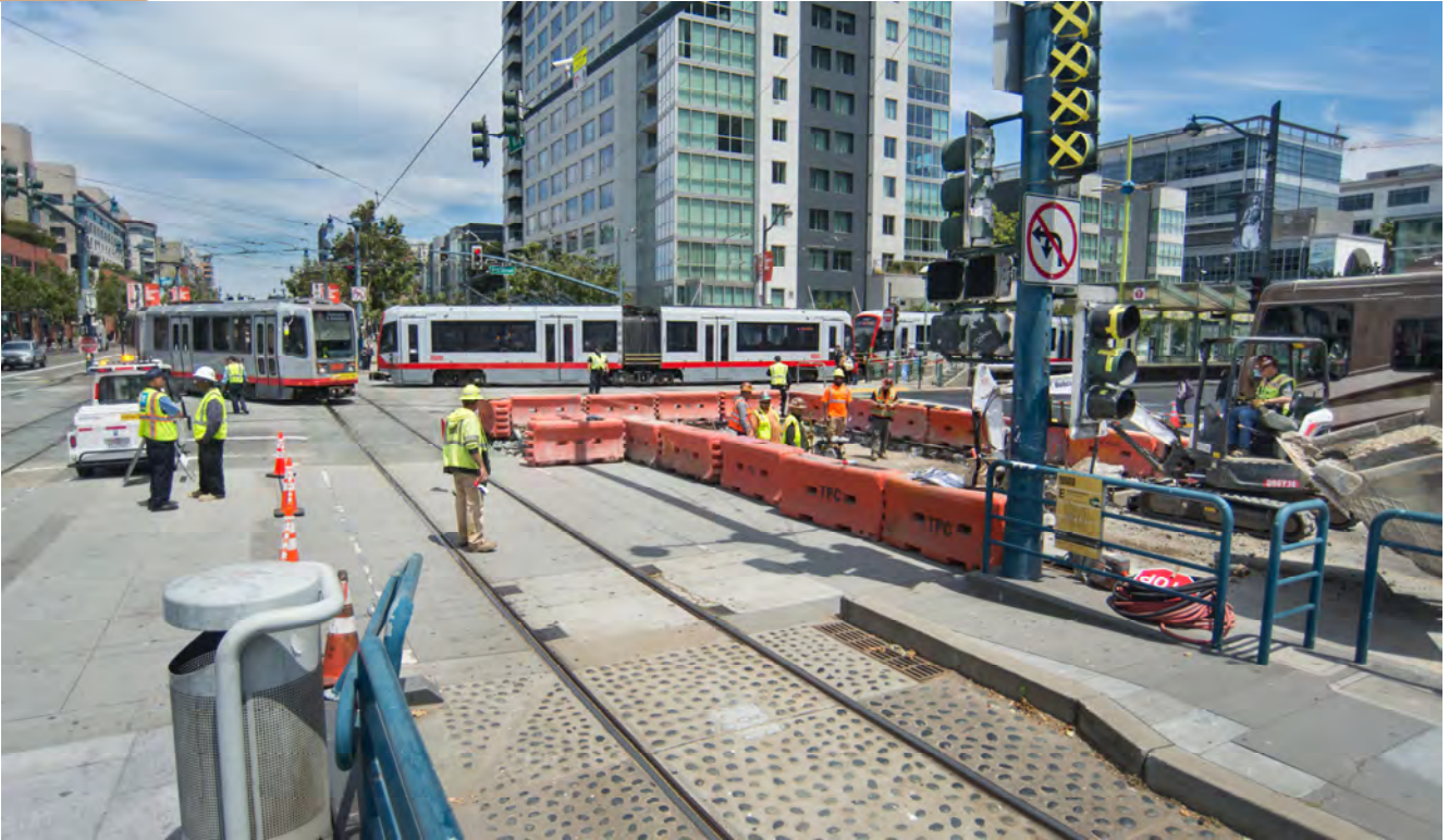
A new T Third Line Siemens S200 light rail vehicle passes an older Breda LRV near roadway restoration work at the southwest corner of 4th and King Streets.
