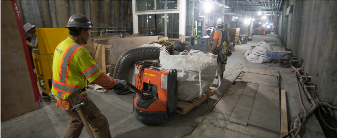
Two men carefully navigate a pallet jack around temporary floor panels, ventilation, and electrical cables near the concourse level elevators for Union Square/Market Street Station.
