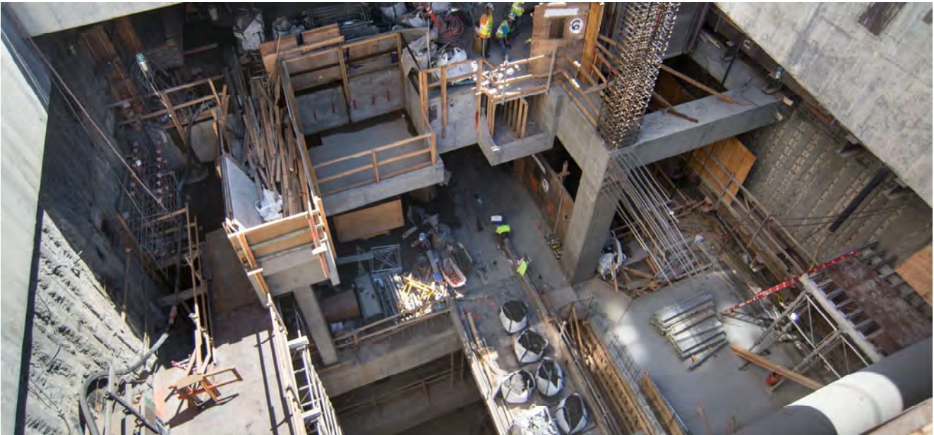
Looking down through the main access shaft, a vast array of major structural elements are going up inside the Chinatown Station headhouse.
