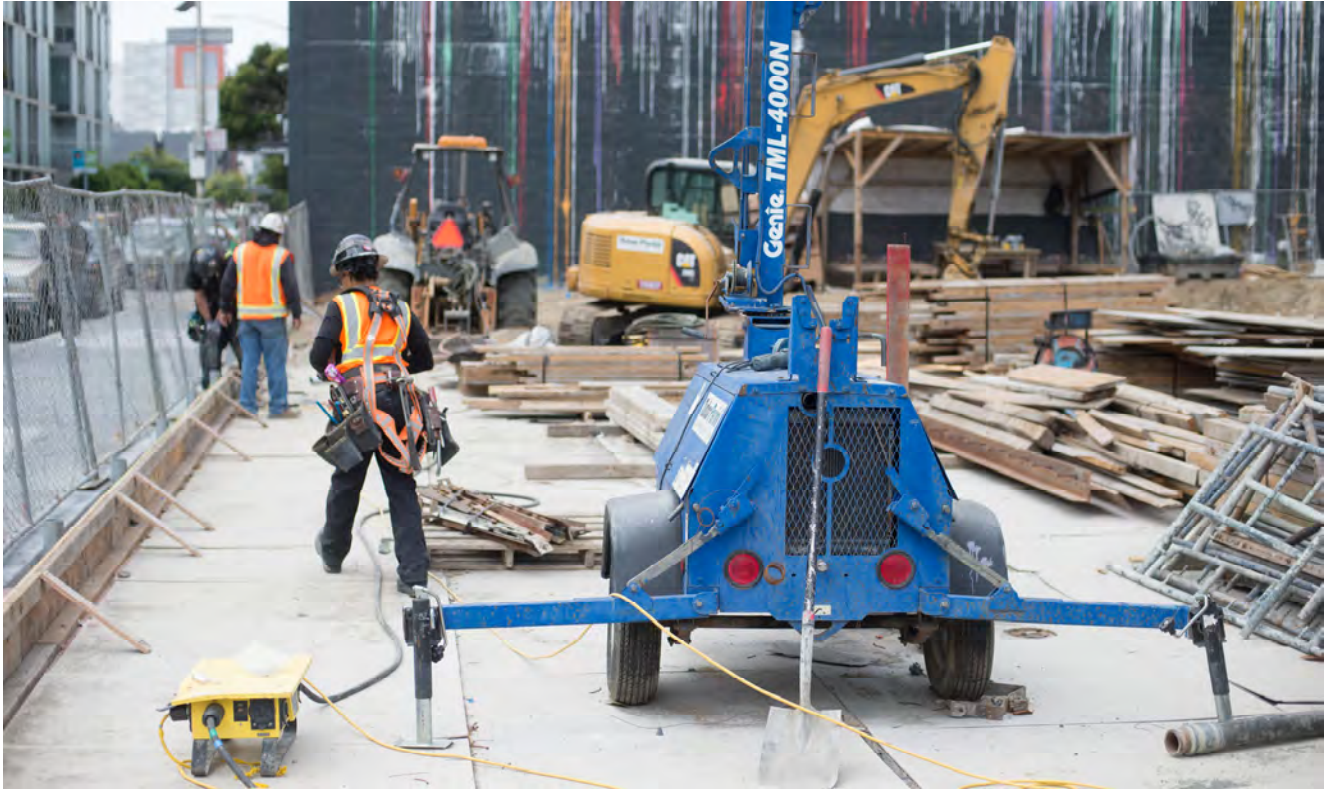
A crew constructs concrete forms for the footer of a temporary fence around the edge of the work site.
