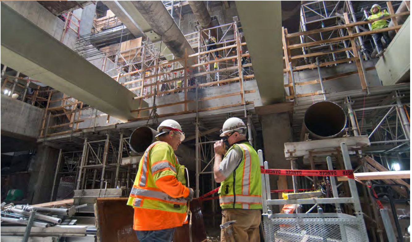
Two workers take a moment to chat on the concourse level of the Chinatown Station headhouse, while workers install scaffolding to build additional floor slabs far above.
