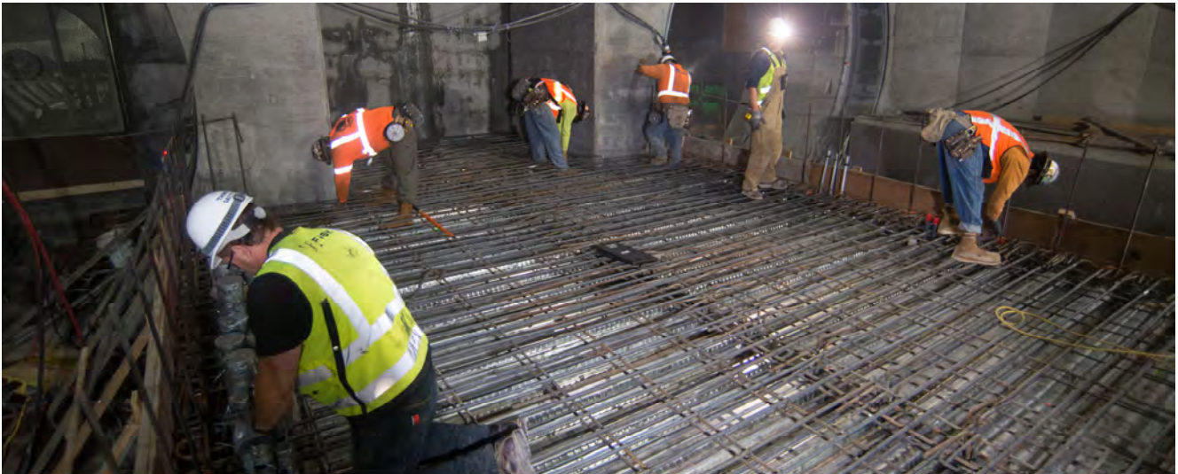
A crew places rebar to build out the last section of Union Square/Market Street Station platform, at the north end of the station.
