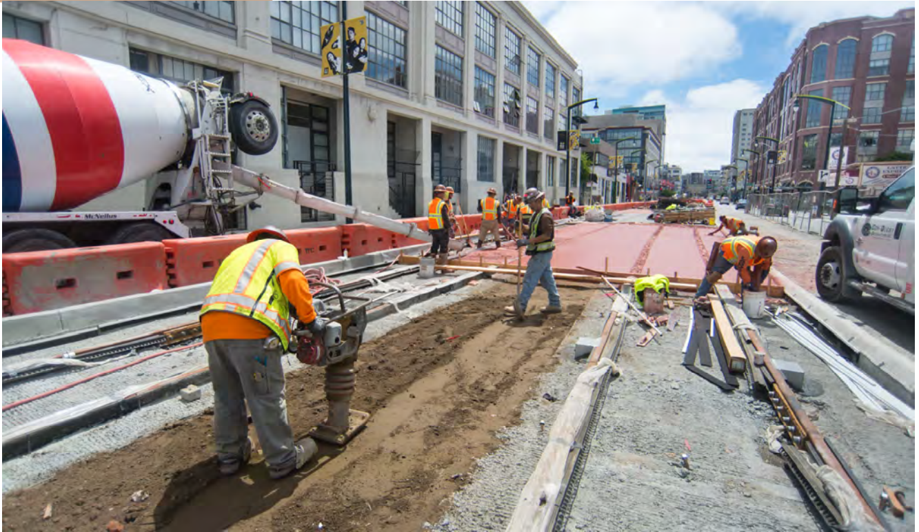
Soil is smoothed in the median between the north and southbound tracks just south of Brannan Street, where workers are pouring a concrete to fill in the space between tracks.
