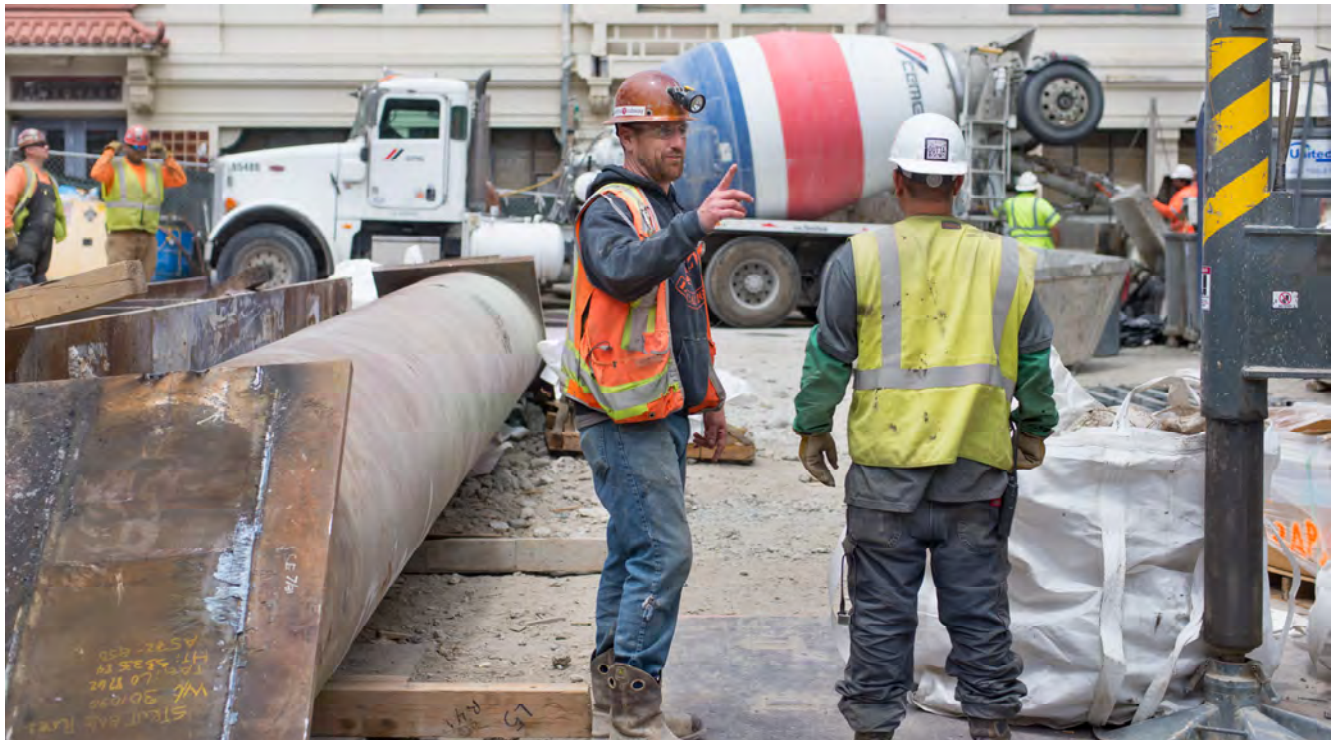
A concrete truck is unloaded into a hopper and pump along Washington Street atop the surface site for Chinatown Station.
