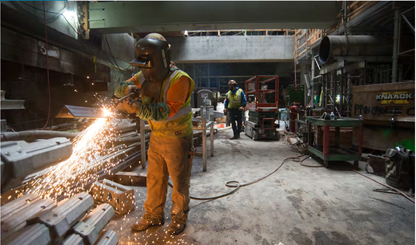
A worker uses a cutting torch to fashion sections of angle iron into brackets, on the concourse level of the Chinatown Station headhouse.
