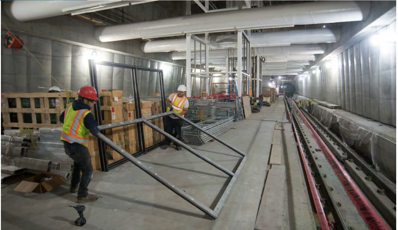
Two men organize framing for glass panels being installed on the dual elevator shafts leading from the concourse level to the station platform.
