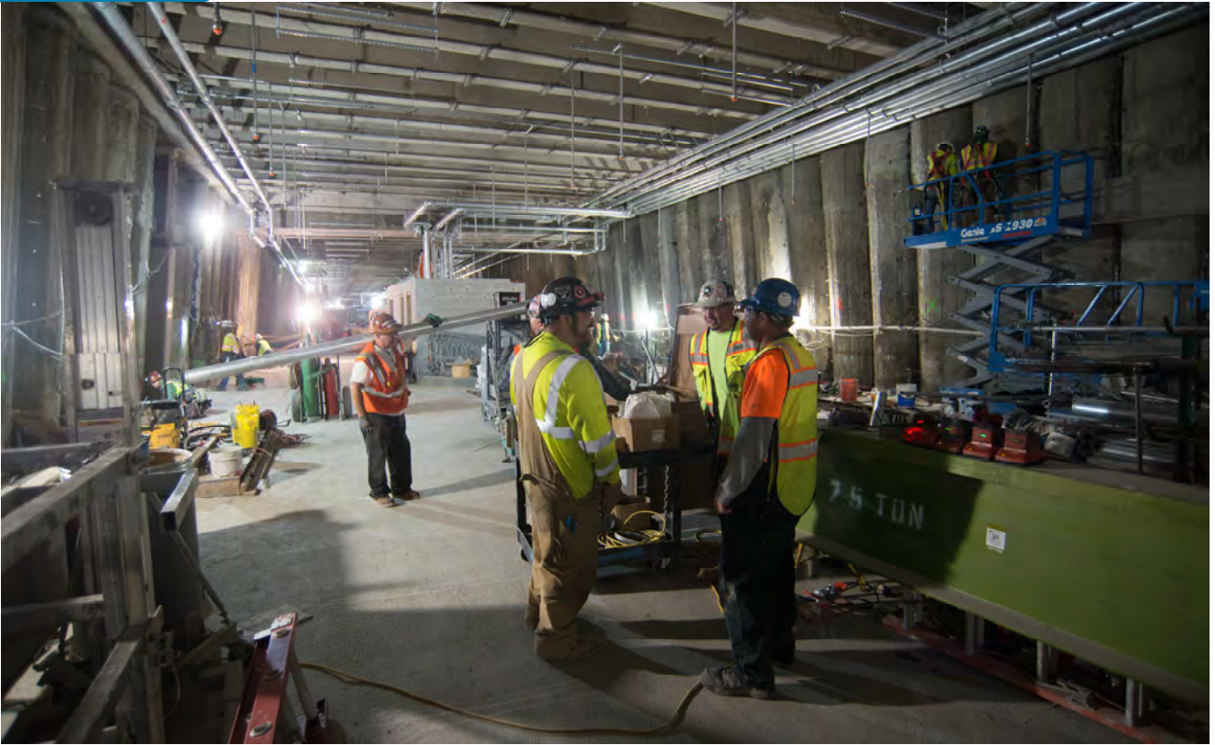
Workers on the concourse level of the Union Square/Market Street Station discuss operations while others install utility conduits nearby.
