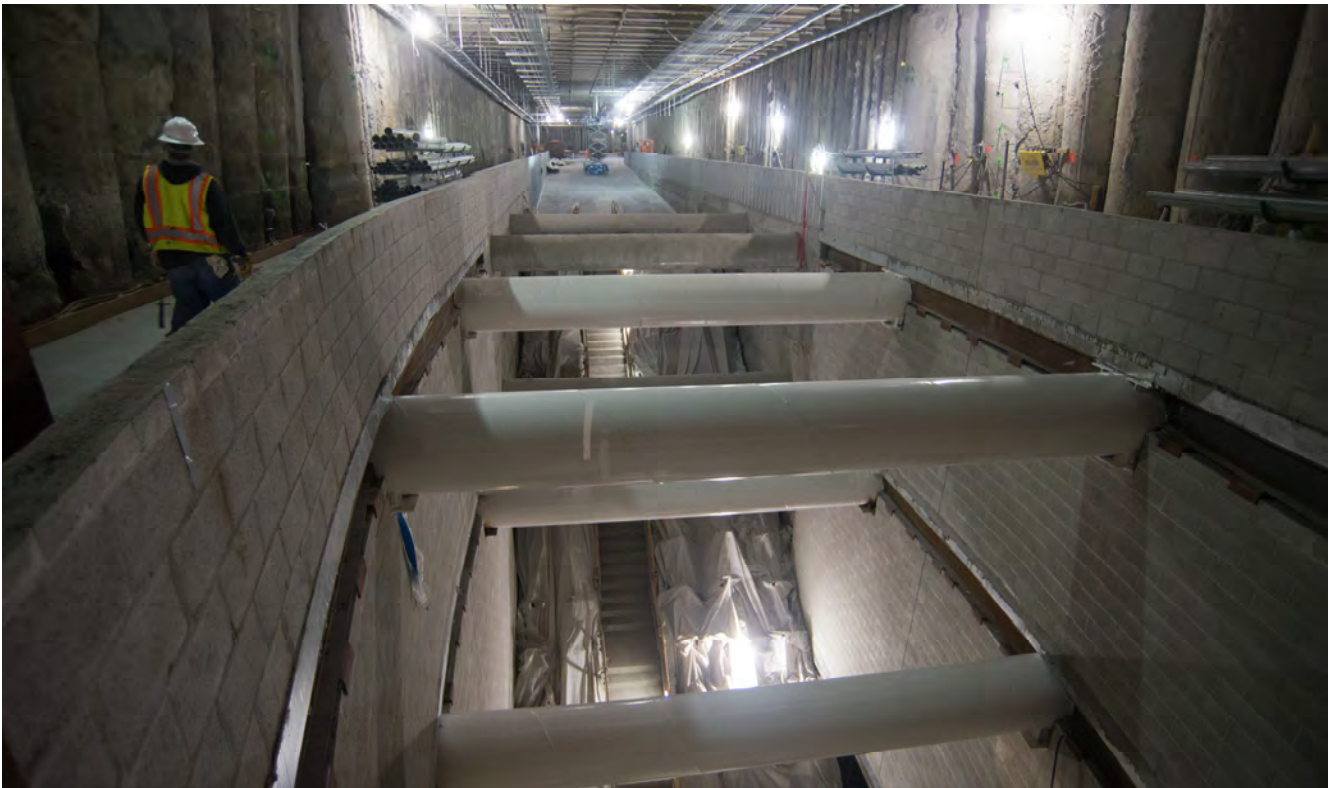
Struts span across the curved opening from the concourse level to the platform level at the south headwall, just south of O'Farrell.
