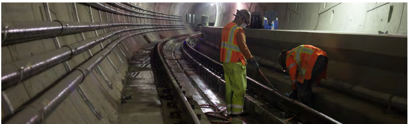
Workers remove excess concrete from rail foundations inside the northbound tunnel S-curve.
