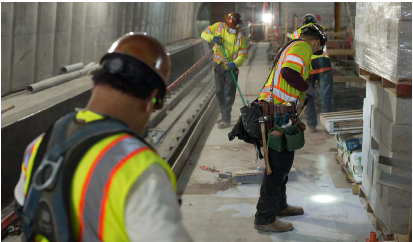
A crew cleans up after a concrete sawcutting operation along the west side of the platform, where trains will travel southbound.
