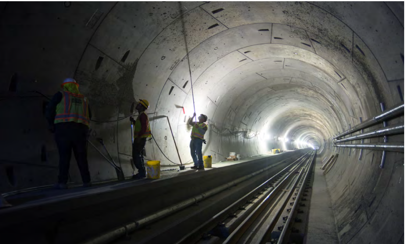
A crew inside the northbound tunnel resurfaces sections of the outer shell of the tunnel for installation of conduits and other infrastructure.
