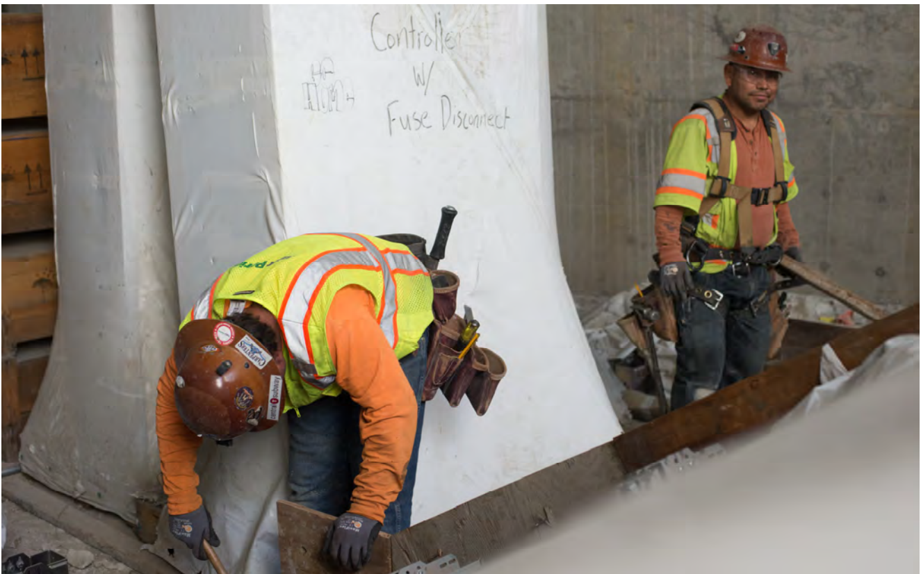
Carpenters build concrete forms to build the main staircase entering into the head-house's concourse level from the future street level plaza.
