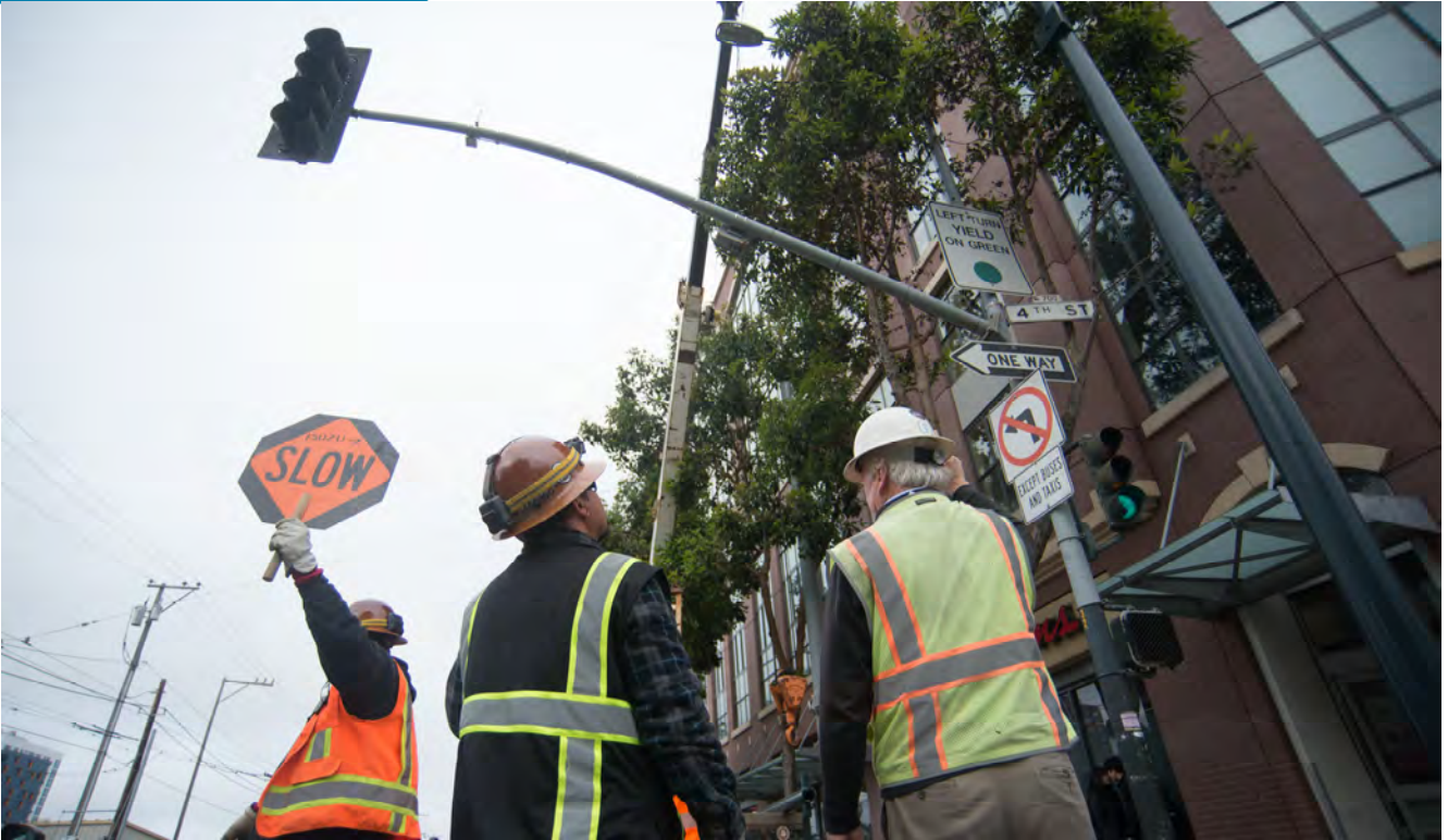
A flagger helps traffic flow through the 4th and Townsend intersection where a new traffic pole is being installed.
