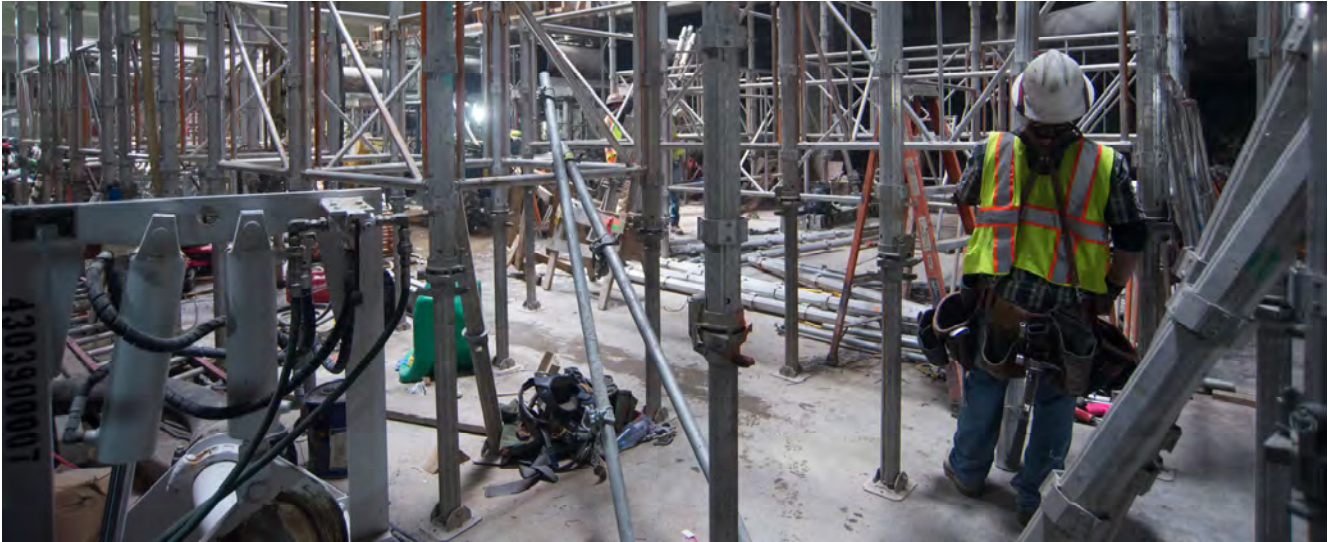
A worker assists associates high above installing scaffolding to support the weight of future interior floors being constructed inside the Chinatown Station headhouse.
