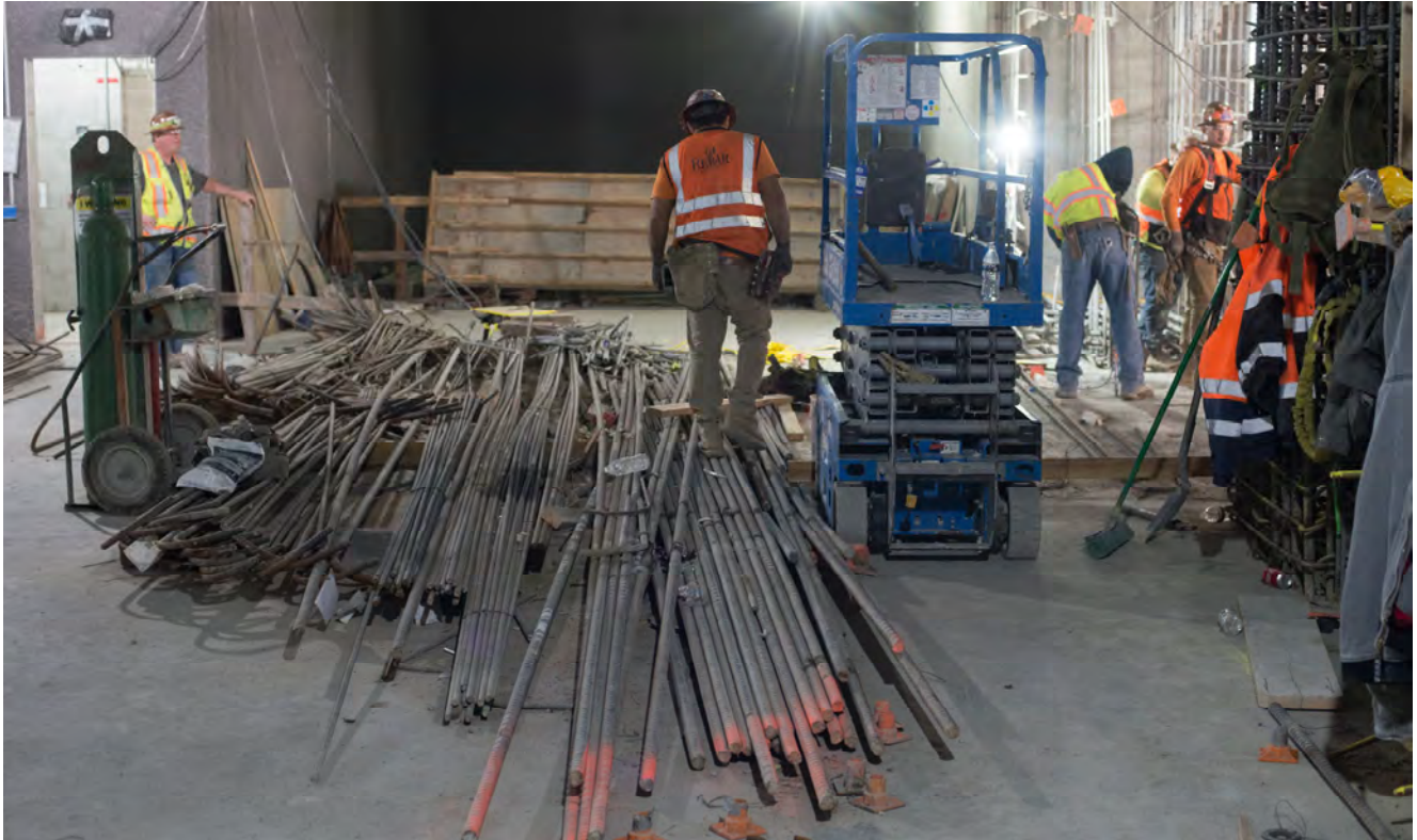
Rebar is stacked and sorted for installation as part of work to fill in a large section of wall between the station box and headhouse.
