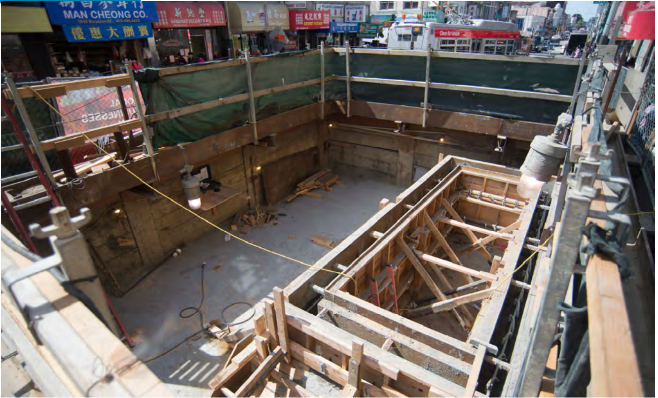
Formwork can be seen for the top of the north egress shaft just. With work to build the shaft nearly complete, the worksite footprint has been reduced.
