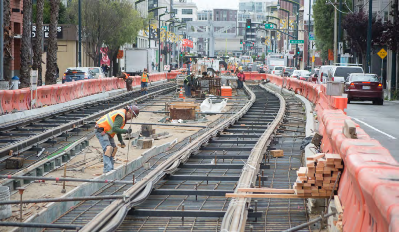
A worker realigns sections of steel forms adjacent to recently-installed rails and foundation rebar just north of the 4th and Brannan surface station platform.
