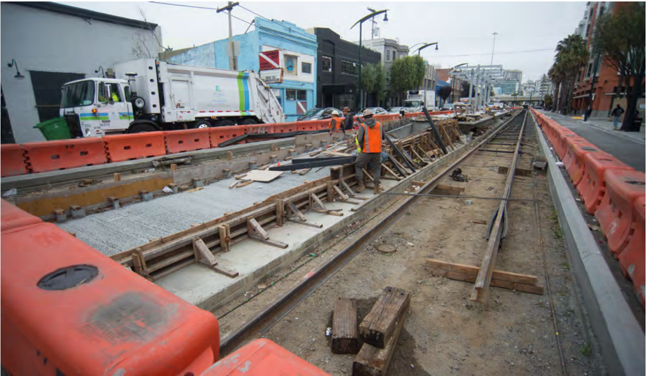
Sections of rail can be seen being installed alongside the 4th and Brannan surface station platform.
