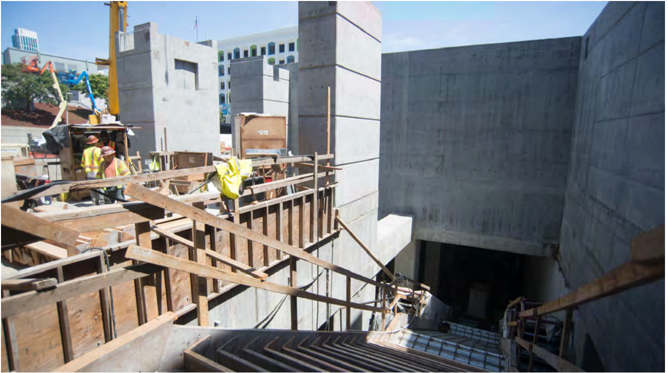
Formwork and even some rebar for the future entrance stairwell can be seen going in where the street level plaza descends into the future station entrance.
