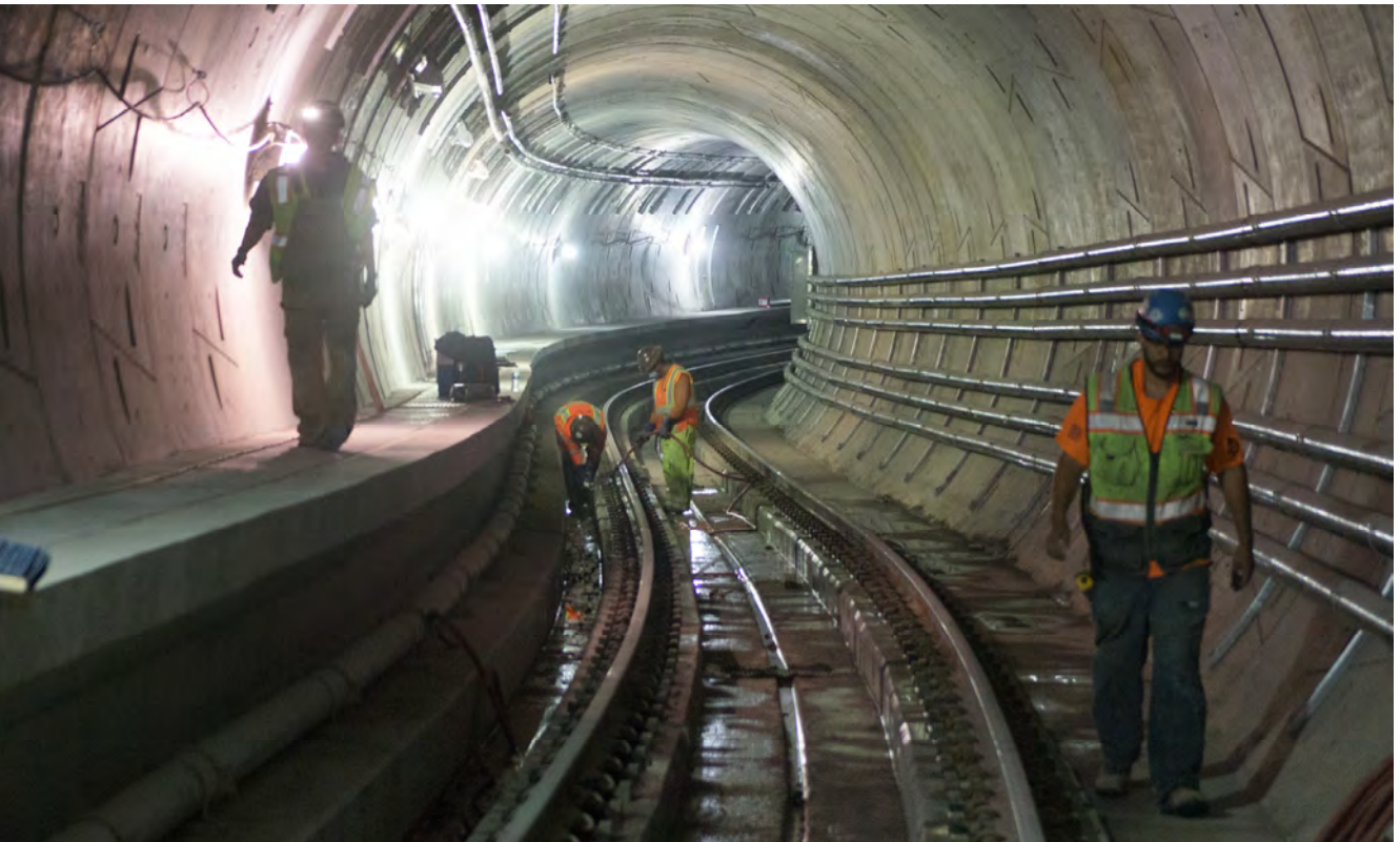
Crewmembers conduct site cleanup inside the S-curve of the northbound tunnel, just south of the Union Square/Market Street Station platform.
