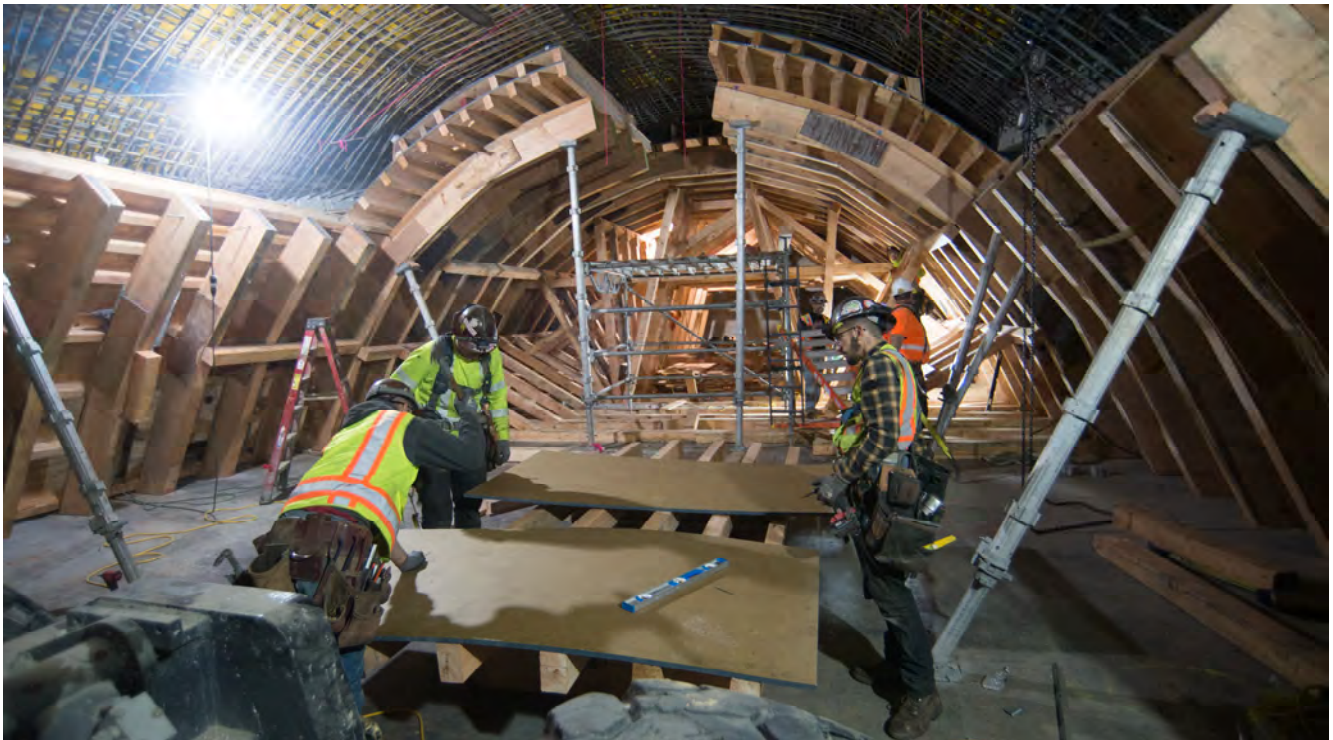
Complex wood cribbing and concrete forms have been going in to prepare for the cross-cut cavern's vaulted ceiling, an immensely complex feat of engineering.
