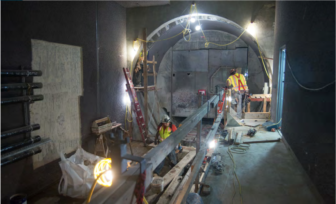
Workers clean out a drainage trough and install rebar to build a transition structure where the southbound tunnel meets the north end of Yerba Buena/Moscone Station.
