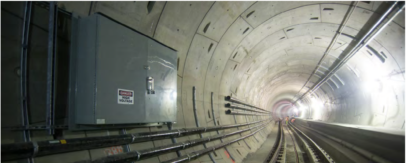
Electrical infrastructure is being installed in phases inside the northbound tunnel, as seen just south of the Union Square/Market Street Station.
