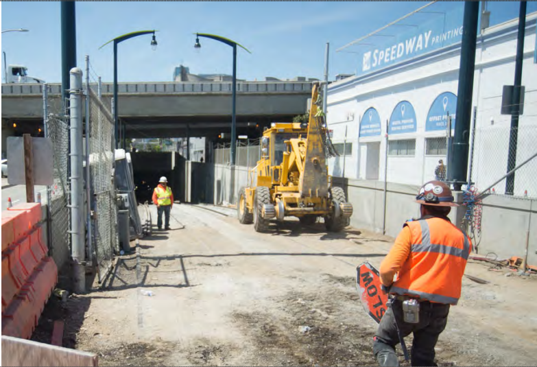
1 Crews remove the road slab in sections just outside the tunnel portal
