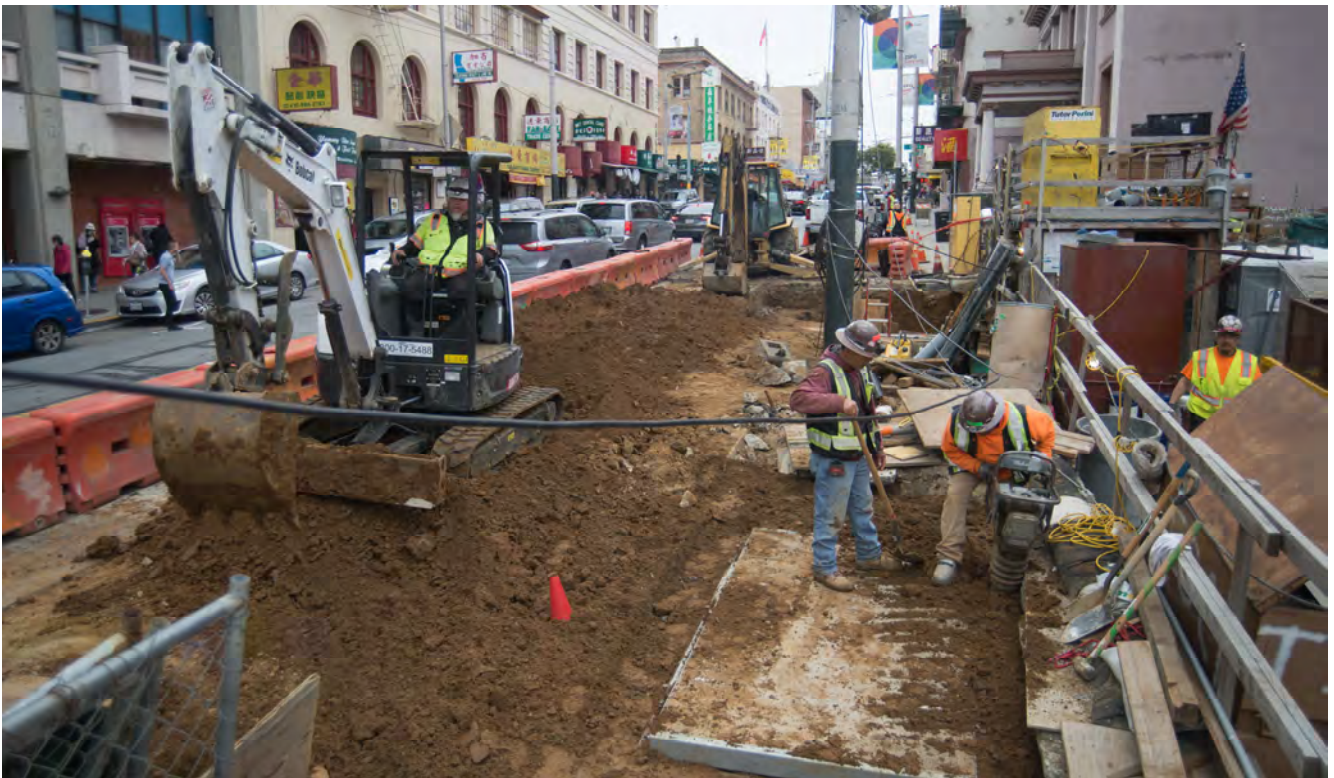
Workers backfill around massive utility vaults, installed for electrical and other utilities along the east side of the surface worksite.
