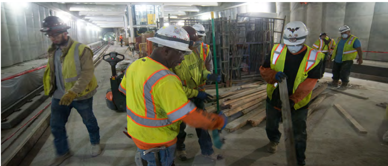
A crew collects pieces of concrete forms to be reused on the Union Square/Market Street Station platform.
