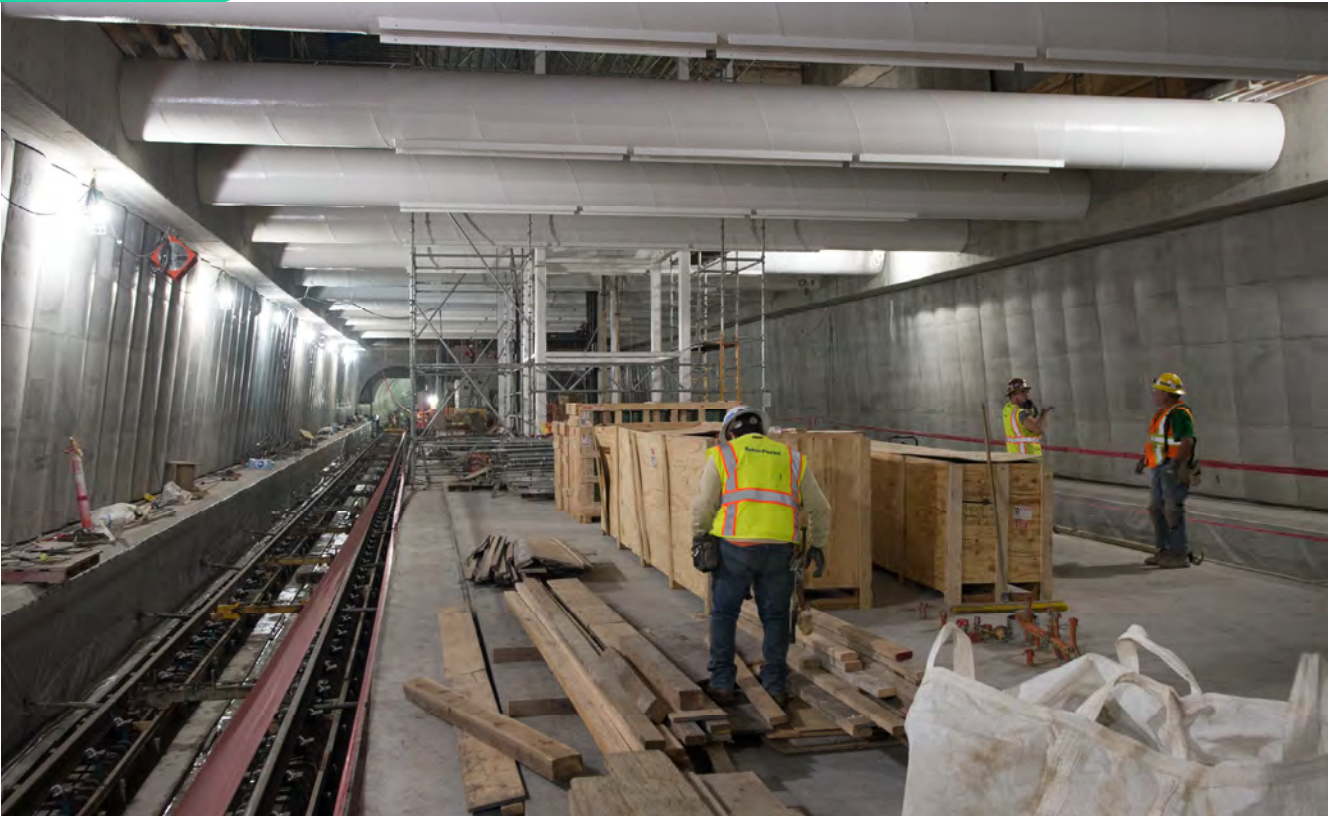
A crew unpacks interior elements slated to be added to the dual concourse-to-platform elevators, with steel framing visible in the center of the platform to the north.
