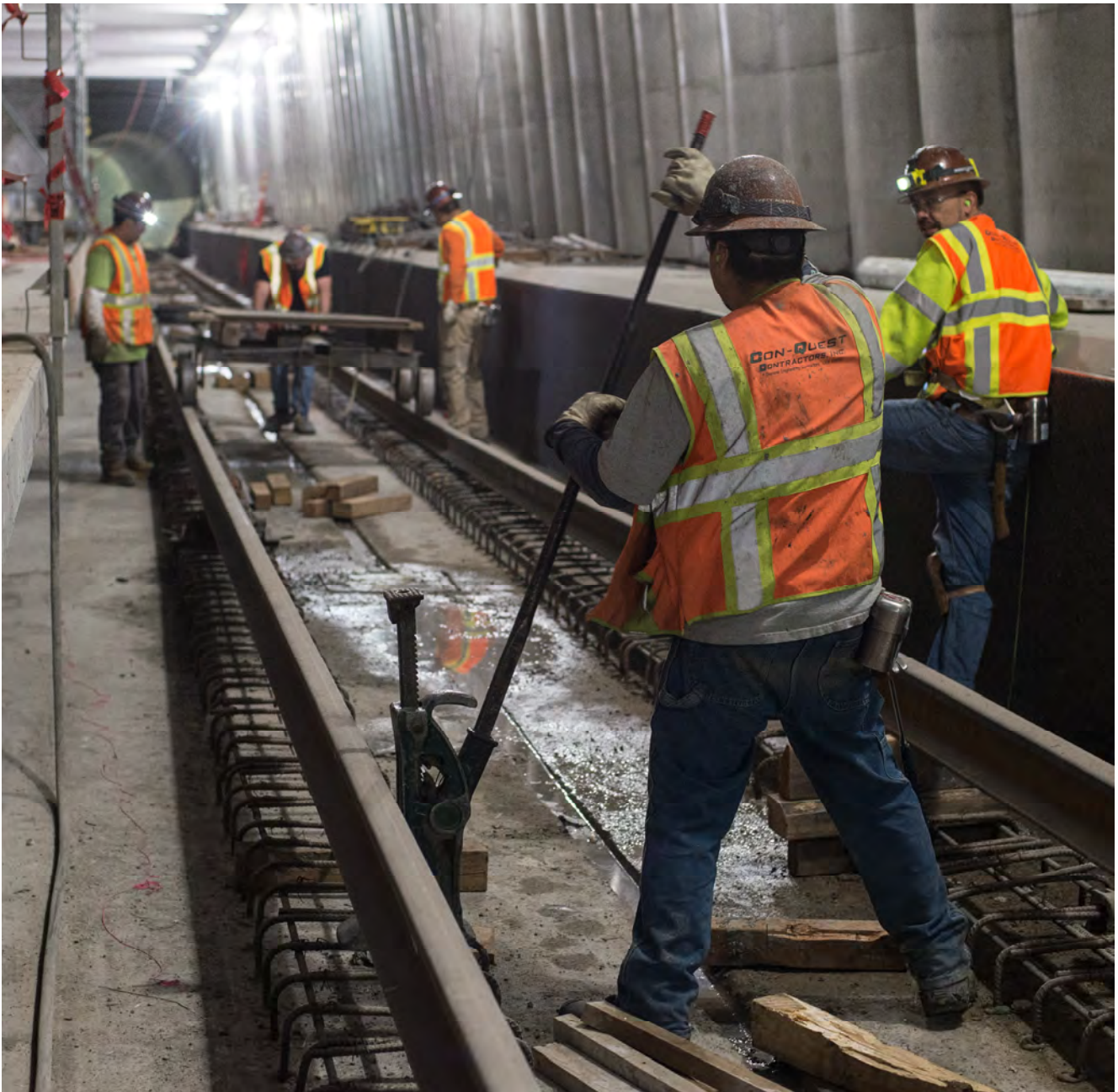
Workers jack up and align sections of rail during track installation work on the south-bound side of the Union Square/Market Street Station platform.
