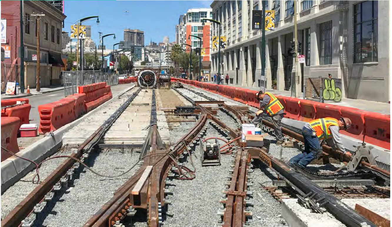
Workers set up to use thermite welding to join sections of rail together on 4th Street near Bluxome.
