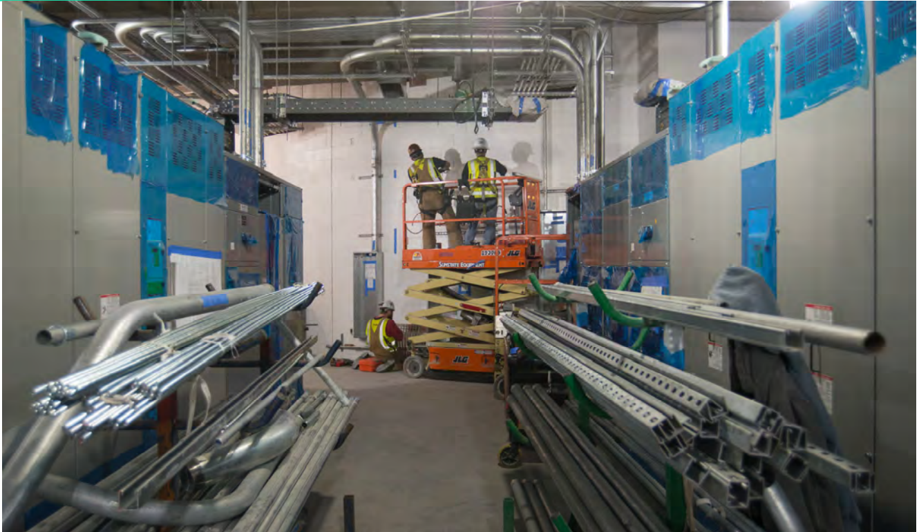
A truly immense network of conduits for all manner of systems and utilities are being installed inside the upper level of the north concourse for Union Square/Market Street Station.
