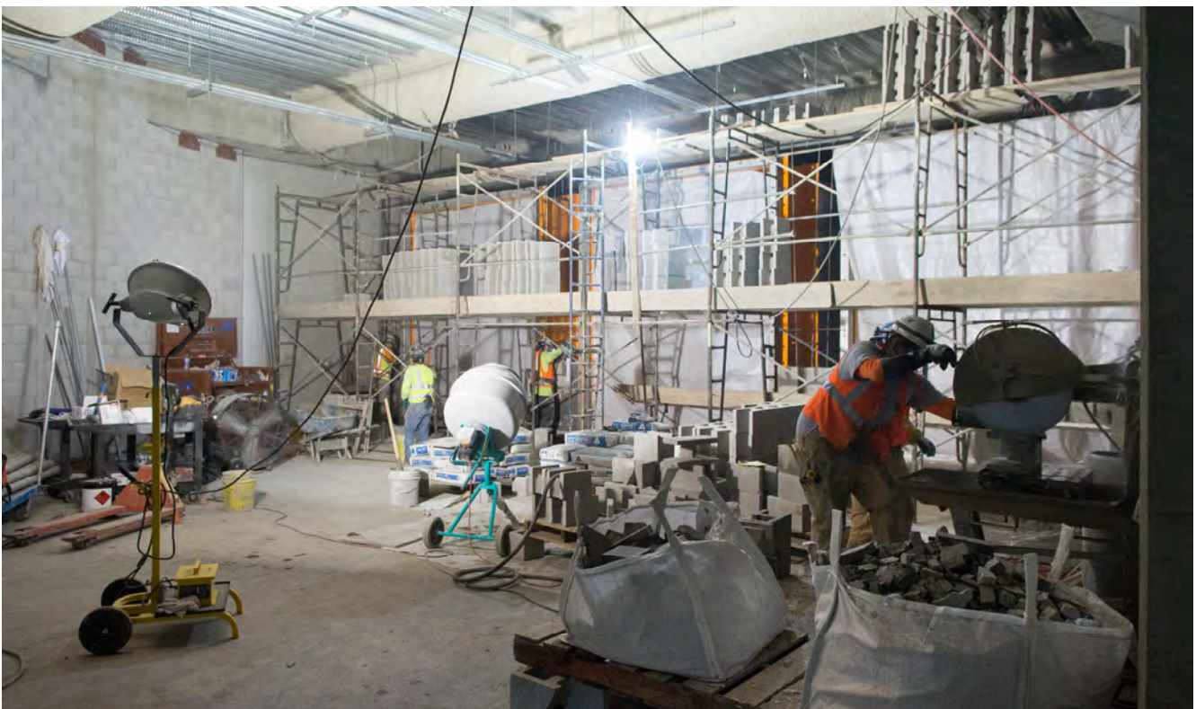
Masons cut and place hollow cinderblocks which will become part of reinforced concrete walls inside the fan level of the north concourse for Union Square/Market Street Station.
