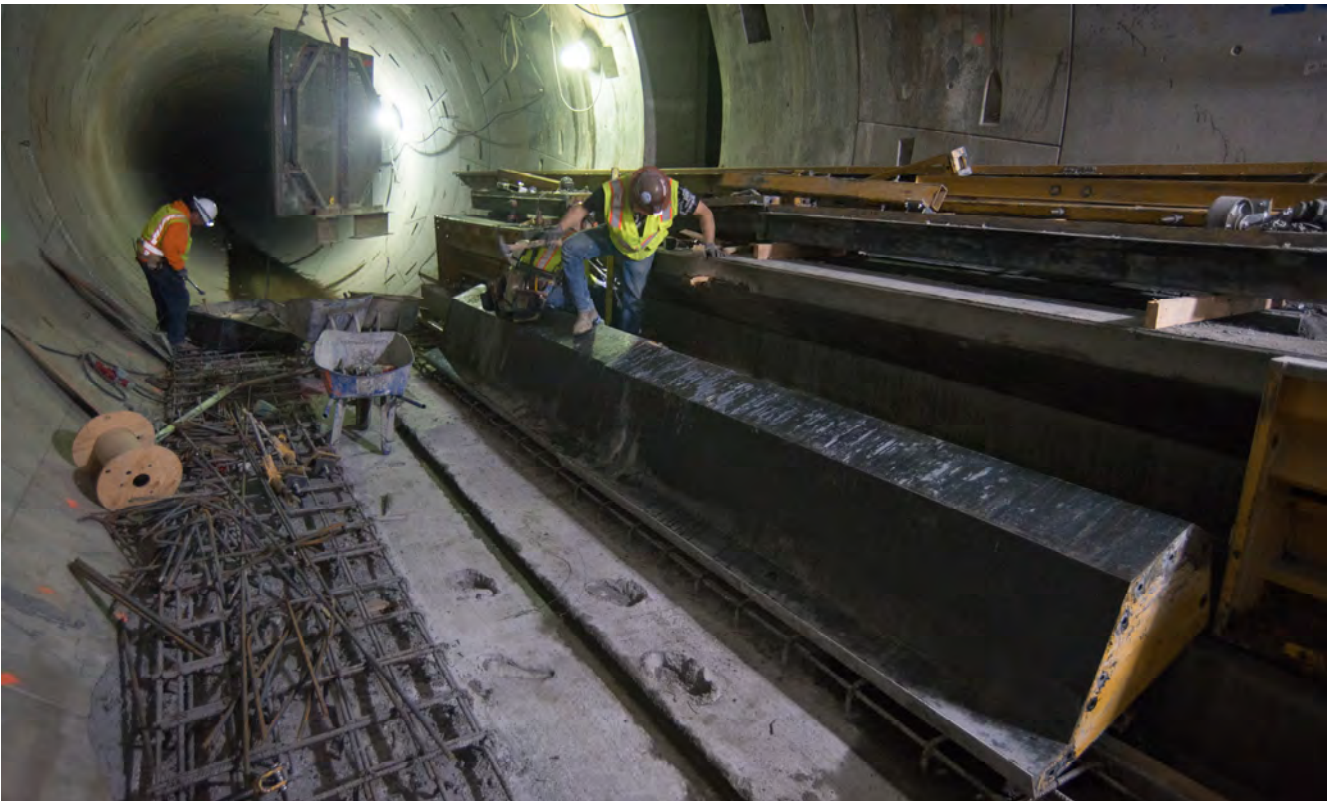
A large section of steel formwork used to build sections of tunnel walkways can be seen during removal adjacent to a tunnel cross-passage just north of Chinatown Station.
