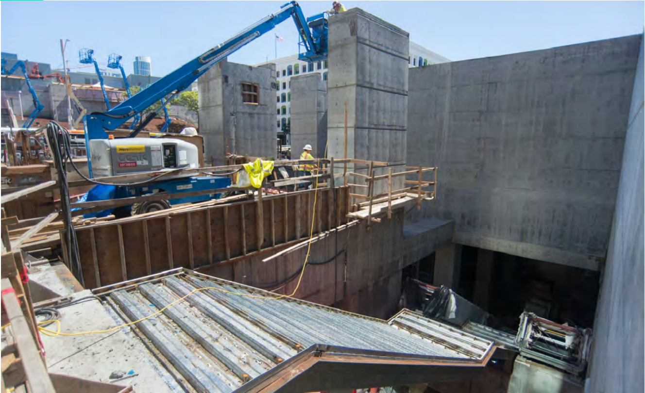
Corrugated Steel and steel framing have been placed to build the future entrance staircase for the Yerba Buena/Moscone Station headhouse.
