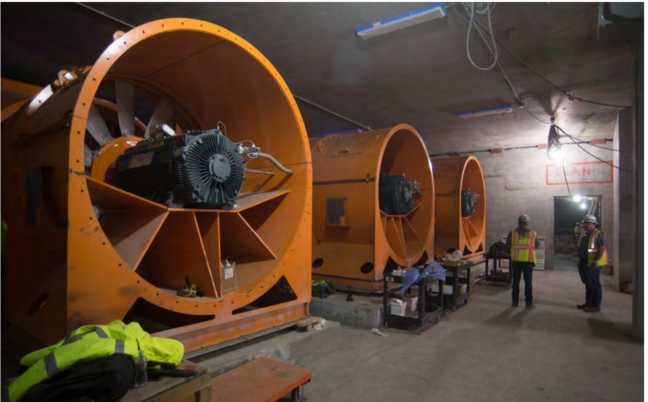
High-capacity fans have been installed on pedestals inside the Yerba Buena/Moscone Station box for emergency tunnel ventilation systems.
