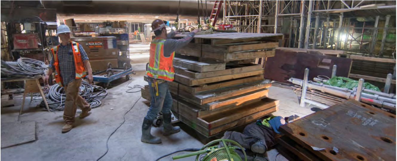
A worker welds brackets onto steel slabs while an associate prepares stacks of concrete form sections to be lifted to the surface from the concourse level of the Chinatown Station headhouse.
