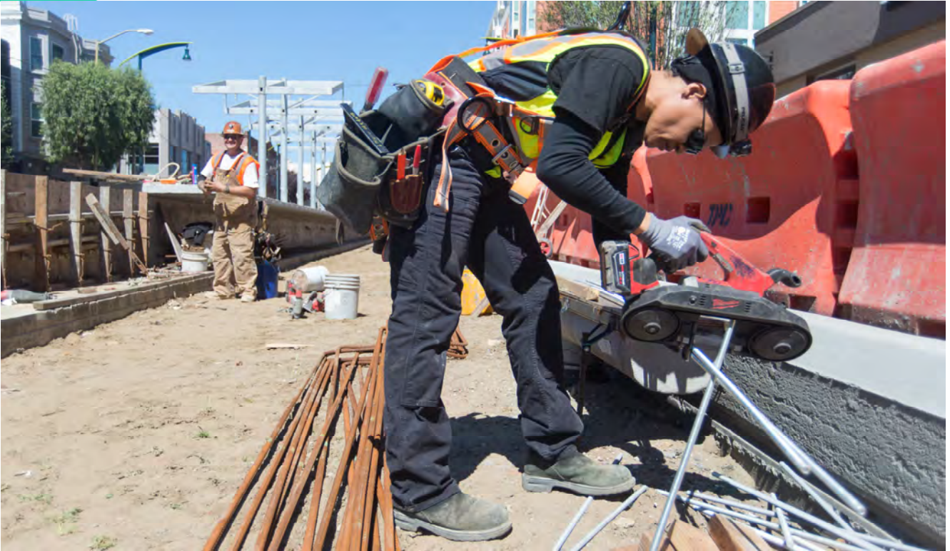
A worker cuts sections of threaded steel used in construction of the entrance ramp for the 4th and Brannan surface station platform.
