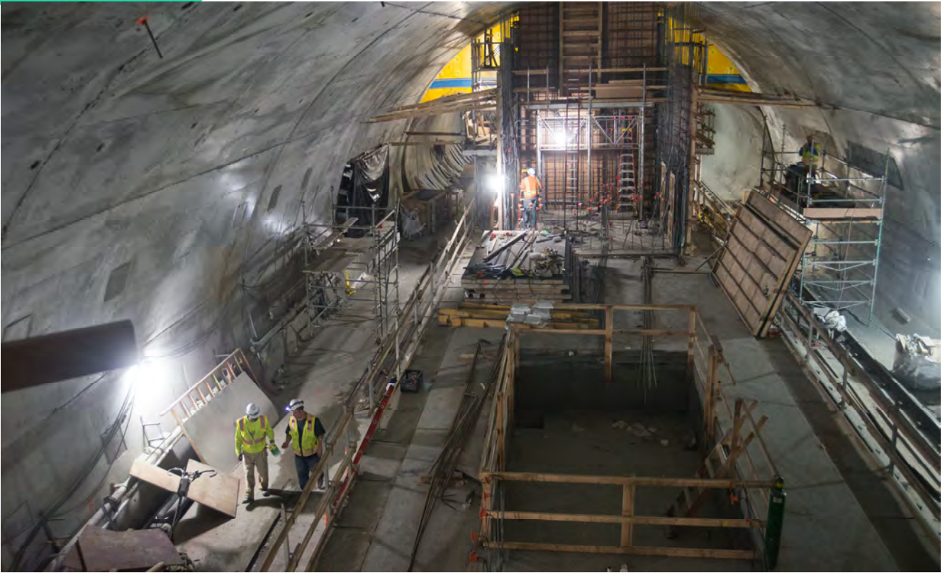
Large recesses in the station platform will eventually receive escalators from the concourse level, with work to build an emergency egress staircase ongoing beyond.
