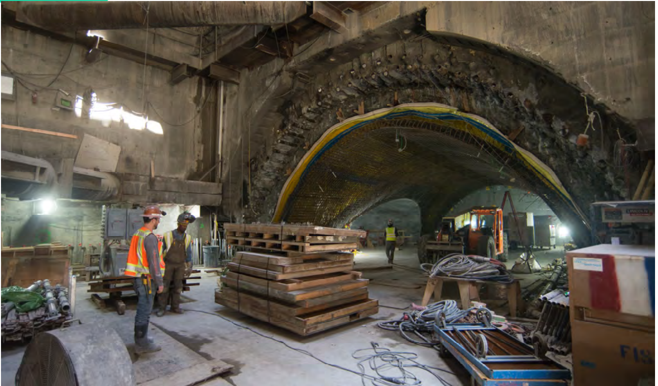
Stacks of concrete form sections await to be lifted to the surface near the arched future entrance of the Chinatown Station platform cavern.
