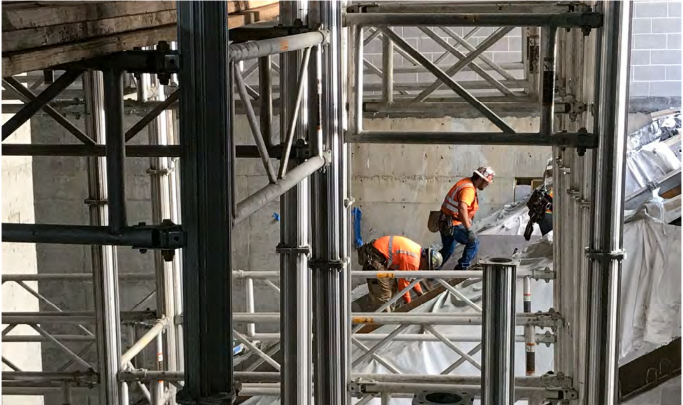
Two crewmembers can be seen through a gap in support scaffolding building the initial formwork for the entrance staircase to Yerba Buena/Moscone Station.
