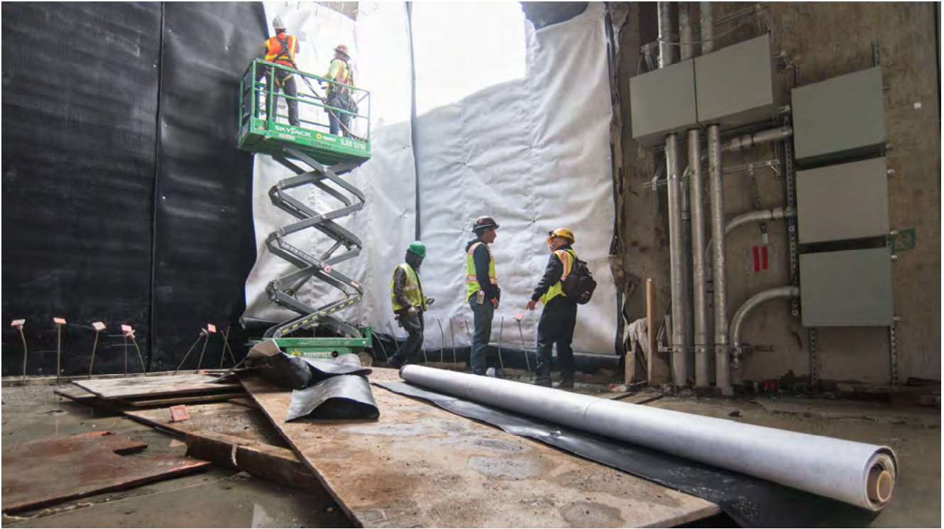
Light shines into the mezzanine level of the Yerba Buena/Moscone Station headhouse from the ventilation structure at the surface, while workers install waterproofing against the exterior slurry walls.
