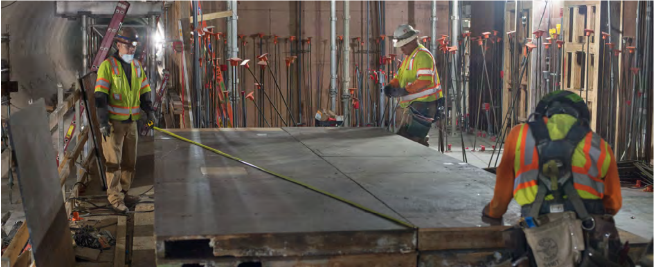
Carpenters take measurements of concrete formwork set to be reused at the north end of the Chinatown Station platform cavern.
