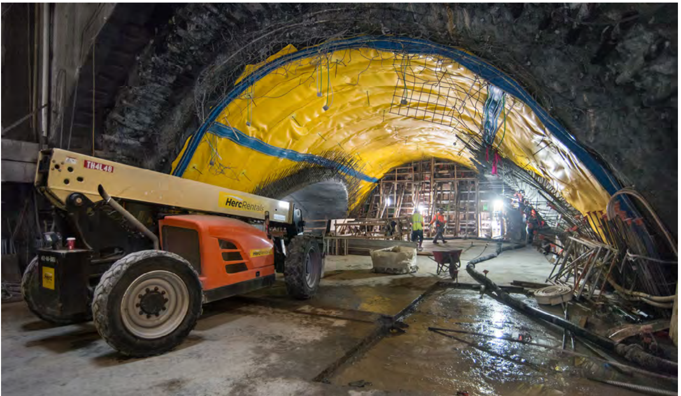
A forklift waits at the arched entrance to the Chinatown Station platform beyond and below, while workers install formwork to construct a finished wall on the far side.
