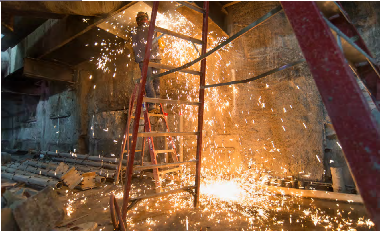
A worker descends the ladder from the concourse level of the Chinatown Station cavern, where formwork is being installed to construct a section of the floor slab.
