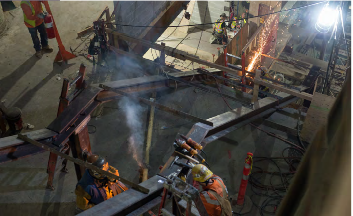
Welders assemble sections of steel I-beams to build structural framing for the future north staircase to and from the Union Square/Market Street Station platform.
