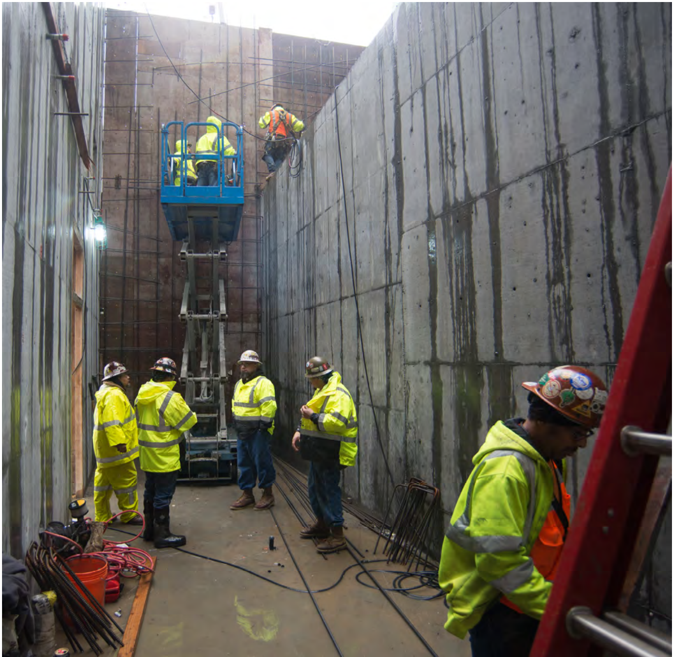
A crew holds a meeting inside the future ventilation structure for Yerba Buena/Moscone Station adjacent to the station entrance.
