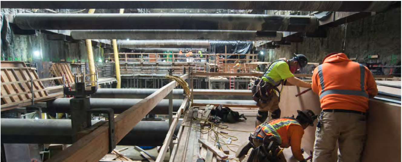
Carpenters build sections of concrete forms on the level above the Chinatown Station concourse, inside the headhouse.
