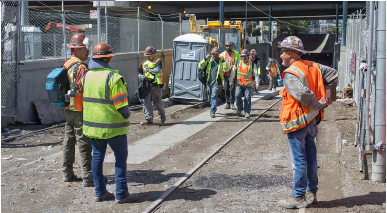
A crew emerges from the tunnels at the 4th and Bryant tunnel portal following the end of the workday.
