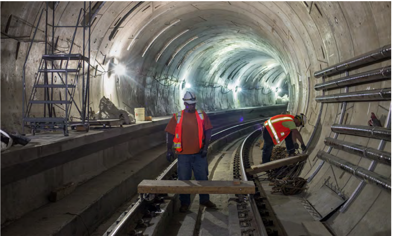
A worker inspects a utility dolly used to roll heavy equipment down the northbound track for utility work at the s-curve under Market Street.
