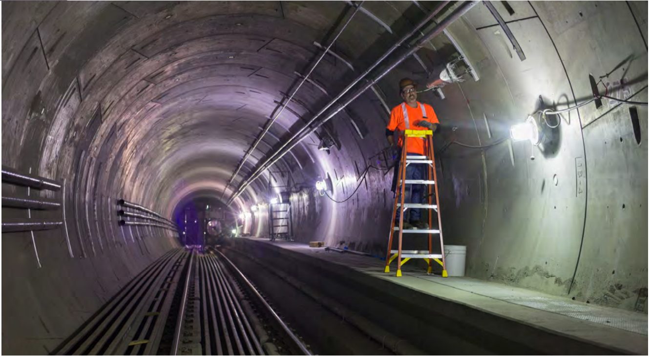
Permanent lighting fixtures are now being installed inside the northbound tunnel just north of the Yerba Buena/Moscone Station platform.
