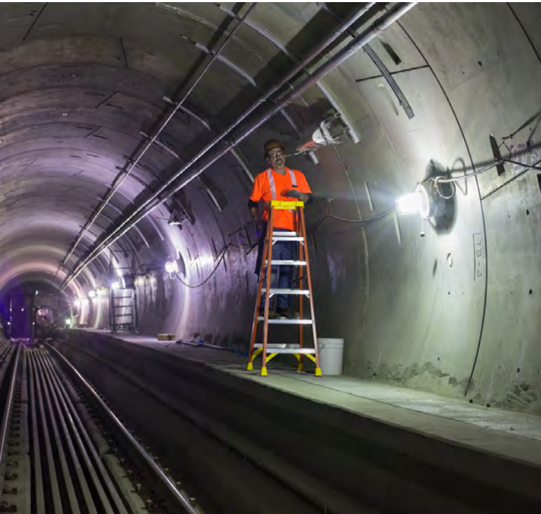
2 Light fixtures are affixed to steel brackets mounted to the tunnel walls
