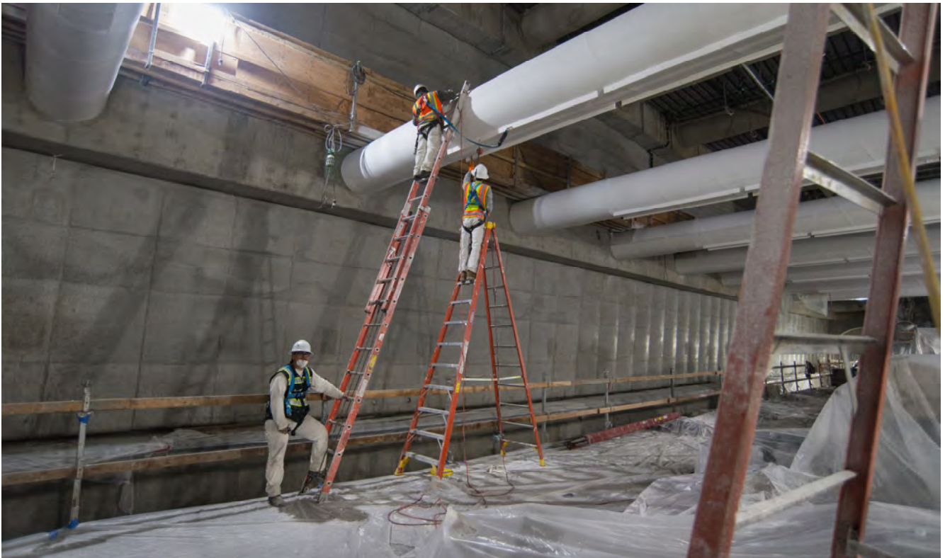
Painters on the northbound track side of the platform level continue to coat the massive steel struts that span across the Union Square/Market Street Station interior.
