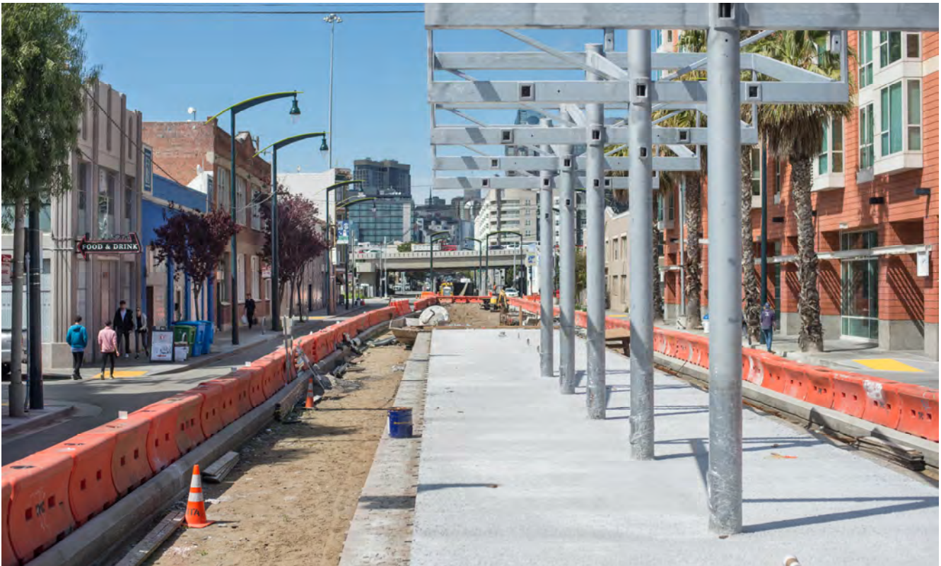
The rough surfaced slab of the future 4th and Brannan surface platform has recently been poured.
