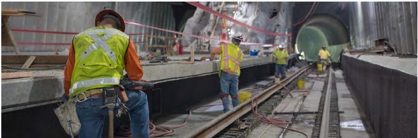
A crew uses pneumatic tools to smooth concrete surfaces on the southbound track side of the Union Square/Market Street Station platform.
