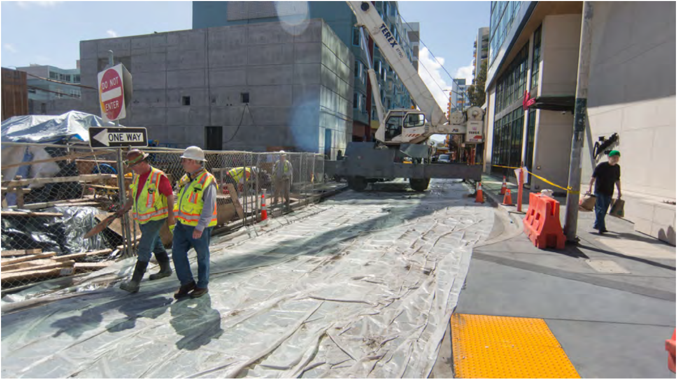
A massive concrete form has been constructed to build a wall at the south end of the main entrance to the Yerba Buena/Moscone Station concourse, 40 feet below.
