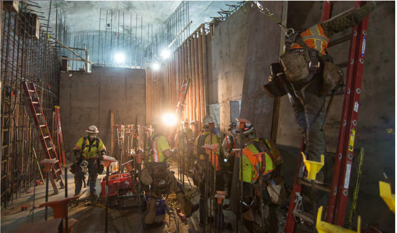
A crew positions a tall section of concrete formwork after removing it as part of wall construction near the south end of the Chinatown Station platform.
