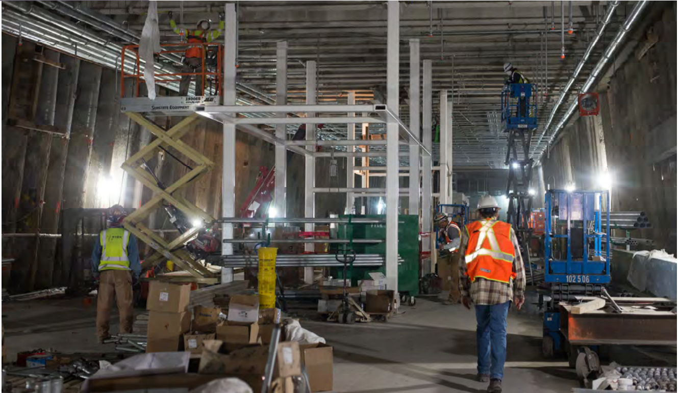
The site superintendent makes rounds as workers continue installing conduits and brackets for future interior elements on the concourse level of the Union Square/Market Street Station.
