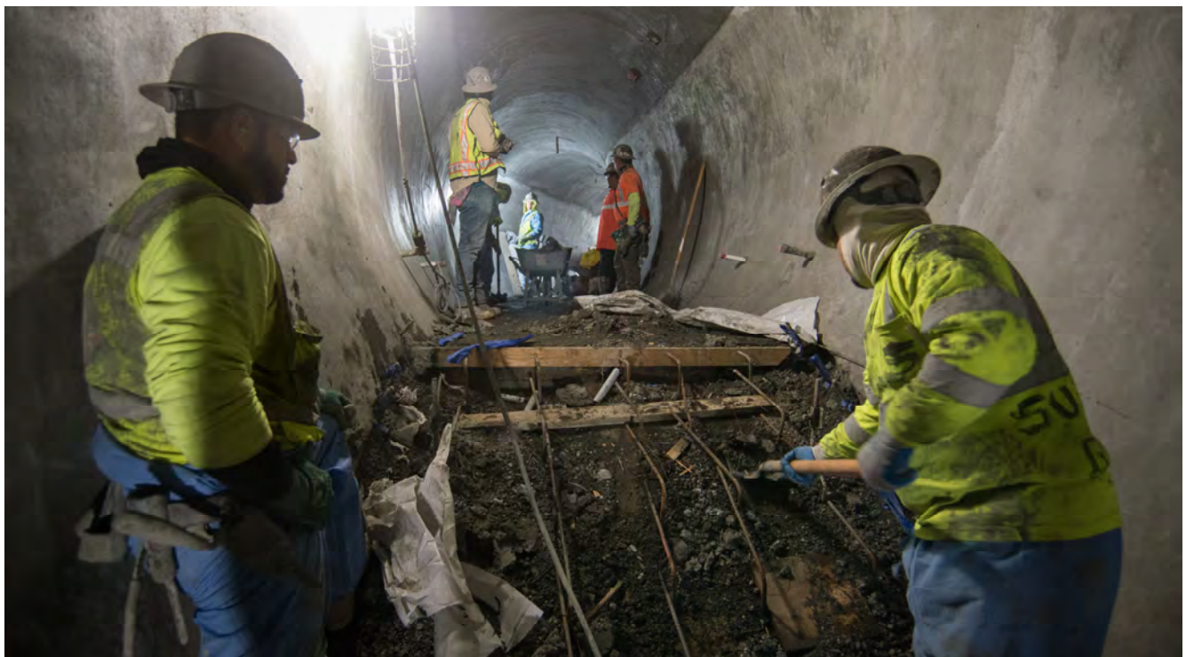
A crew cleans up this work area following shotcrete spraying to build the tunnel lining for the north egress shaft connecting the Chinatown Station platform cavern with an emergency exit stairwell just south of Jackson Street.
