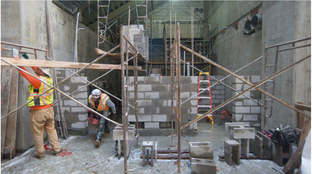
Crews have been hard at work building interior walls on the concourse level of the Yerba Buena/Moscone Station headhouse.
