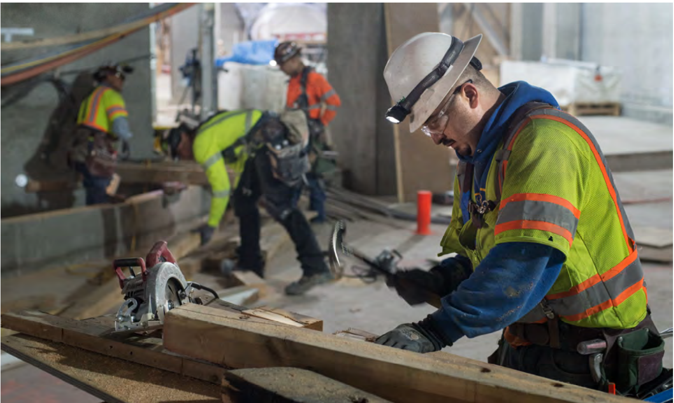
Carpenters fashion pieces of 4x4s as part of cribbing for wall work inside the north concourse of Union Square/Market Street Station.
