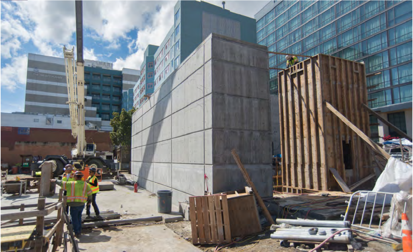
Large concrete structures continue to go up on the surface of the Yerba Buena/Moscone Station site. These structures will become part of the future station entrance at 4th and Clementina.
