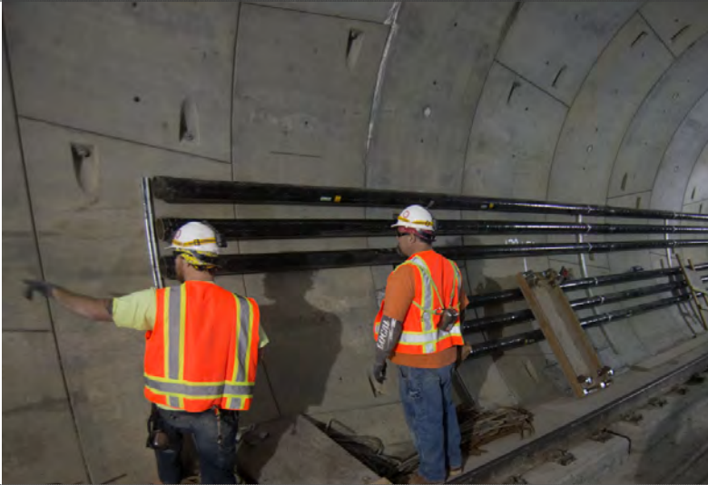
1 Workers install brackets and conduits to be used for tunnel utility systems
