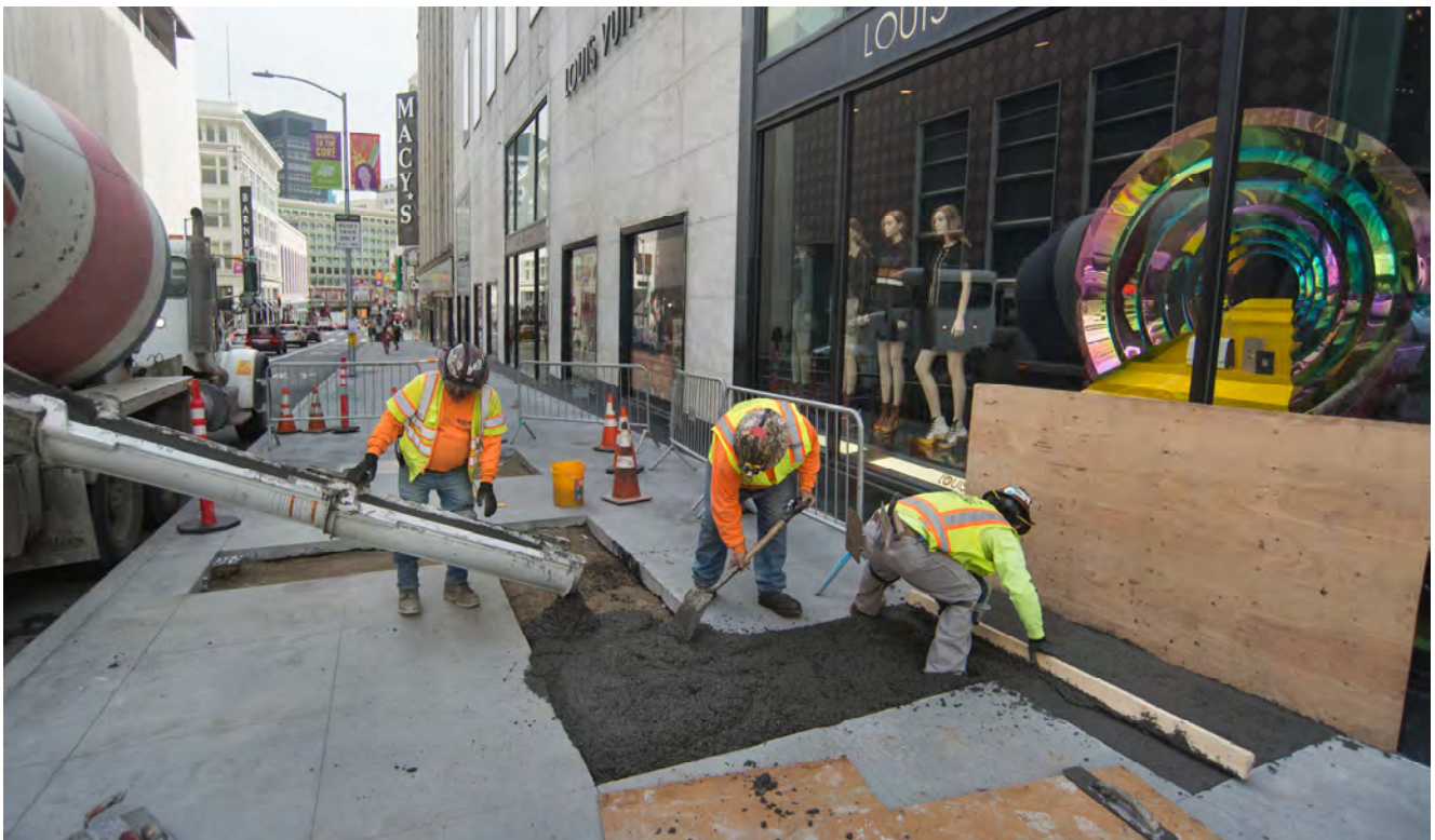
A crew pours concrete on the west side of Stockton to fill a last few panels of sidewalk following the completion of utility work and the reopening of Stockton between Geary and Ellis to vehicular traffic.
