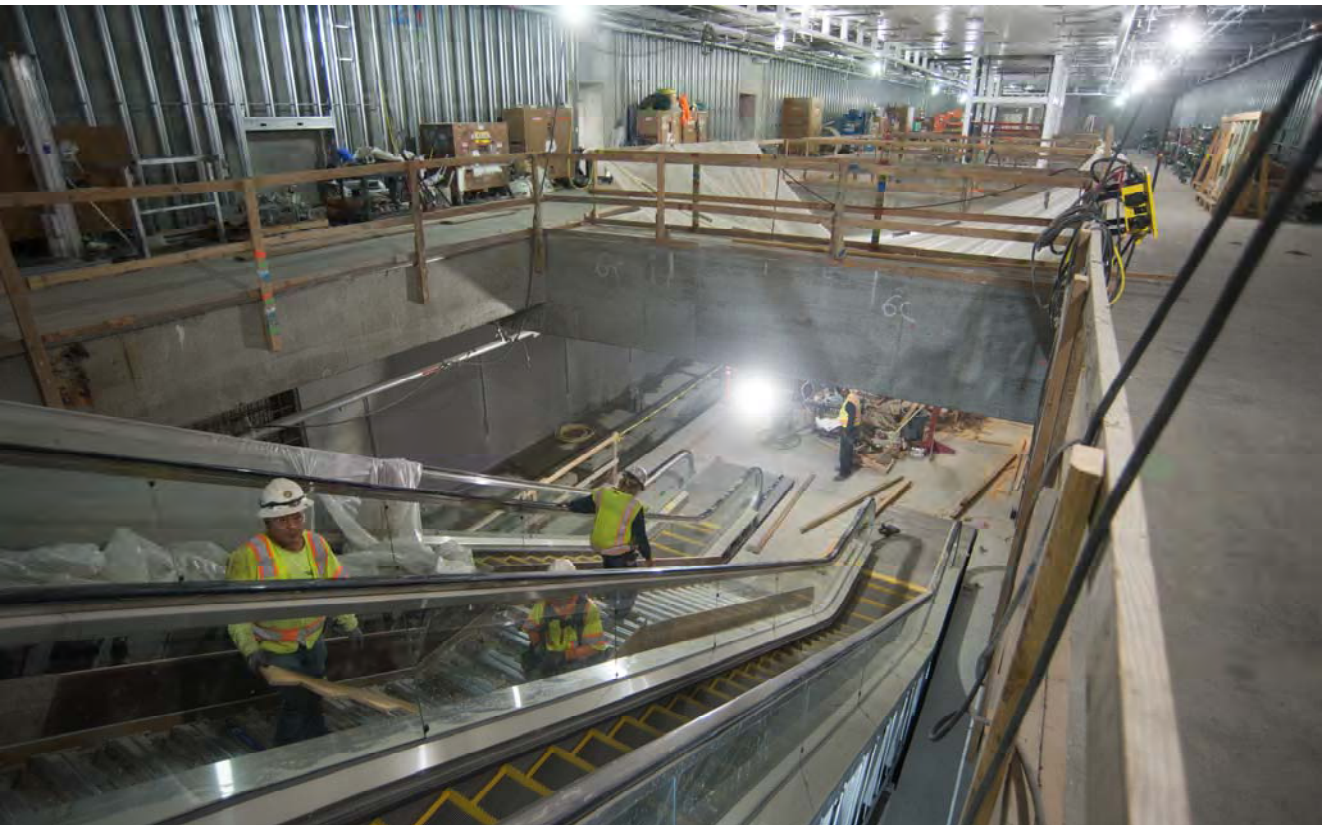
Rebar is being installed atop corrugated steel used as an underlay to build stairs between two escalators leading to the station platform from the concourse level.
