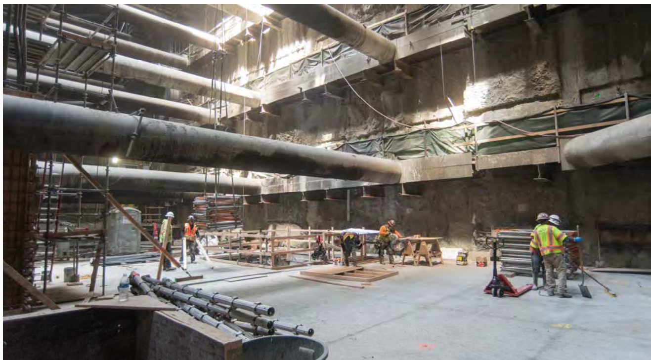
Carpenters construct concrete formwork atop a finished section of the platform level floor slab inside the Chinatown Station headhouse.
