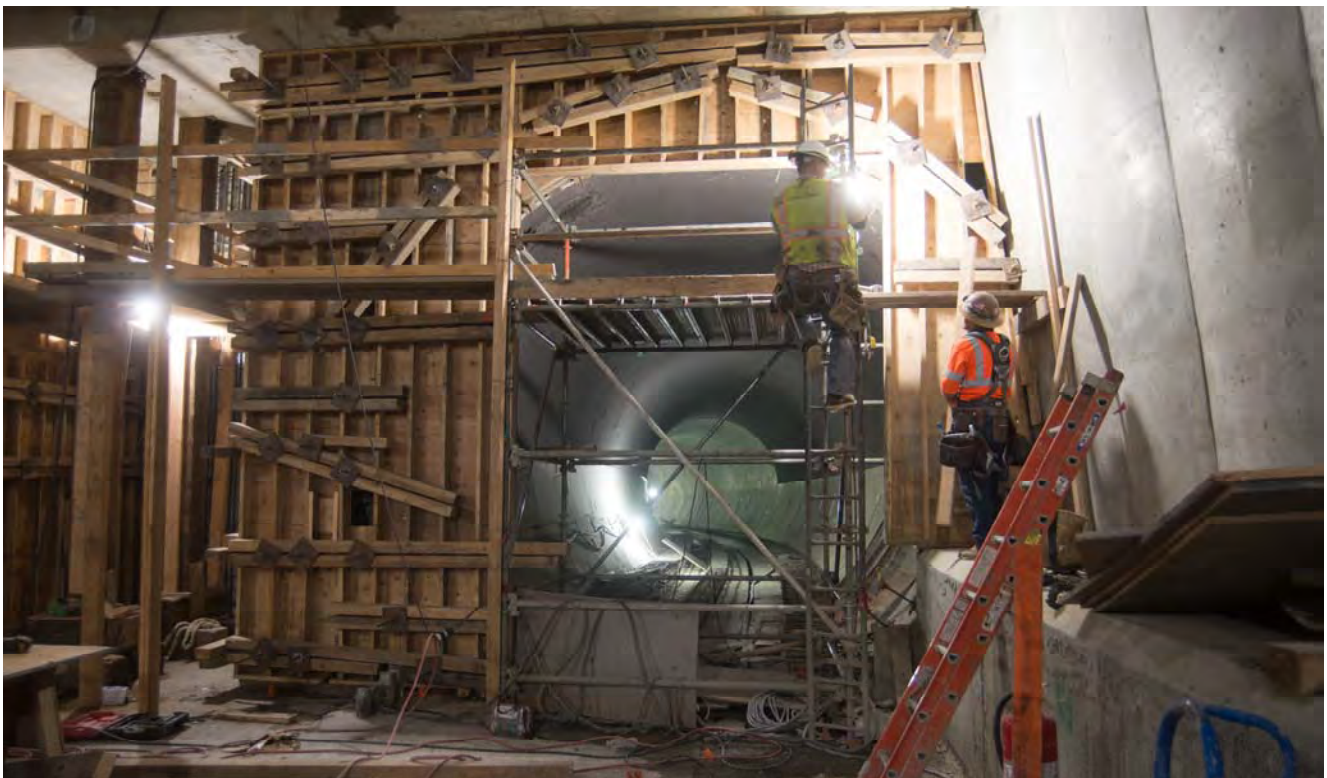
Massive concrete forms were built around rebar cages at the south headwall of the platform level, to build final structural walls at the south end of the station's lowest level.
