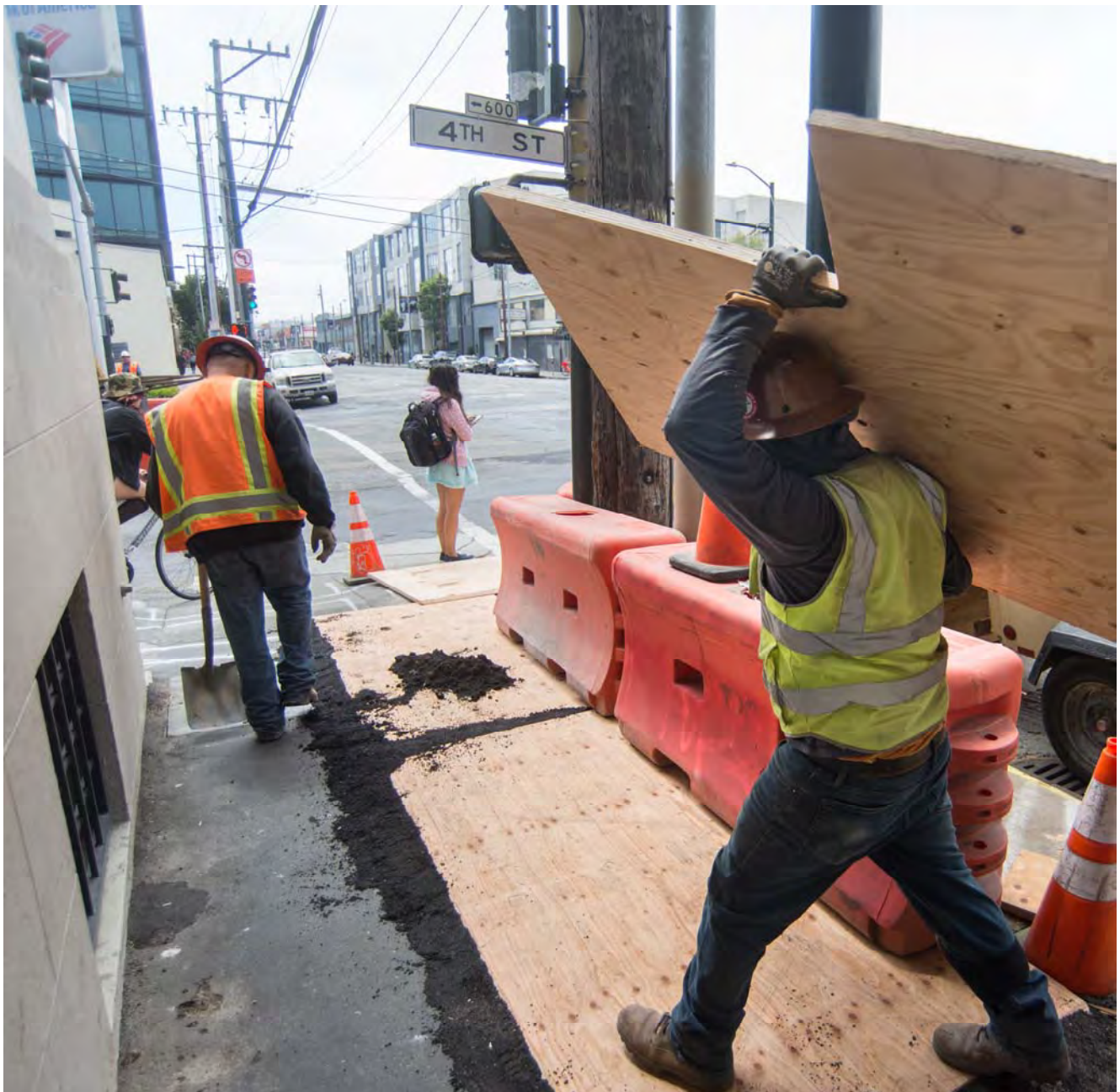
A worker hoists a piece of plywood used to cover a portion of shallow utility trenches along the sidewalk at 4th and Brannan.
