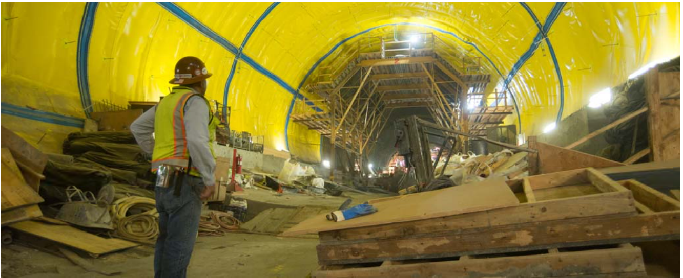
A safety inspector looks down the Chinatown Station platform cavern to a large scaffolding used to install rebar against the outer shell and yellow waterproofing.
