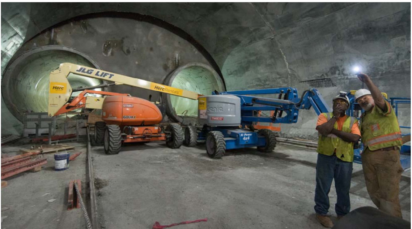
Workers review construction of the inner shell of the Chinatown Station track crossover cavern, a cavern just south of the future station platform where trains will be able to cross between tracks and turn around before heading outbound.
