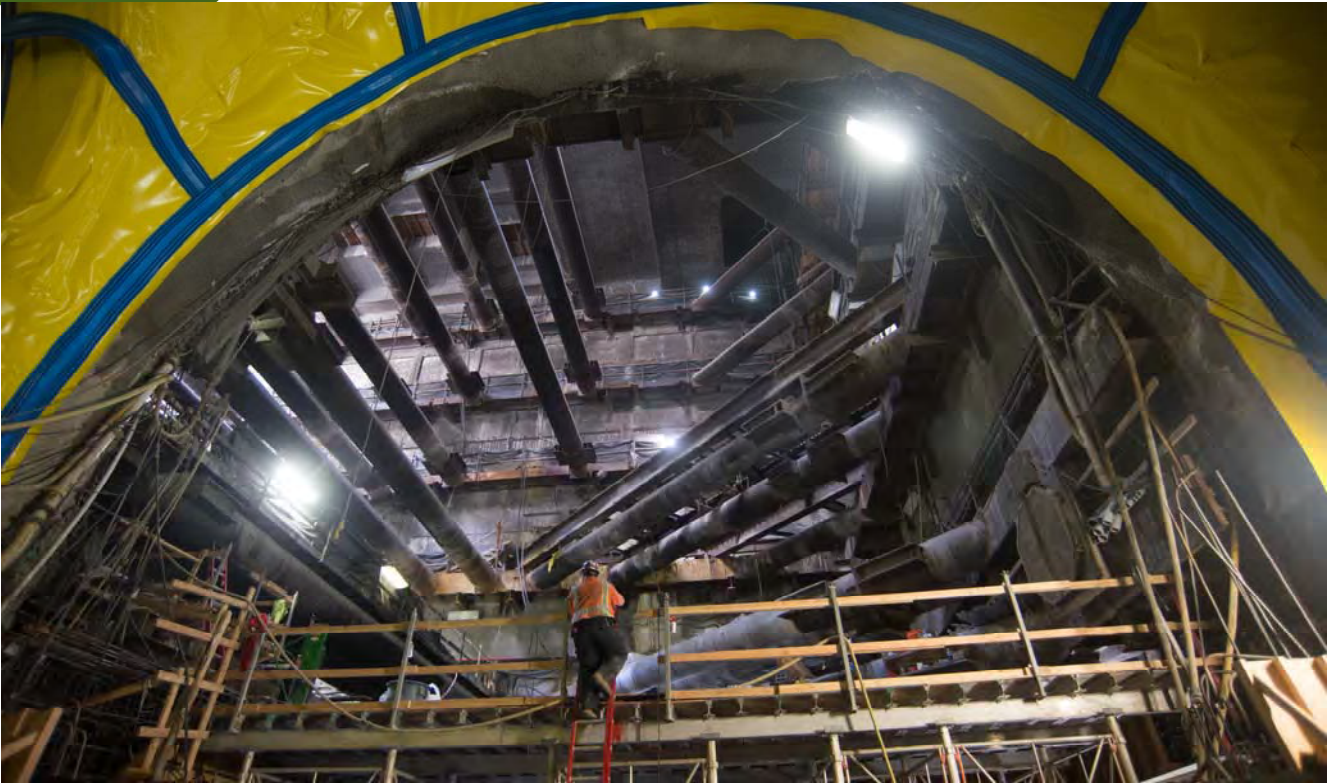
A worker climbs the ladder from the under-platform level to the platform level at the entrance archway between the headhouse and station cavern.
