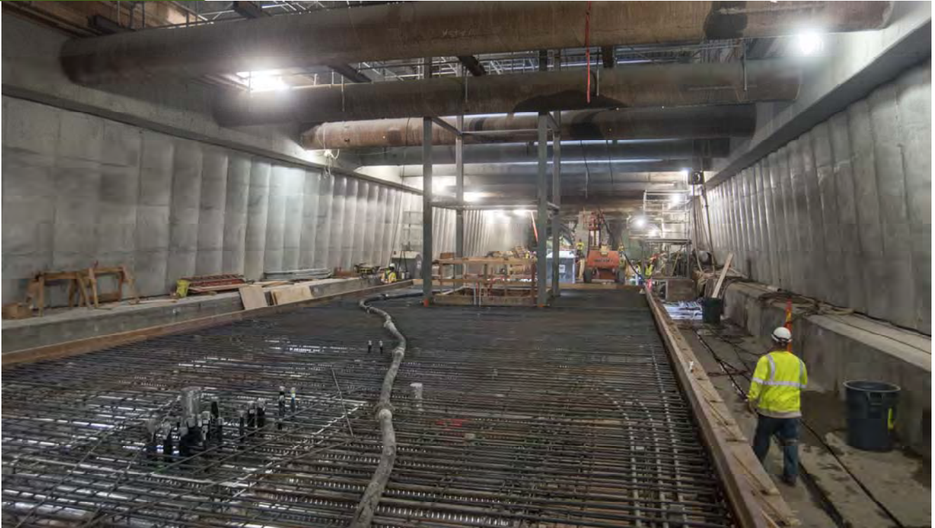
Rebar and formwork has been placed to construct the first section of structural slab for the Union Square/Market Street Station platform.
