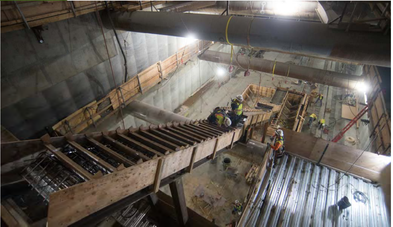
Concrete forms and rebar can be seen in place to construct stairs leading from the south concourse down to the station platform. These future stairs will be flanked by escalators.
