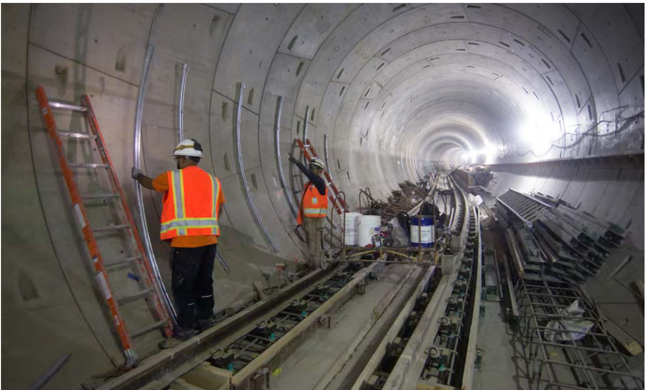
Workers install curved strut brackets against the outside walls of the northbound tunnel at the Market Street S-curve. These brackets will be used to mount utility conduits.
