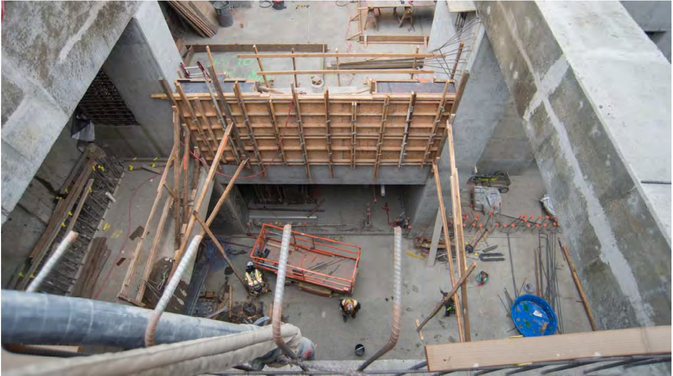
Looking down into an opening in the Yerba Buena/Moscone Station headhouse roof slab, workers are building additional concrete forms for future escalator supports.
