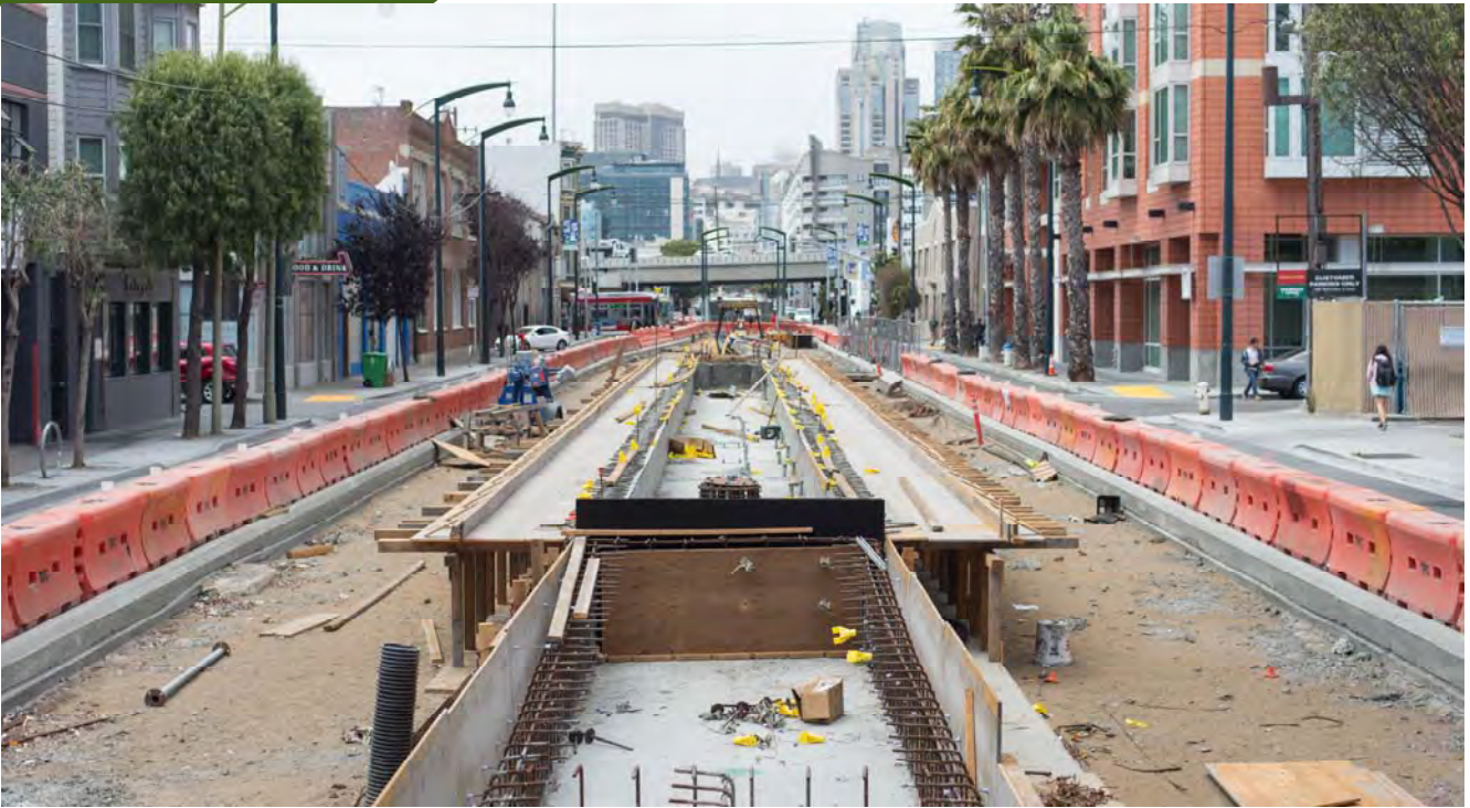
Concrete forms and temporary reinforcing have been built to prepare for construction of the 4th and Brannan surface station platform.
