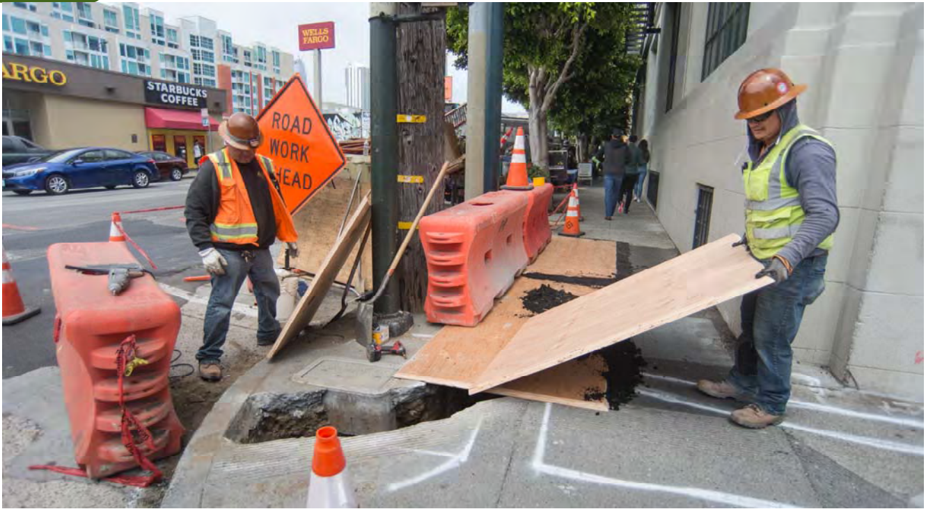
Workers cover open holes following trenching work to install underground electrical conduits at the 4th and Brannan intersection.
