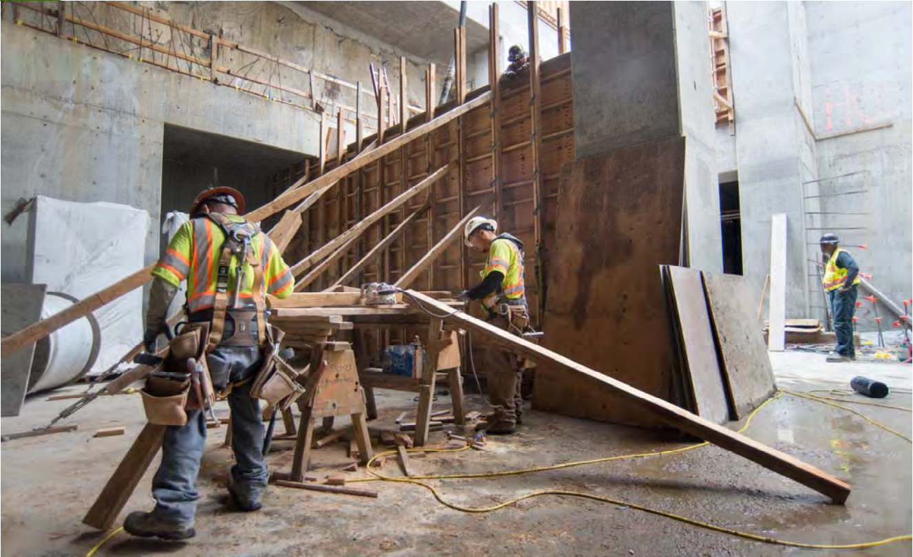
Carpenters build formwork to construct internal support walls where escalators will eventually be installed inside the Yerba Buena/Moscone Station headhouse.
