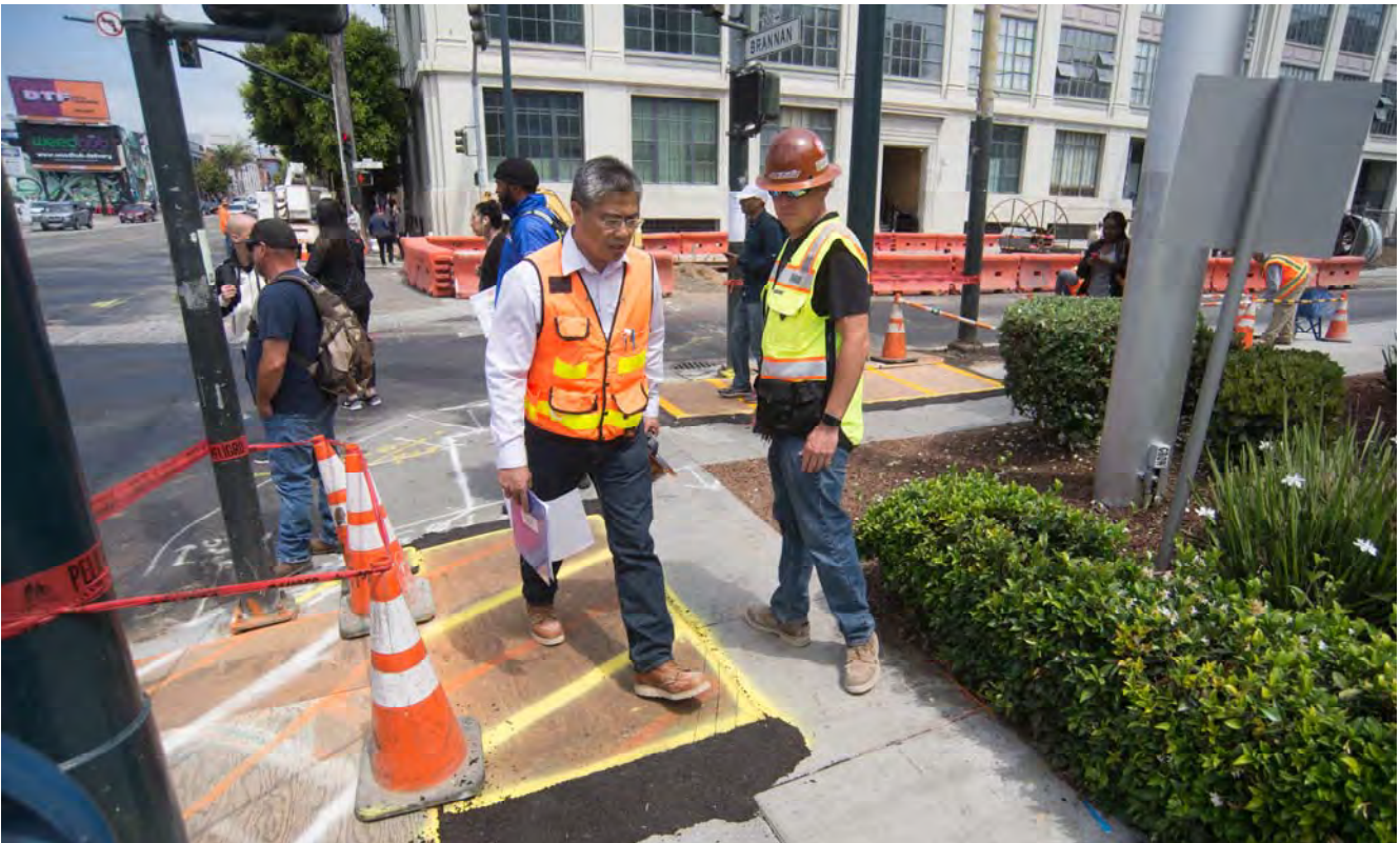
Plywood sheets cover holes dug to expose and examine the locations of existing utilities at the 4th and Brannan intersection.
