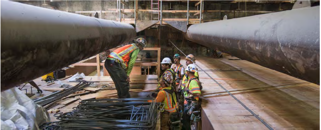
A crew meets to discuss next steps during construction of rebar cages for the platform level floor slab inside the Chinatown Station headhouse.
