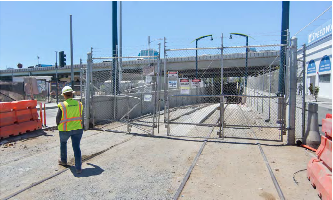
A site attendant finishes locking the access gates at the top of the tunnel portal ramp following the end of the workday.
