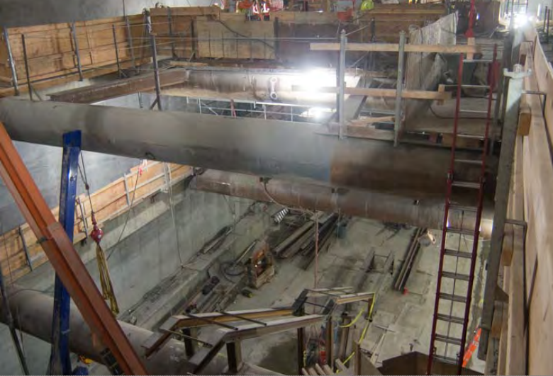
1. Structural steel is built from the platform level upward, attached to struts
