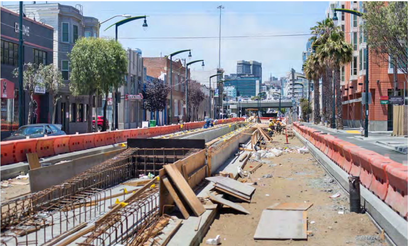
Looking up 4th Street from Brannan, the initial stages of prep work to construct the 4th and Brannan Station's platform have begun.
