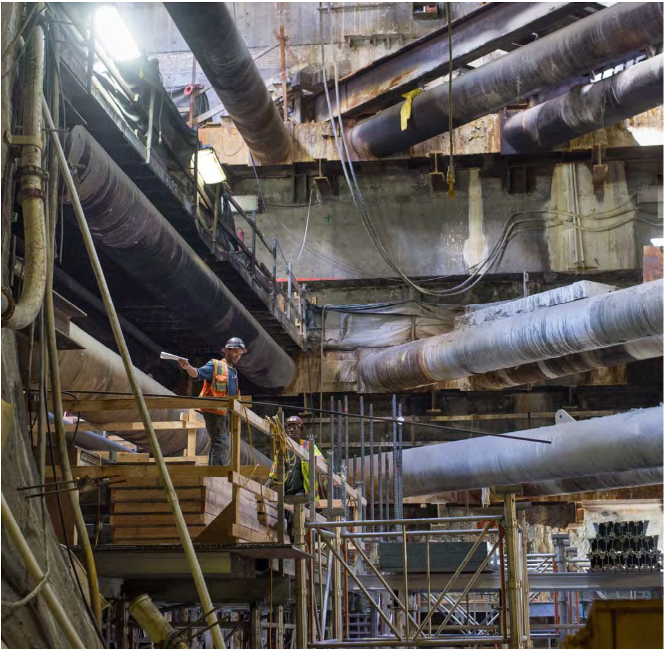
Large steel reinforcing elements span across the Chinatown Station headhouse while workers discuss operations atop platform level concrete formwork.
