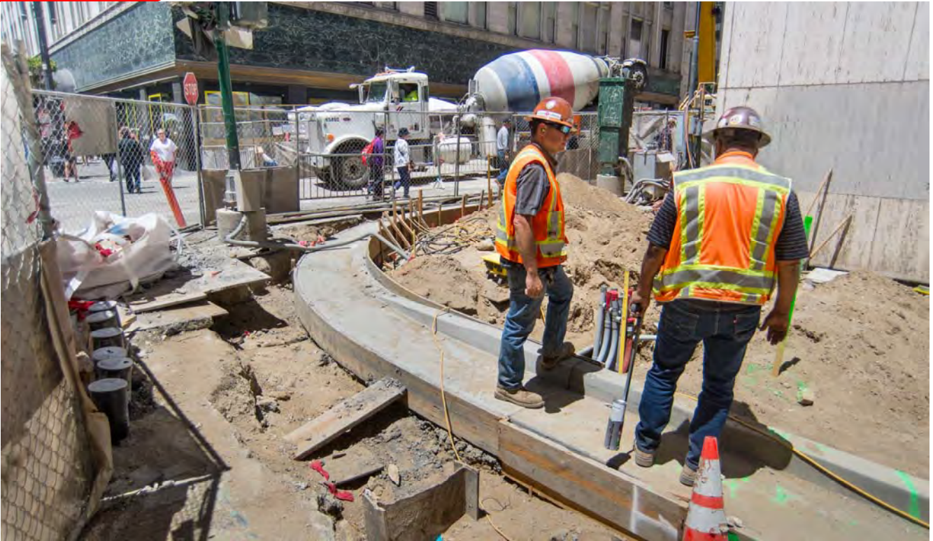
A new curb has been constructed at the northeast corner of Stockton and O'Farrell as part of roadway and sidewalk restoration work, following the completion of emergency egress stairs.
