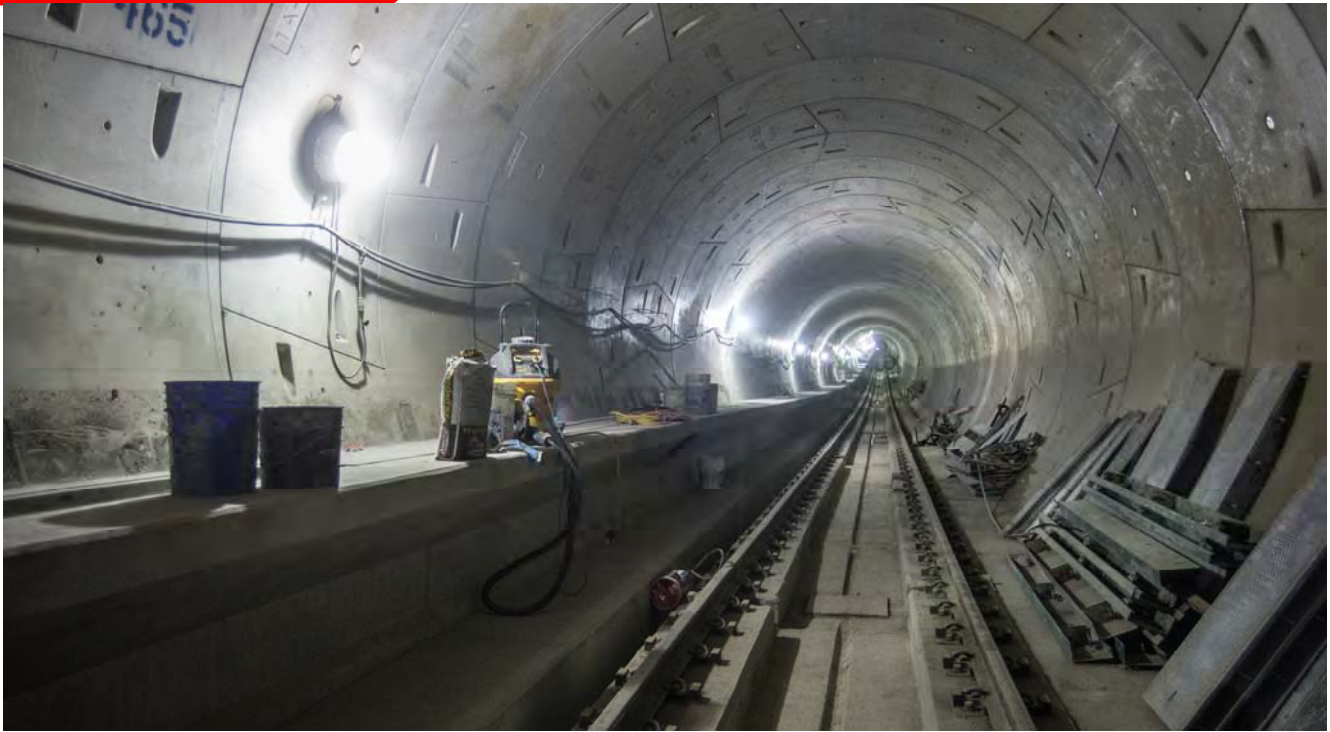
Crews have conducted some tunnel and equipment cleanup work near cross-passage five, just south of the Market Street S-curve.
