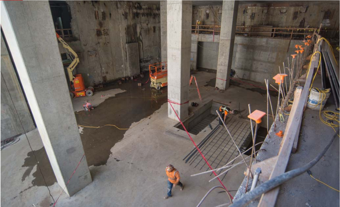
Looking southeast inside the Yerba Buena/Moscone Station headhouse, the recessed footing for an escalator is being filled in with rebar and later concrete.
