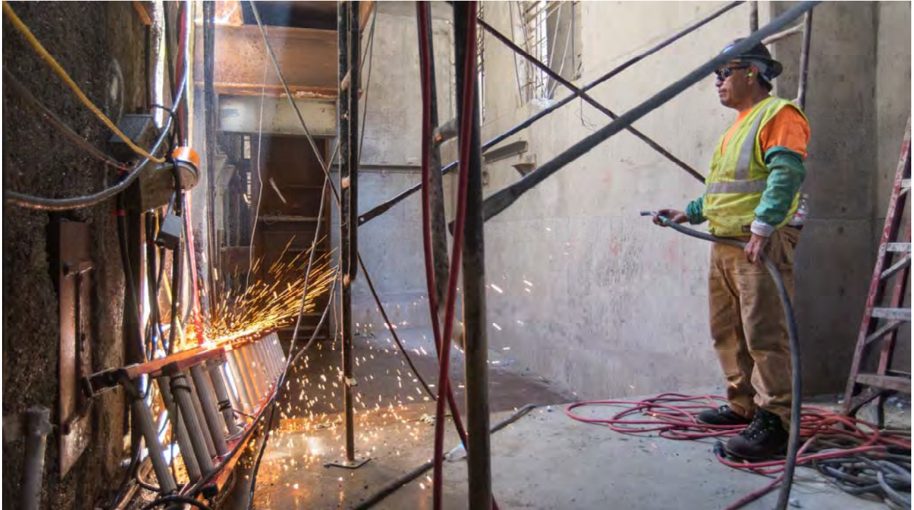
A man waits to spray water on sparks falling from an associate cutting temporary reinforcing beams on the east wall of the Yerba Buena/Moscone Station headhouse.
