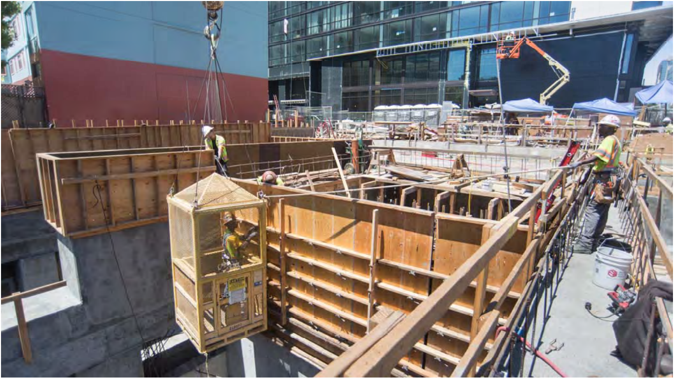
A worker in a man cage constructs concrete forms, while being supported by two associates on the street level roof slab for the Yerba Buena/Moscone Station headhouse.
