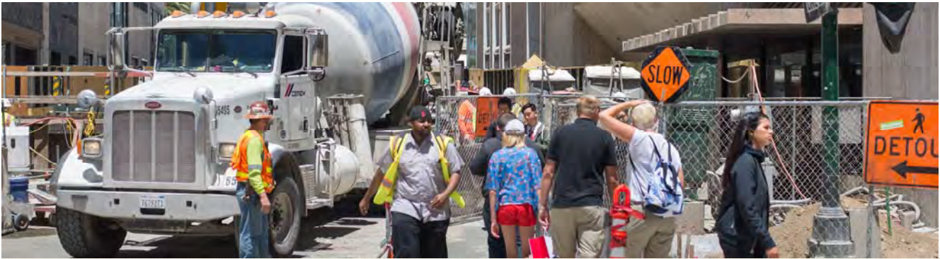
Pedestrians at O'Farrell and Stockton pass by an active concrete pour for shotcrete work in the Union Square/Market Street Station below.
