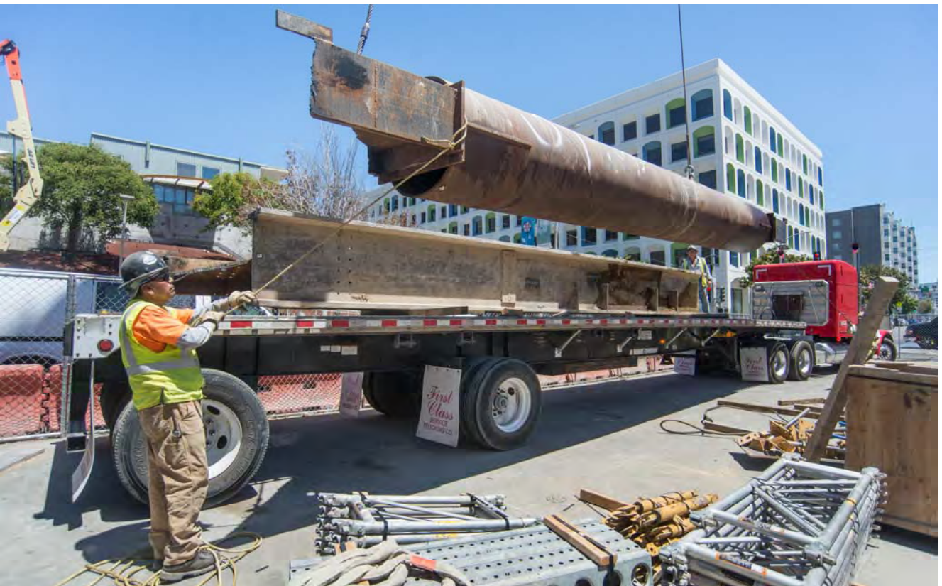
At the surface staging area on the west side of 4th north of Folsom, a large strut is carefully lowered into place atop a flatbed truck for removal offside.
