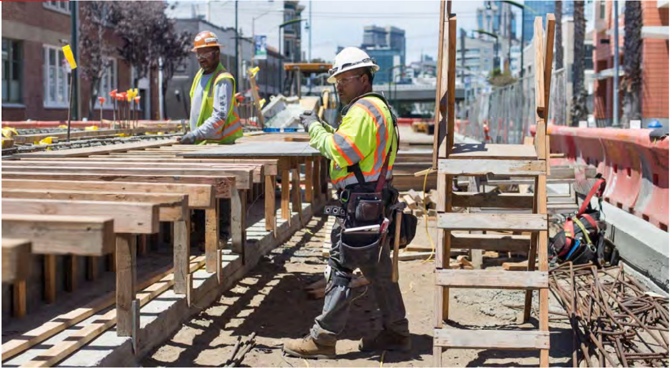
Carpenters construct formwork for the east side of the 4th and Brannan Station platform.
