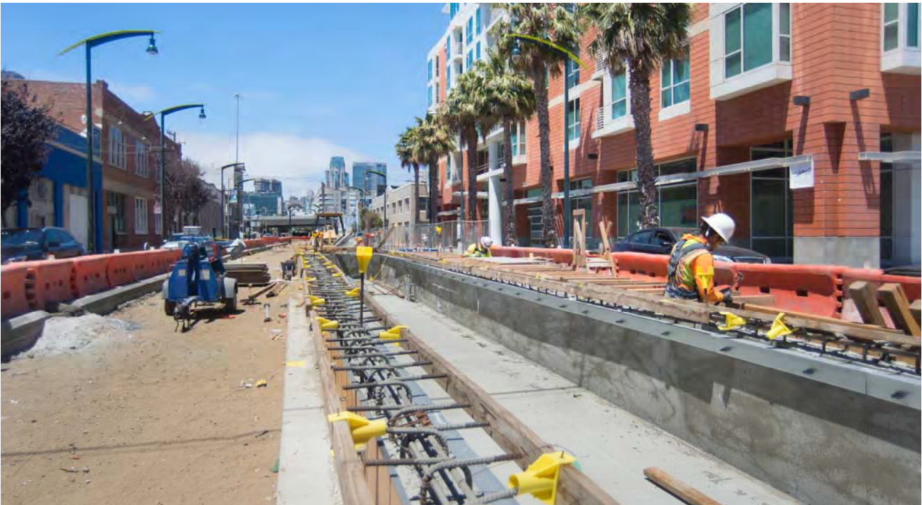
Crews have resumed work constructing the platform of the 4th and Brannan surface station in SoMa.
