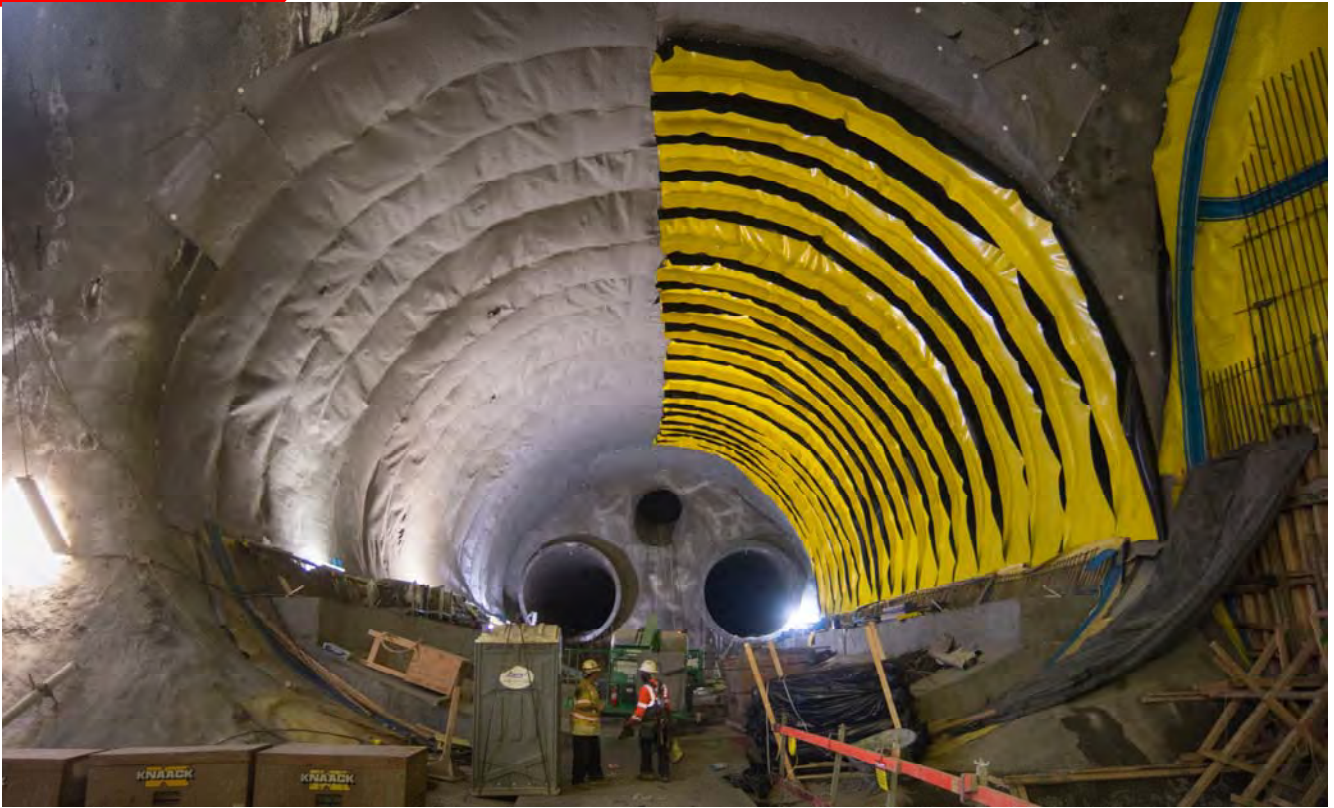
Workers have begun to install sheets of vinyl waterproofing against the east wall and ceiling of the north platform cavern.
