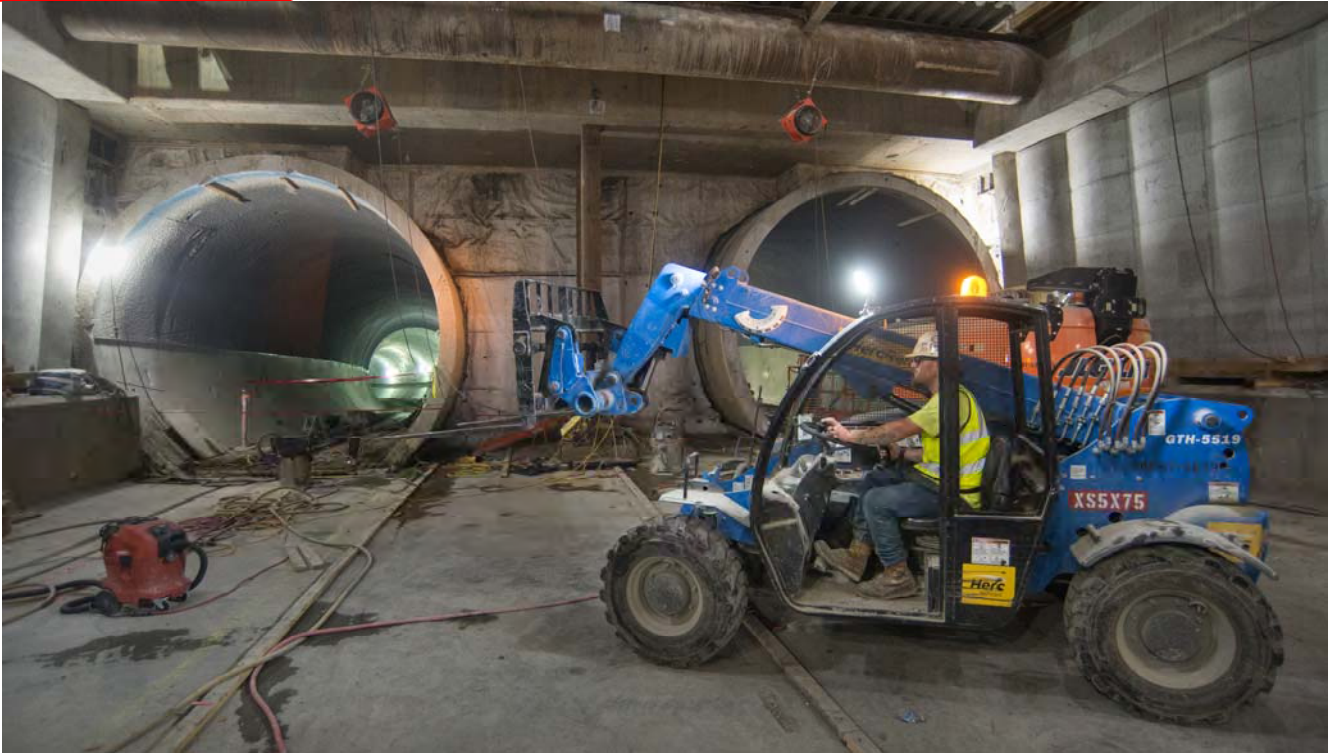
A forklift operator navigates equipment at the south end of the Union Square/Market Station's platform level.
