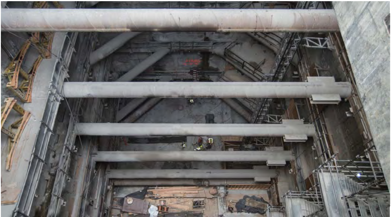
Multiple levels of temporary cross-bracing span the width of the Chinatown Station headhouse as seen from the edge of the main access shaft looking south.
