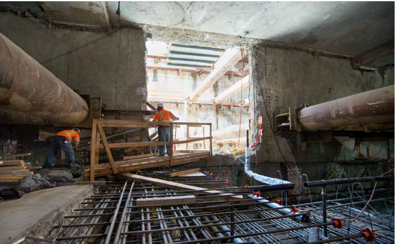
Sections of PVC conduit are brought in following the completion of the southernmost section of platform level invert slab. One section remains, adjacent to the headhouse access portal.
