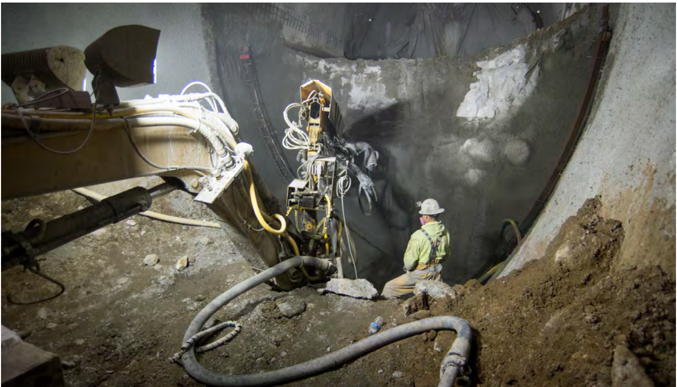
A crew sprays shotcrete on reinforcing steel mesh inside the left side drift invert of the north platform cavern.
