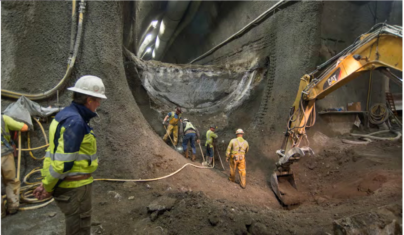
Workers loosen material inside the left side drift invert, which is then transferred by excavator to a waiting bulldozer for storage inside the headhouse before being brought to the
