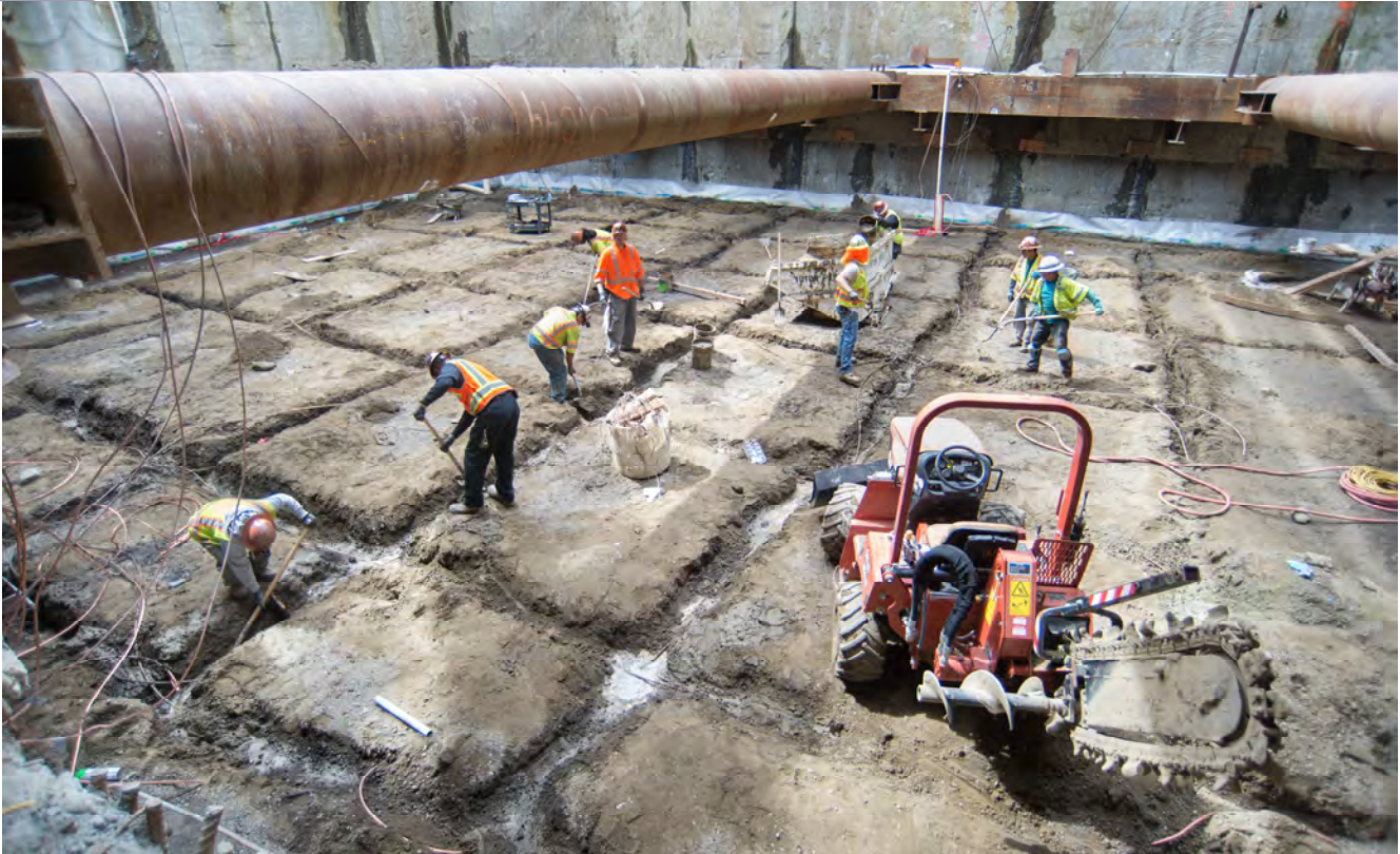
A crew clears out small trenches following rain inside the headhouse, where the massive lattice of copper grounding wire will be installed.
