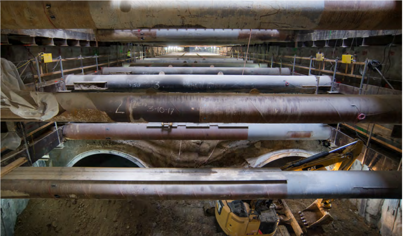
Looking south from the north headwall inside the station box under Stockton Street, crews have excavated far enough down to begin removing tunnel ring segments.
