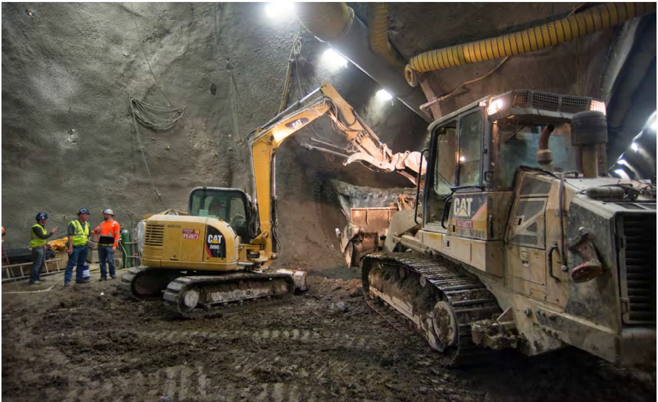
An excavator and bulldozer operate as a team removing material from invert excavation for the left side drift of the south platform cavern.
