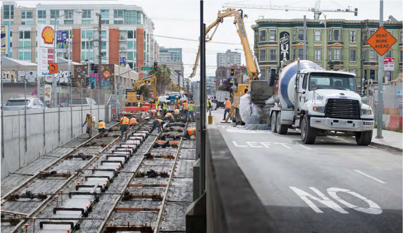
Looking south from under the I-80 overpass, the concrete pour for the remaining portions of the tunnel portal invert slab is wrapping up.
