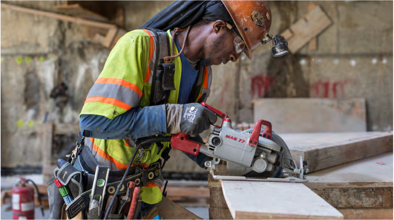
A carpenter fashions a piece of plywood as part of concrete form assembly near the west wall of the headhouse.
