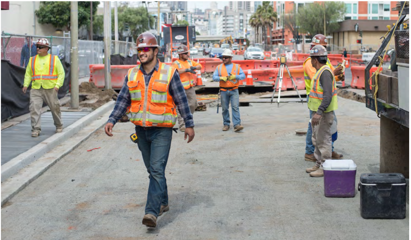
Workers break after grading a section of 4th Street north of an already-completed concrete road slab south of Brannan.
