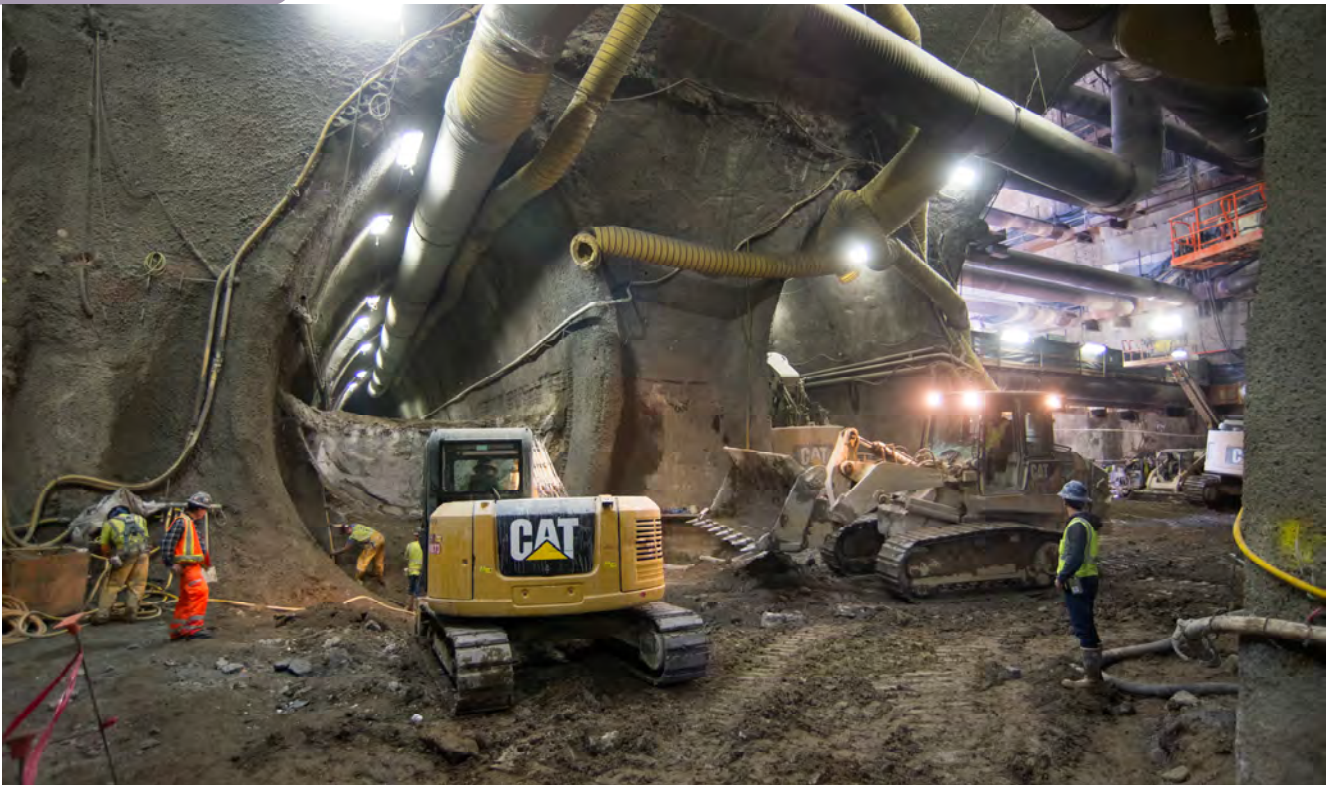
Bulldozer and excavator operators coordinate excavation operations inside the cross-cut cavern, where left side drift invert work for the south platform cavern has begun.
