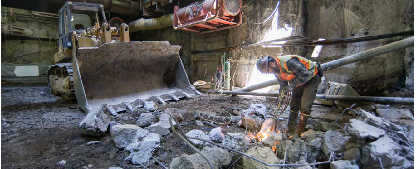
Sections of rebar collected in the Chinatown Station headhouse are cut away from demolished pieces of tunnel ring segments removed during excavation of the side drift inverts.
