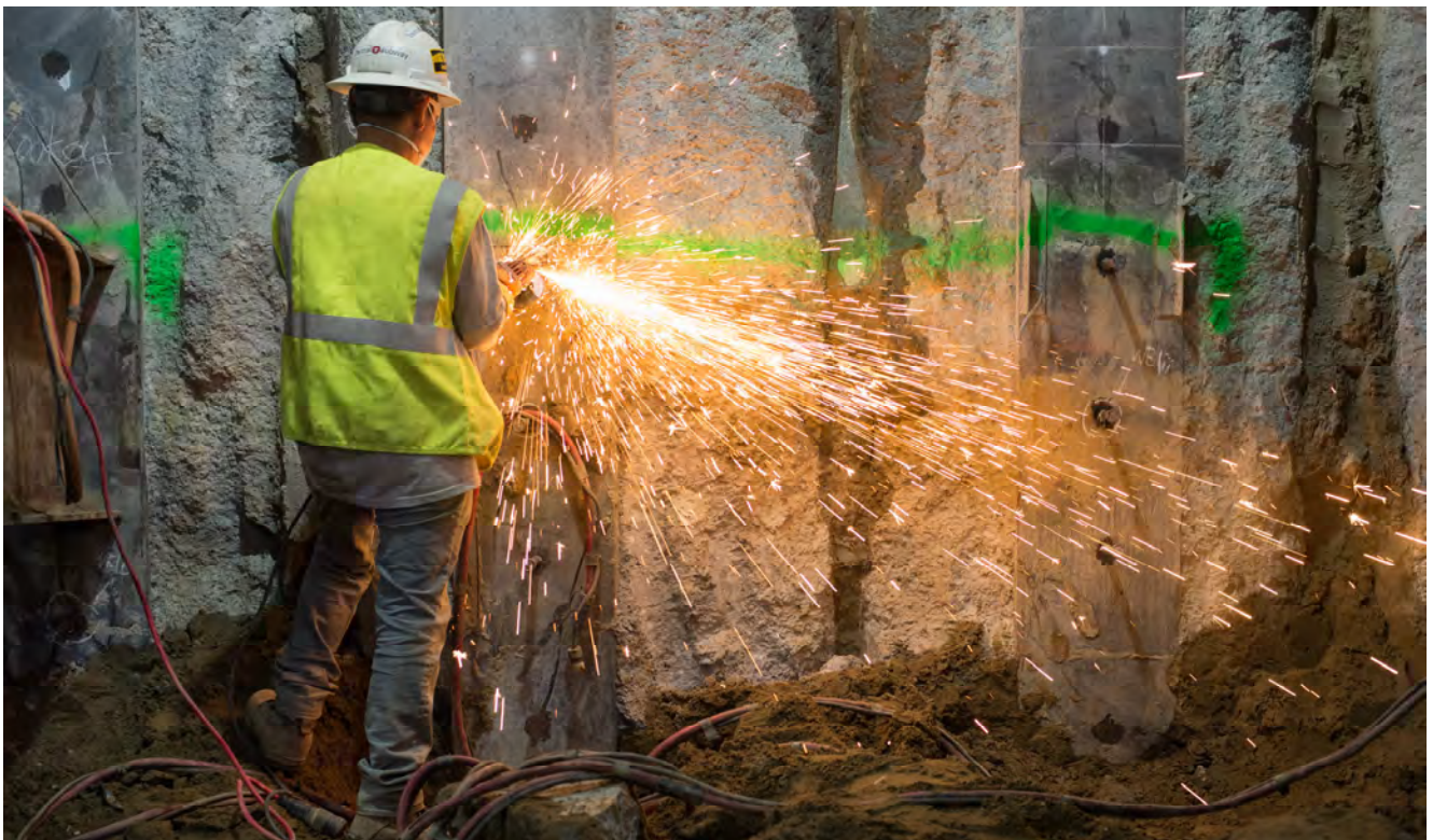
Vertical steel beams embedded in the exterior pile wall are prepared for welding small steel pegs as part of upcoming shotcrete reinforcing work.
