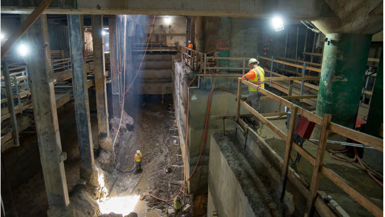
Light beams in through an access shaft at the southeast corner of Union Square, where workers are excavating the north concourse and installing tiebacks.
