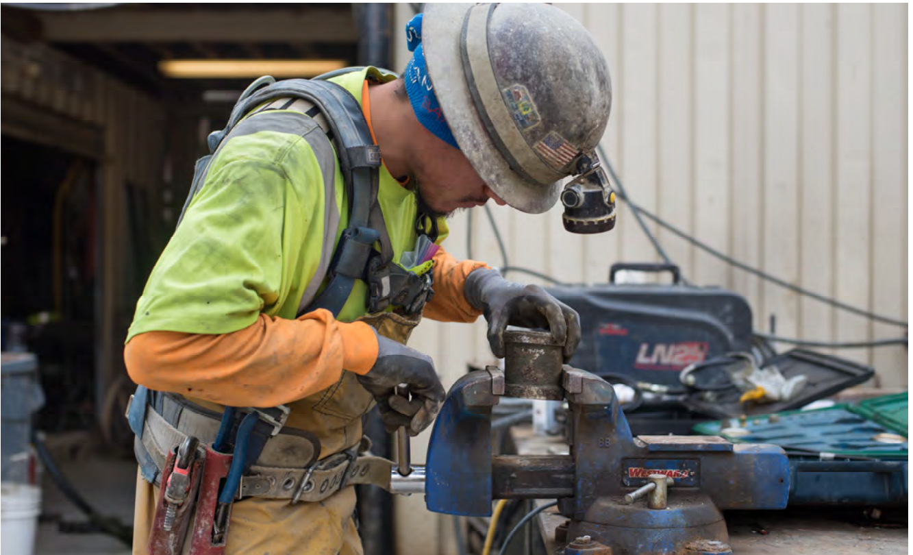
A worker prepares to alter a pipe joint at the surface work area on the south end of the roof deck of Chinatown Station.
