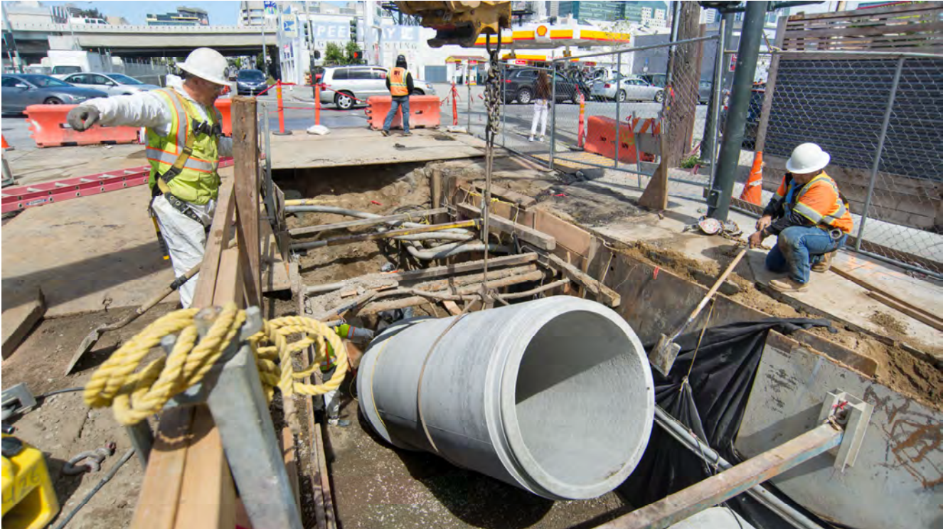
A new section of sewer pipe is carefully lowered into place on the east side of 4th just south of Bryant.
