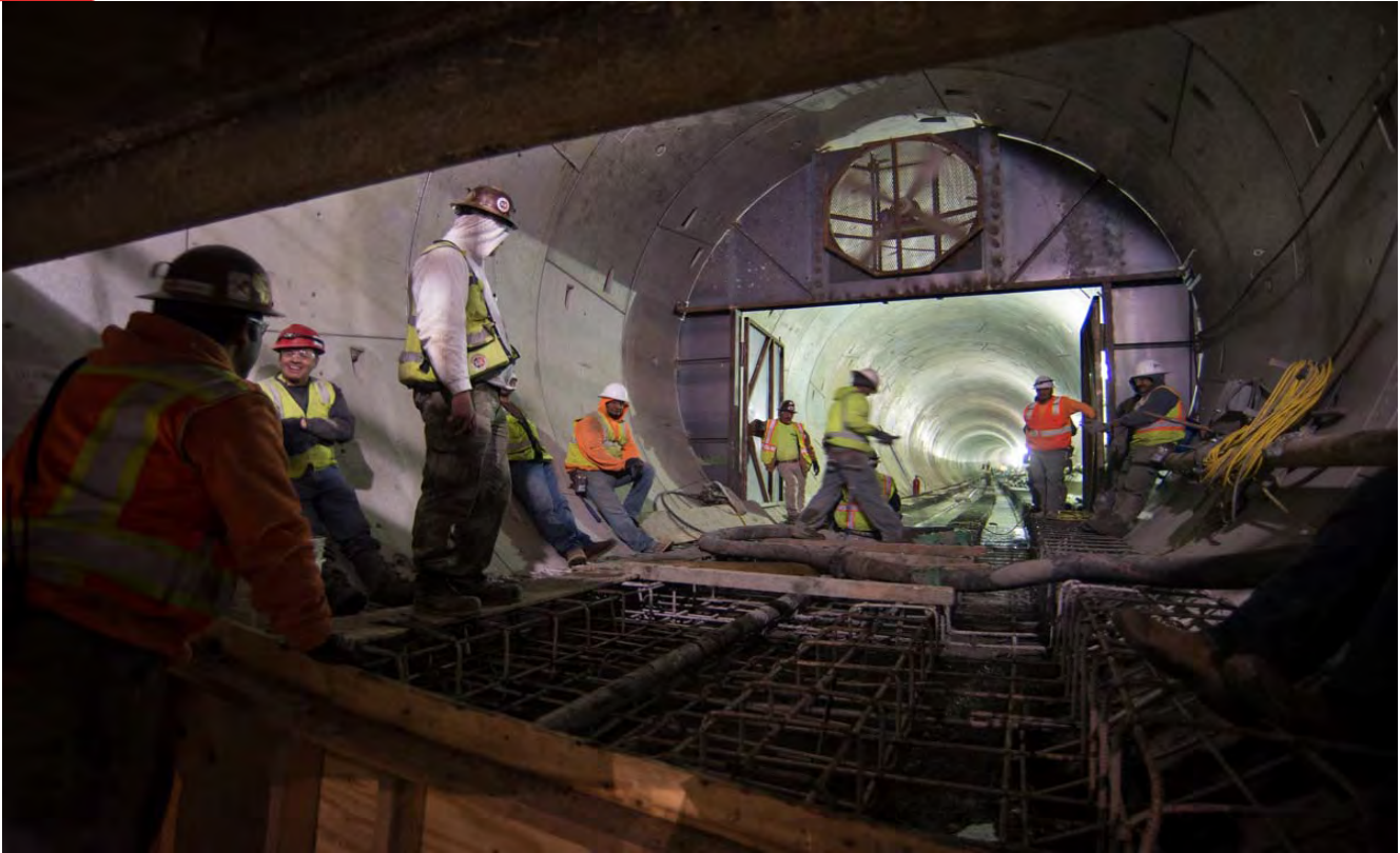
Workers placing rebar in preparation for pouring concrete for the invert into the tunnel at YBM.
