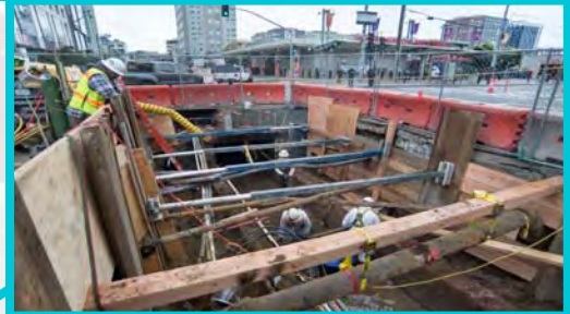
4th St. Surface Track, Systems (STS)
