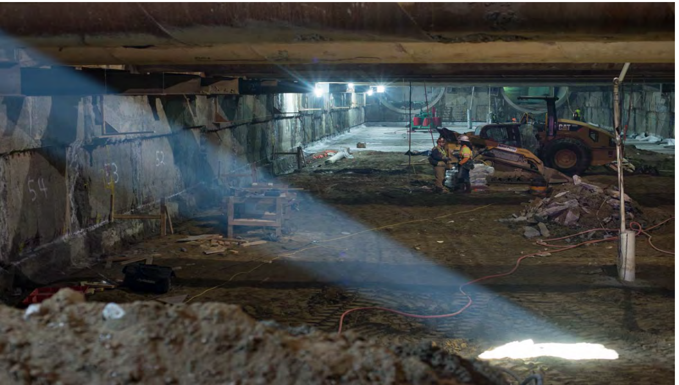
Workers install concrete forms at the base of the exterior slurry walls to prepare for eventual invert slab construction.
