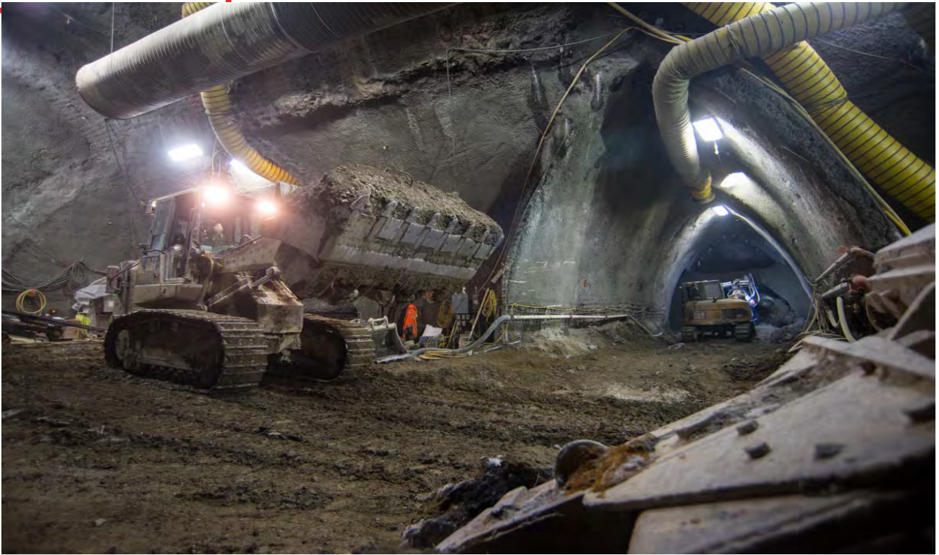
A worker coordinates with a bulldozer at the bottom of the headhouse to offload soil excavated from the cross-cut cavern and station cavern.
