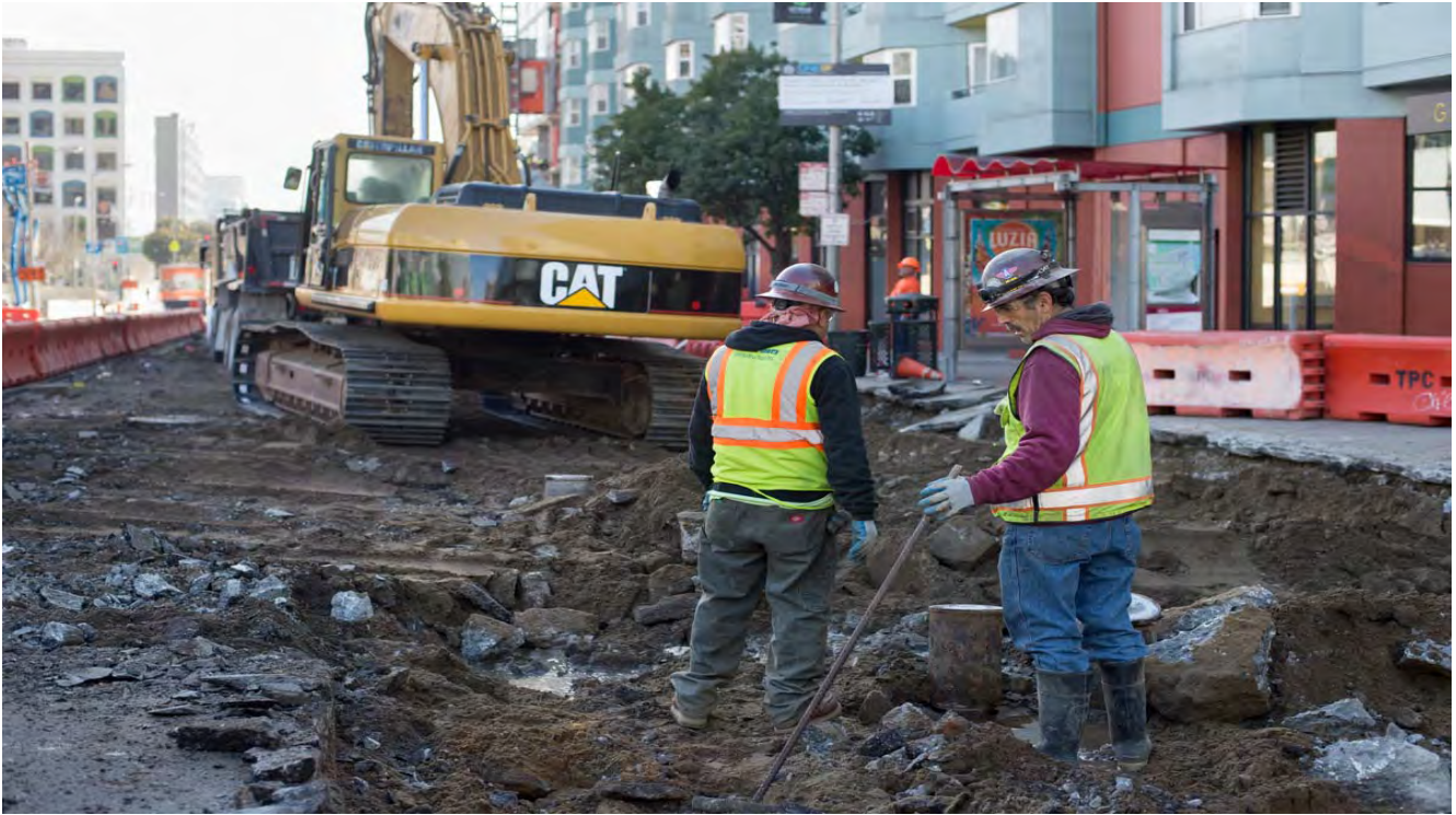
Workers in the process of performing demolition of roadway to allow required utility work to take place within 4th Street south of Howard.
