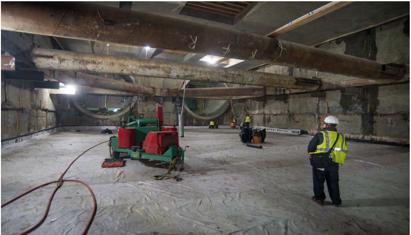
Workers are installing waterproofing beneath the invert level at YBM station. Temporary strut level 6 is in place prior to invert construction.
