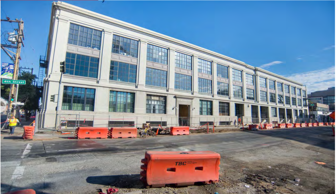
Workers have been restoring sections of 4th Street following the end of utility work in certain areas.
