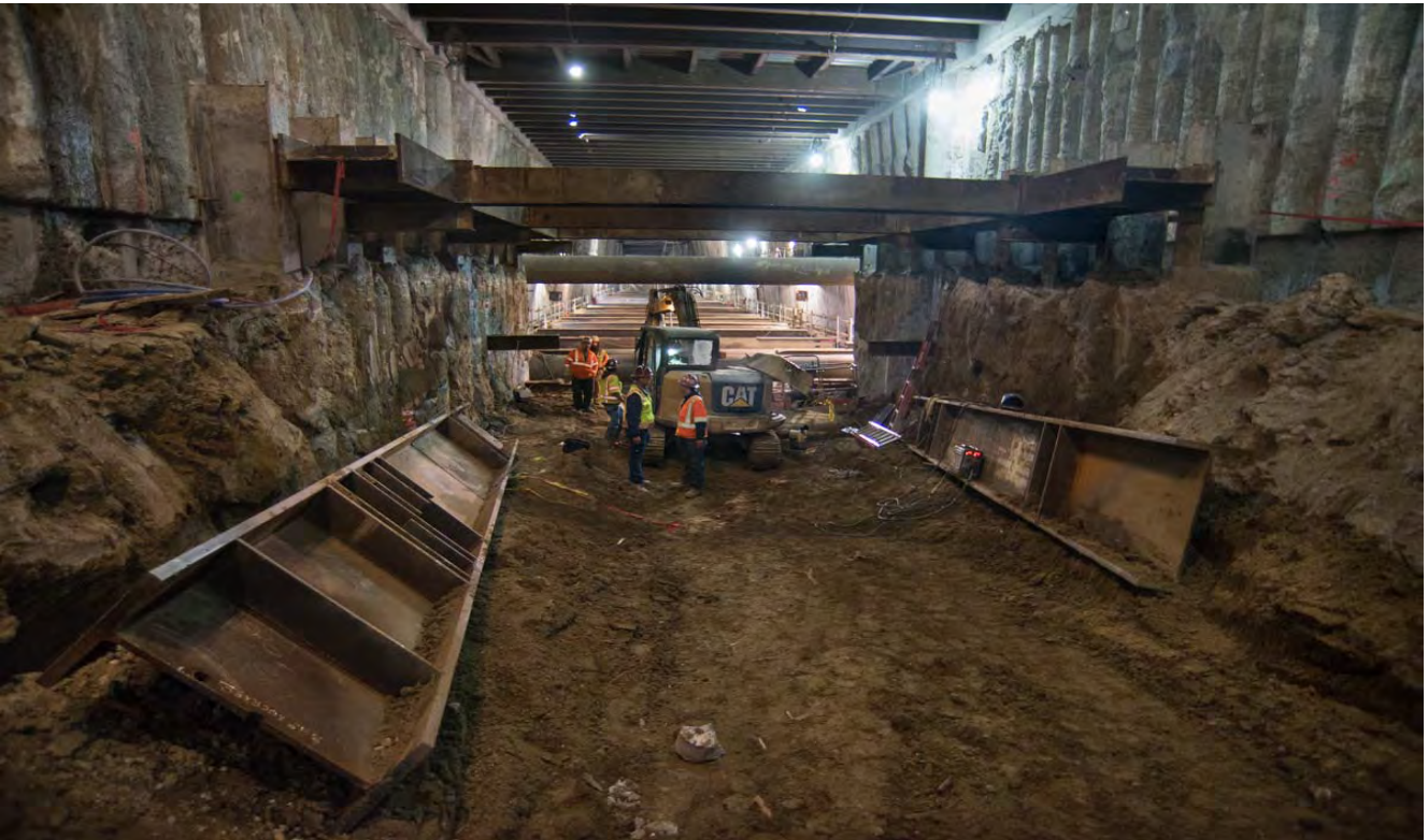
Work to excavate the next level of the station box continues under Stockton Street. This work is carried out underneath the Winter Walk and soil is removed at night.
