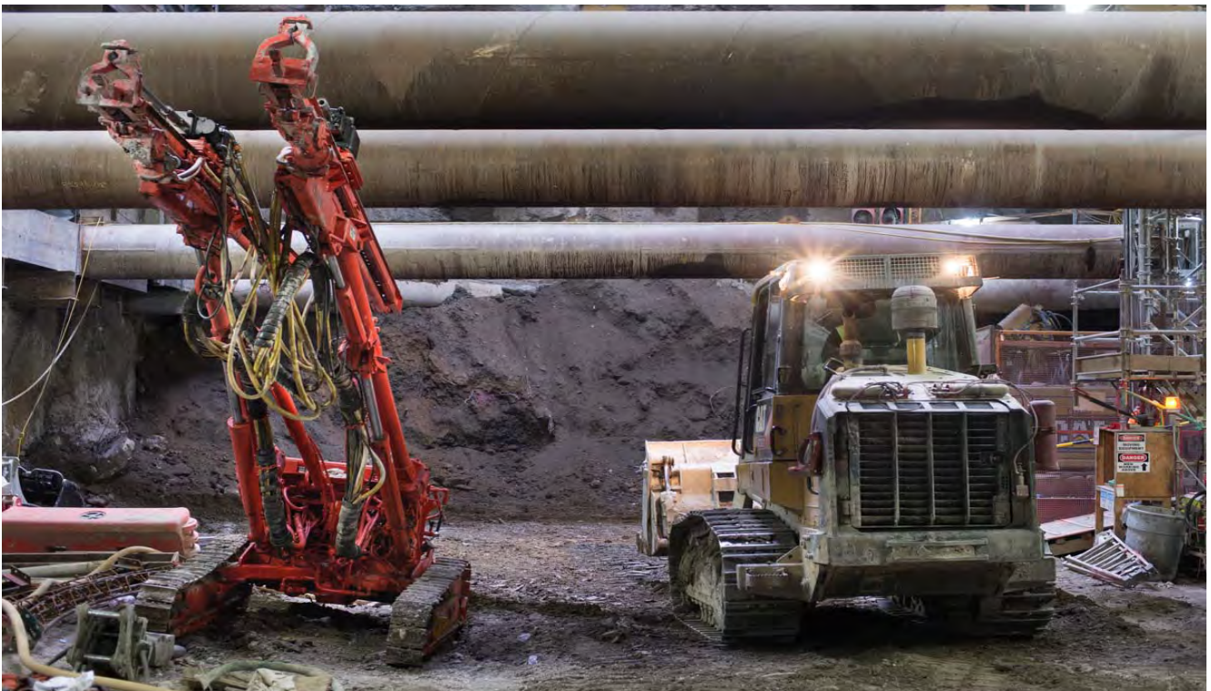
Stockpiled dirt waiting to be hauled up to street level and then off hauled to landfill.
