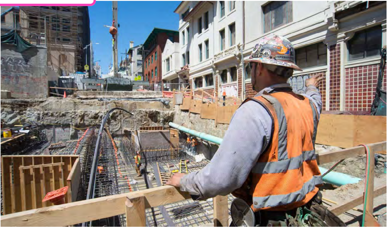
A worker gives hand signals to the crane operator to carefully lower rebar segments.
