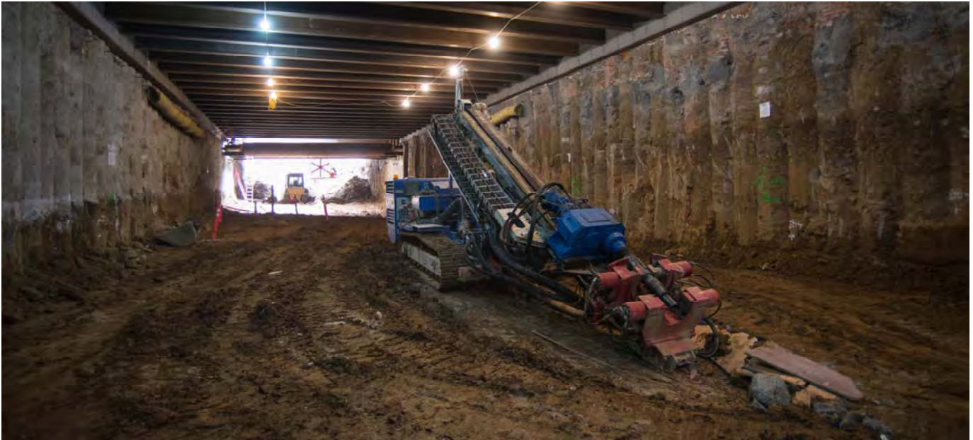
Underneath Stockton Street north of Ellis, a drill rig sits idle in the future south concourse to the Union Square/Market Street Station. This void was excavated during the latter half of 2014 and decked over.
