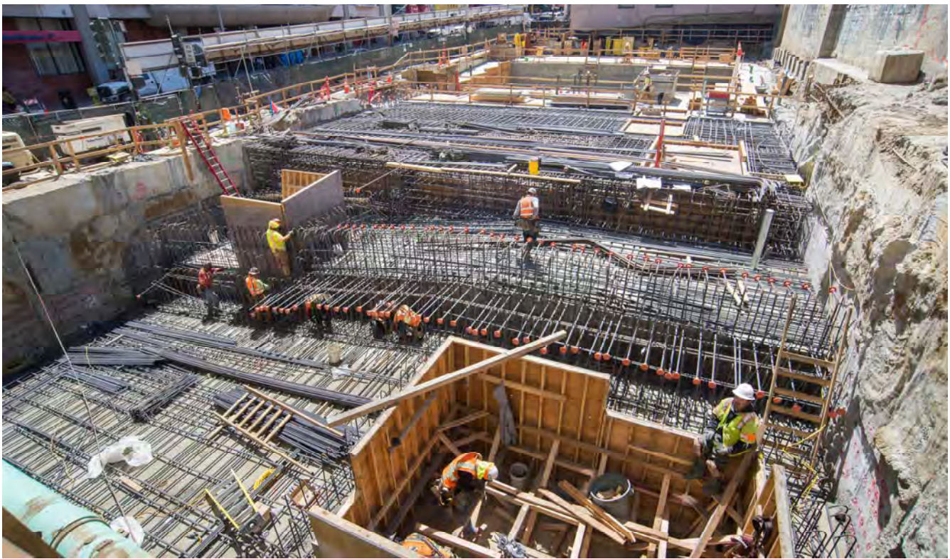
Toward the end of April, you can see varying stages of completion of the roof slab, with finished sections to the top of the photo, and initial stages of rebar laying at the bottom.
