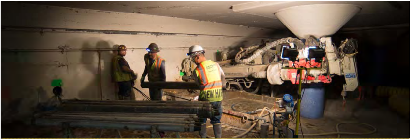
Inside the Union Square Garage, workers are currently drilling holes in the exterior walls to install tiebacks. These will help reinforce existing walls during reconstruction.
