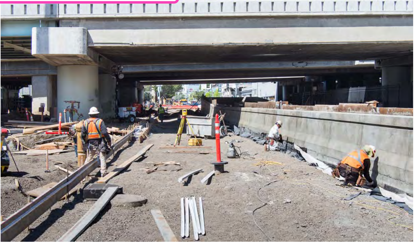
Workers install waterproofing near the bottom surface of the separating wall of the tunnel portal, while forms are constructed to pour the new curb and roadway.
