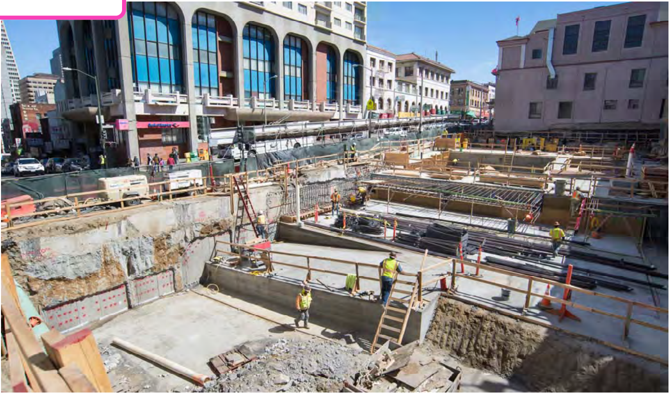
At the beginning of April, a temporary form slab can be seen being constructed.
