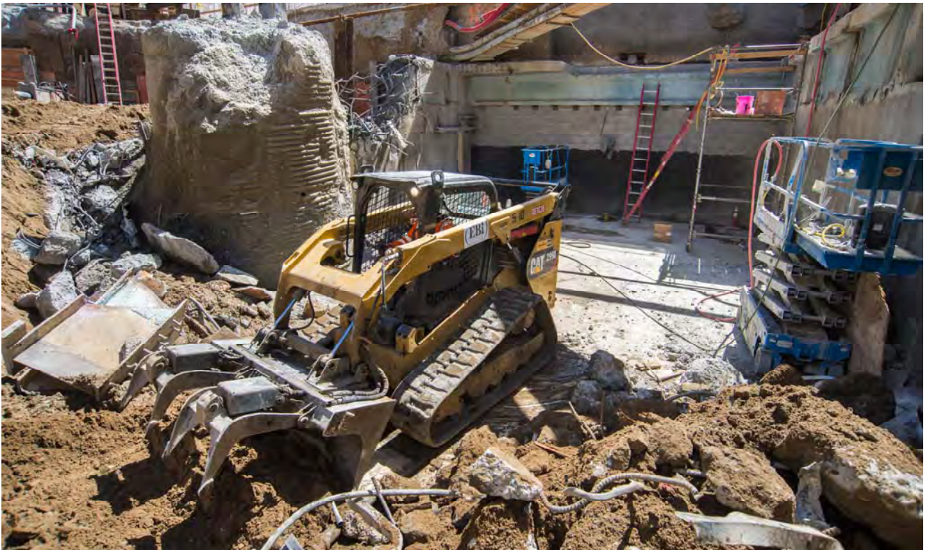
A bobcat operator sorts demolished material inside the former Ellis Street entrance to Powell Station.
