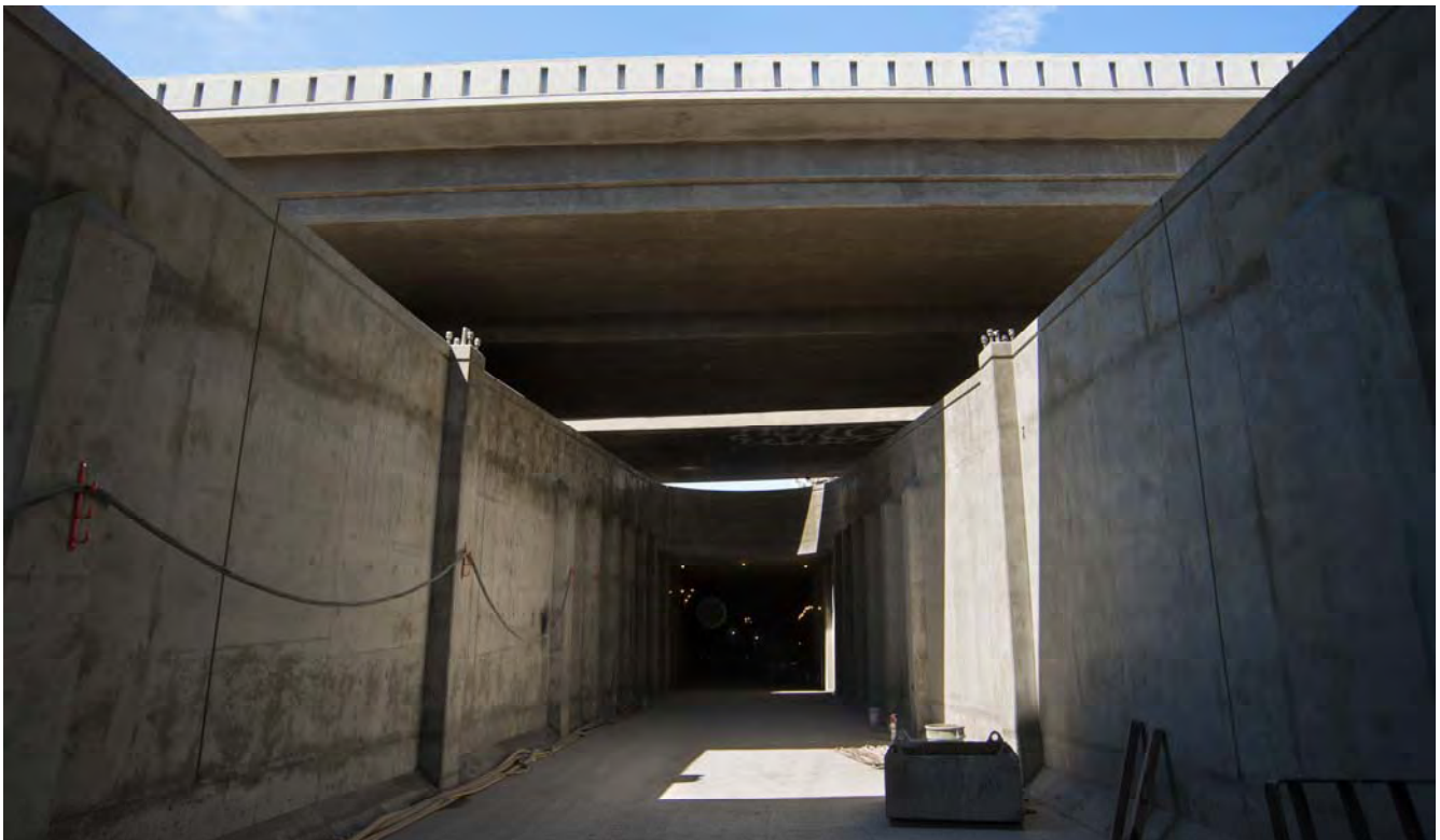
Looking down the tunnel portal, all the major structural elements are complete and ready to be handed to the systems contractor.
