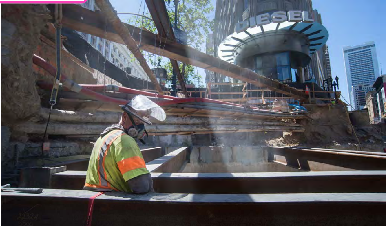
Work to construct the structural roof elements continues with live utilities suspended overhead. Eventually, the area above the roof will be backfilled and the roadway restored.
