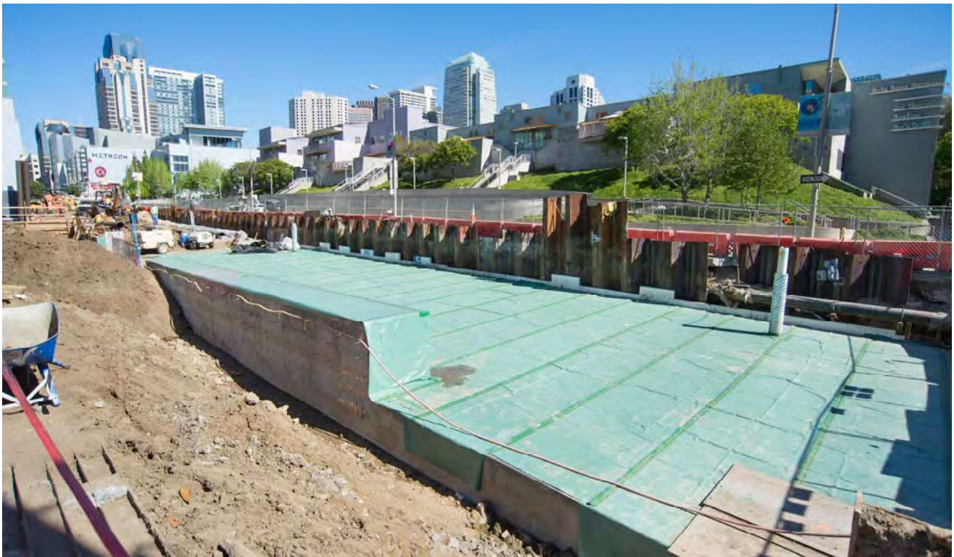
With the western portion of the roof slab complete, waterproofing material is installed.
