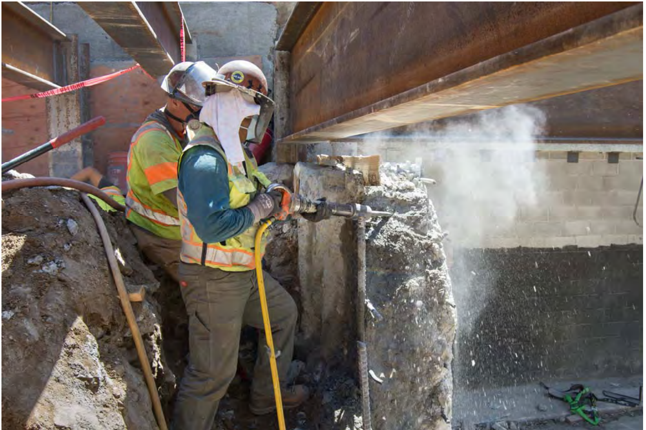
Workers remove former structural walls from the Ellis Street entrance to Powell Station, as part of efforts to reconstruct the entrance and connect with the new Union Square/Market Street Station.
