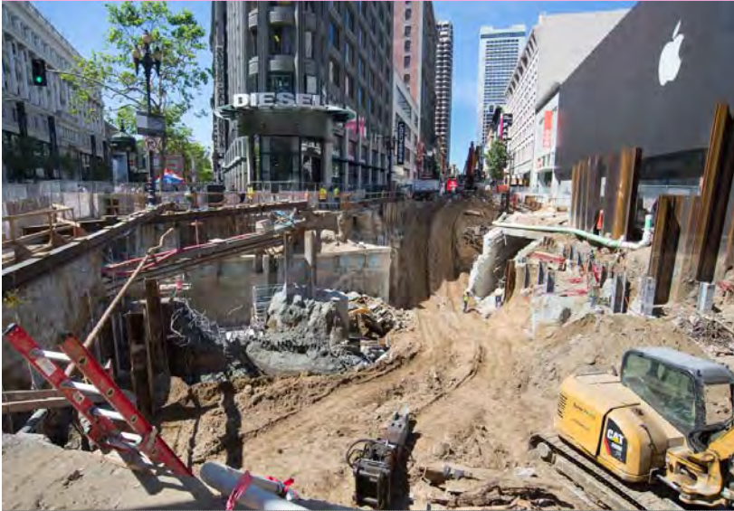
1 Soil is removed and legacy shoring walls from BART construction are removed
