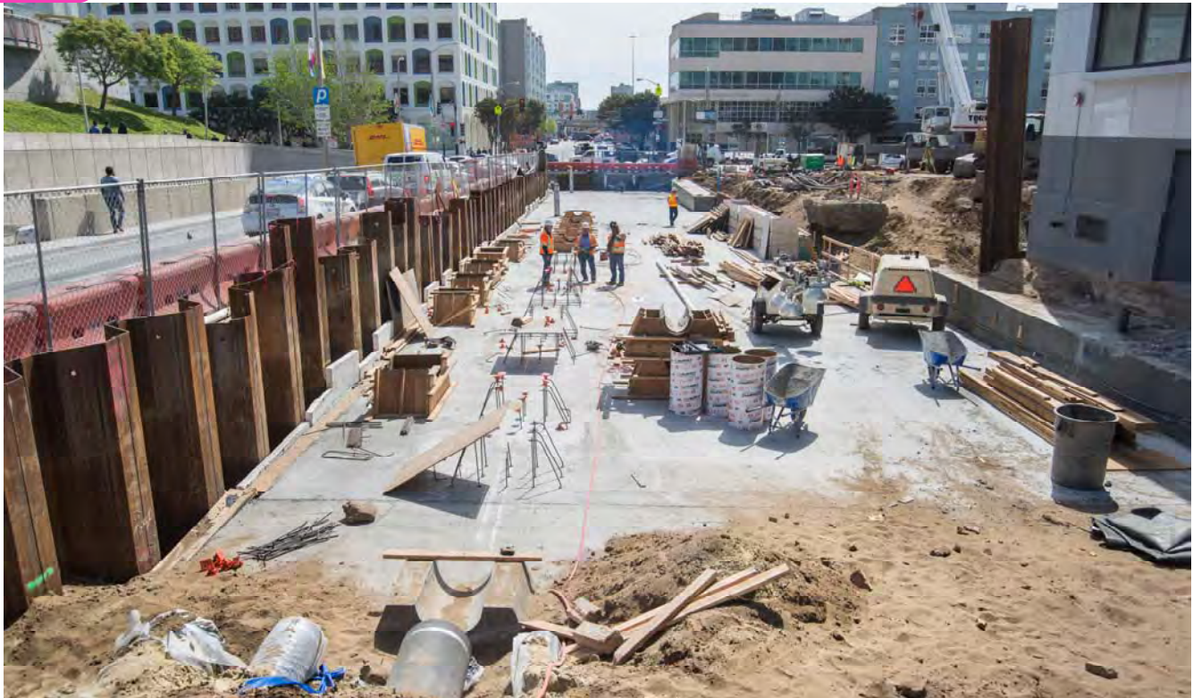
Now that the roof slab has been completed on the west side of 4th Street, utilities are being placed on top, backfilled, and a new concrete road slab will be built.
