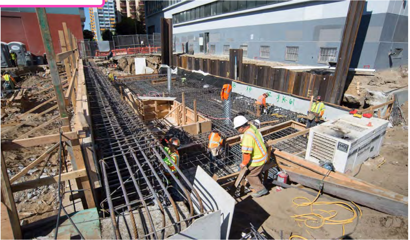
Rebar cages can be seen being constructed for the portion of the roof slab on Clementina Alley. Once concrete is poured, utilities will be installed, and this area will be backfilled.
