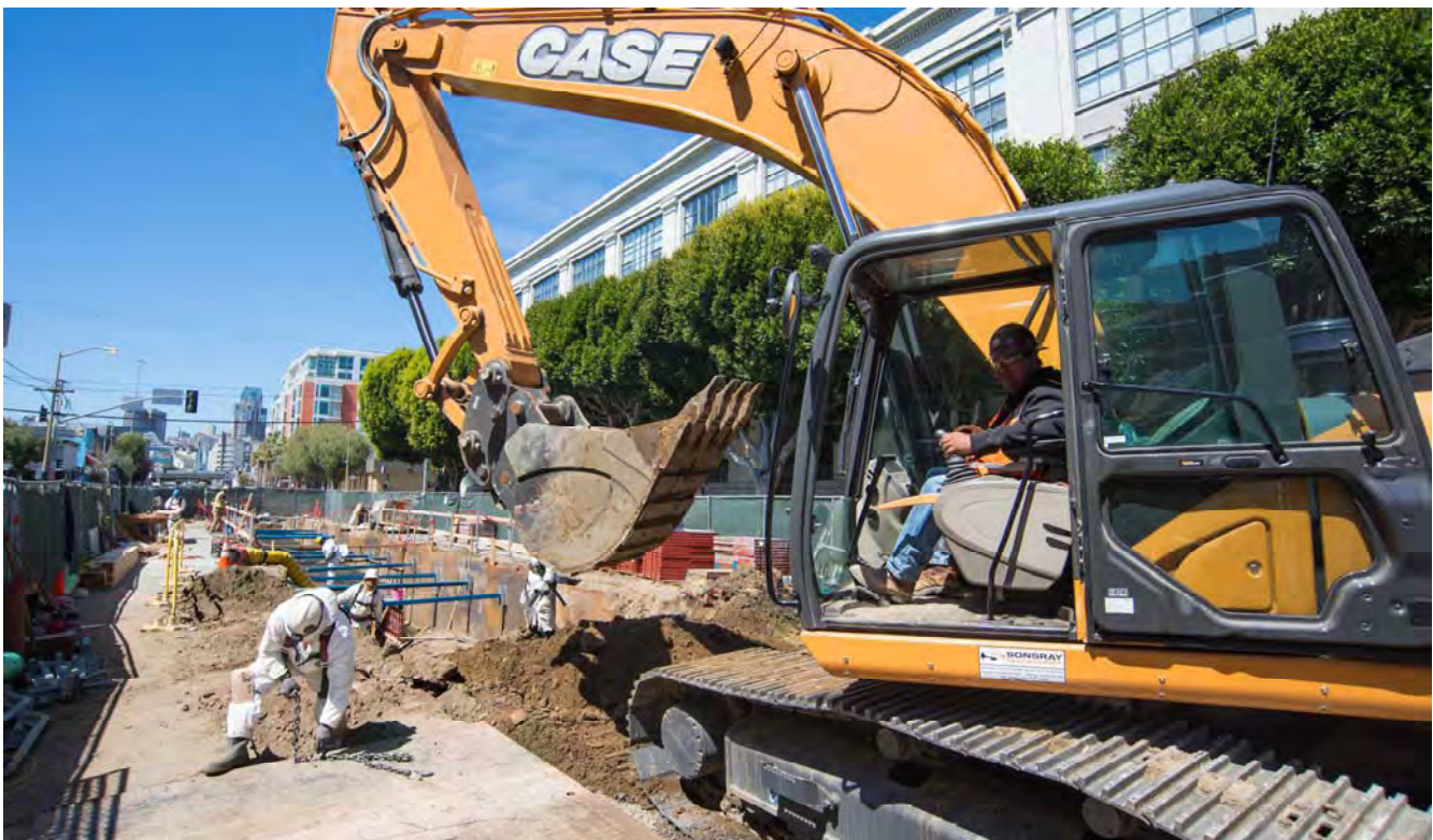
An excavator waits to remove material from the century-old brick sewer being reconstructed with a new reinforced concrete roof, on 4th south of Brannan.
