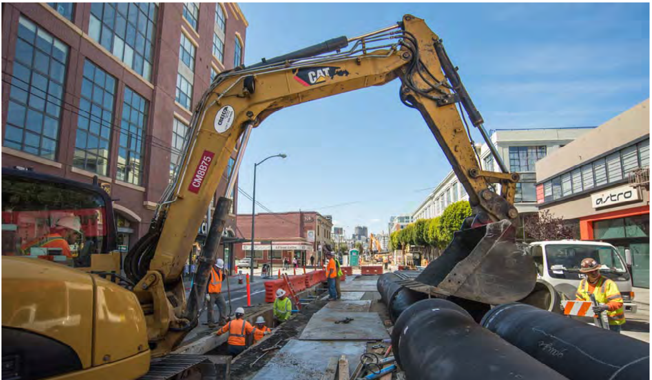
A mini excavator is used to lift pipe sections during utility work on 4th near Bluxome and Townsend.
