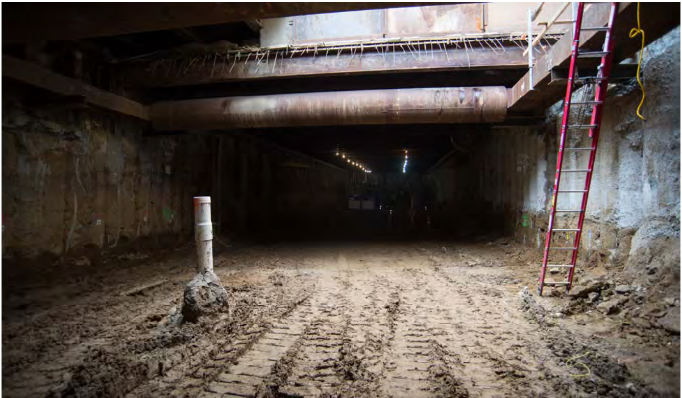
Light streams in from the access shaft on Stockton just north of Ellis. Ahead, the partially-excavated station concourse can be seen.
