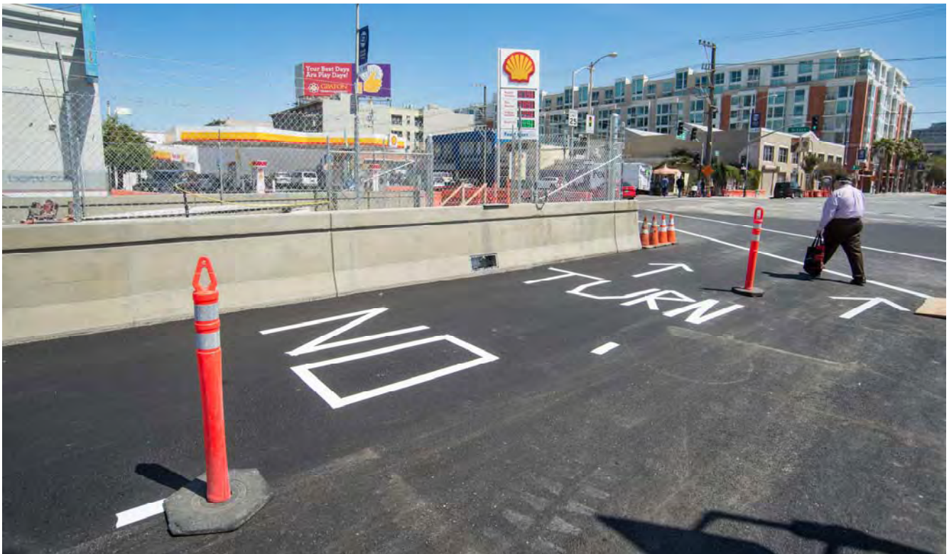
On the west side of the tunnel portal, two "through" lanes have been restored for traffic traveling south on 4th Street. No turns are allowed at this intersection.
