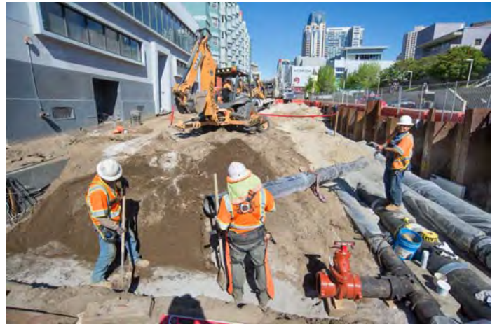
Workers install pipes for water and sewer lines at the intersection of Clementina and 4th Street.
