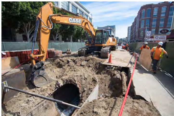
This century-old brick sewer is getting a new lease on life with a reinforced concrete roof, on 4th Street south of Brannan.
