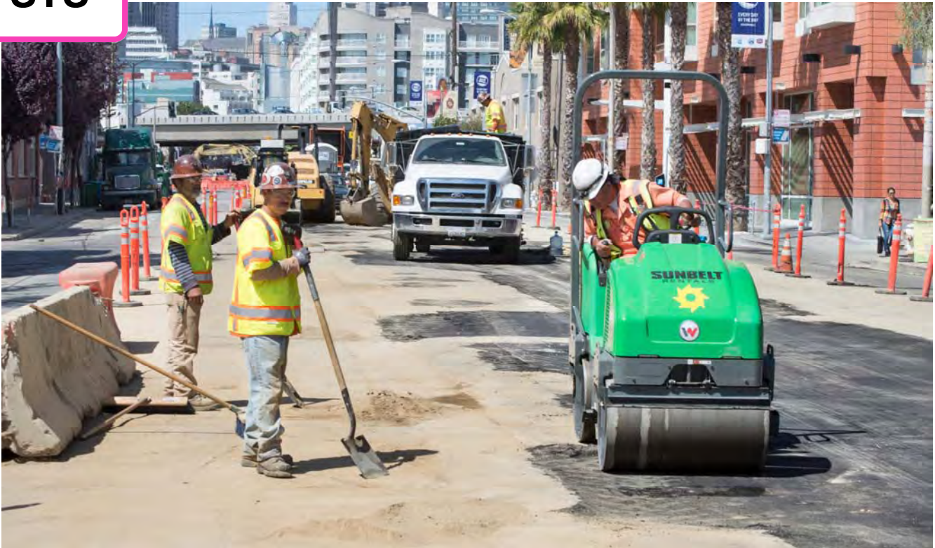
After foundation piles for the future 4th and Brannan surface station platform were installed, a worker runs a steamroller over fresh asphalt during street restoration efforts.
