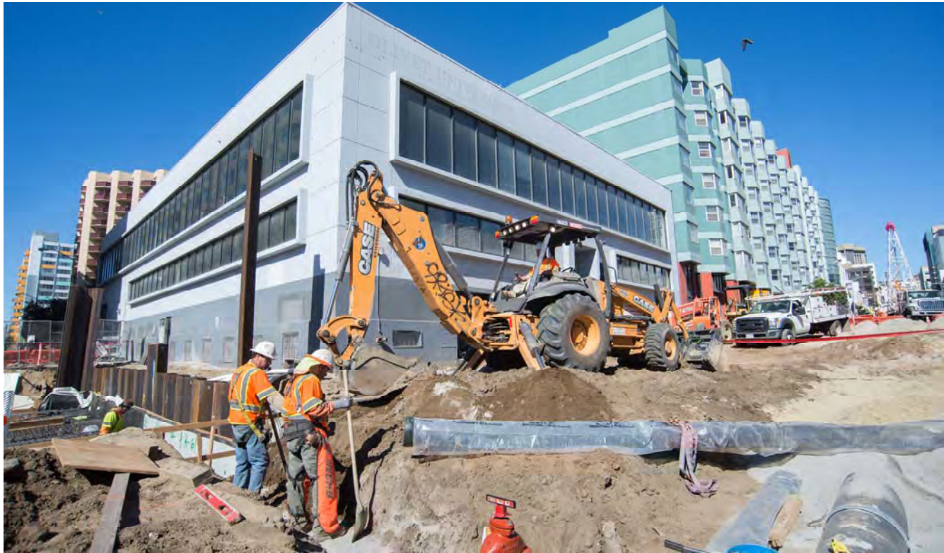
Workers install utility pipes and a valve. These pipes will carry water down Clementina Alley.
