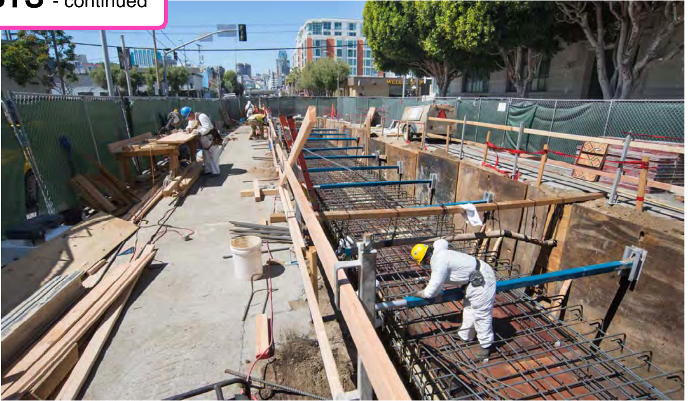
Workers install rebar and forms ahead of pouring concrete for the reconstructed 78-inch sewer just south of Brannan on 4th.
