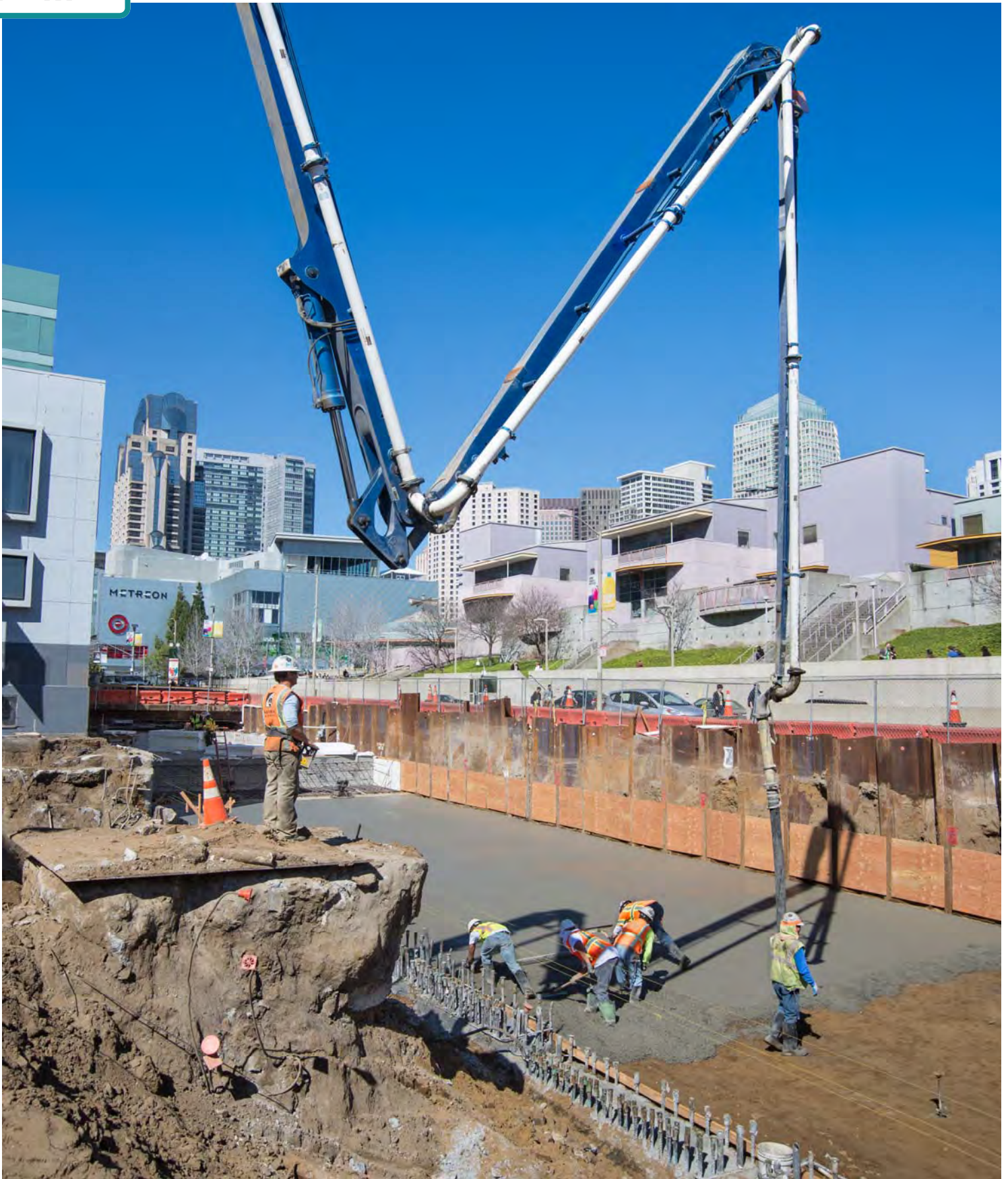
A worker stands with a remote control system, moving the arm of the concrete boom pump around the site for easy access.
