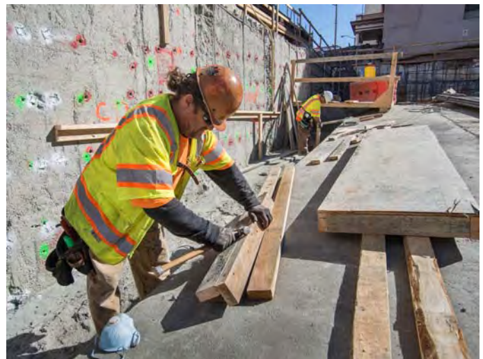
A carpenter works to construct concrete forms used to build the station roof slab.
