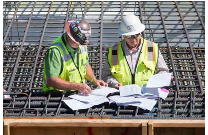
Workers review site drawings surrounded by a large rebar cage which will become part of the station roof.
