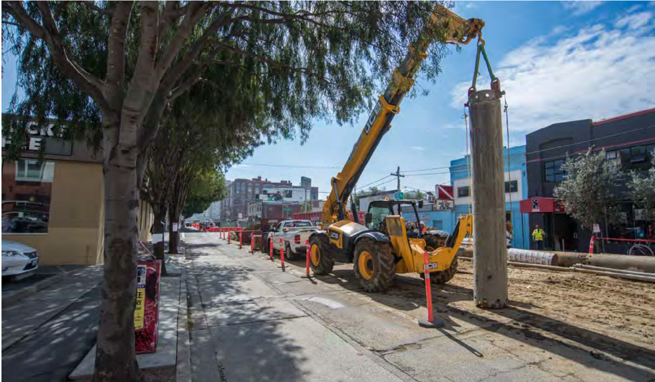
A telehandler lifts one of several steel pile casings used to construct foundation piles at the 4th and Brannan Station site.
