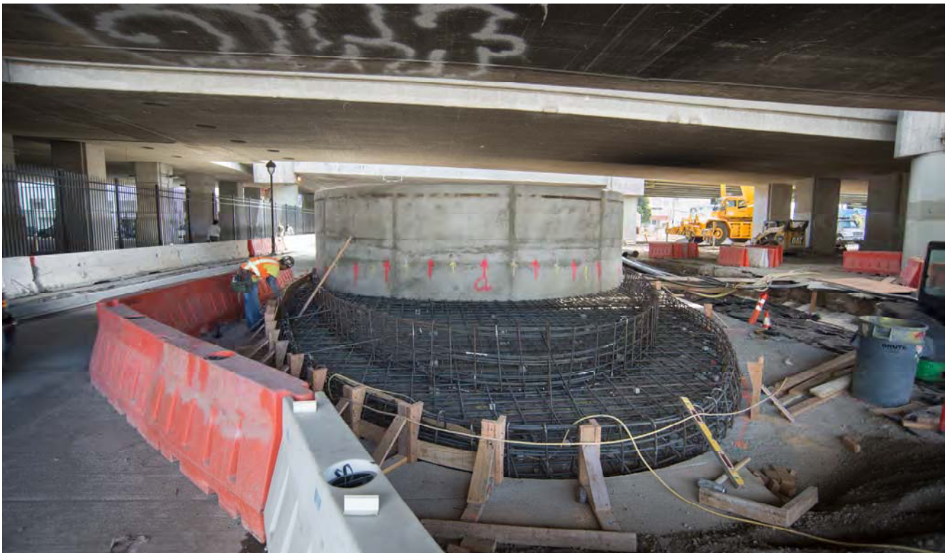
The barrier and curbs approaching the tunnel portal entrance can be seen here being constructed. Rebar is laid down, and concrete is poured creating a curved structure.
