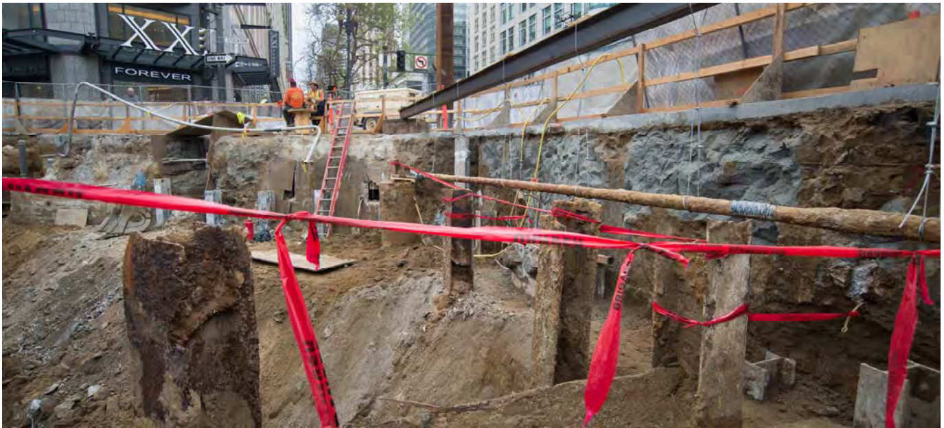
50-year-old steel I-beams have been uncovered at Ellis and Stockton. These beams were used to hold temporary shoring used in the original construction of the Powell BART/Muni Station and will be removed.
