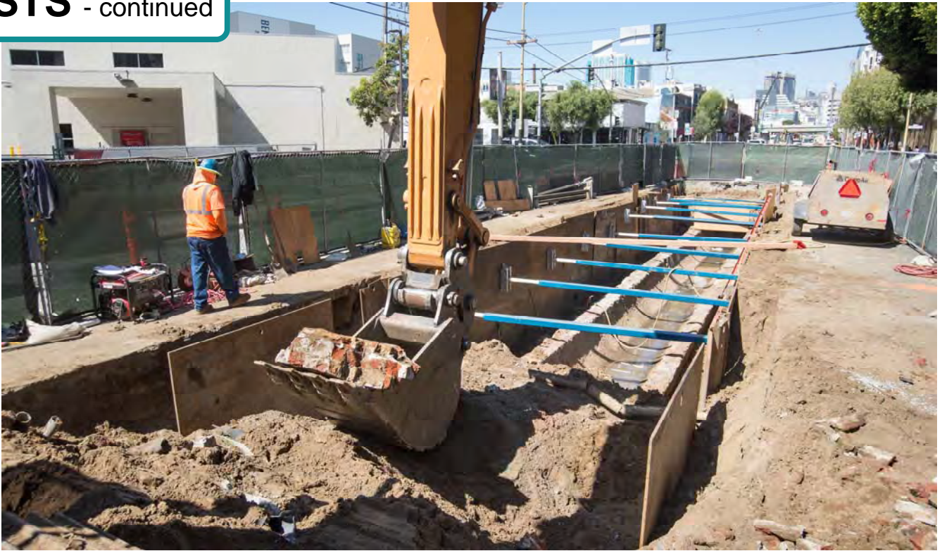
Before a road bed can be constructed for surface tracks south of Brannan, a century-old sewer is being uncovered and rebuilt with reinforced concrete.
