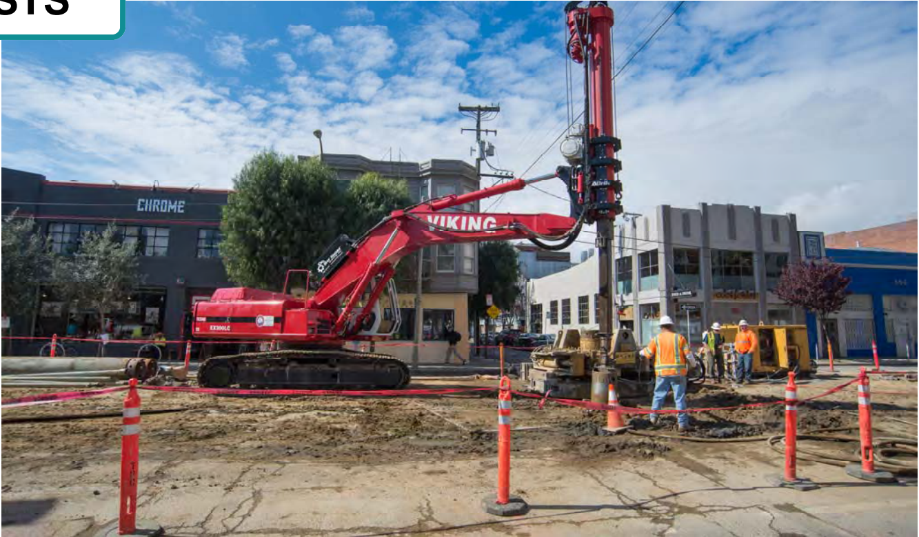
A rotary drill rig with greater vertical clearance was brought in to finish the last half dozen piles for the foundation of the 4th and Brannan Station platform.
