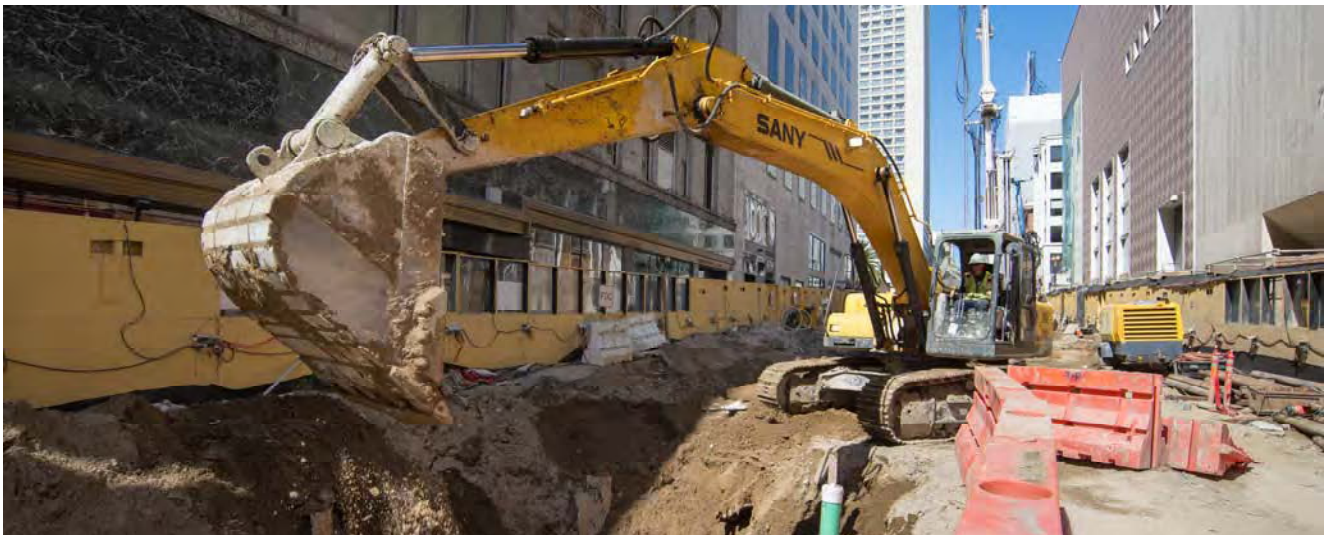
An excavator constructs a muck pit used in drilling operations north of O'Farrell.
