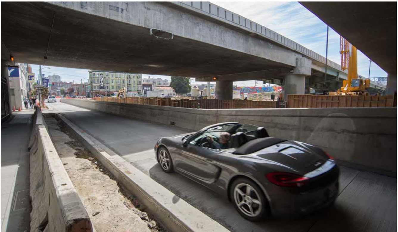
A finished concrete wall can be seen after traffic has been reopened along 4th Street between Harrison and Bryant.
