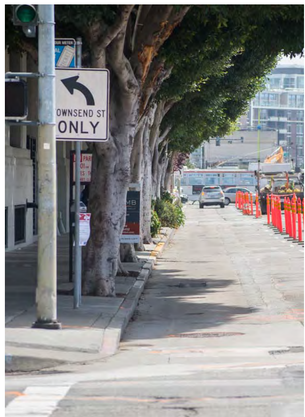
A single lane of traffic is open on both the east and west side of the street south of Bryant, surrounding sewer re-construction operations in the middle of the roadway.
