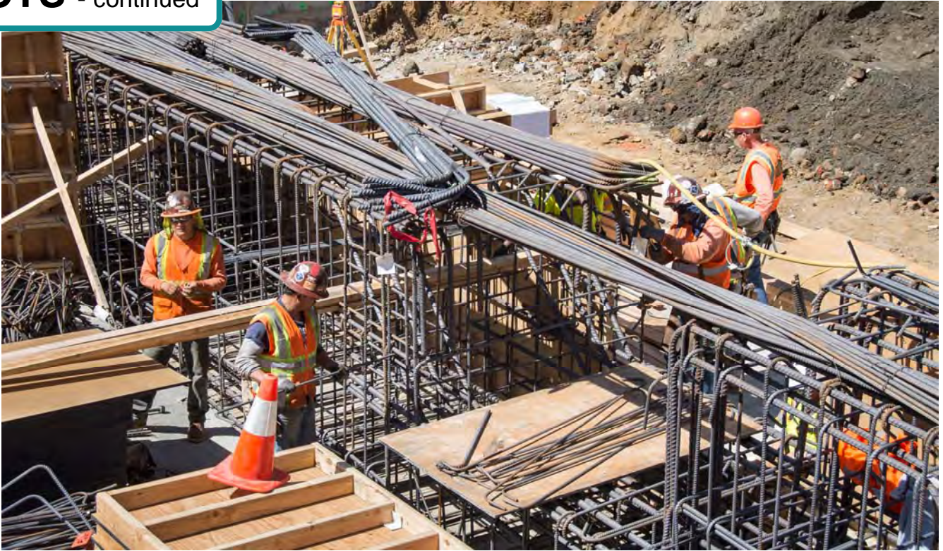
This large rebar cage will become a beam spanning the width of the site. Escalators will descend from this point, bringing customers to the station interior.
