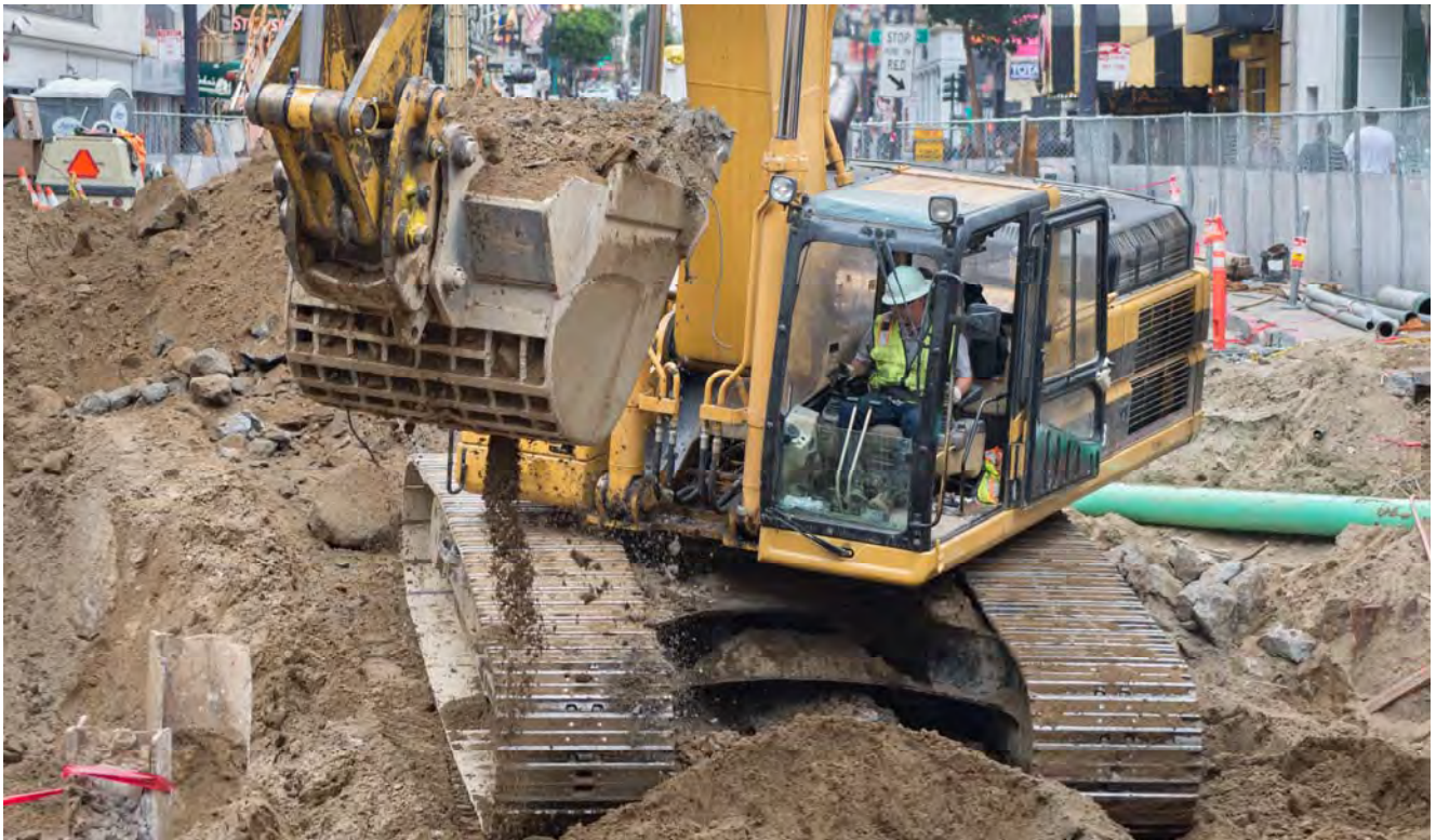
An excavator removes soil at the intersection of Ellis and Stockton. Here, workers will first excavate and then reconstruct the pedestrian passageway accessing Powell Station.
