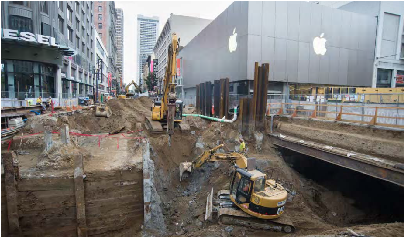
Work to excavate the Ellis Street entrance to Powell BART/Muni Station uncovered temporary shoring used to construct the original interior walls.
