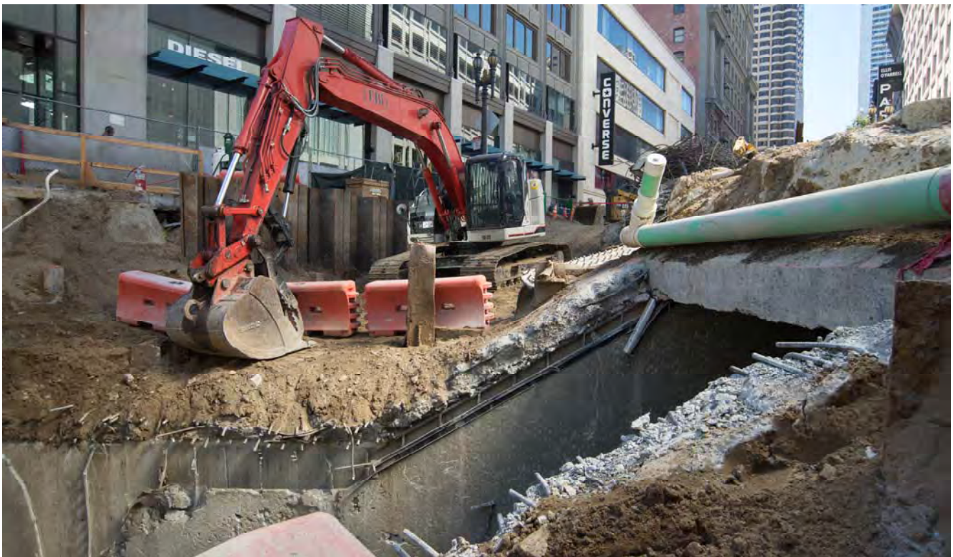
The slanted roof of the former escalator adjacent to the Apple Store can be seen here, recently removed ahead of further excavation and demolition work.
