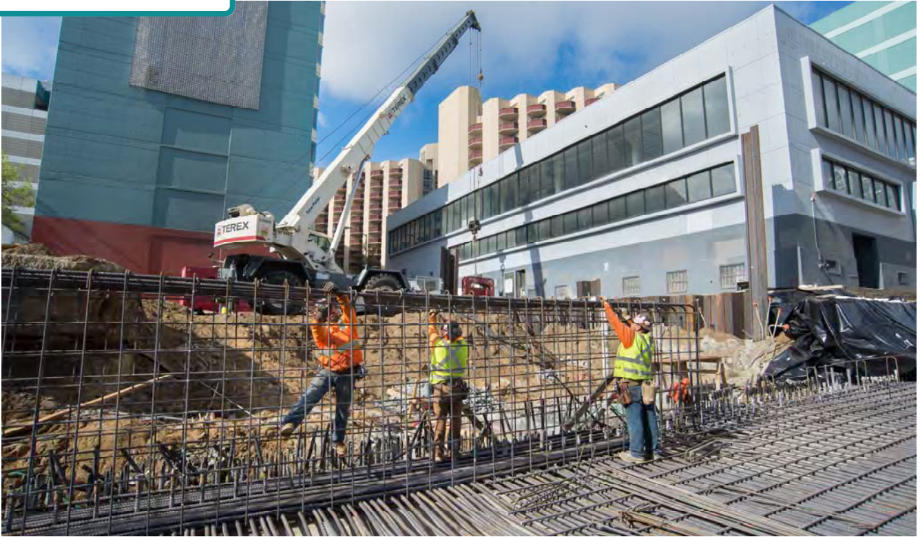
Workers begin installing rebar for a beam crossing the point separating the station head-house and the platform roof.
