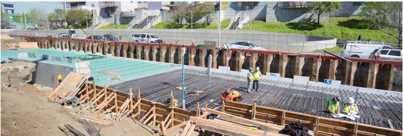
Rebar cages and waterproofing can be seen being installed for the final sections of the west roof slab at the Yerba Buena/Moscone Station site.
