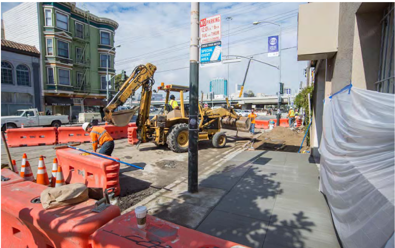
This sidewalk south of Bryant has now been restored, following the installation of a new AT&T duct bank.
