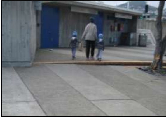
Figure 35: Lack of ADA curb ramp on South Geneva Transit Plaza between kiss-and-ride and stairs Photograph showing curb at the South Geneva Transit Plaza with no ADA curb ramp.
