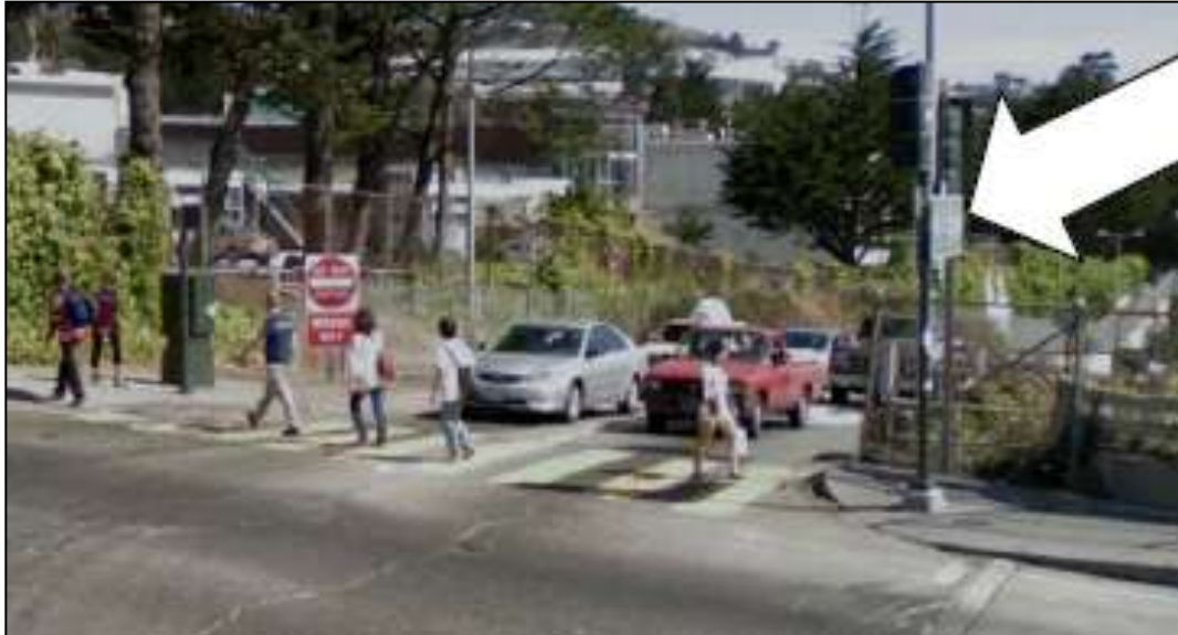
Figure 36: Traffic Signal Obstructing North Sidewalk Photograph shows the traffic signal is in the middle of the sidewalk, not leaving enough clearance for pedestrians.
