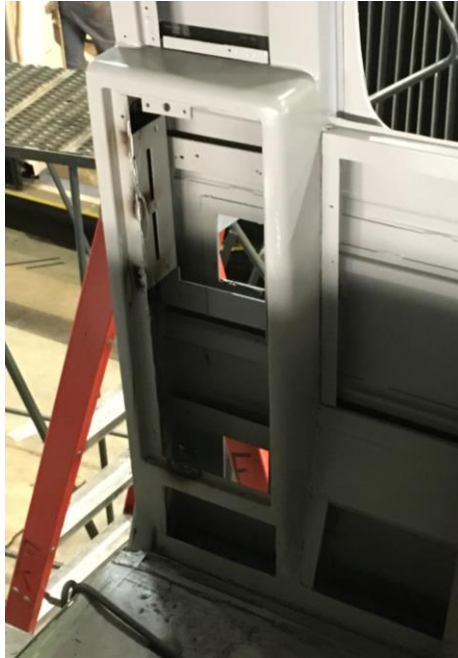
Figure 33 – New Resistor Compartment
