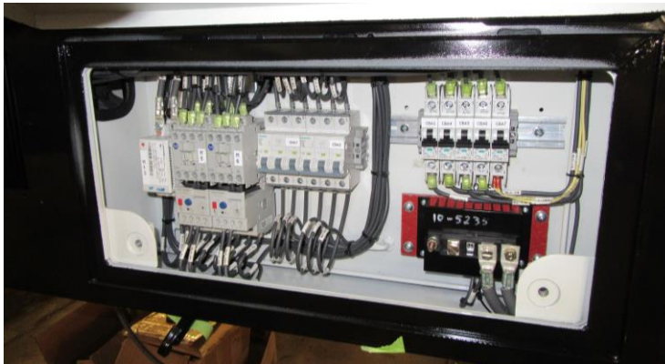
Figure 13 – LVPS Access Panel
