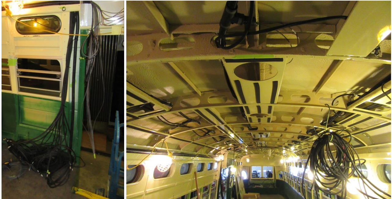
Figure 7 – Interior Wiring View
