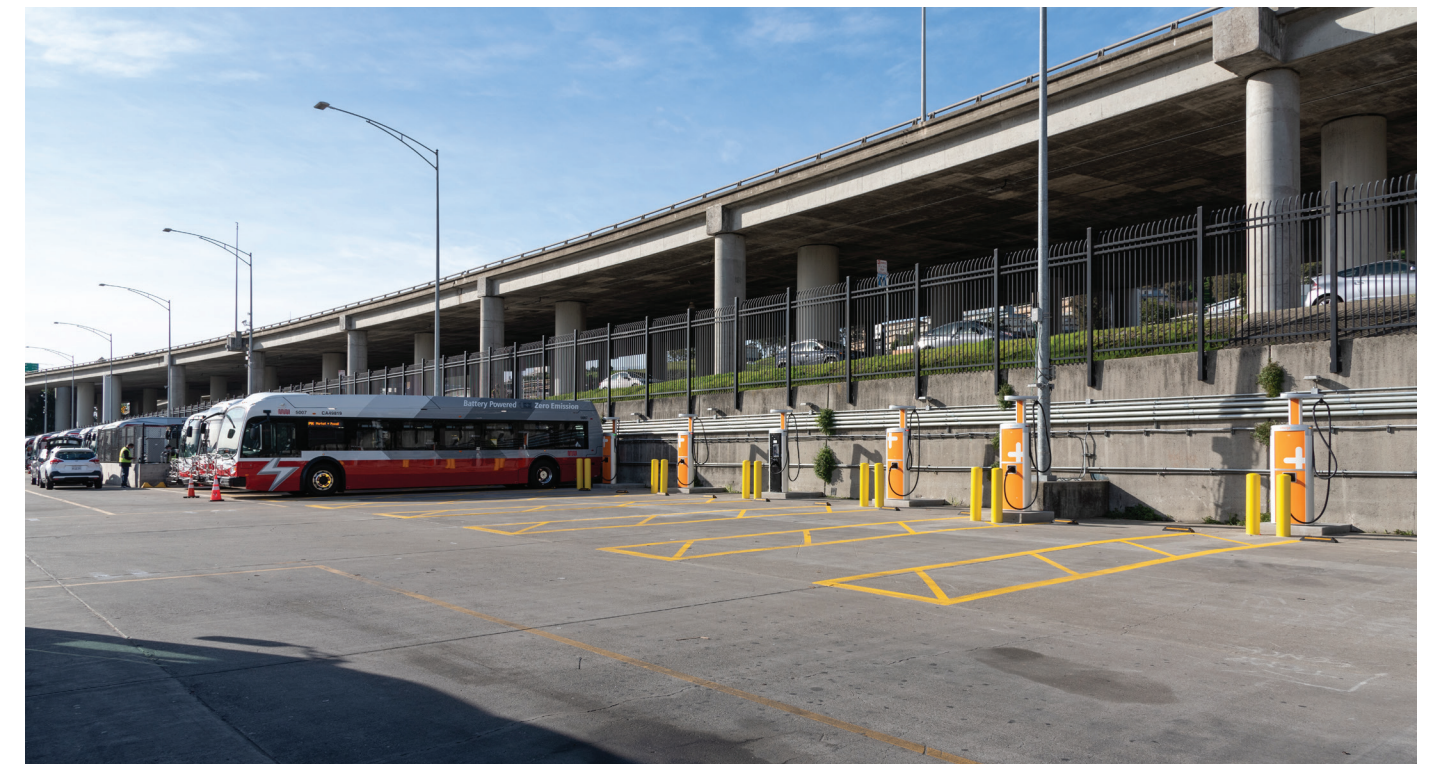
Figure 8-3: Charging Station at Woods Facility
