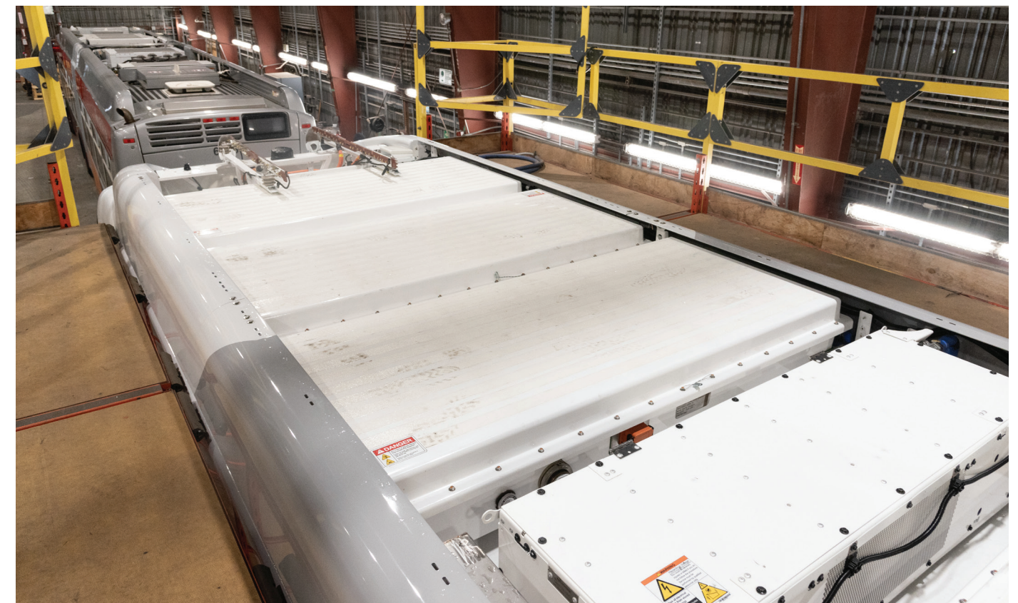
Figure 1-2: Rooftop Battery Units on the SFMTA's First Battery Electric Bus (New Flyer 5001)
