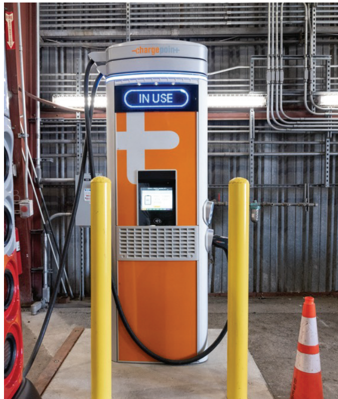
Figure 6-5: Charging Station at Marin Facility
