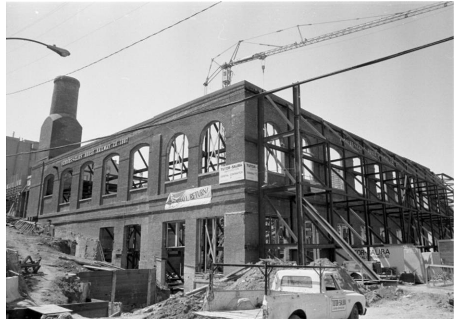
Reconstruction Work at the Cable Car Barn, August 7, 1983 SFMTA Photo Archives 830807B_04.jpg
