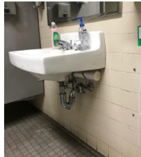
Non-compliant lavatory (Women 106).
