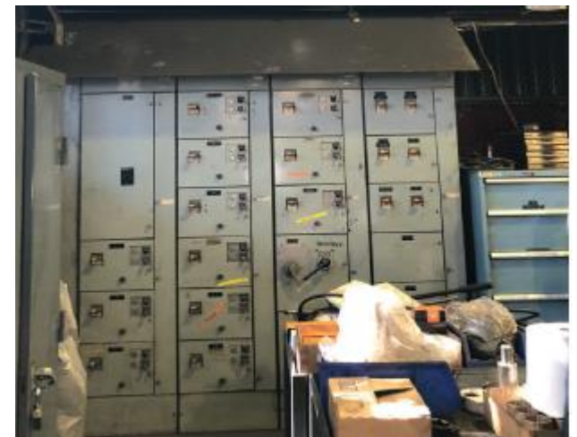
Motor Control Center (MCC)
