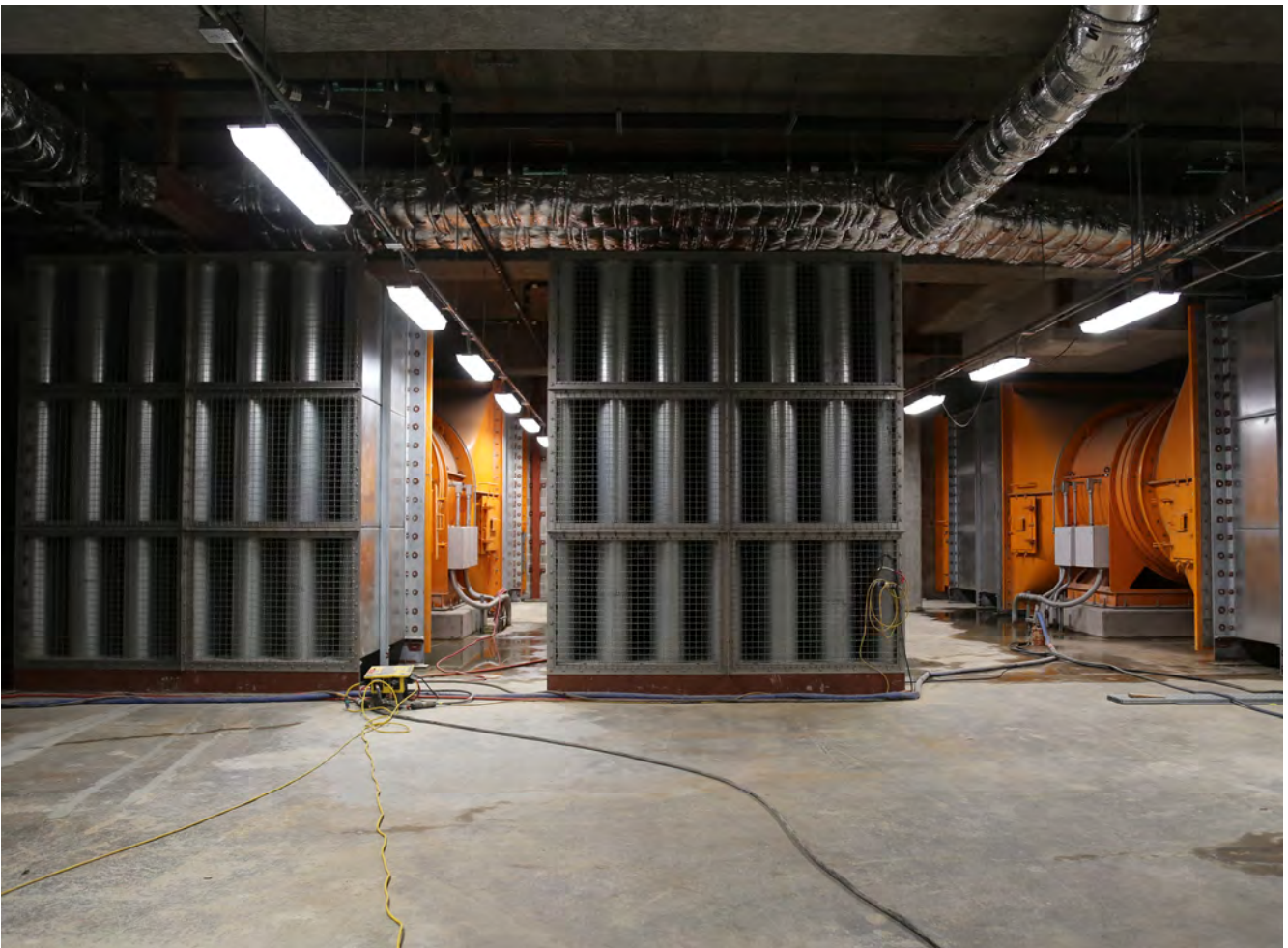
Ev exhaust fans in CTS
