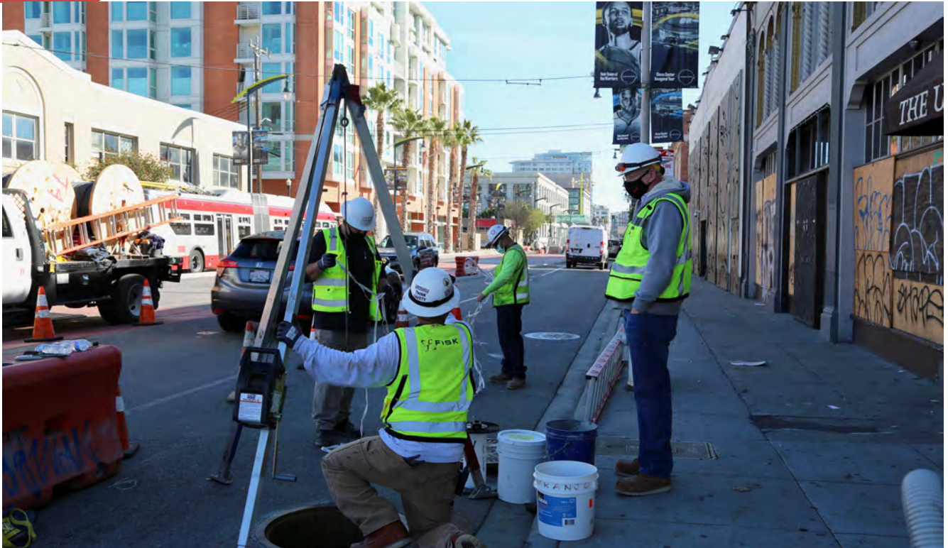
Crew performing street work for the surface station at 4th and Brannon
