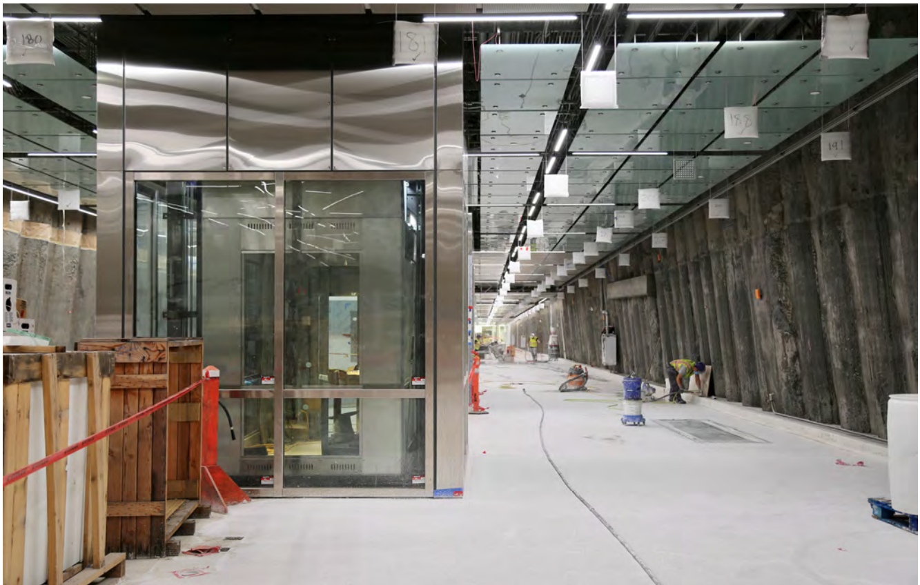
Workers finishing the floor on the Concourse Level of Union Square Station
