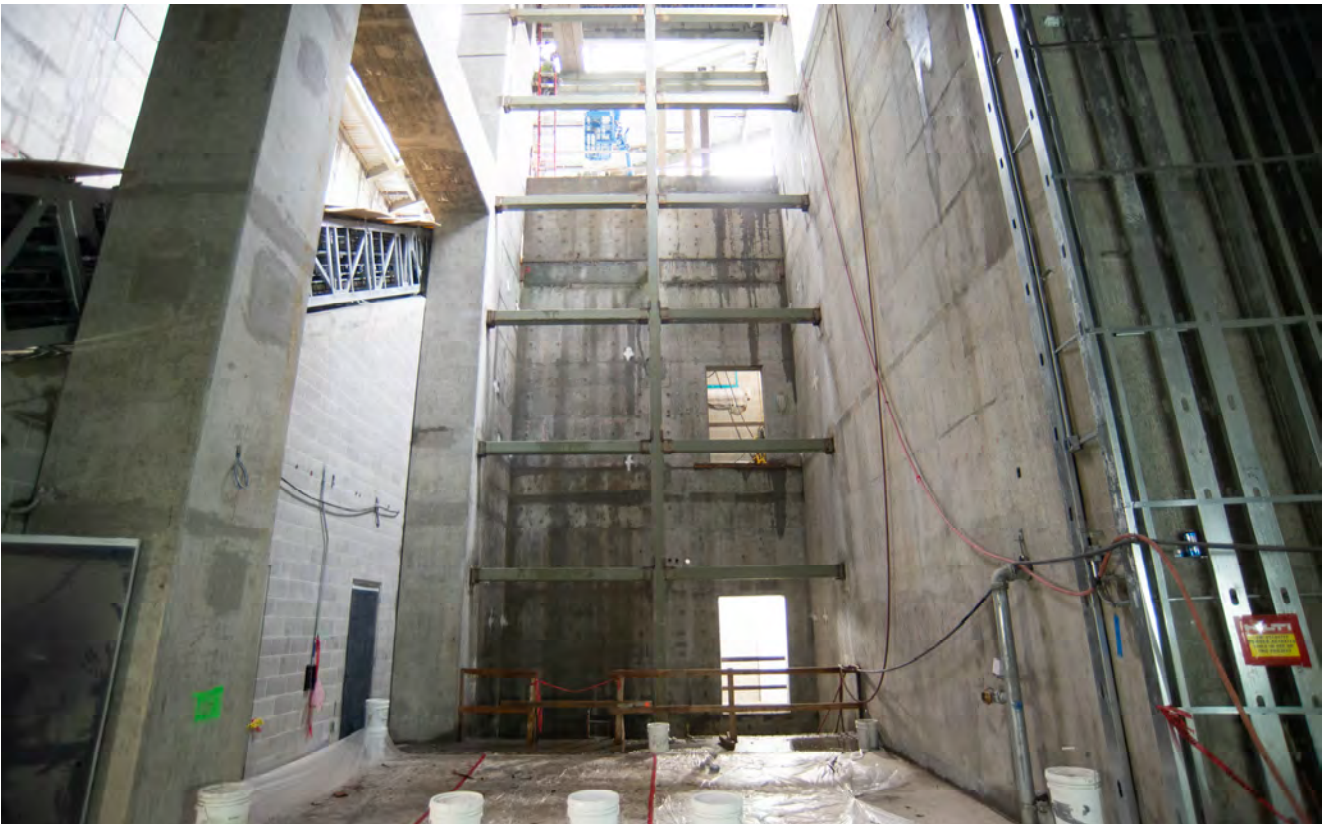
Steel framing has been installed as part of initial elevator installation work between the street level station entrance structure and the concourse lobby for Yerba Buena/Moscone Station.
