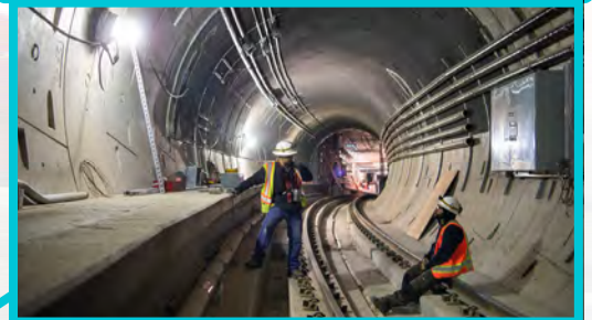
4th St. Surface Track, Systems (STS)
