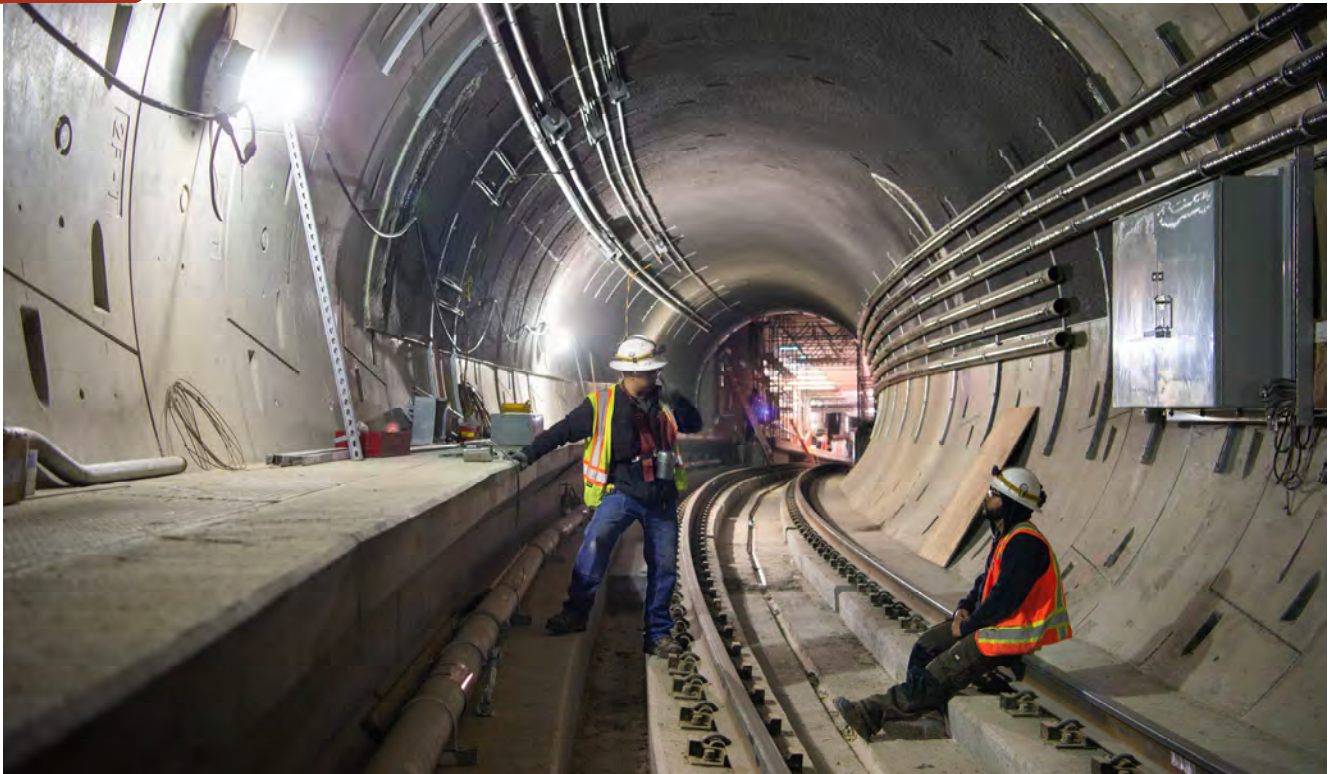
Workers continue installing conduits for lighting and electrical systems inside the twin tunnels, seen here inside the northbound tunnel as it approaches Union Square/Market Street Station.
