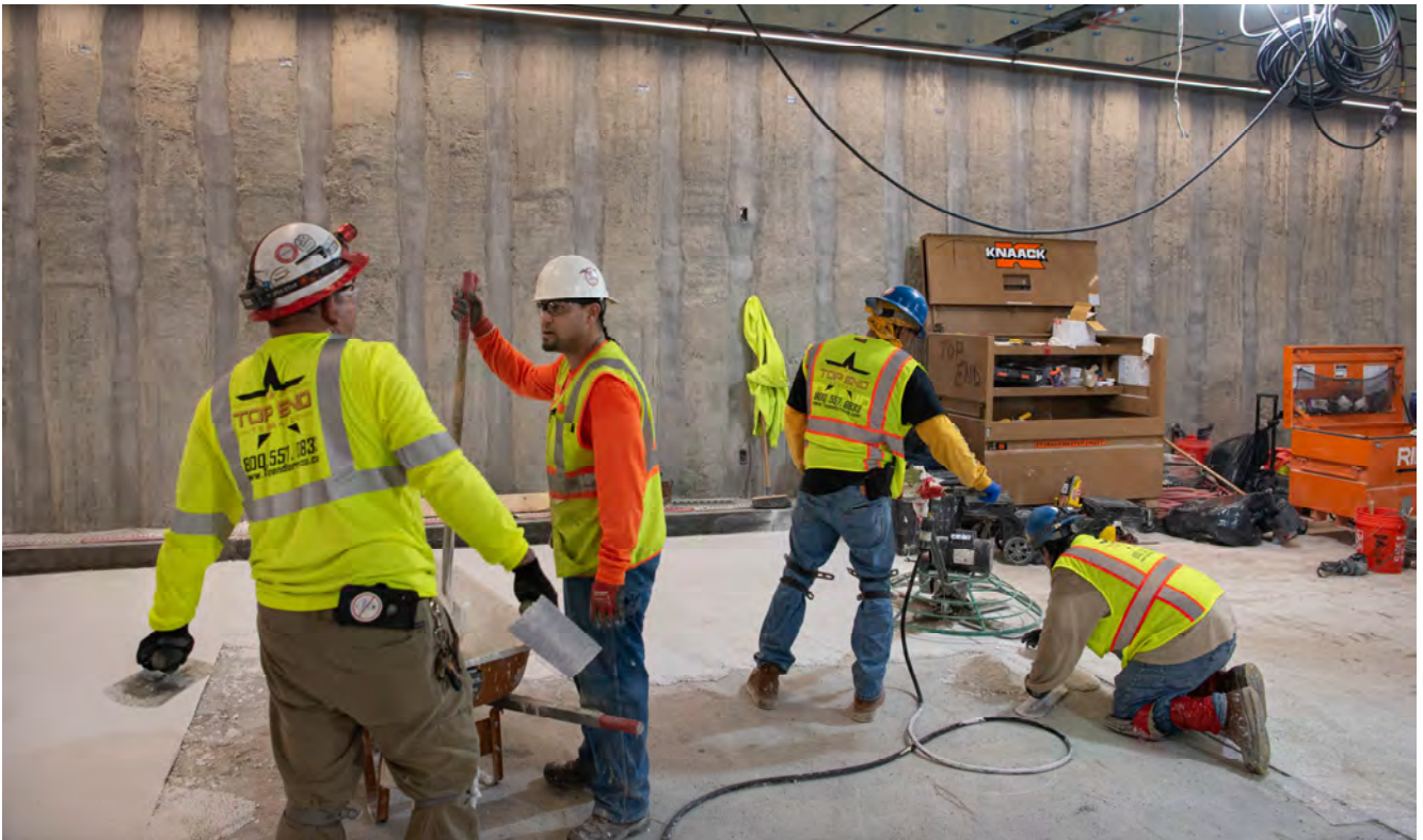
A crew mixes and pours sections of terrazzo floor coating on the east side of the south concourse for Union Square/Market Street Station.
