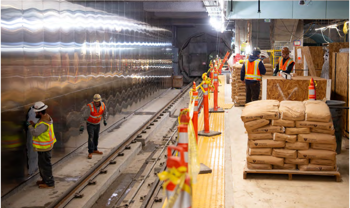
Workers remove sheets of protective plastic coating from stainless steel wall panels on the platform level for Yerba Buena/Moscone Station.
