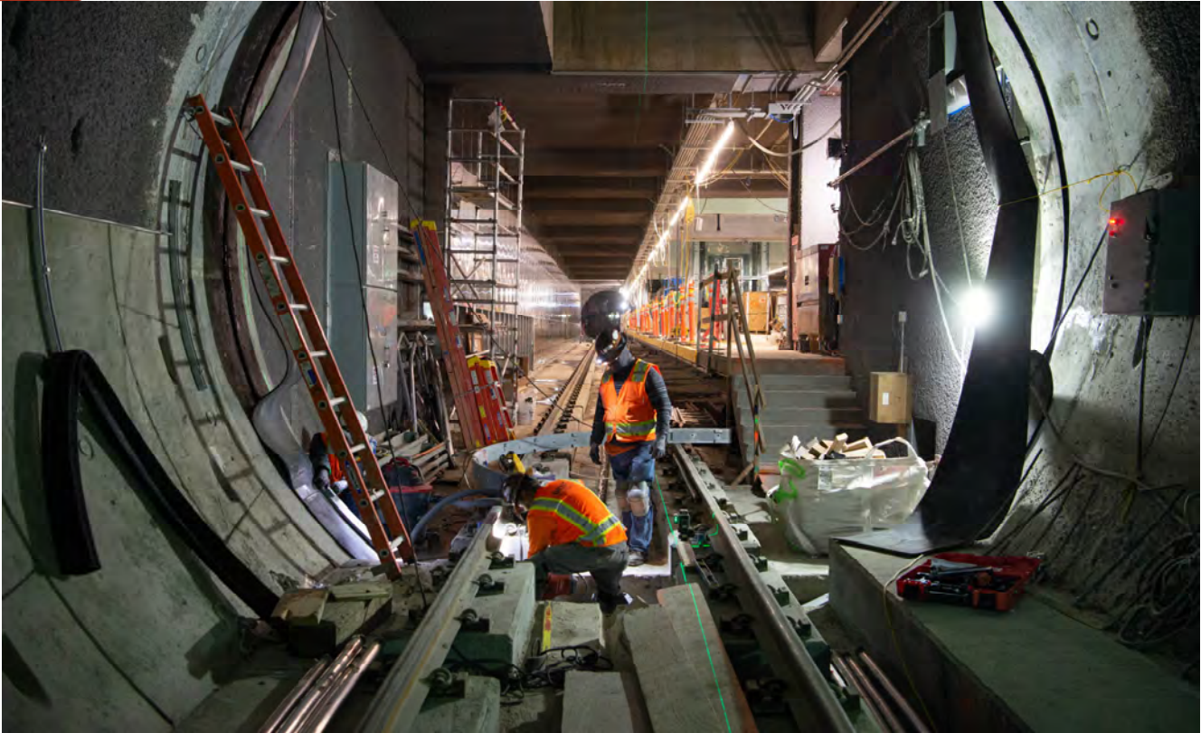
A transition joint between the northbound track side of Yerba Buena/Moscone Station and its entrance back into the northbound tunnel continues to be built.
