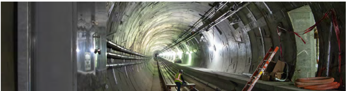
A worker rolls by cross-passage 5 on a small rail cart, traveling southbound inside the northbound tunnel near where workers have been installing lighting and electrical systems.
