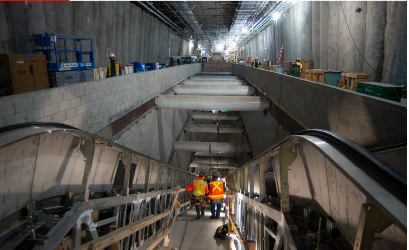
Dual escalators and a center staircase descend from the concourse level to the platform of Union Square/Market Street Station as the station interior continues to be built out.
