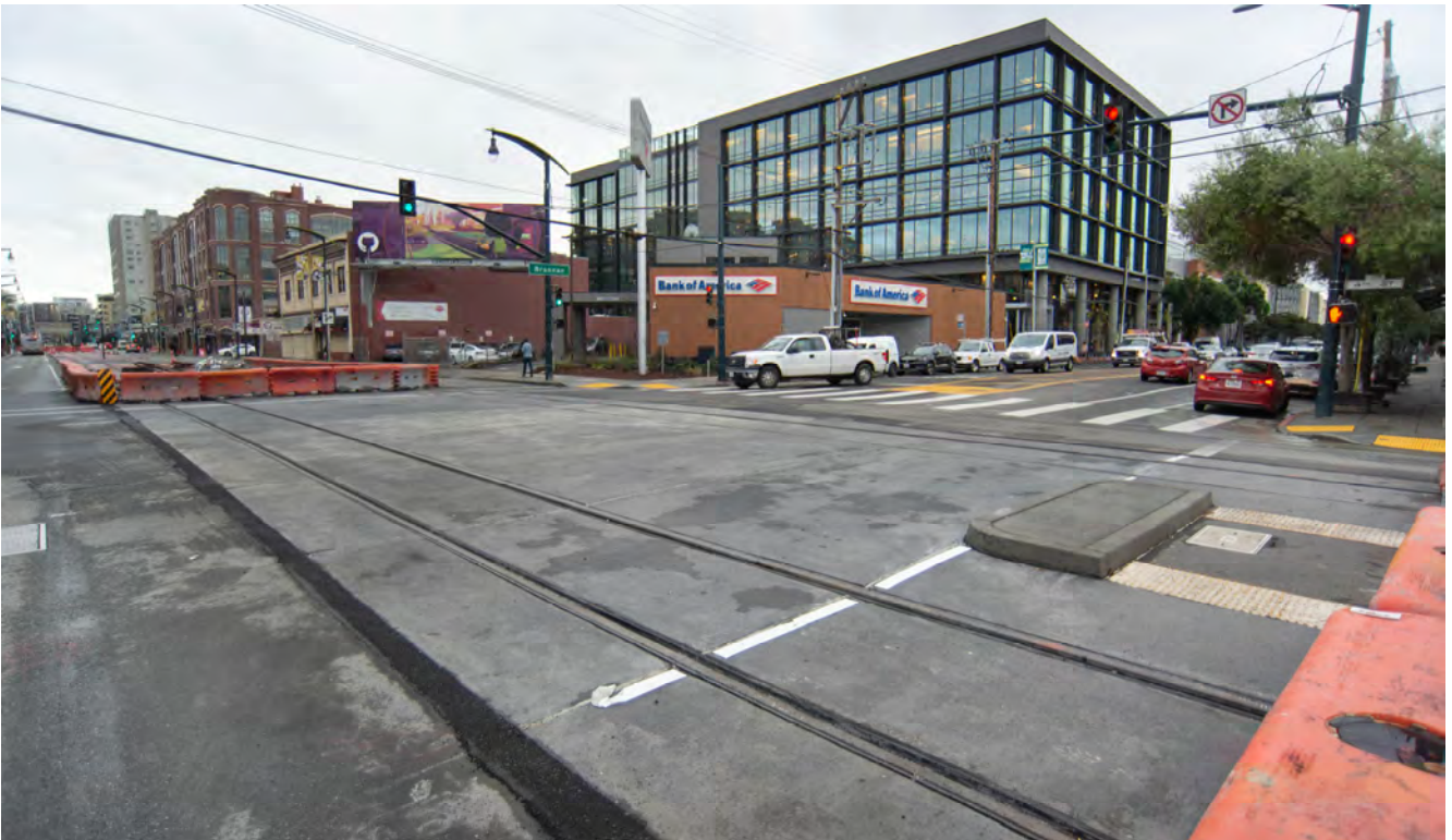
Tracks and the surrounding concrete rail bed have been installed across the 4th and Brannan intersection.
