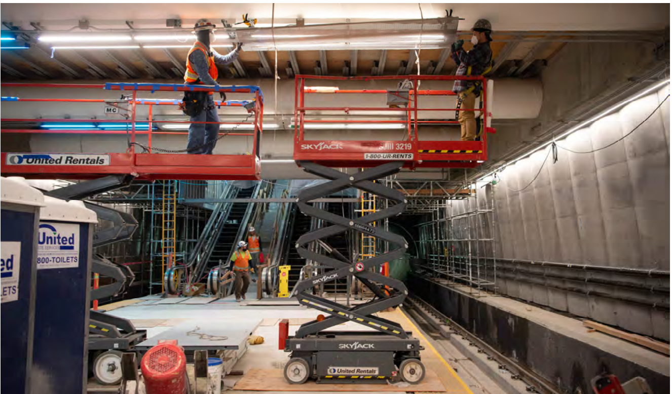
Workers install lighting covers near the south end of the Union Square/Market Street Station platform.
