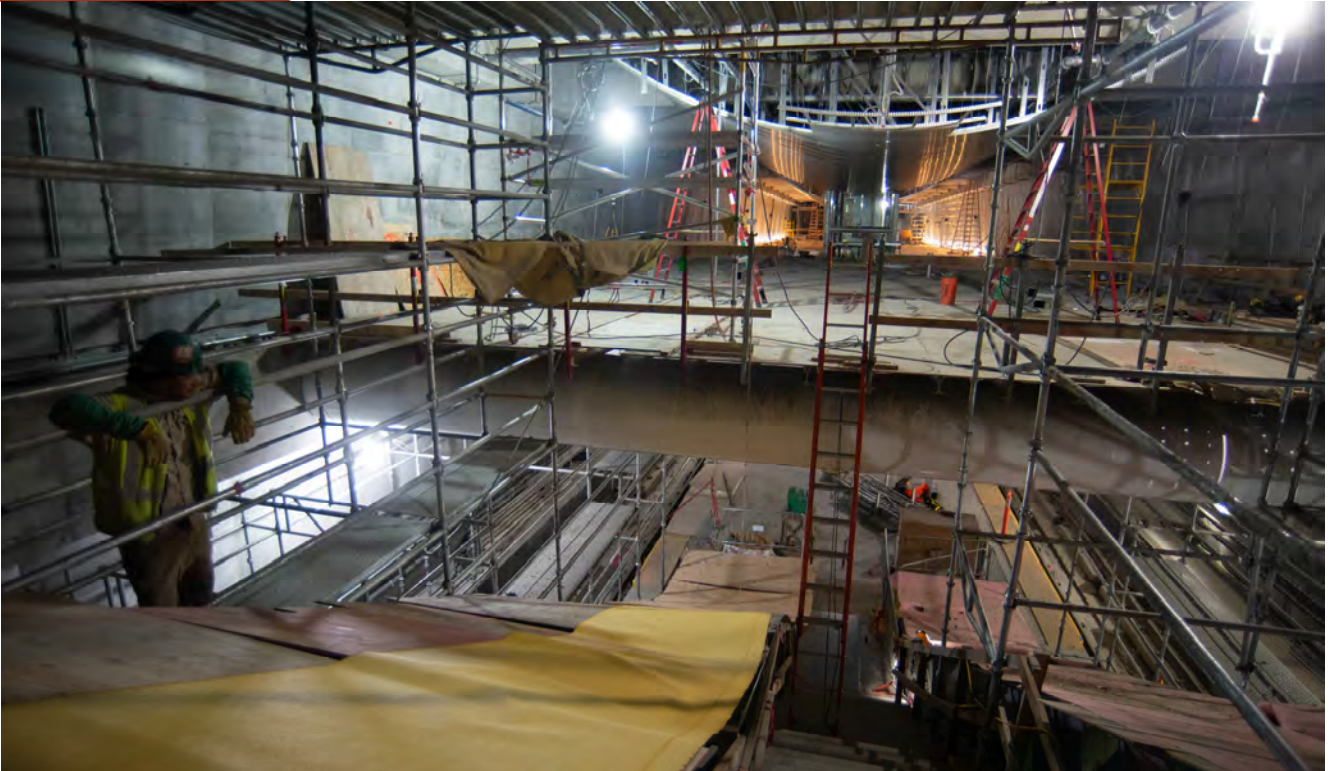
A curved decorative design element suspended above the platform level for Union Square/Market Street Station is coming together piece by piece.
