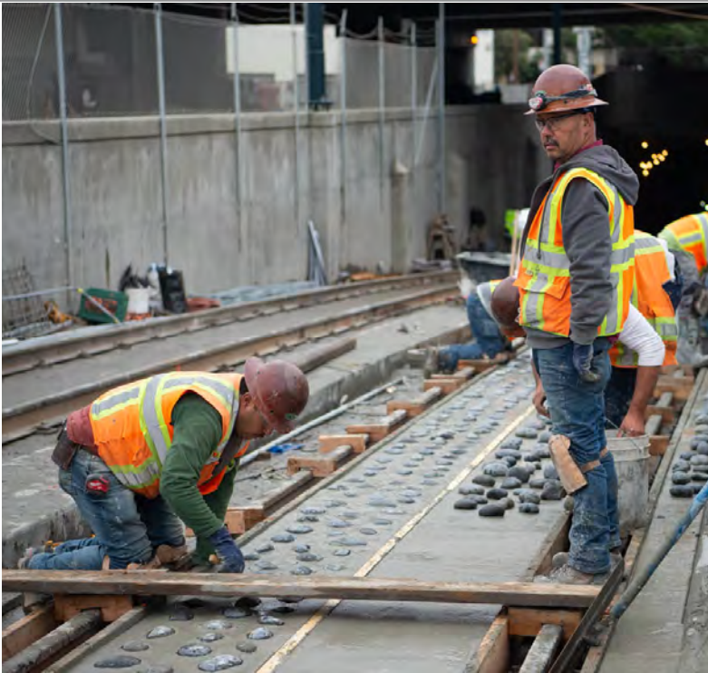
Workers pour and level concrete in sections between the rails and place river rocks into the wet concrete.
