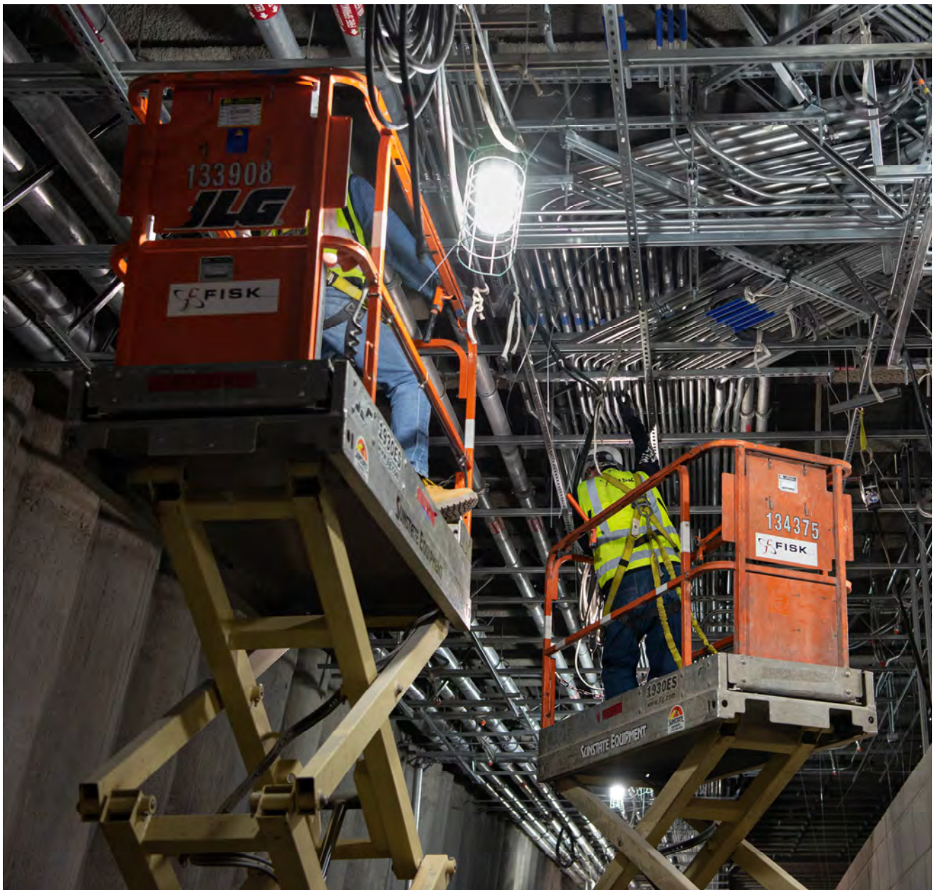
Multiple layers of dense conduits fly past one another above the future drop ceiling inside the Union Square/Market Street Station concourse.
