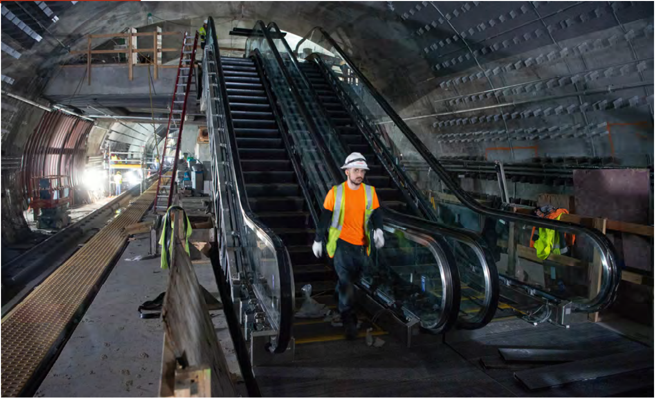
Escalators from the concourse leading down to the station platform level continue to be assembled.
