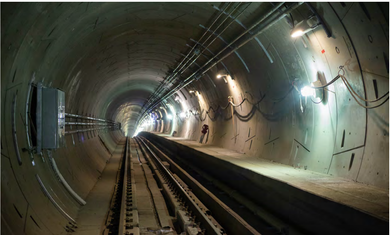
New permanent LED lighting has been installed inside the northbound tunnel, as seen operating adjacent to temporary lighting, just south of the Chinatown track crossover cavern.
