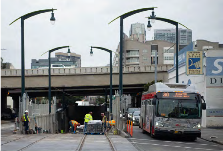
The site is cleaned, and concrete and river rock are brought in.
