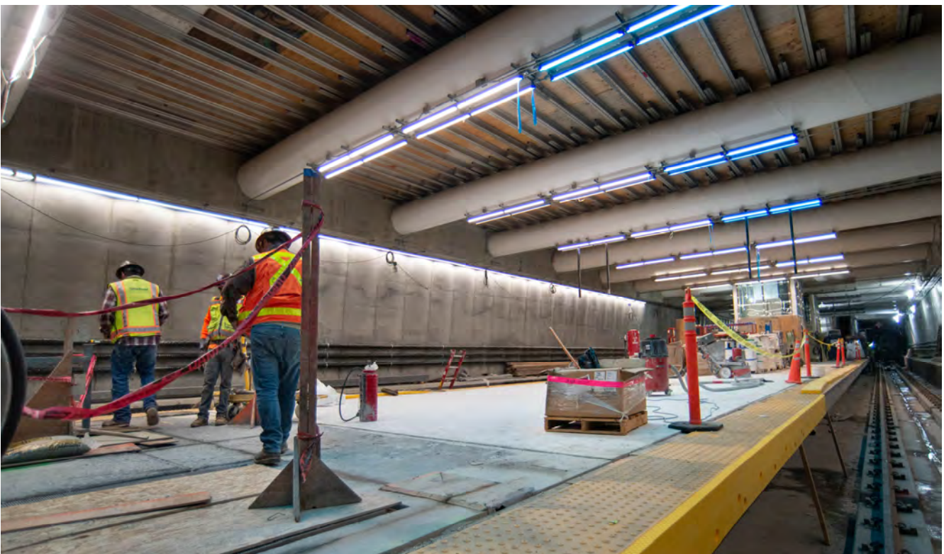
Permanent lighting has been installed across struts above the platform area for Union Square/Market Street Station.
