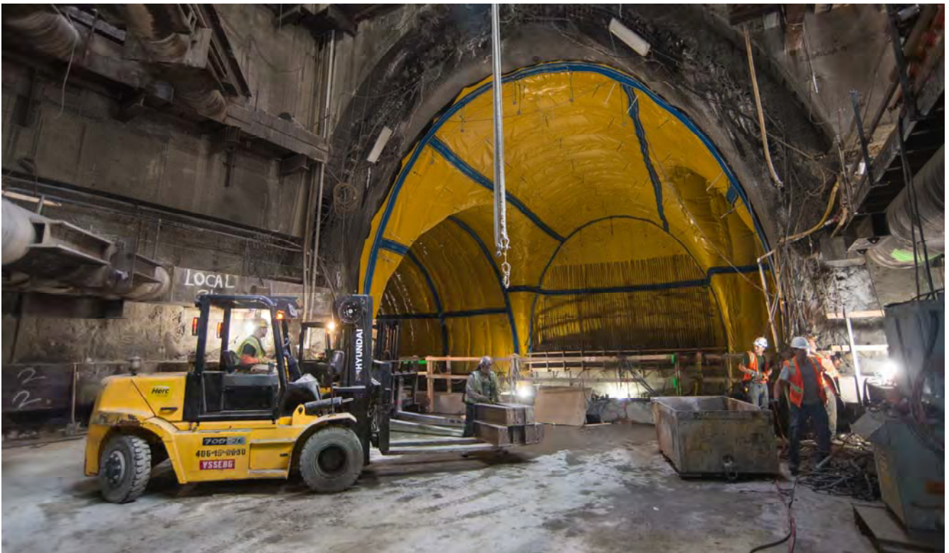
A forklift positions steel brackets into place for removal below an access shaft inside the Chinatown Station headhouse, at the entrance to the cross-cut cavern.
