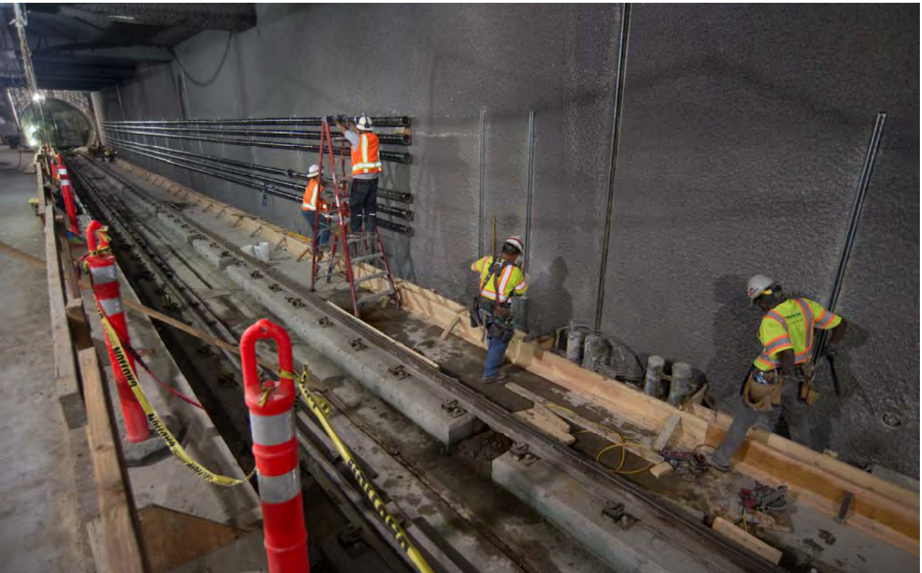
Workers install steel pipe along the east wall of the Yerba Buena/Moscone Station's platform level, which will be used for future utilities and systems.
