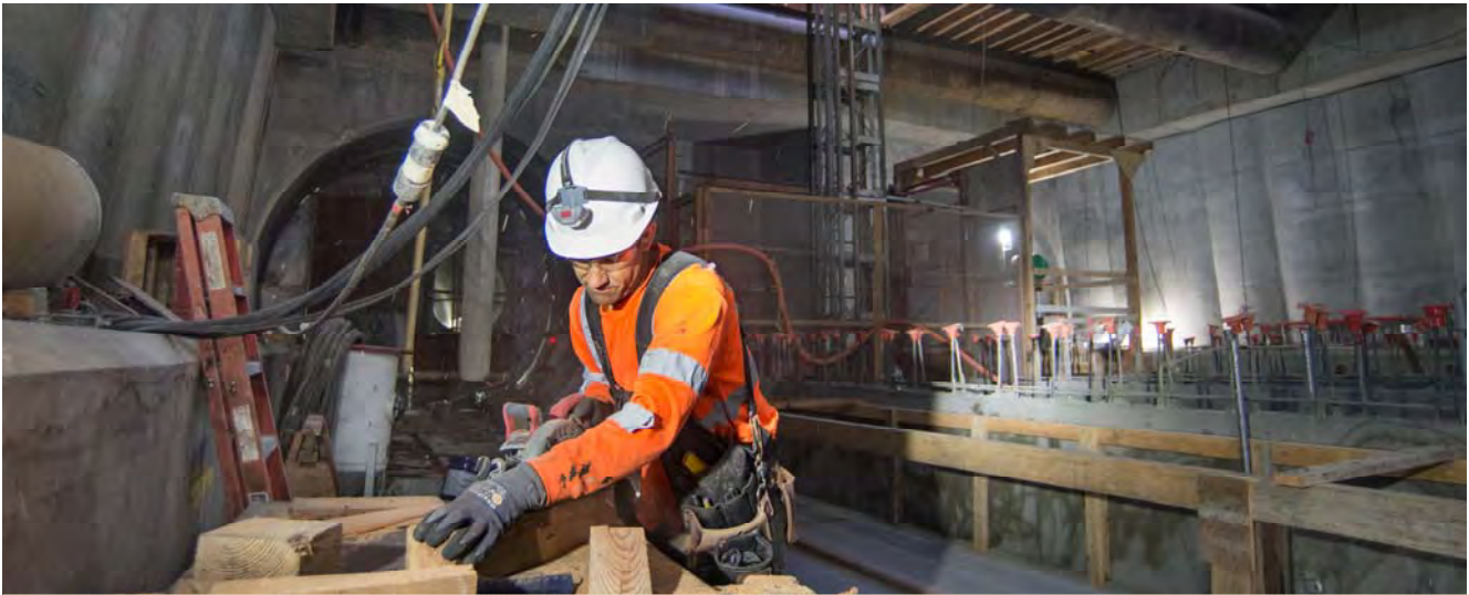
Carpenters build formwork for the northernmost slab overhang of the Union Square/Market Street Station platform.
