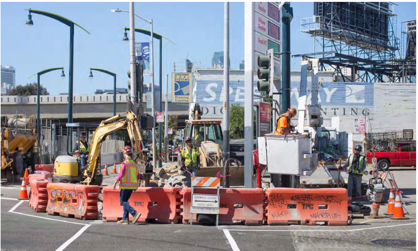
Multiple teams conduct operations inside the work area at 4th and Bryant, where sidewalk and roadway restoration efforts are underway.
