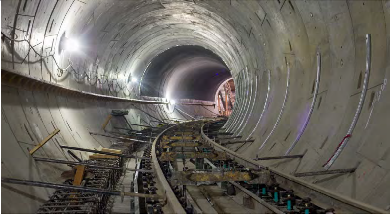
Rail is now being installed inside the S-curve for the northbound track, as it approaches Union Square/Market Street Station.
