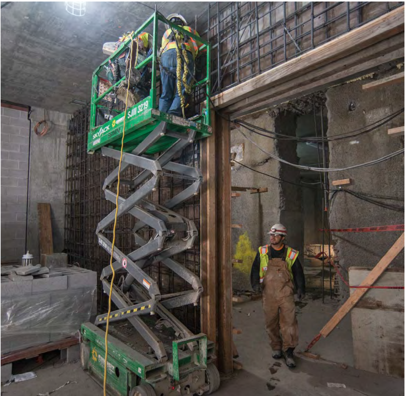
The rebar cage for a future reinforced concrete internal wall is assembled on the mezzanine level of the Yerba Buena/Moscone Station headhouse.
