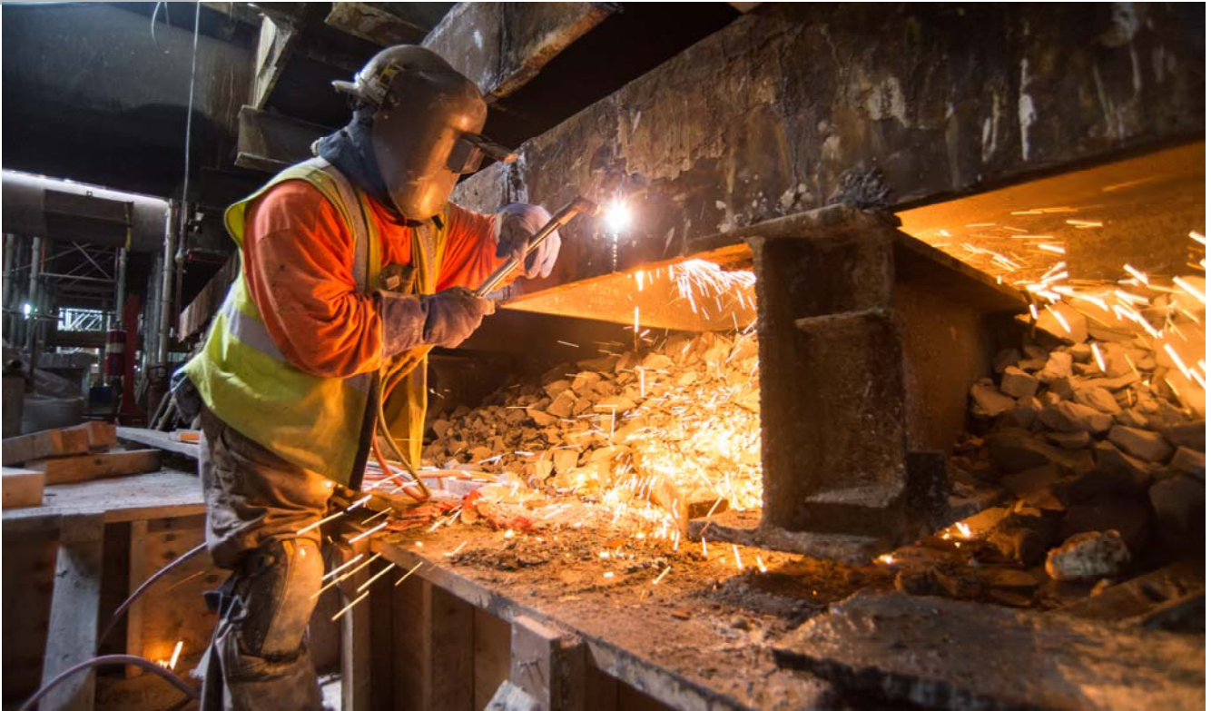
A worker cuts apart massive steel I-beams called walers used as part of temporary reinforcing inside the Chinatown Station headhouse. With internal floor slabs going in, some elements of temporary bracing are no longer needed.
