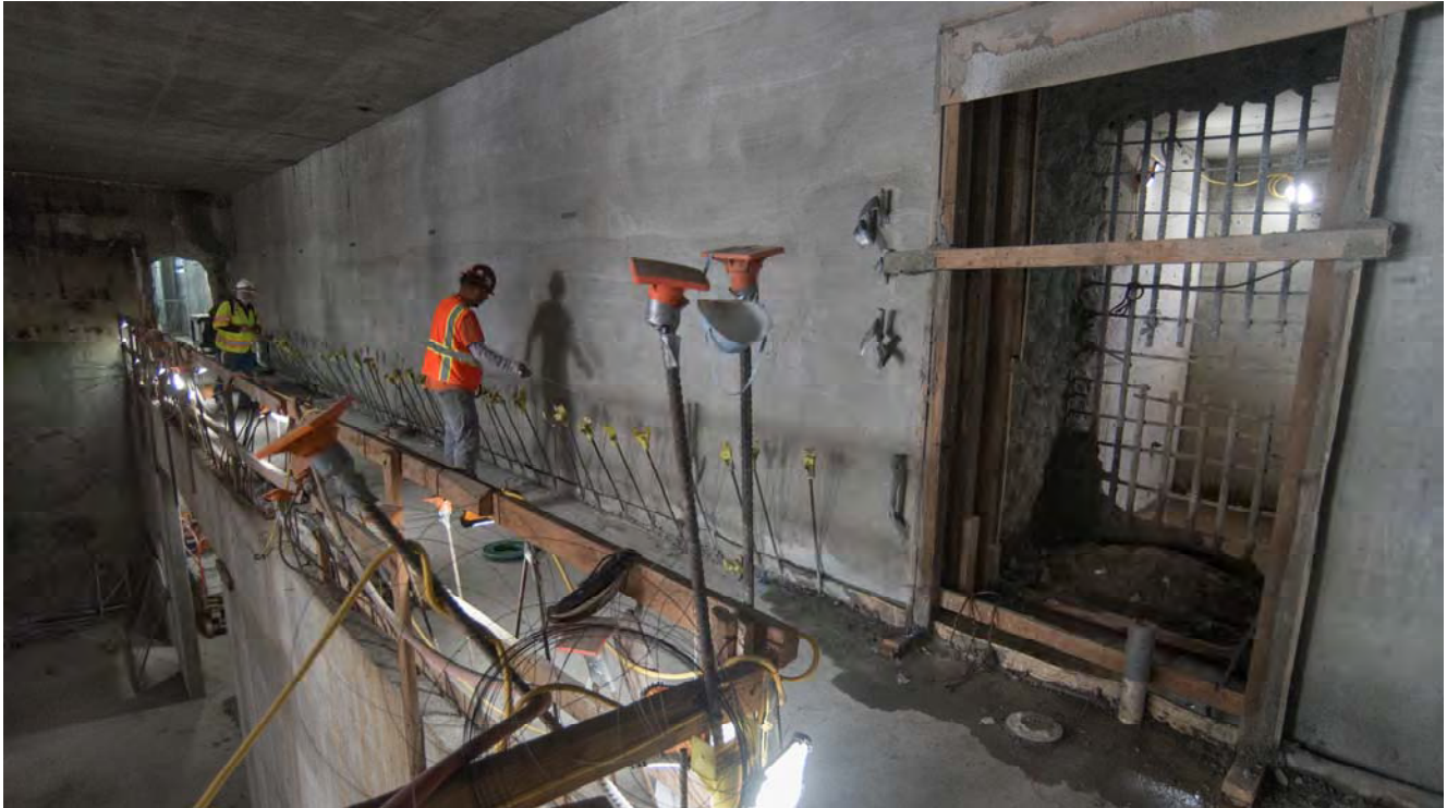
A worker checks a snap line along the south wall of the Yerba Buena/Moscone Station headhouse near where a hole is being made through the slurry wall to tie into an emergency exit staircase.
