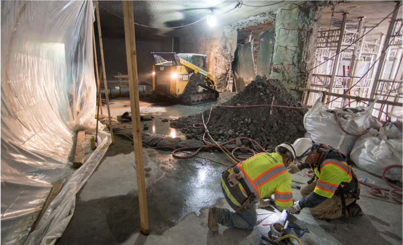
A bobcat fitted with a jackhammer removes excess concrete from the slurry wall dividing the mezzanine level of the station box and the headhouse, while workers maintenance a handheld jackhammer nearby.
