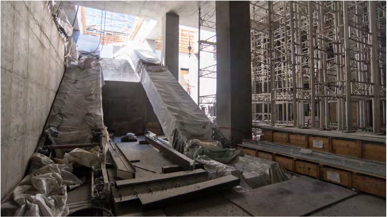
Sections of future escalators have been installed into the lower portion of the Yerba Buena/Moscone Station headhouse, while a network of struts support the roof slab for surface level work.
