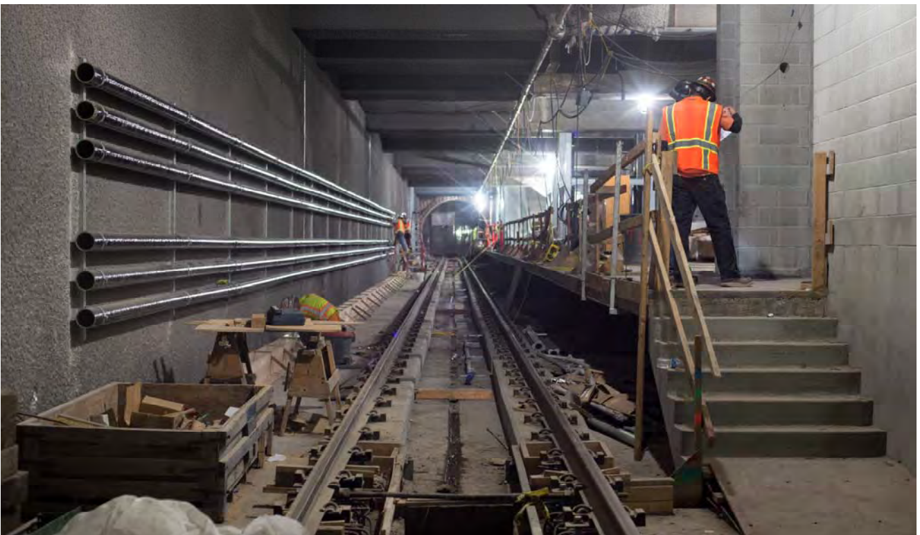
Looking down the northbound track at Yerba Buena/Moscone Station, steel pipe for utilities is being mounted on the wall to the left, while additional elements of the station platform are coming together.
