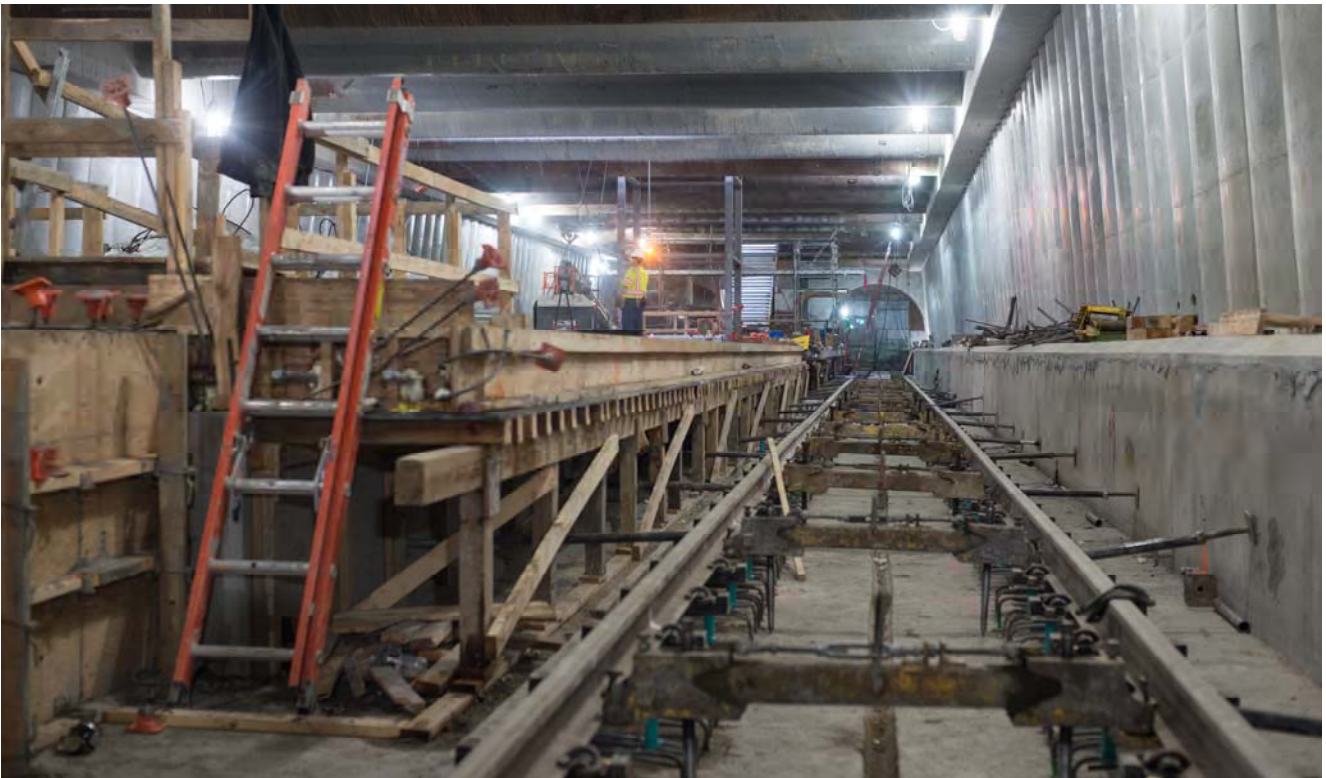
Spacers have been installed to position and align the northbound track adjacent to the future station platform, while formwork to construct the platform itself can be seen to the left.
