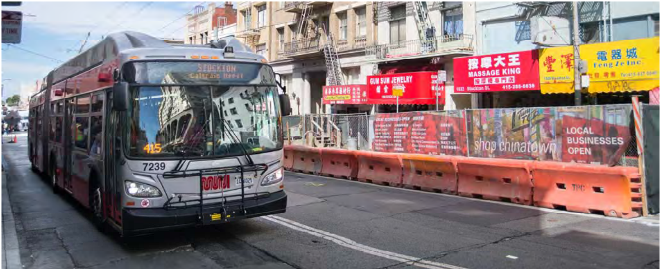
A 30 Stockton bus passes outbound adjacent to the north egress shaft construction site near Washington and Jackson, which has recently been re-expanded to build out the shaft interior.
