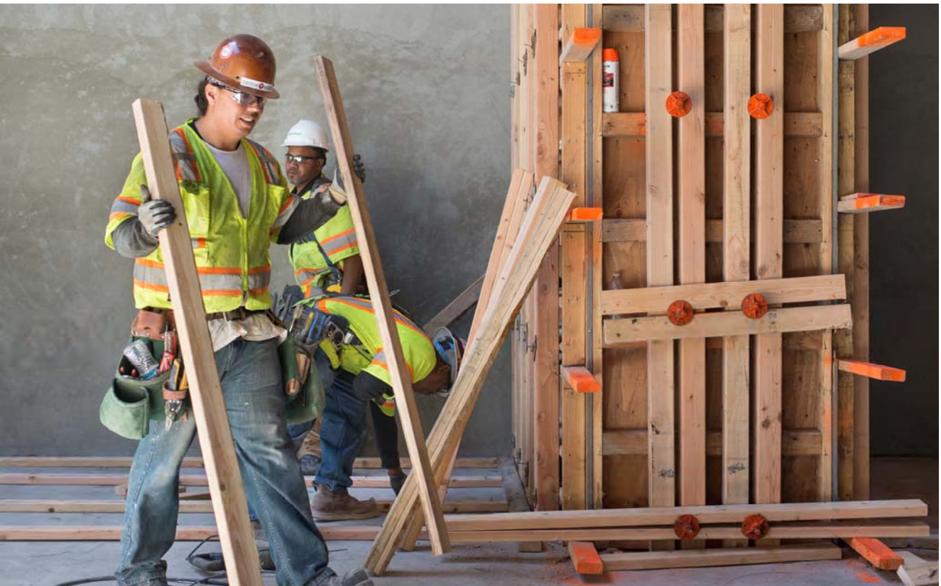
Large concrete forms for vertical columns are being built inside the station headhouse, as structural work will continue to push upward.
