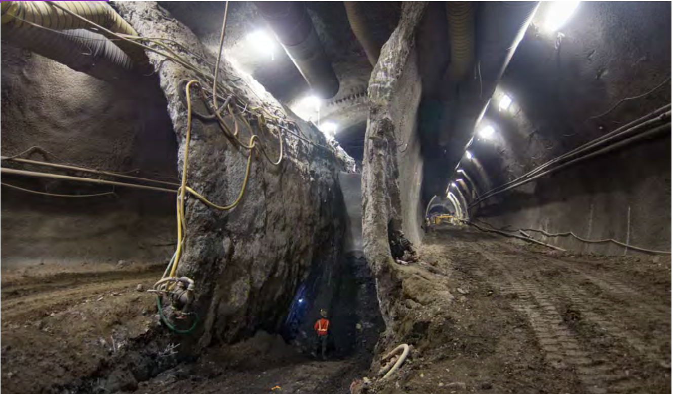
The massive separating walls of the right and left side drifts from the center drift and invert can be seen prior to removal in the CTS south platform cavern.
