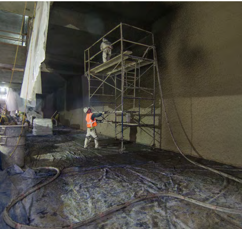
2 A material called Pyrok is sprayed for to lower noise inside the station
