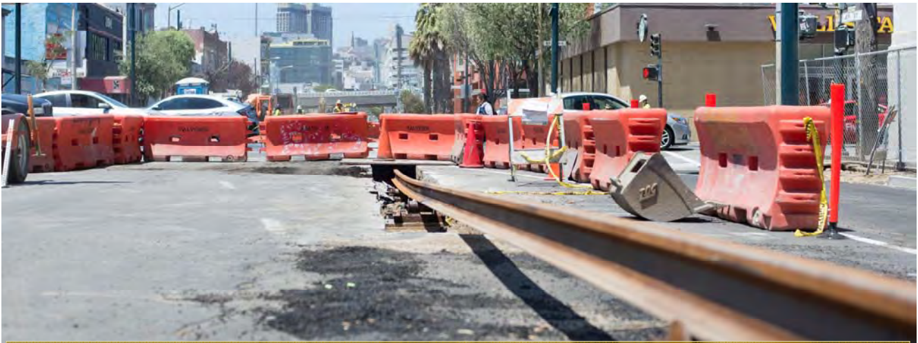
A section of rail is pushed north under the 4th and Brannan intersection using rollers and a trench as it is completed.
