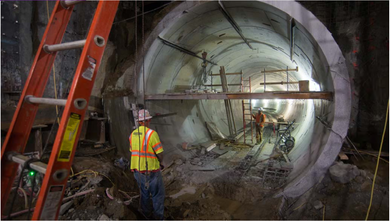
Steel reinforcing is installed against the tunnel walls where they emerge into the south end of the UMS platform level.
