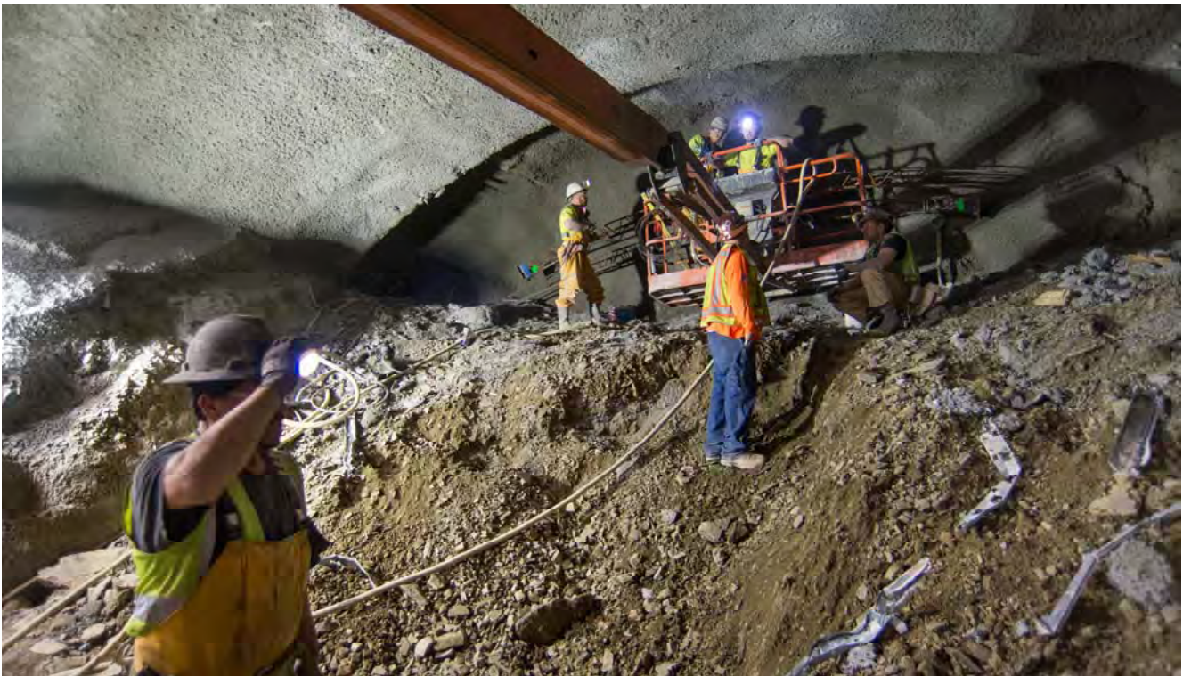
Steel mesh and other steel reinforcing is installed against the ceiling arch of the south platform cavern, prior to spraying shotcrete.
