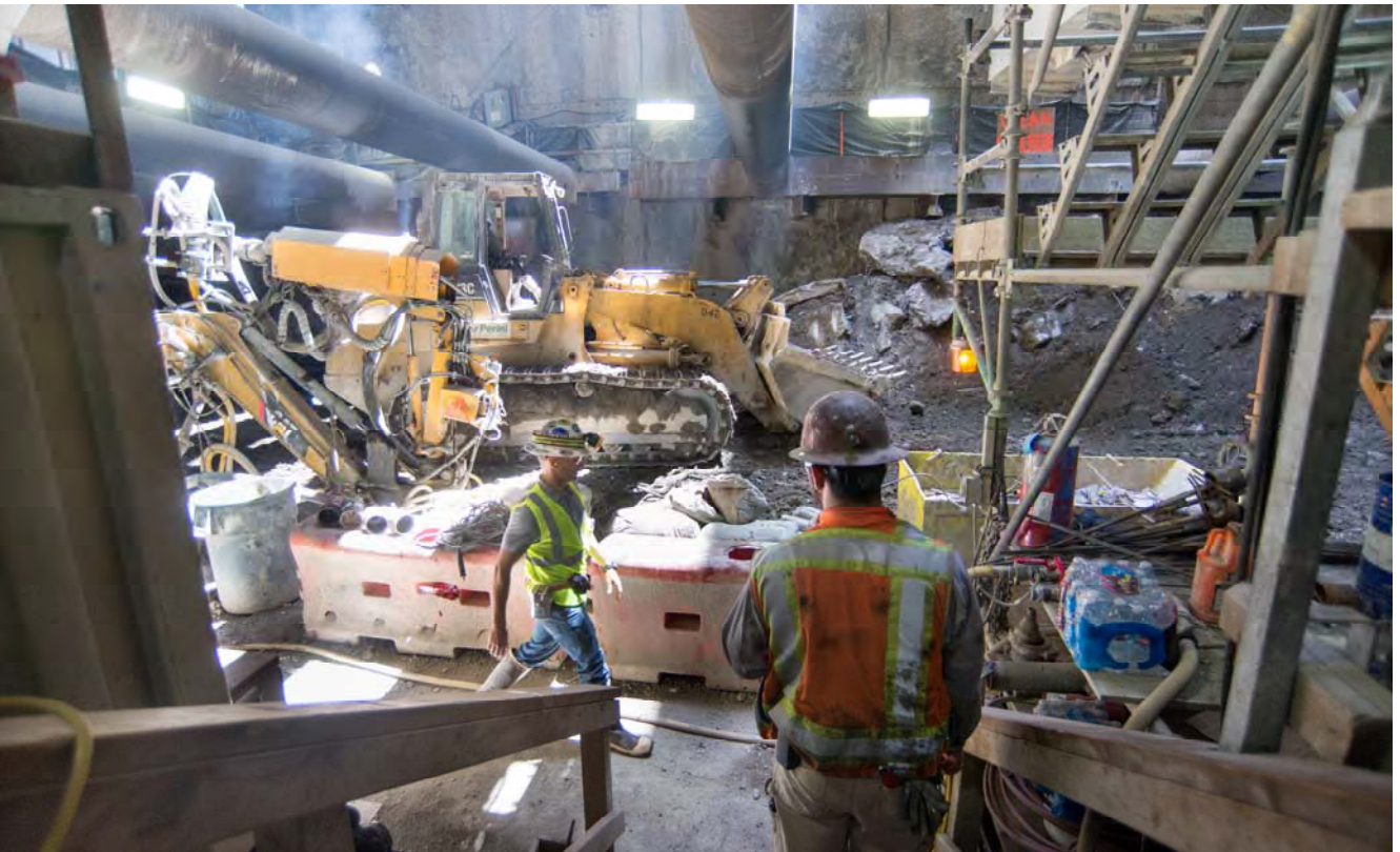
A bulldozer sifts materials removed from inside the south platform cavern, at the collection area inside the station headhouse.
