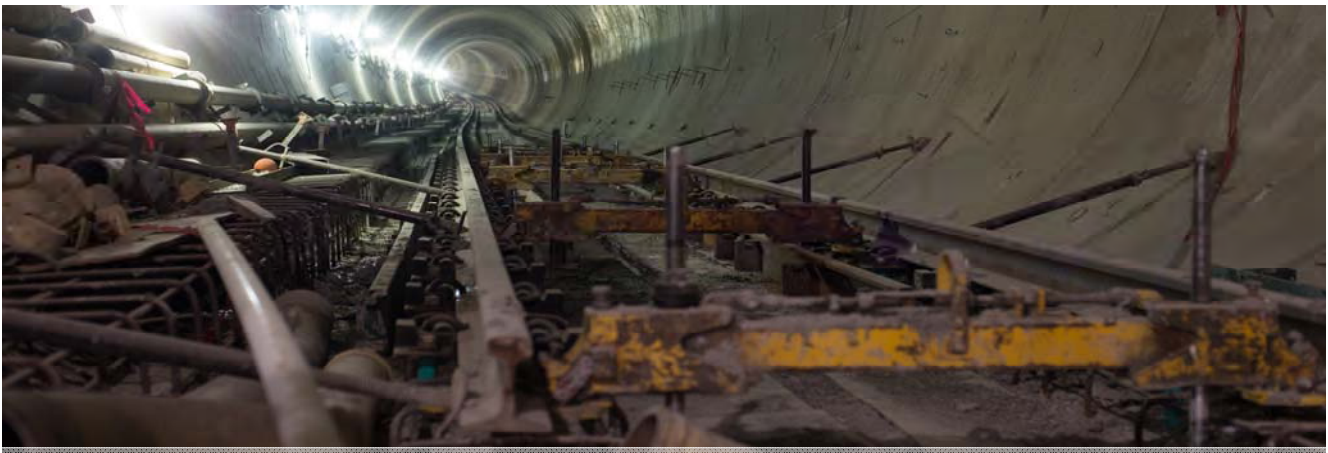
Clamped track spacers help keep rail segments properly aligned during invert construction.
