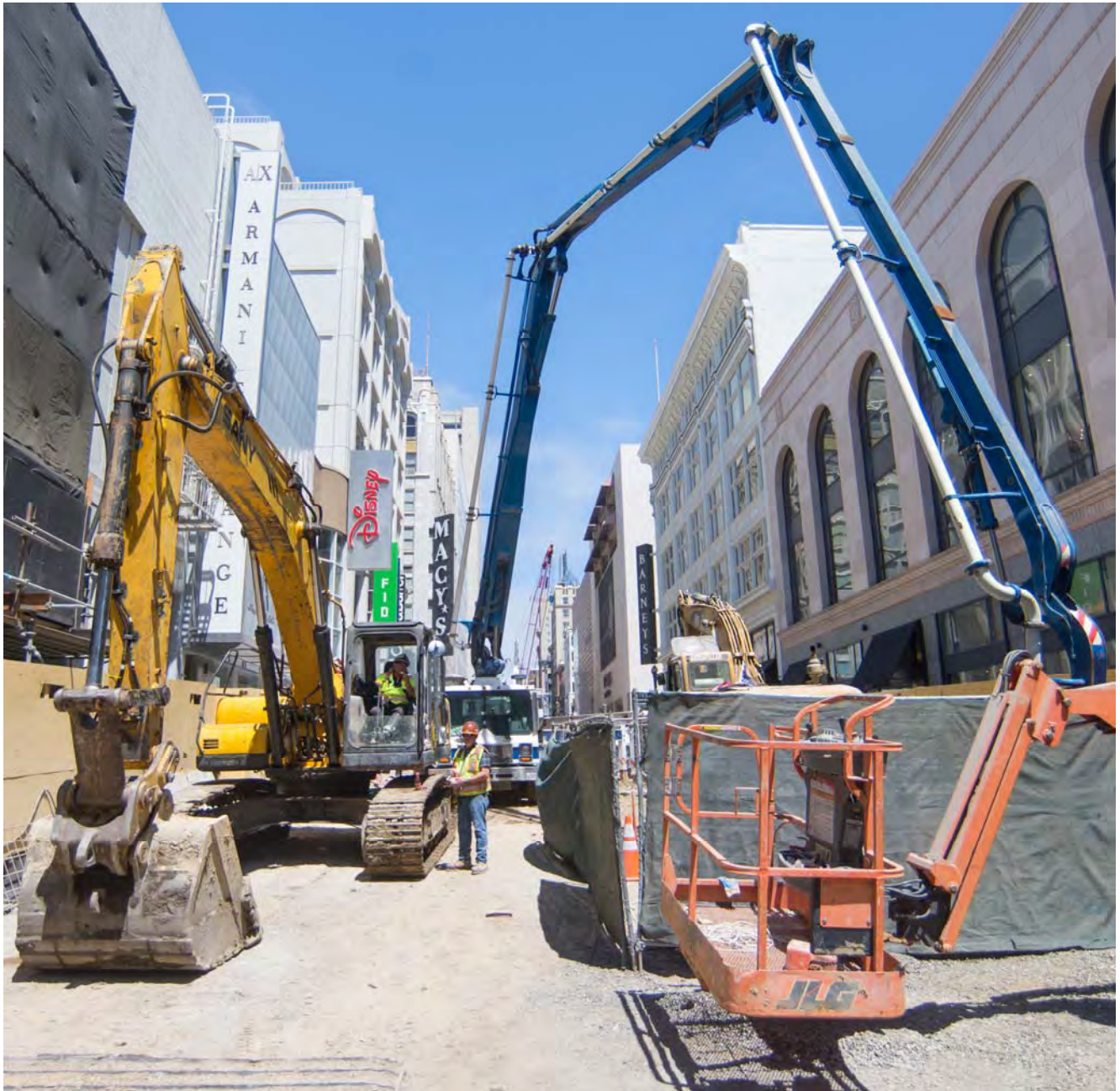
An excavator and concrete boom pump wait at the surface site for the Union Square/Market Street Station just north of Ellis on Stockton.
