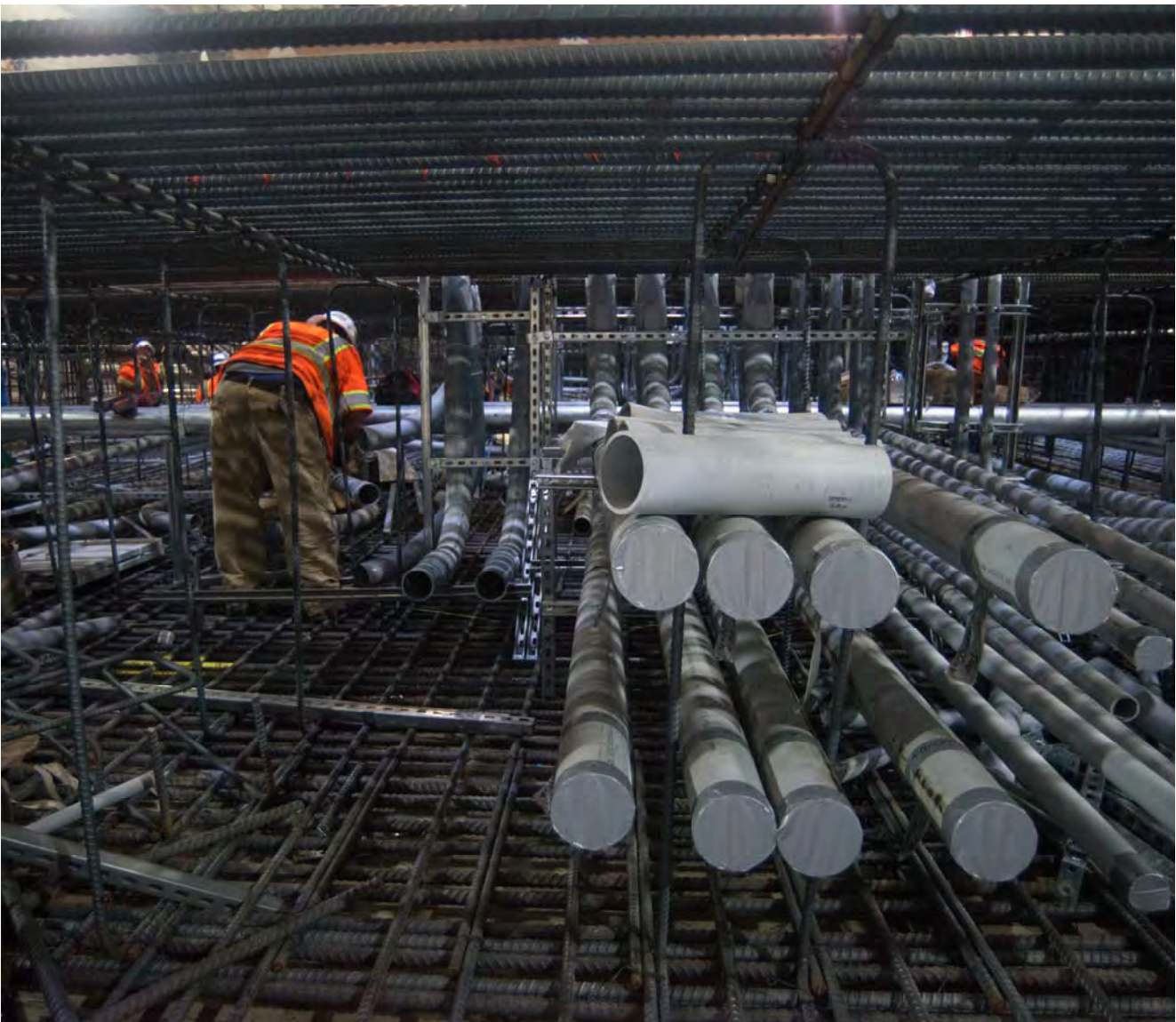
A web of utility conduits are installed among rebar and plumbing inside the future Union Square/Market Street Station's invert slab.
