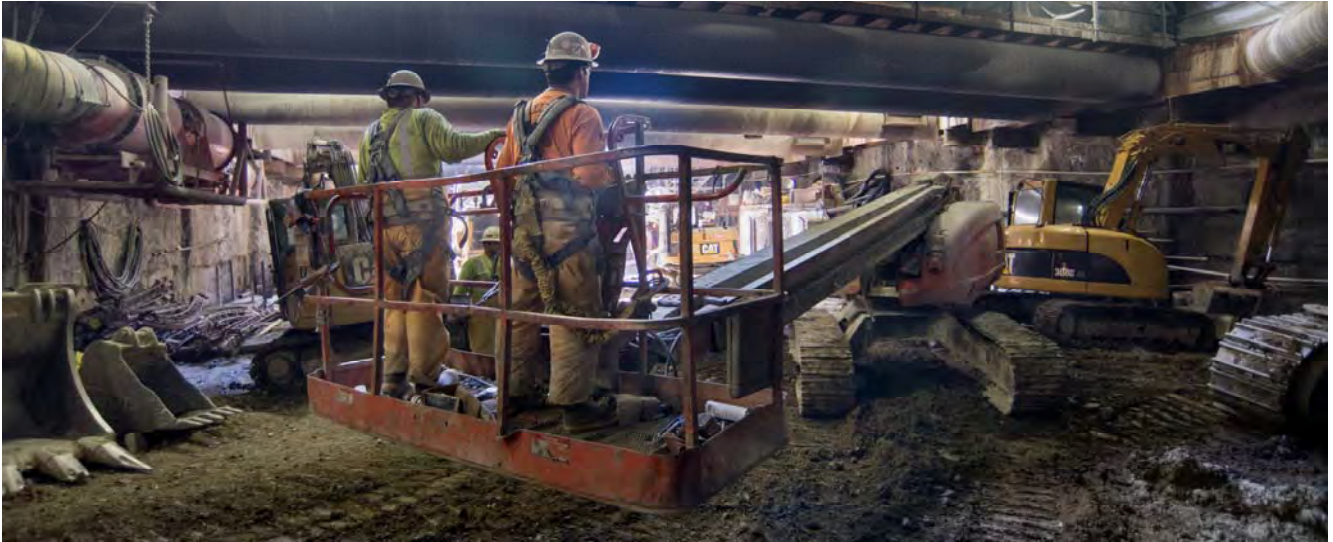
Workers in a hi-lift carefully maneuver out of the platform cavern and into the headhouse, following inspection of drill casings in the arched roof of the cavern.
