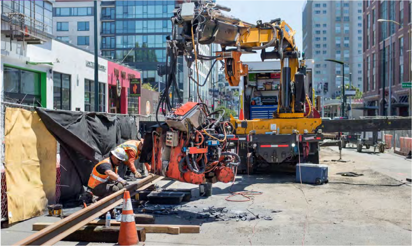
Two men using a rail welding machine inspect their work at 4th and Bluxome.
