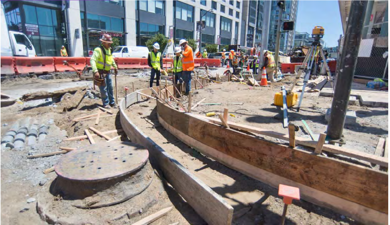
Curved concrete forms used in curb construction are installed at the southeast corner of 4th and Townsend where curb and sidewalk restoration work is underway.
