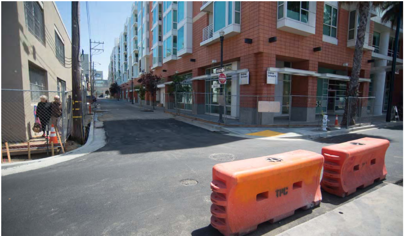
Fresh asphalt marks the entrance to Welsh alley, which has recently been reopened for vehicular traffic to 4th Street.
