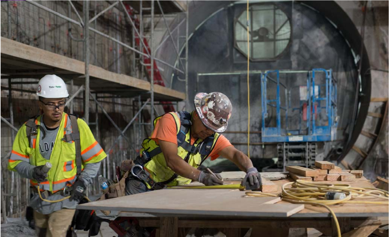
Carpenters mark on sheets of MDF where cuts will need to be made, during concrete form construction inside the platform level of the station box.
