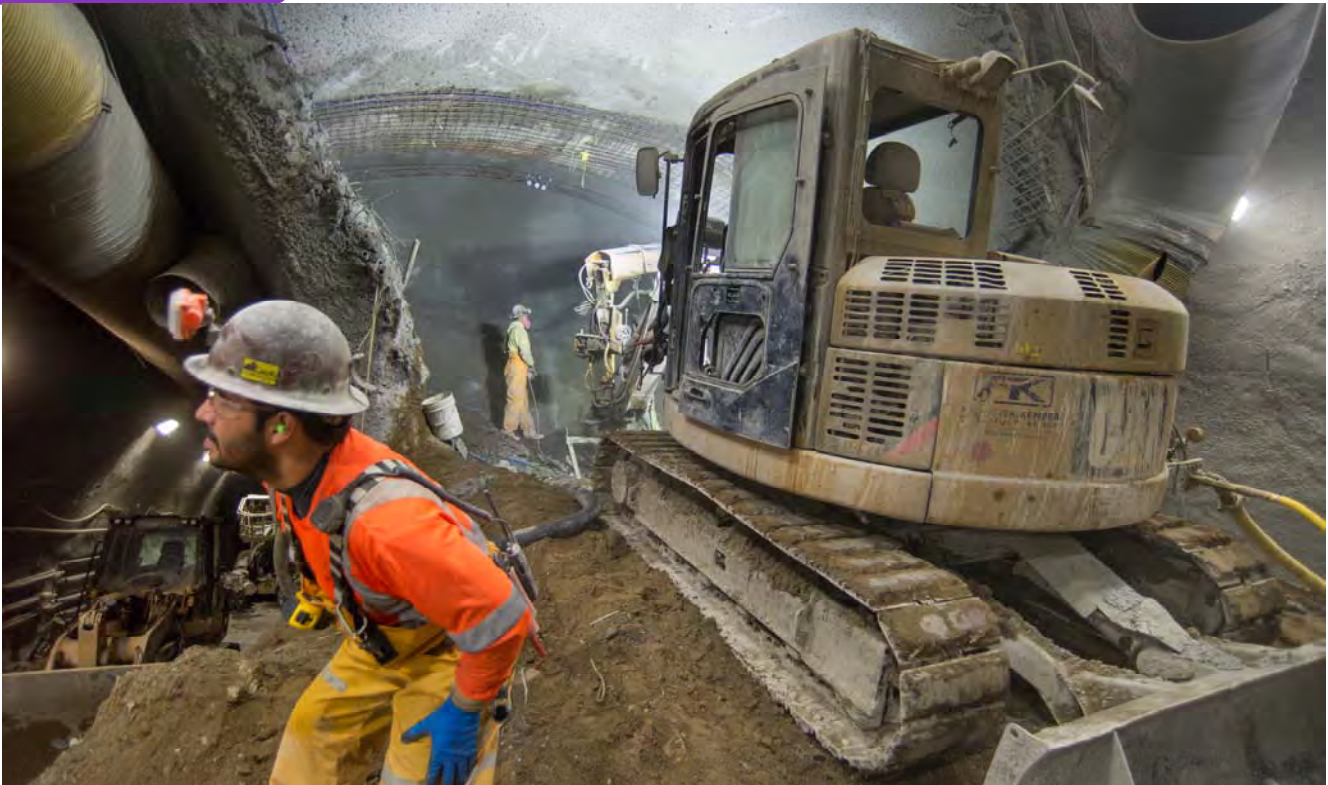
Excavation of the top heading for the north platform cavern has begun. Here, workers are spraying shotcrete on exposed rock, following a push of excavation.
