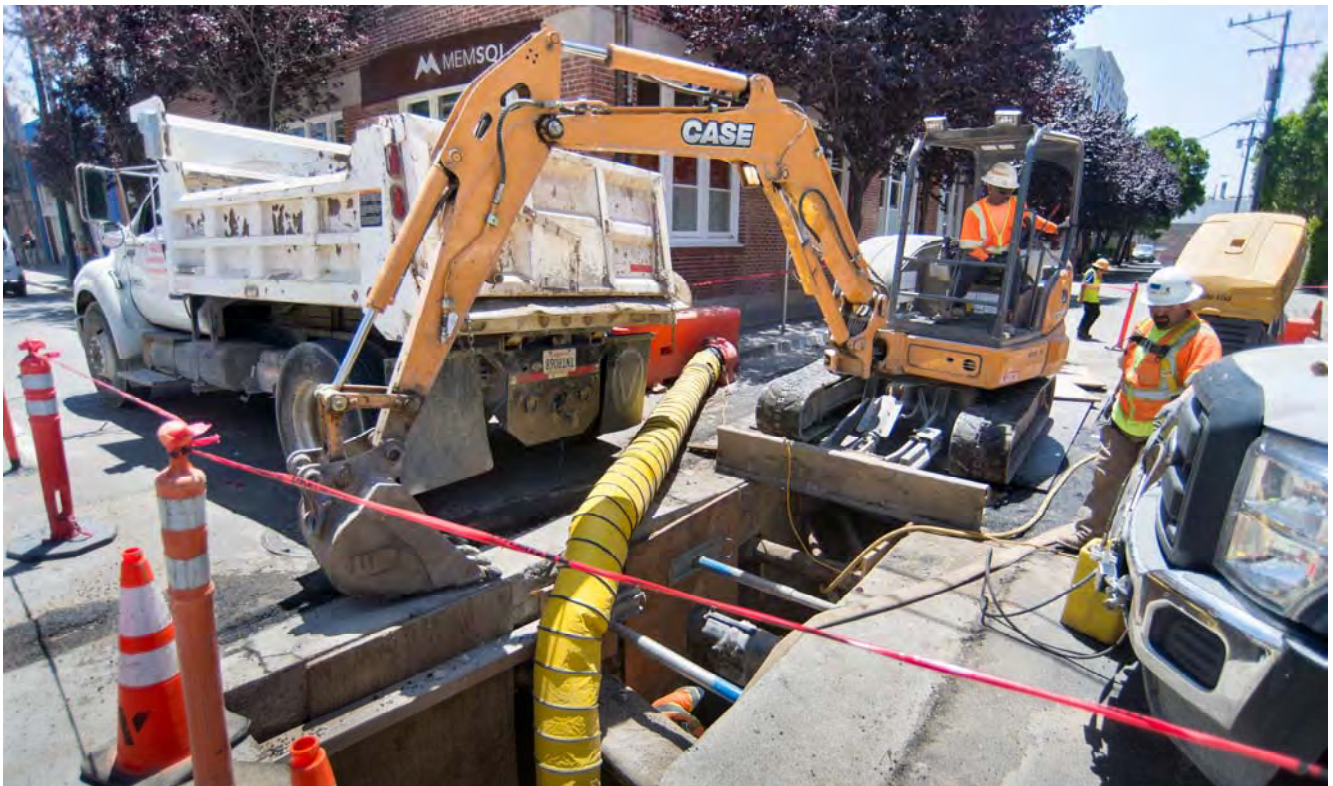
A trench for new sewer lines leads from 4th Street down Freelon Alley along the surface portion of the alignment in SoMa.
