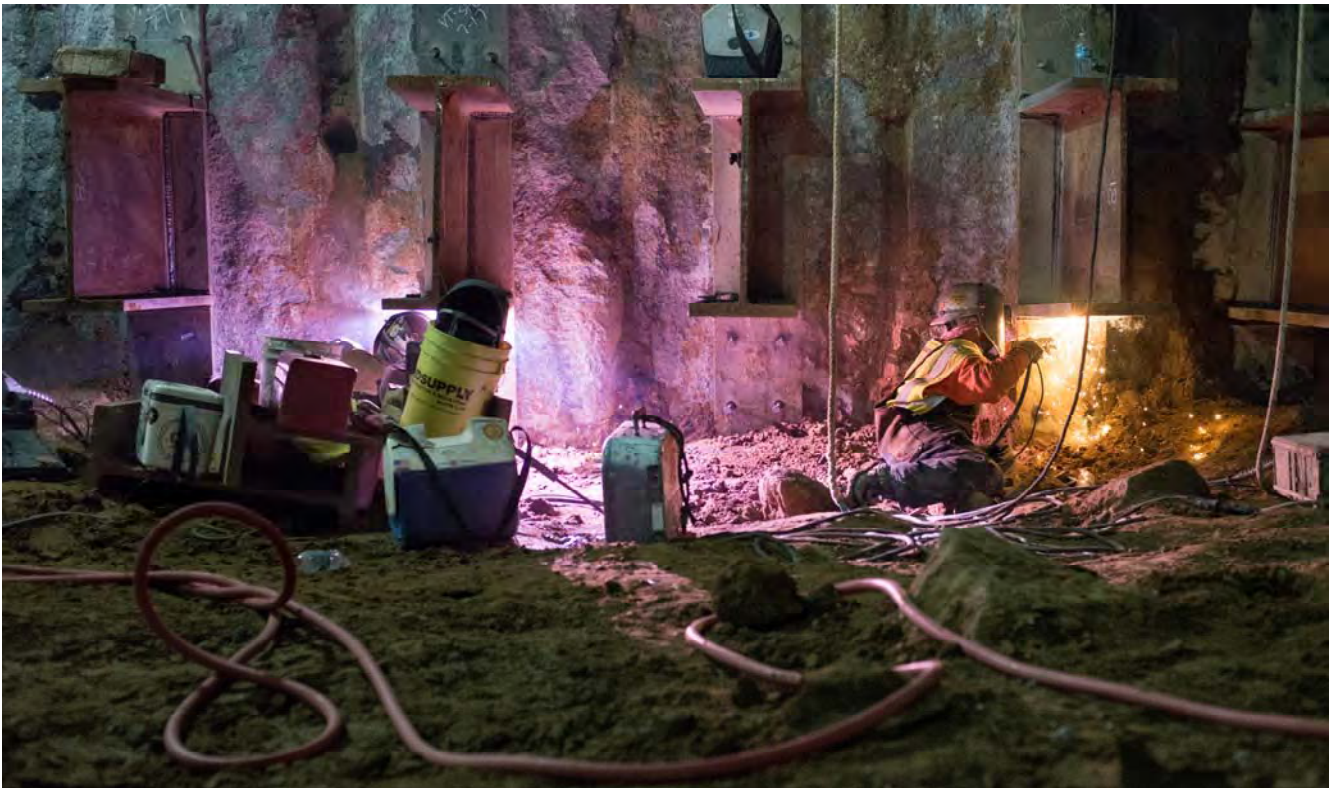
Two welders work on huge steel I-beam brackets along the east wall of the station box, prior to pouring the initial “rat slab” of the station box in this section.
