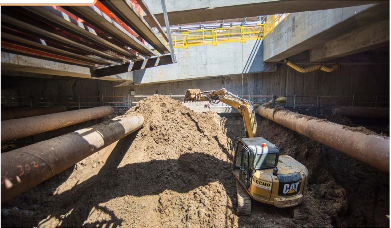
A mini excavator piles soil high for the large excavator on the temporary deck above to lift away.
