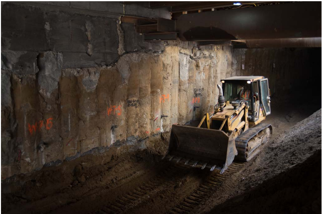
A bulldozer ferries back and forth sifting excavated material inside the future south concourse of the Union Square/Market Street Station.
