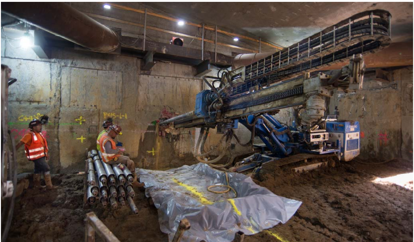
Drilling to inject grout and improve soil conditions is ongoing around the exterior of the station headhouse.
