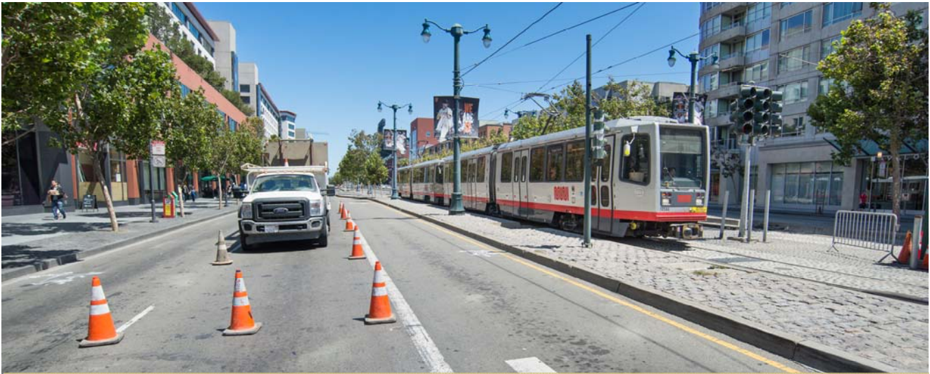
An N Judah train approaches the intersection of 4th and King. Utility work at this intersection is ongoing, ahead of track configuration upgrades over Labor Day weekend.
