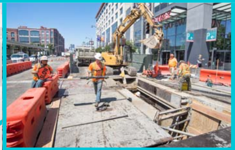
4th St. Surface Track, Systems (STS)
