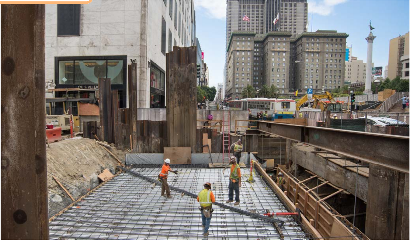
A crew has begun installing a rebar lattice atop a section of corrugated steel sheets used in the construction of the Union Square/Market Street north concourse roof deck.
