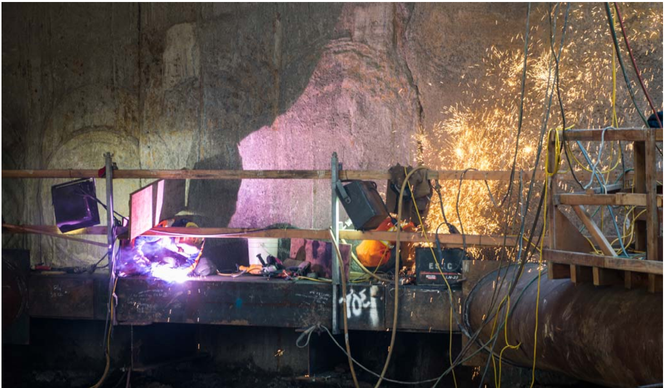
Light flashes and more sparks fly with welding and torch cutting atop one of the temporary steel supports.
