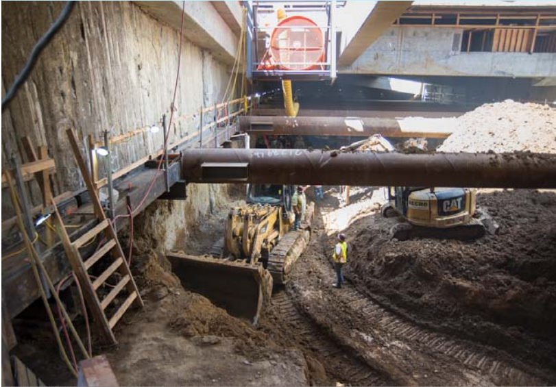
1 With each level of excavation complete, steel supports are installed to support walls
