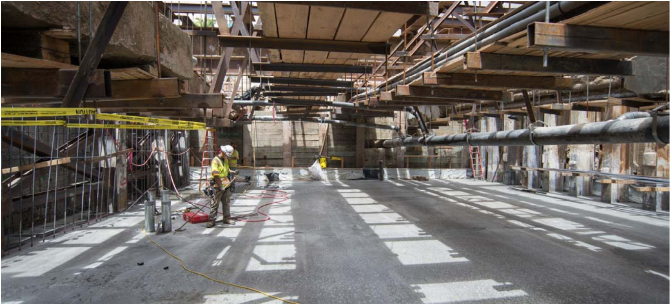
A finished concrete slab rests atop steel beams comprising the roof of this section of the north station concourse at the Union Square/Market Street Station site. Utilities are temporarily suspended above.
