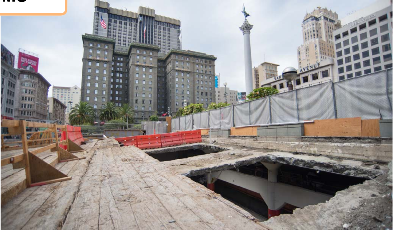
Access holes have been created to remove demolished material from the garage interior.
