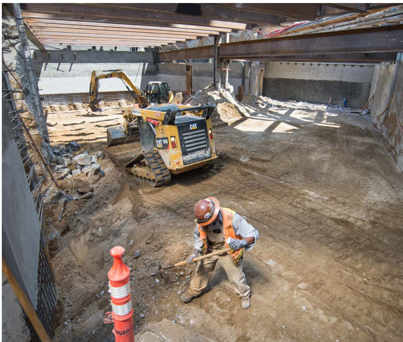
A worker removes excavated debris while interior wall construction and site excavation are ongoing at the south concourse of the Union Square/Market Street Station
