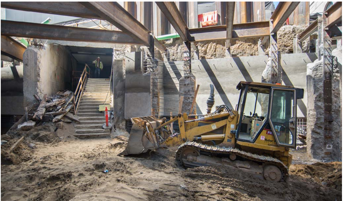
Stairs from the former Ellis Street entrance to Powell BART/Muni Station are visible amid new structural beams and piles integrating the old access point with the new south concourse of the station.
