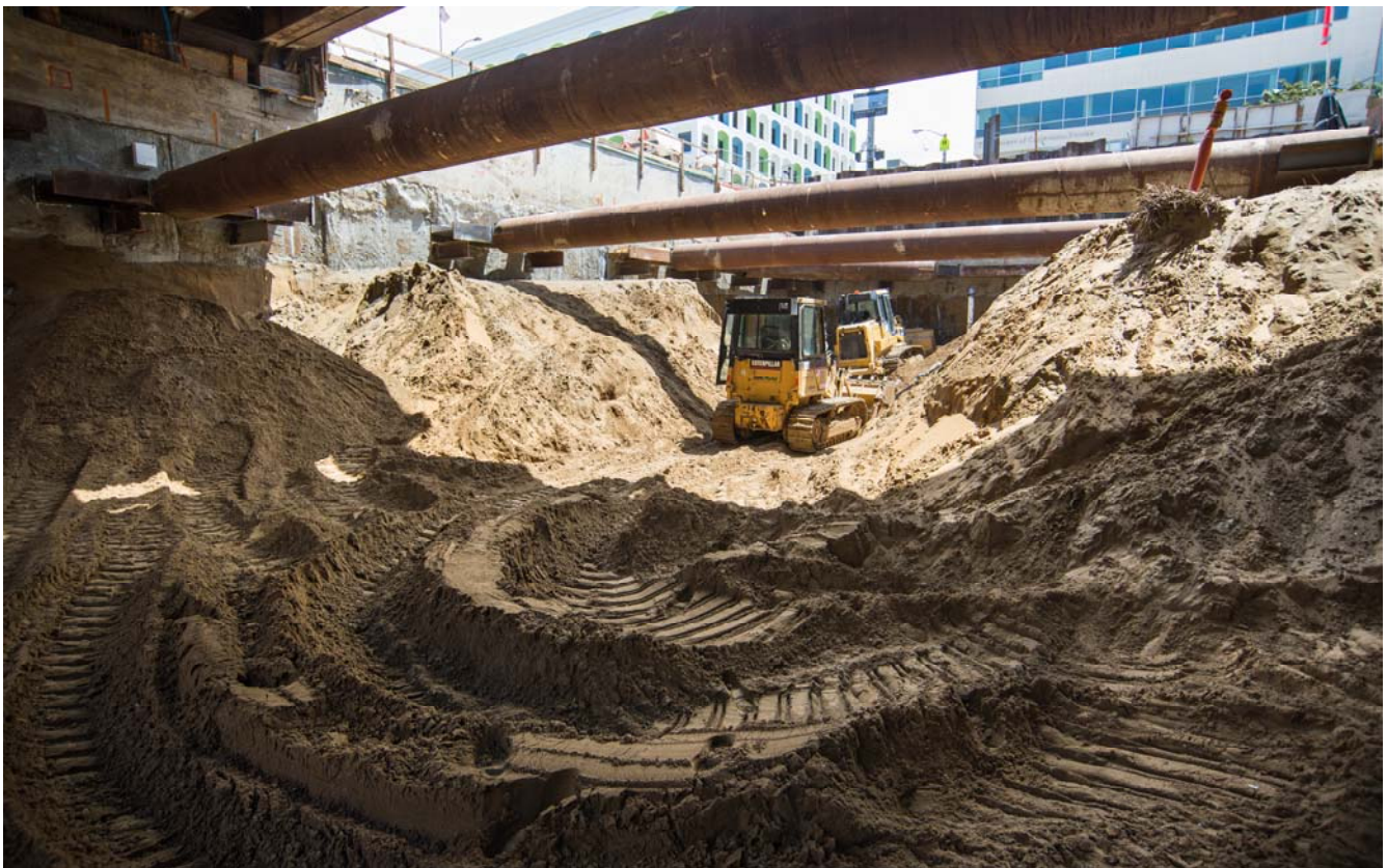
Under the shadow of the temporary deck constructed over the headhouse excavation area, which will be used for cranes and other large equipment.
