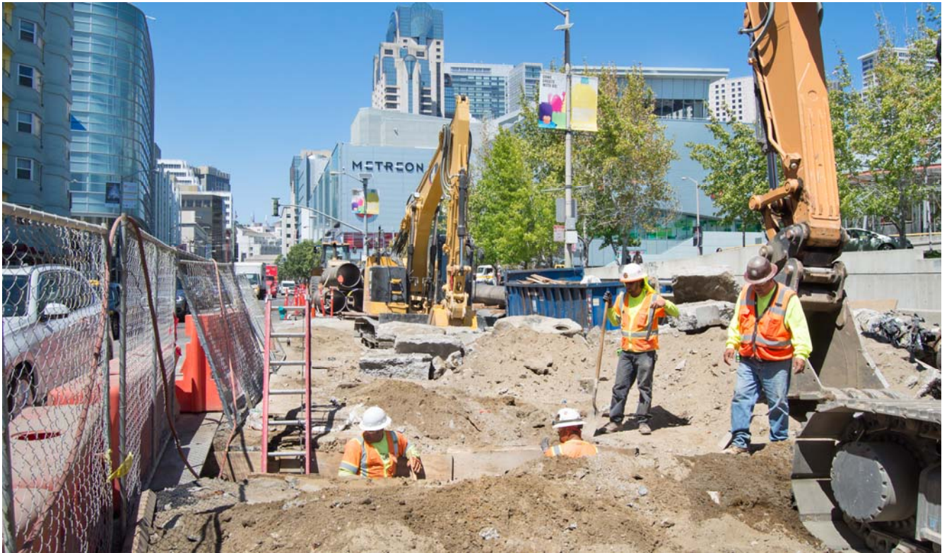
Trenching operations to tie in new utilities following backfilling of the last section of roof slab to be constructed, south of Howard on 4th.
