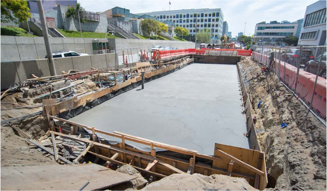
The last section of finished Yerba Buena/Moscone Station roof slab prior to the installation of waterproofing.
