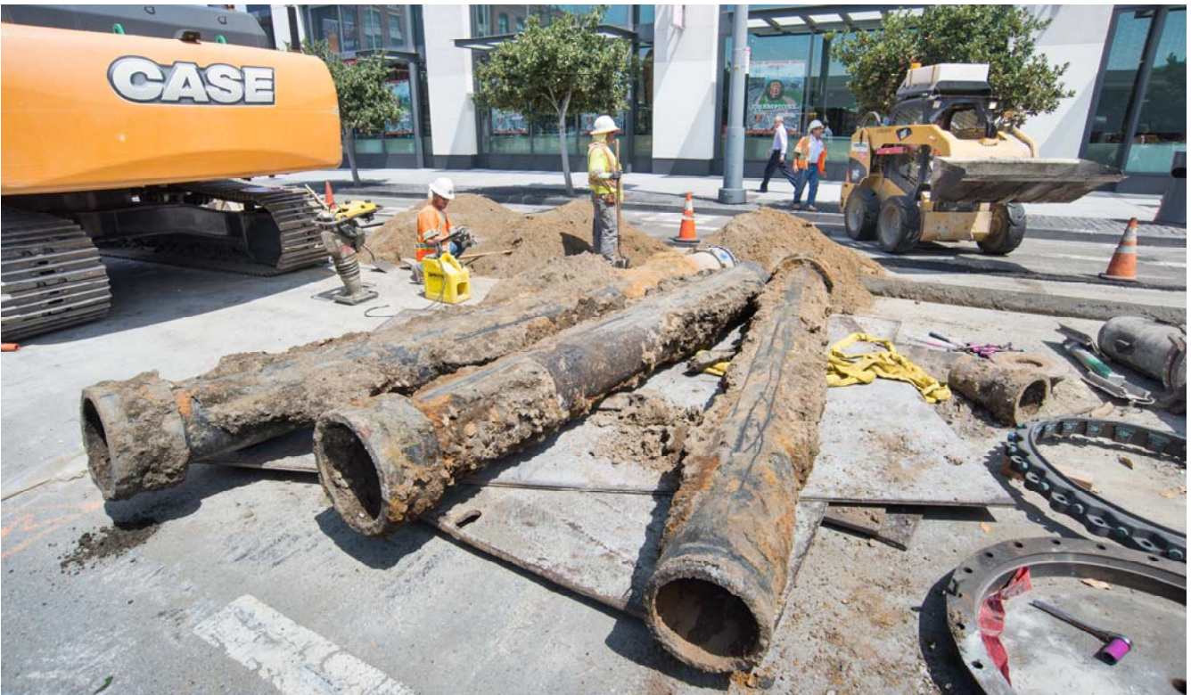
Sections of old sewer pipes see the light of day before being upgraded on 4th south of Townsend.
