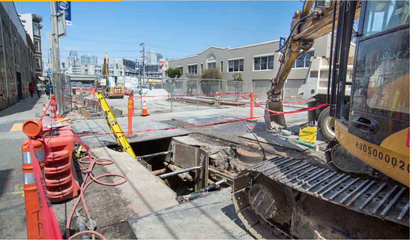
Trenching and utility upgrades are ongoing at 4th Street and Welsh. Here, temporary steel plates cross the utility trench to allow vehicular access.
