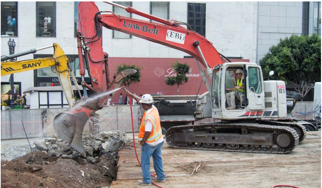
Demolished material is sorted by an excavator operator and wetted down for dust reduction prior to being removed offsite.
