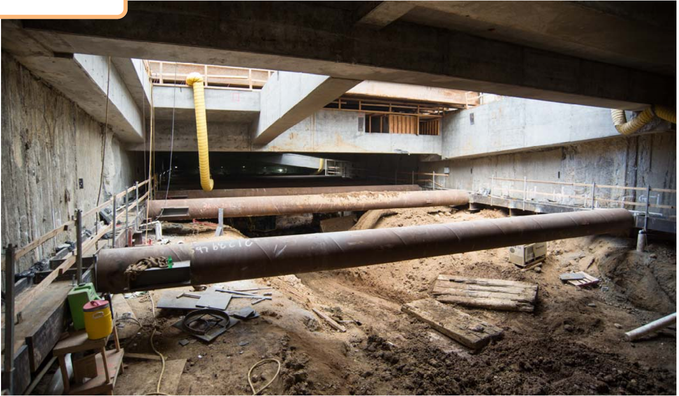
With the first level of excavation inside the station headhouse complete, these temporary steel supports have been installed to equalize soil pressure against interior walls.
