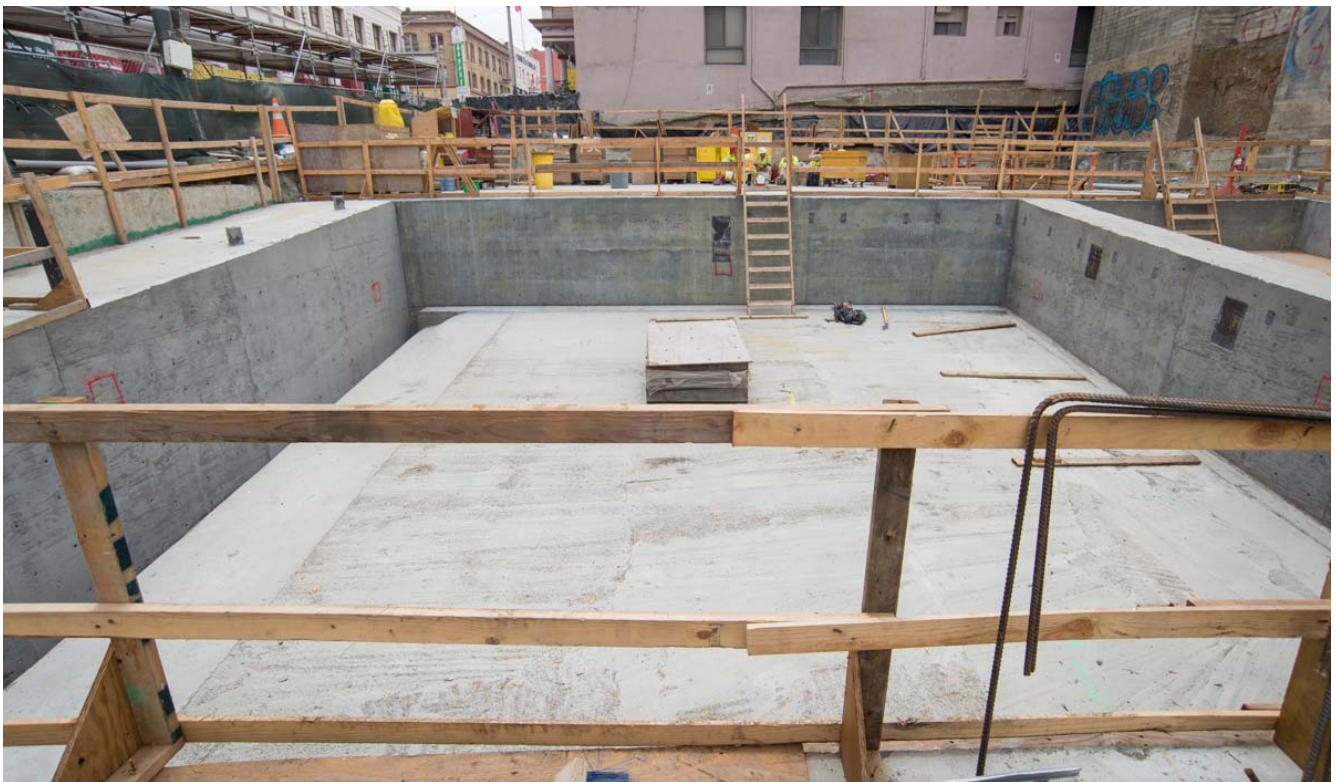
The floor of this pool-like opening will be demolished, creating an opening where the future stairs and escalators will usher customers to the station interior.
