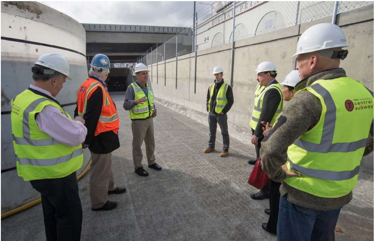
Project Director John Funghi speaks to members of the Community Advisory Group at the tunnel portal ramp.
