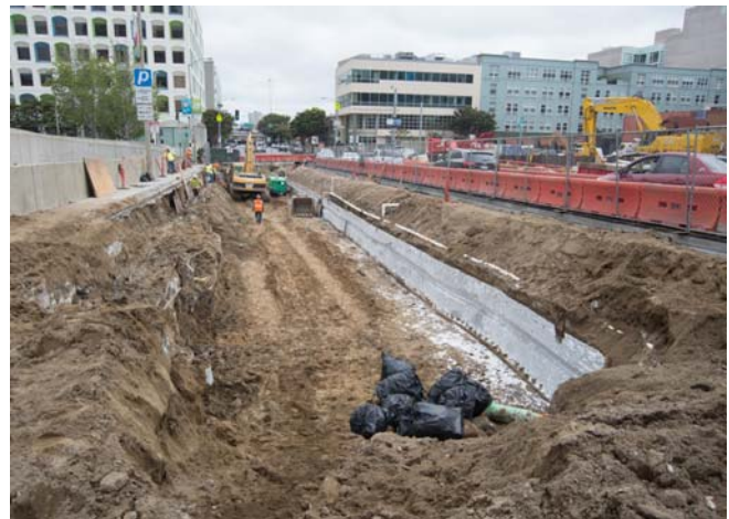
Excavation of the east side of the Yerba Buena/Moscone Station roof slab site is underway.
