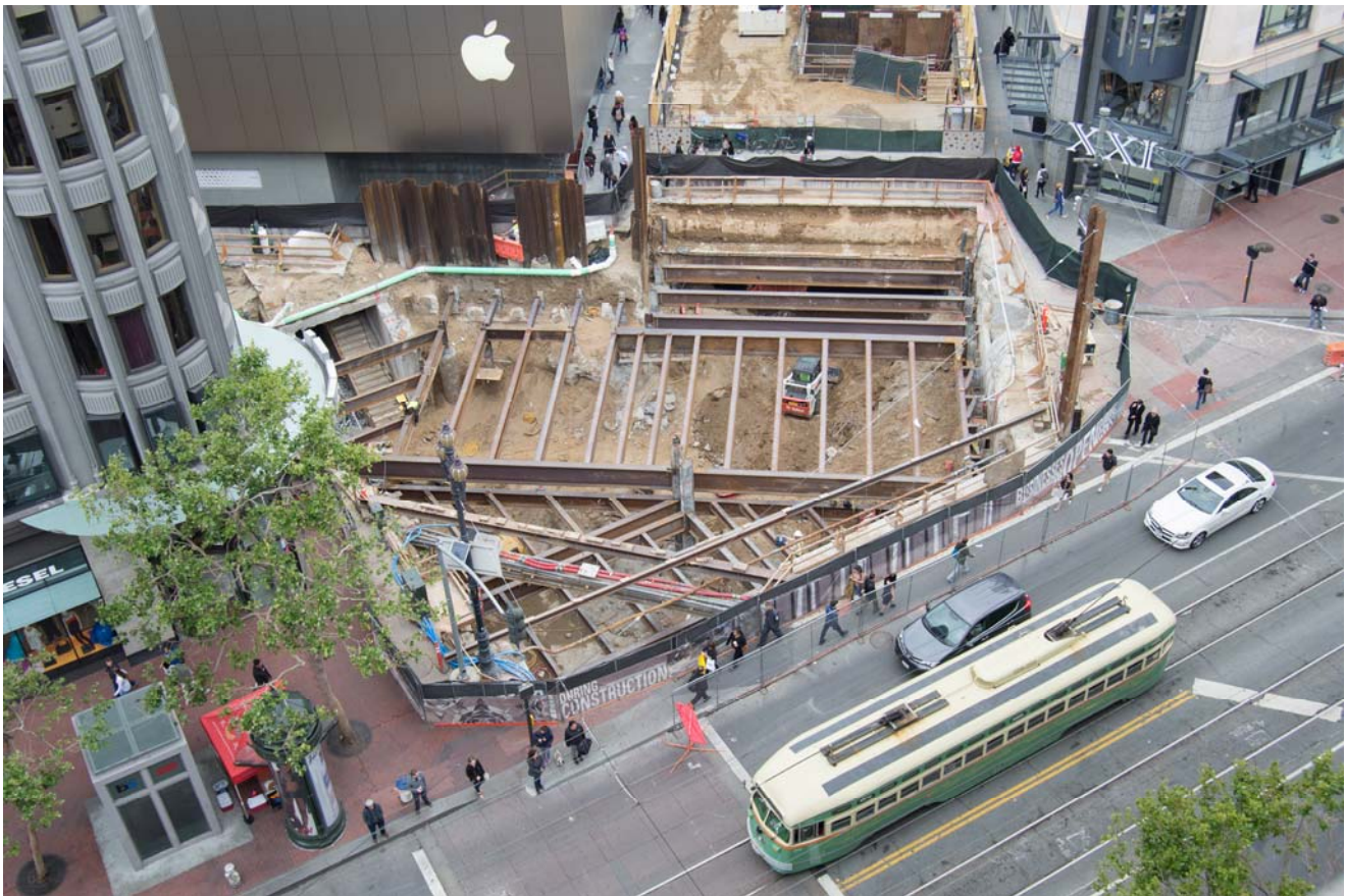
The intersection of Ellis and Stockton, adjacent to Market Street, as seen from the roof of 801 Market. Here, work to construct the roof of the new concourse is underway.
