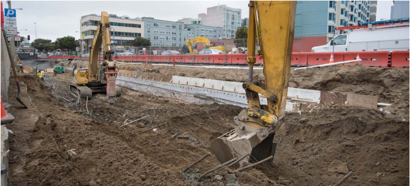
An excavator bucket removes soil from the Yerba Buena/Moscone Station site, where roof construction is being done on the east half of 4th Street, north of Folsom.
