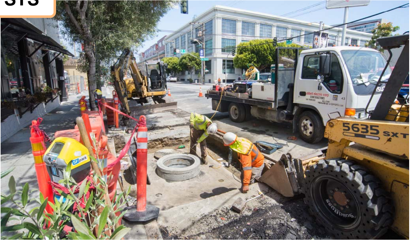
Workers put the final touches on a new manhole and utility duct bank on the northwest corner of 4th and Brannan.
