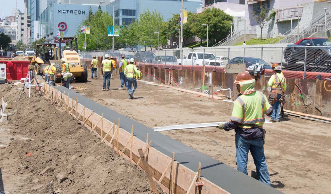
Before switching traffic temporarily to the west side, workers had to rebuild the roadway over what, until recently, had been an active work zone constructing the station roof.
