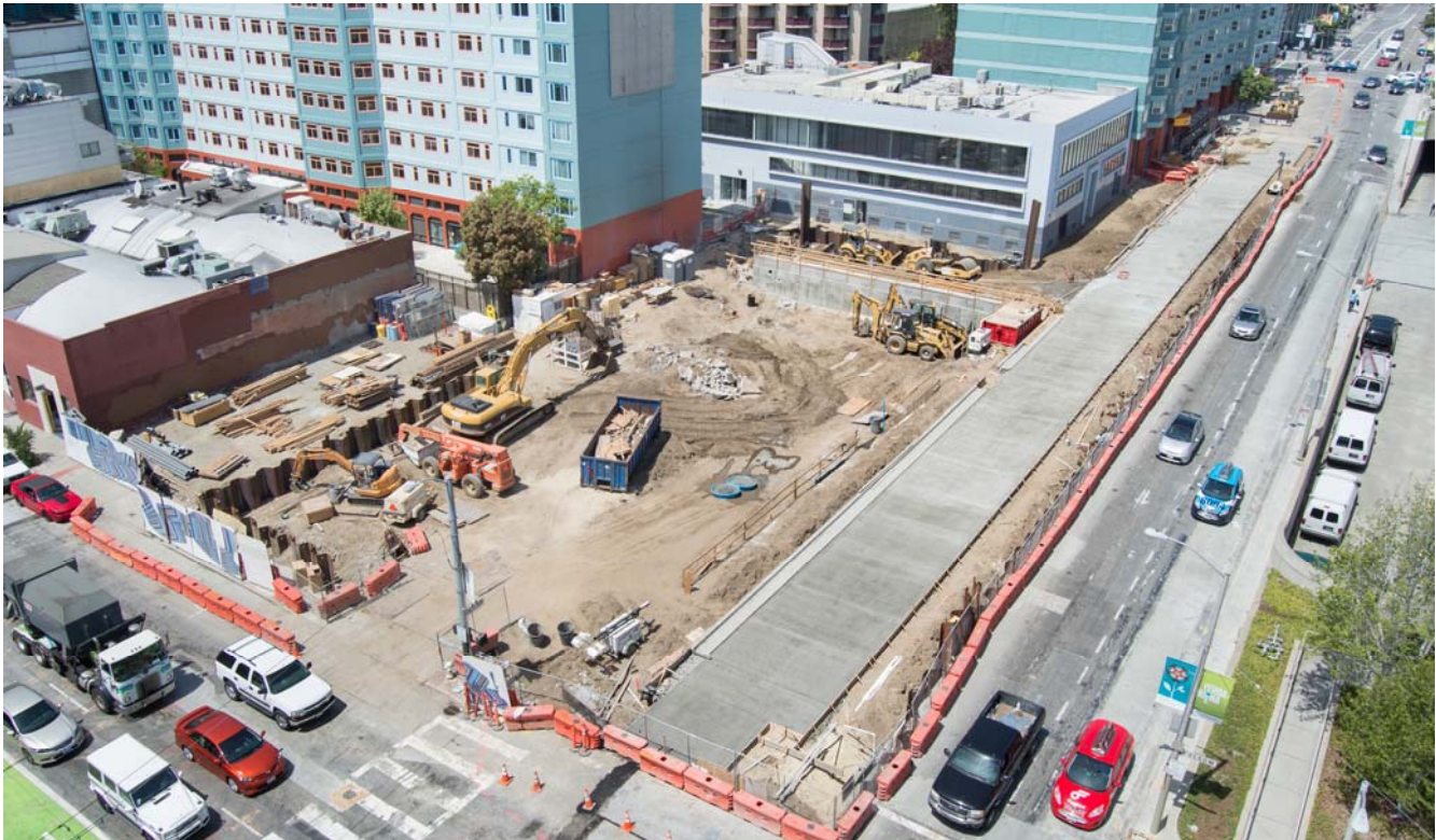
With the curb complete, workers then constructed a portion of the final concrete road bed.
