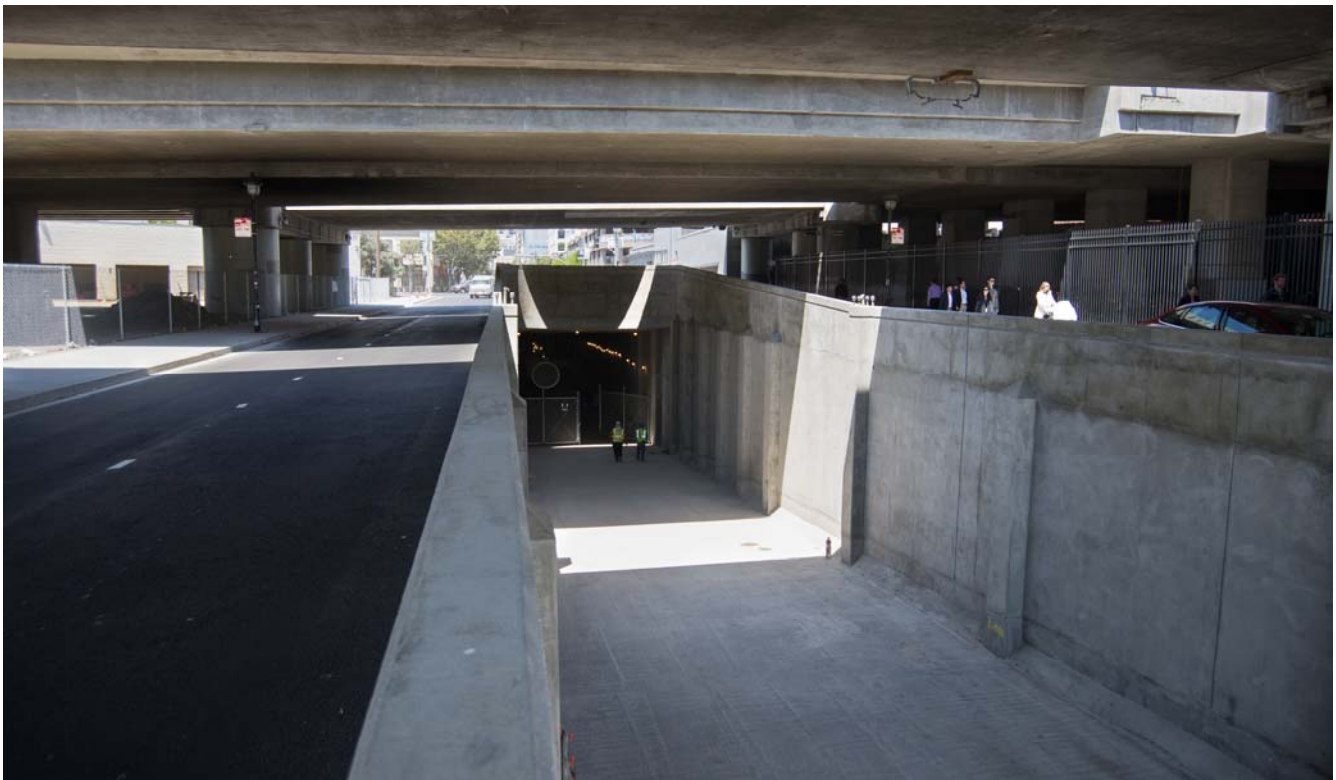
Looking north up 4th Street under I-80, the tunnel portal ramp will be the jump-off point for T Third trains to enter and exit the Central Subway tunnels.
