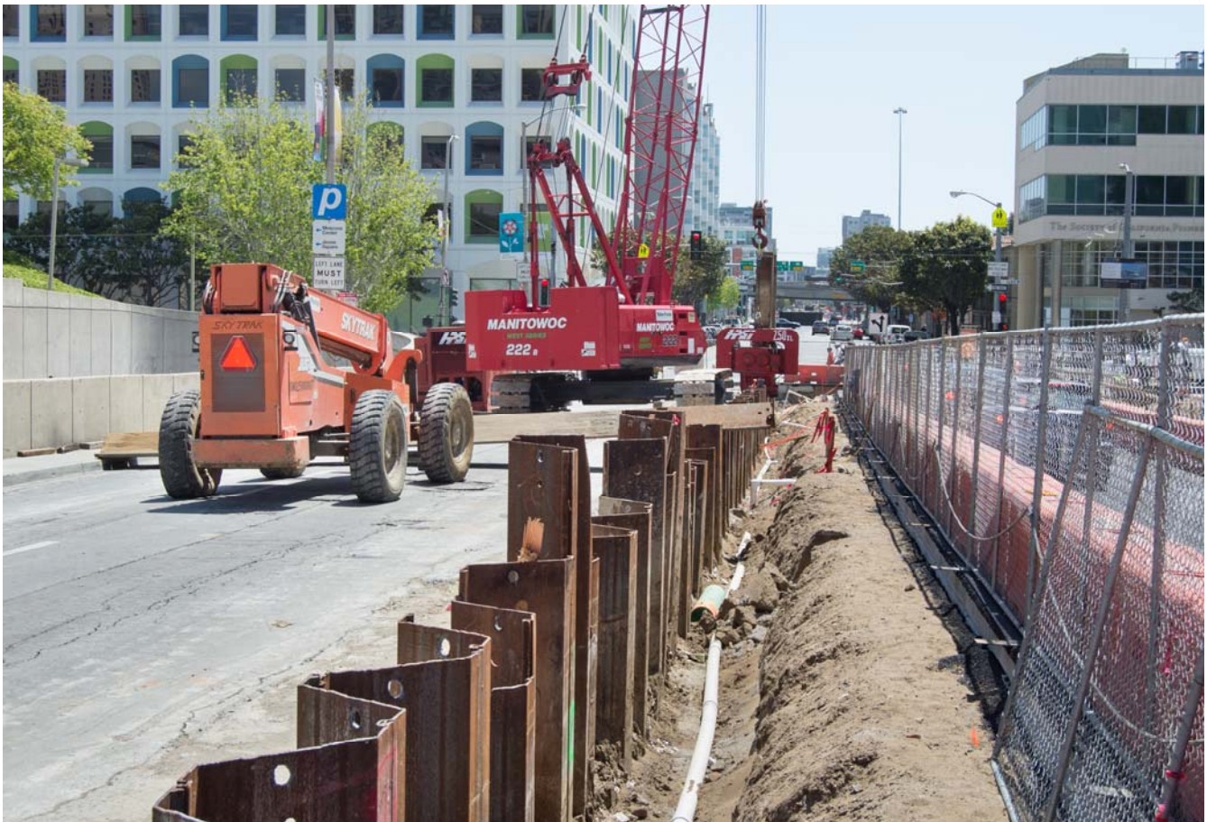
The contractor can be seen removing steel sheet piles prior to excavation of the east side of 4th Street, to construct that portion of the Yerba Buena/Moscone roof slab.
