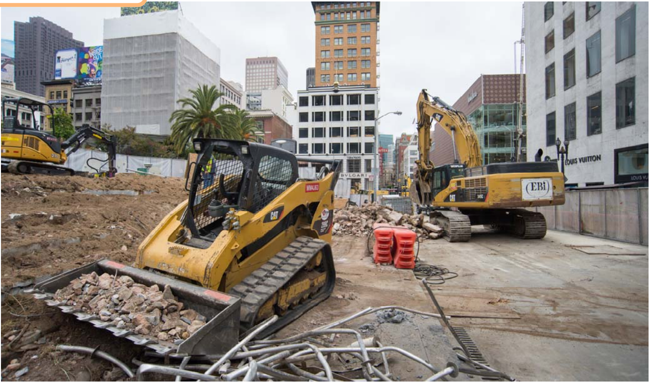
In order to construct the north entrance to the Union Square/Market Street Station, the entrance site must first be cleared of benches, plants, and structures.
