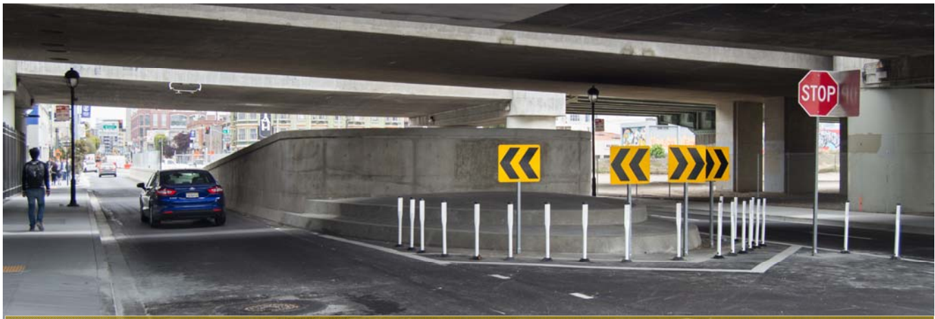
Striping and hazard signage marks the approach to the tunnel portal, located beneath I-80 on 4th Street, south of Harrison.
