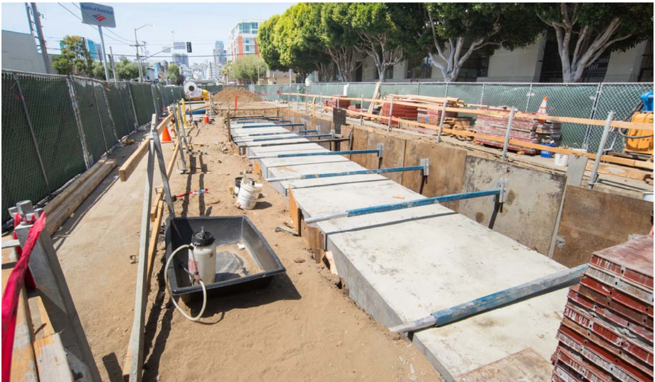
A gleaming new reinforced concrete sewer roof can be seen shortly before being back-filled, south of Brannan on 4th Street.
