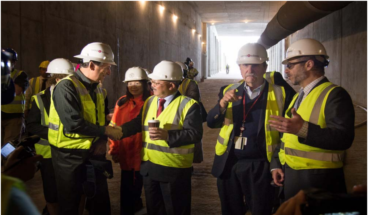
San Francisco Mayor Edwin M. Lee, SFMTA Board Chairman Tom Nolan, Director of Transportation Edward Reiskin and Project Director John Funghi on the tunnel portal ramp.
