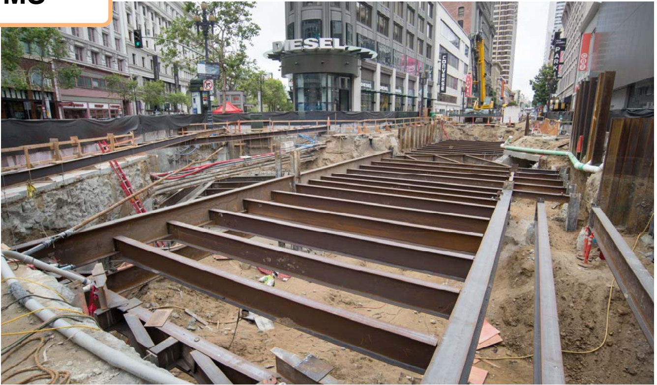
Steel I-beams are now being installed to support the future roof structure of the south station concourse.
