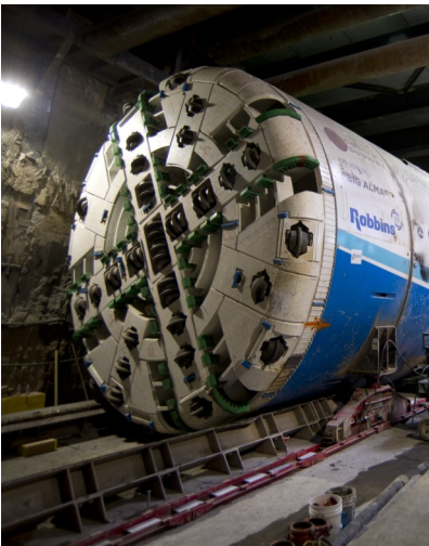
Tunnel boring machine Mom Chung is the first to arrive in San Francisco.
