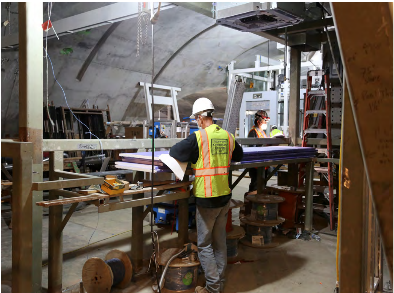
Workers reading plans inside CTS making sure that everything is being installed correctly
