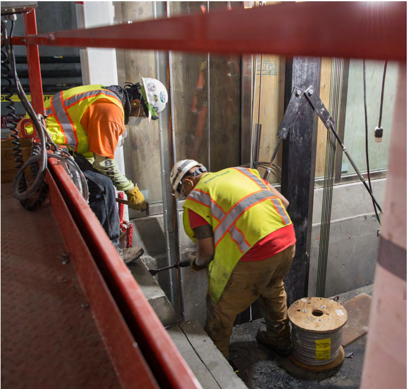
Two men remove excess concrete from around an elevator shaft opening on the Union Square/Market Street Station platform.
