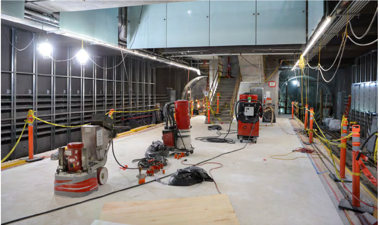
The initial layer of terrazzo has been poured and smoothed near the south end of the Yerba Buena/Moscone station platform.
