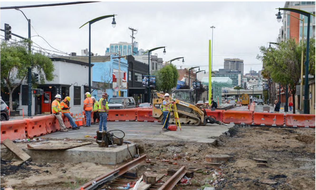
A surveyor checks measurements at the southeast corner of the 4th and Brannan intersection, where roadway restoration is underway.
