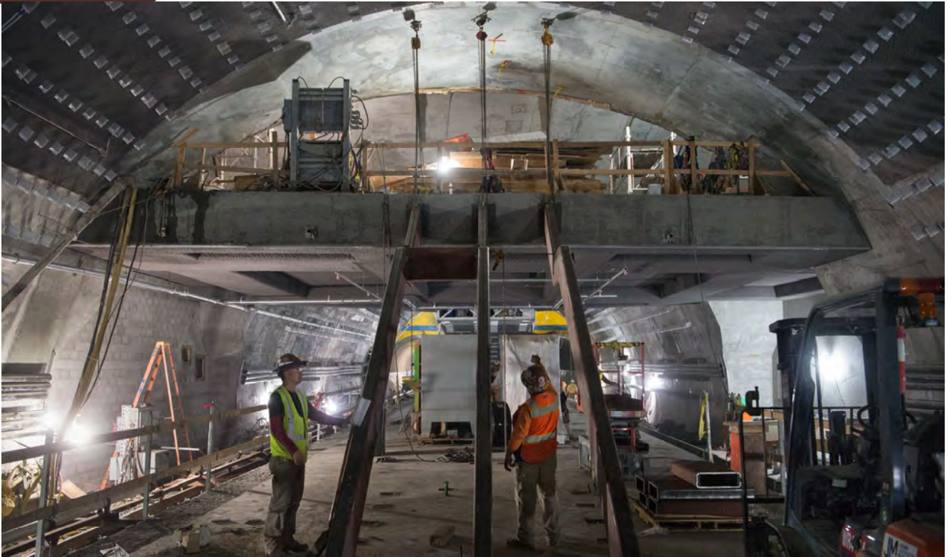
Structural steel elements have been installed as a first step to build the concourse-to-platform staircase inside the Chinatown Station platform cavern.
