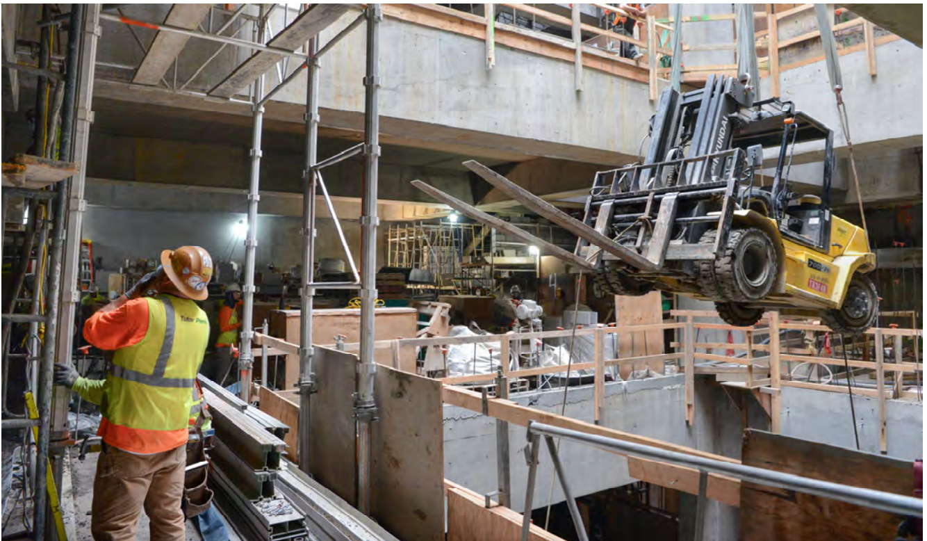
With much of the major structural work now complete inside the lower levels of Chinatown Station, large equipment is being brought to the surface to make room for interiors and systems.
