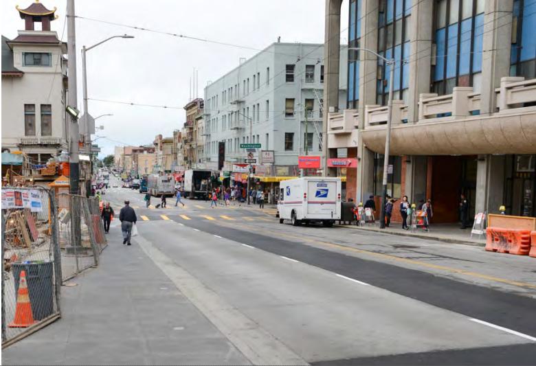
New curbs, pavement, sidewalks, and a bus stop pad have been built.
