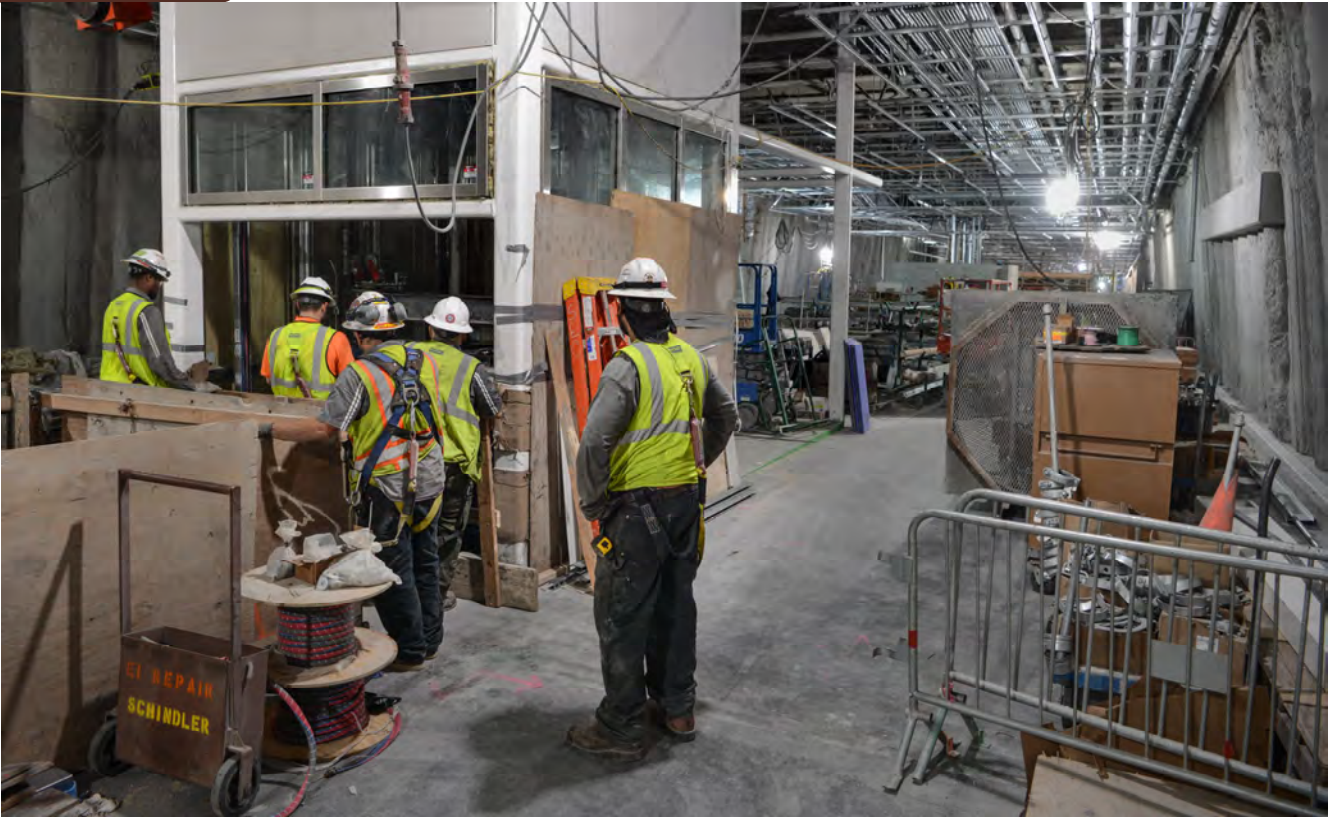
Crews have been hard at work assembling elevator components and testing systems, looking south on the concourse level for Union Square/Market Street Station.
