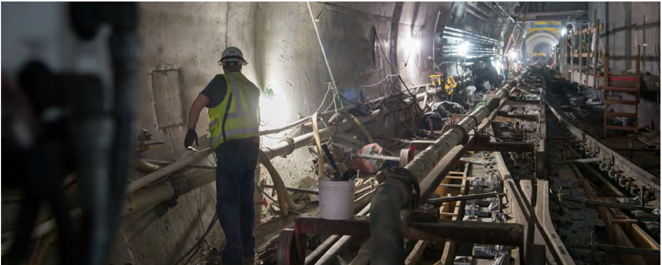
A worker carefully pulls an electrical cord along the west wall of the Chinatown Station platform cavern, as part of systems and utility installation work.
