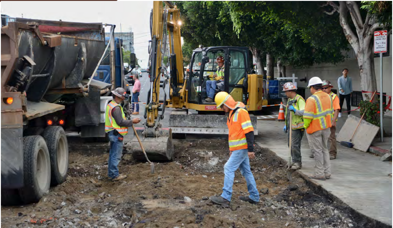
Workers carefully excavate around existing utility access manholes at the southeast corner of 4th and Brannan, where roadway restoration and repaving are underway.
