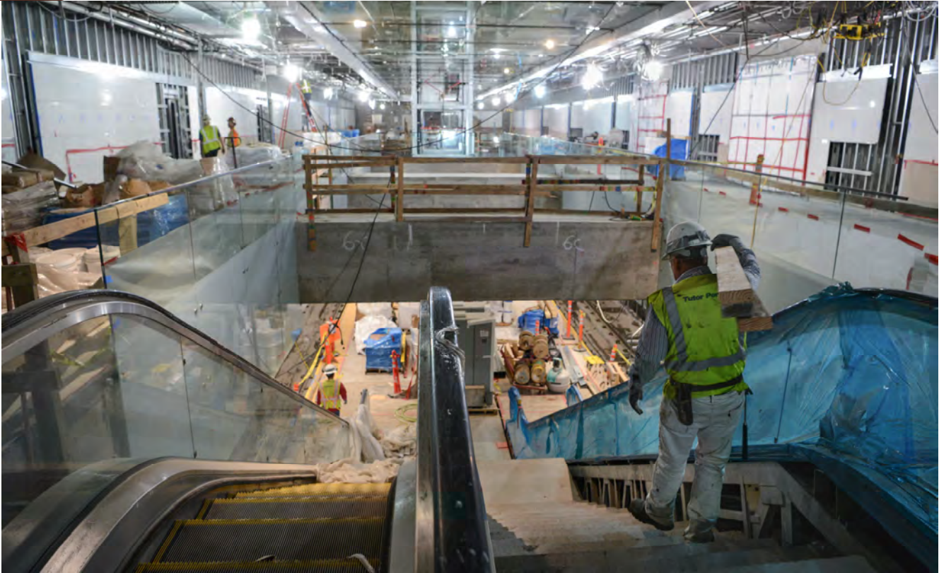
A worker hauls 2x4s from the concourse level down to the station platform inside Yerba Buena/Moscone Station.
