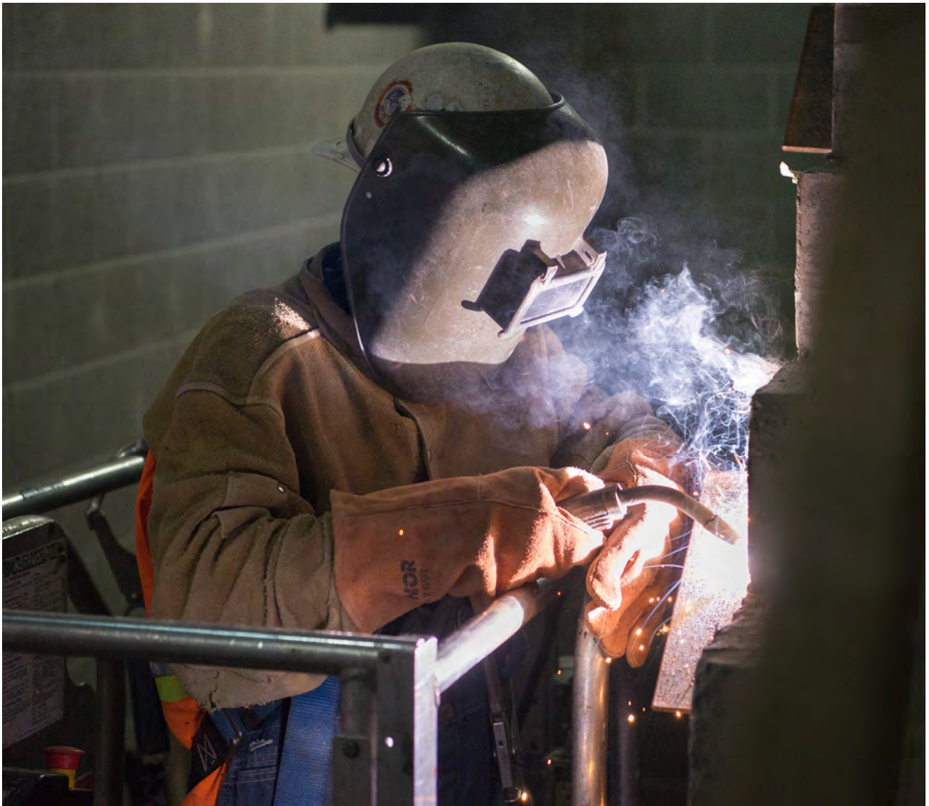
A welder attaches brackets to the side of the south staircase inside Union Square/Market Street Station, to prepare for the installation of escalators.
