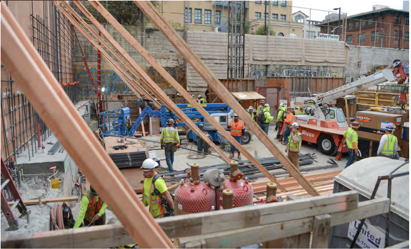
Massive wooden reinforcements temporarily hold up formwork as part of reinforced concrete wall construction at the south end of Chinatown Station's street-level entrance.
