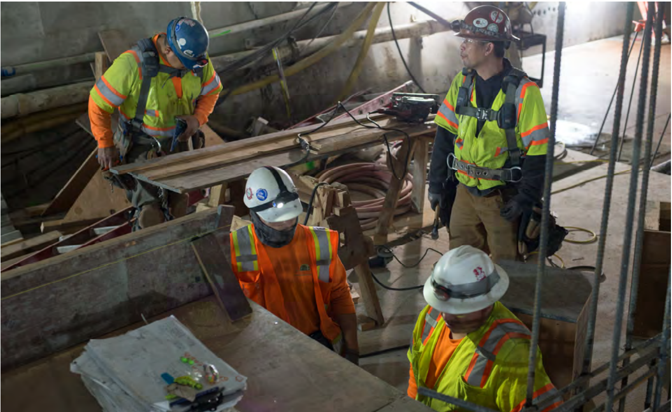
Carpenters and other laborers cross paths at the edge of the Chinatown Station platform along the future southbound track side.
