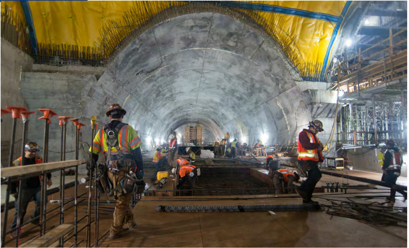
Teams work feverishly to construct the platform level of Chinatown Station, seen looking south from the cross-cut cavern under the Washington and Stockton intersection.
