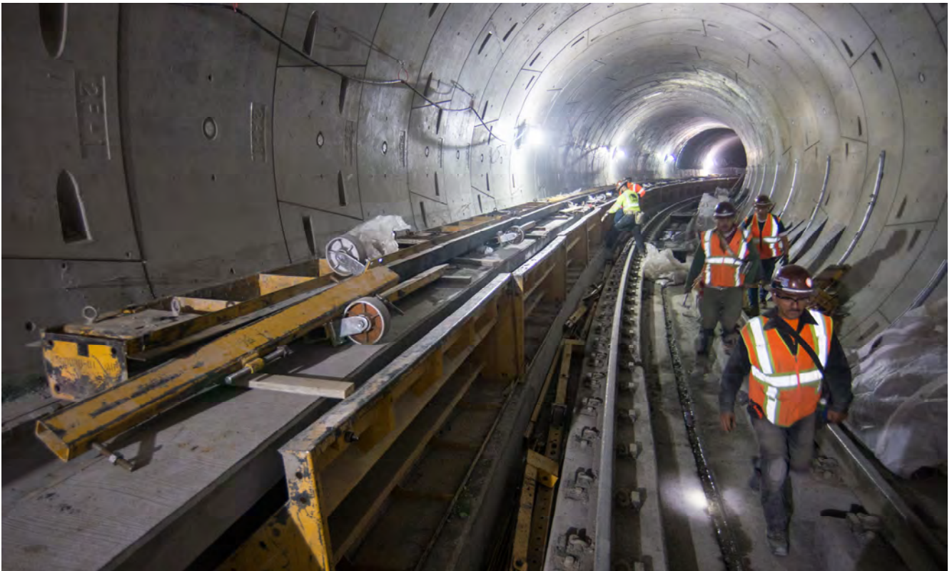
A crew moves sections of steel concrete forms used to construct tunnel walkway segments inside the northbound tunnel as it approaches Union Square/Market Street Station.
