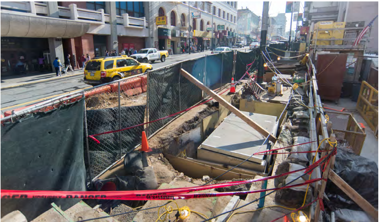
New utility vaults are being installed along the west side of Stockton adjacent to the Chinatown Station headhouse site.
