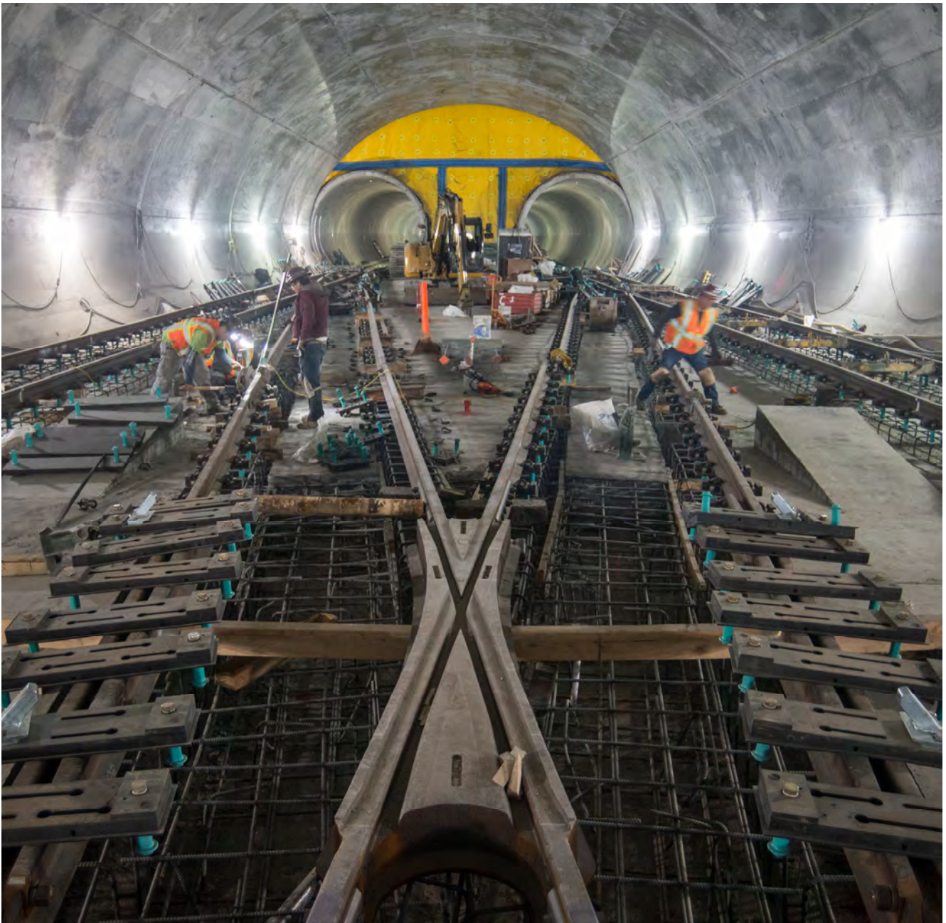
Crews are wrapping up installing rail sections for the massive track crossover just south of the future Chinatown Station platform cavern.
