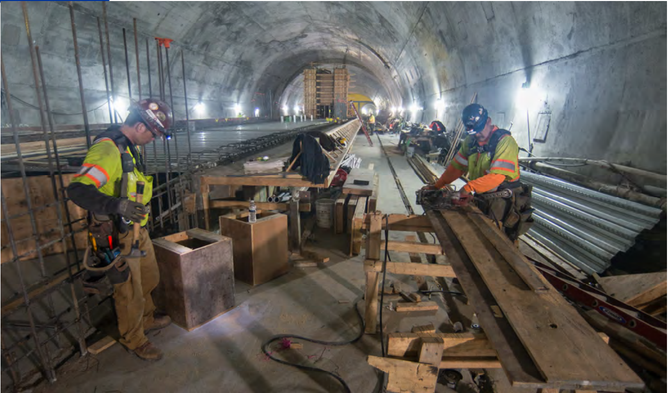
Carpenters build sections of concrete forms as part of Chinatown Station platform construction.
