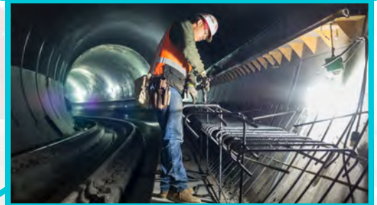
4th St. Surface Track, Systems (STS)
