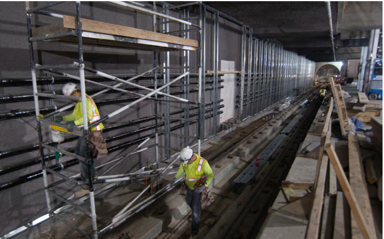
Steel studs for a furring wall are being installed along the southbound side of the Yerba Buena/Moscone Station platform.
