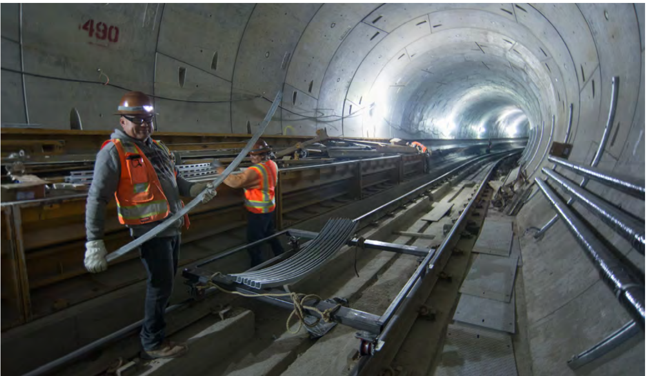
Steel struts used to mount utility conduits to the tunnel walls are unloaded from a rolling dolly inside the northbound tunnel at the Market Street S-curve.
