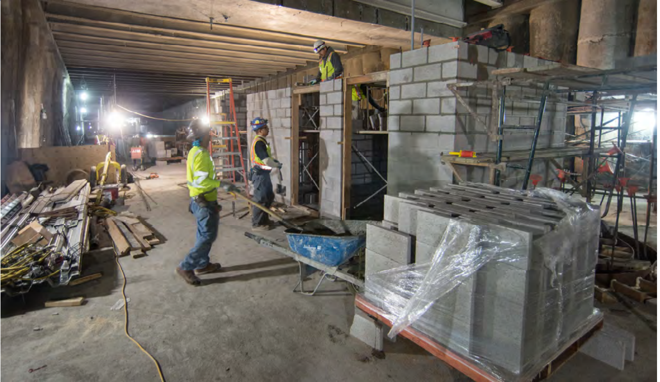
A crew on the mezzanine level of the Union Square/Market Street Station assembles interior cinderblock walls under the intersection at Stockton and O'Farrell.
