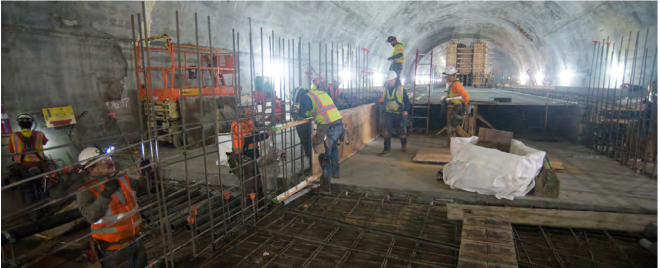
Looking south inside the platform cavern where it meets the cross-cut cavern, a crew assembles a rebar cage for a portion of the Chinatown Station platform.
