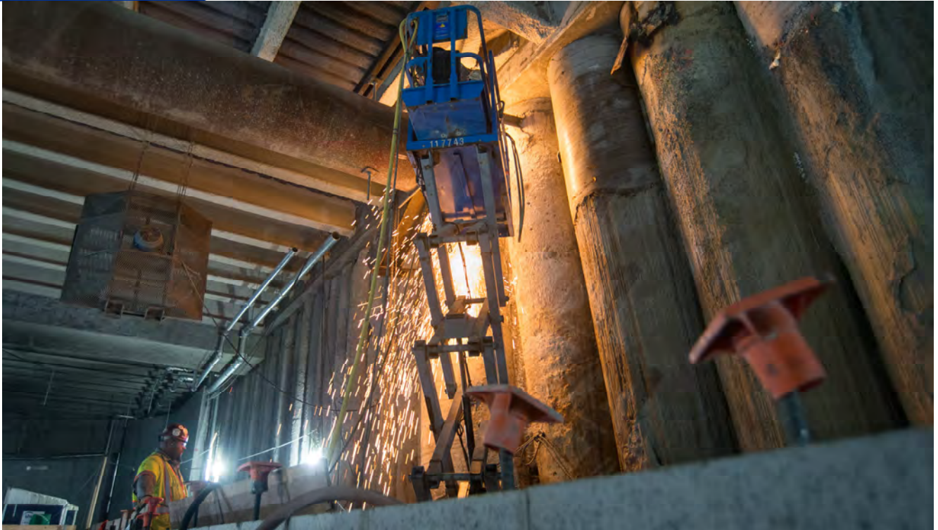
A shower of sparks falls from a scissor lift under the intersection at Stockton and Geary as workers continue removing extraneous reinforcing and prepare the interior for permanent structural elements.
