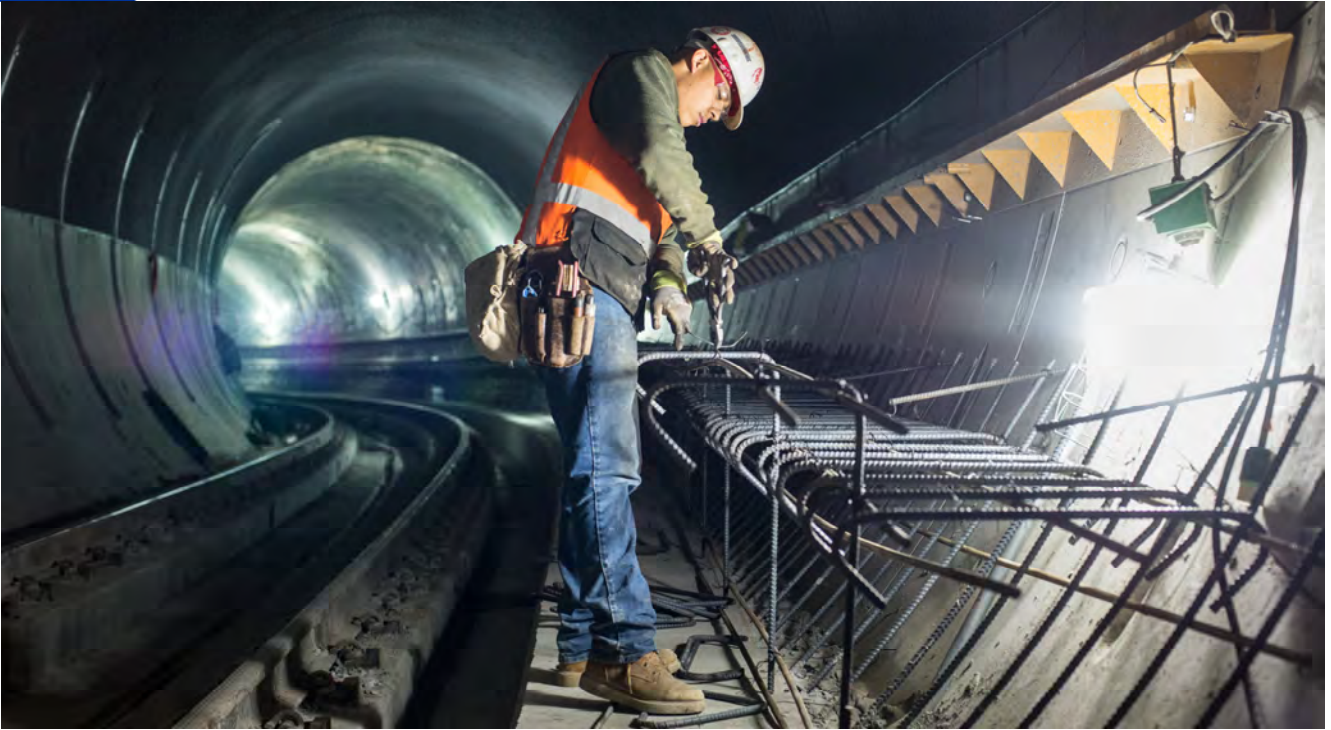
A worker ties sections of rebar together with wire as part of tunnel walkway construction in the northbound tunnel just south of the Union Square/Market Street Station platform.
