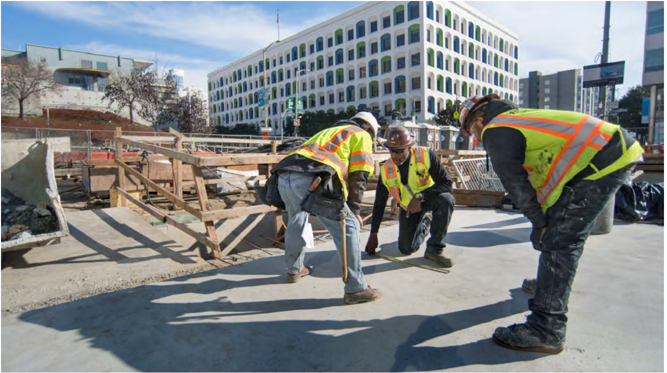
A supervisor gives instruction atop the Yerba Buena/Moscone Station headhouse at the corner of 4th and Folsom.
