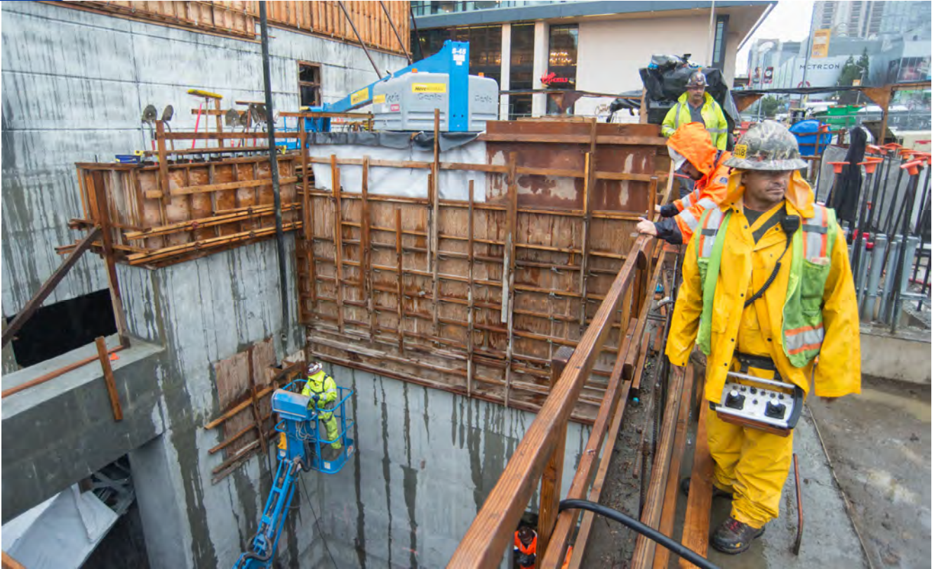
Rain or shine, a crew coordinates pumping concrete from a boom pump into sections of wall near the roof slab of the Yerba Buena/Moscone Station headhouse.
