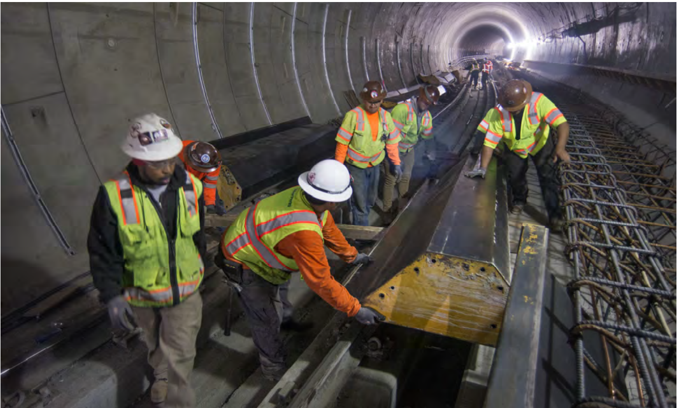
A crew places sections of steel formwork ahead of pouring concrete for a new section of elevated tunnel walkway.
