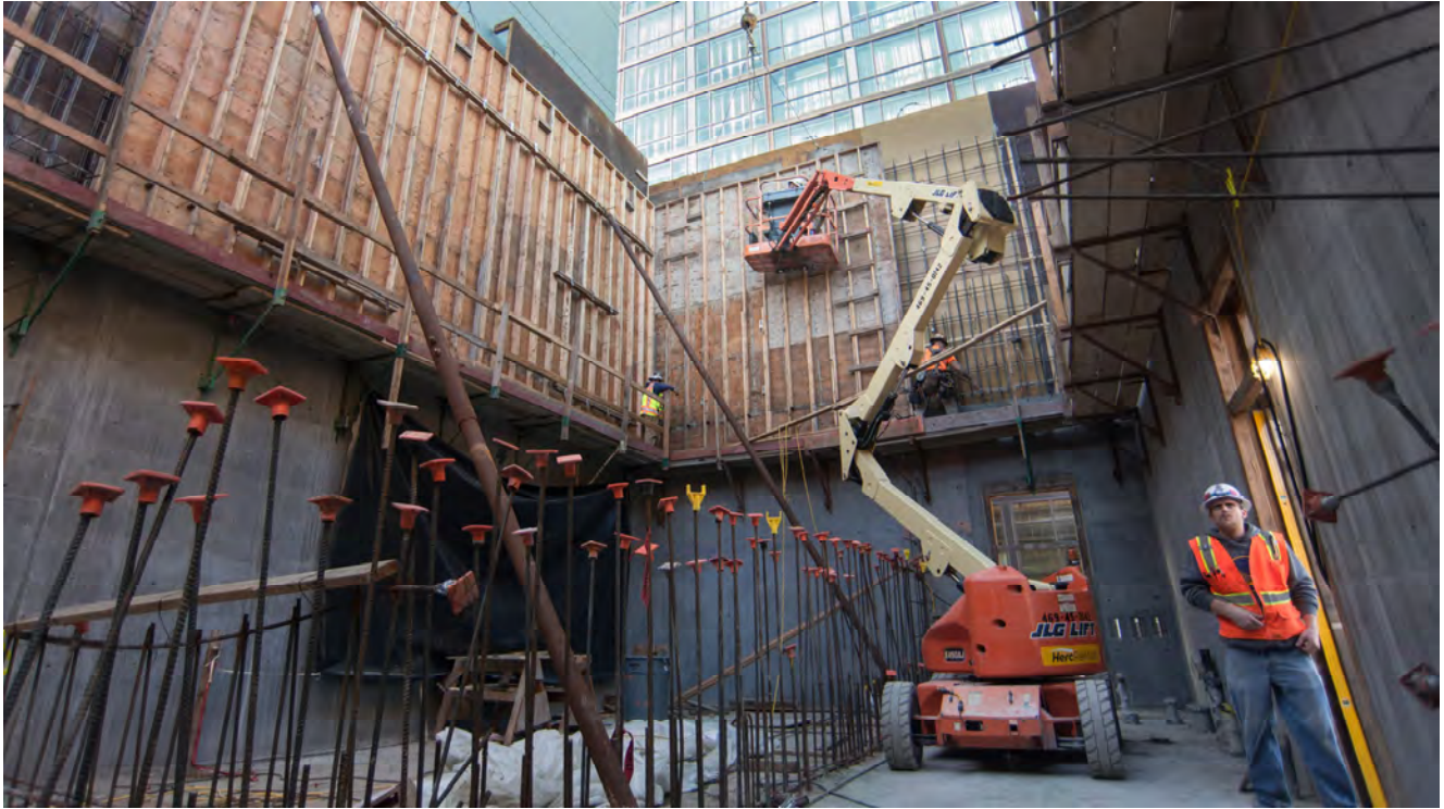
Formwork continues going up to build the next level of a large headhouse ventilation structure adjacent to Clementina Alley.
