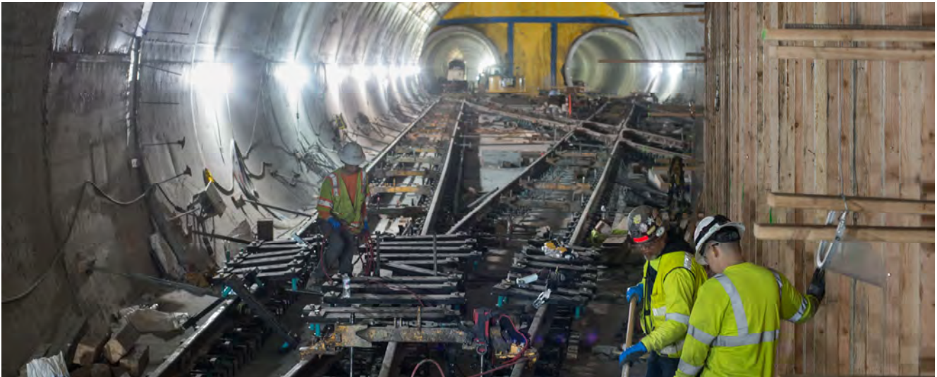
Clamps, spacers, and other equipment are used to move sections of rail into permanent position at the southern end of the Chinatown Station platform cavern.
