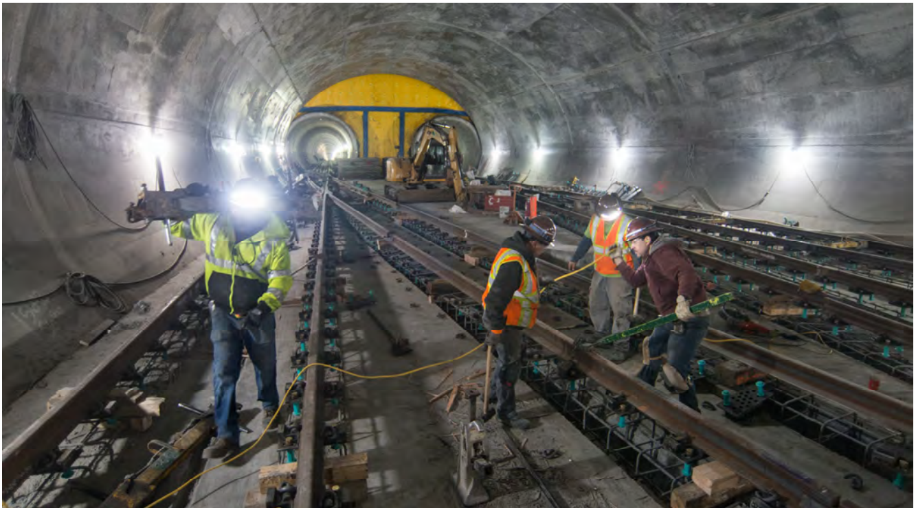
Workers use leverage, clamps, and adjustable spacers to precisely place sections of rail inside the Chinatown track crossover cavern.
