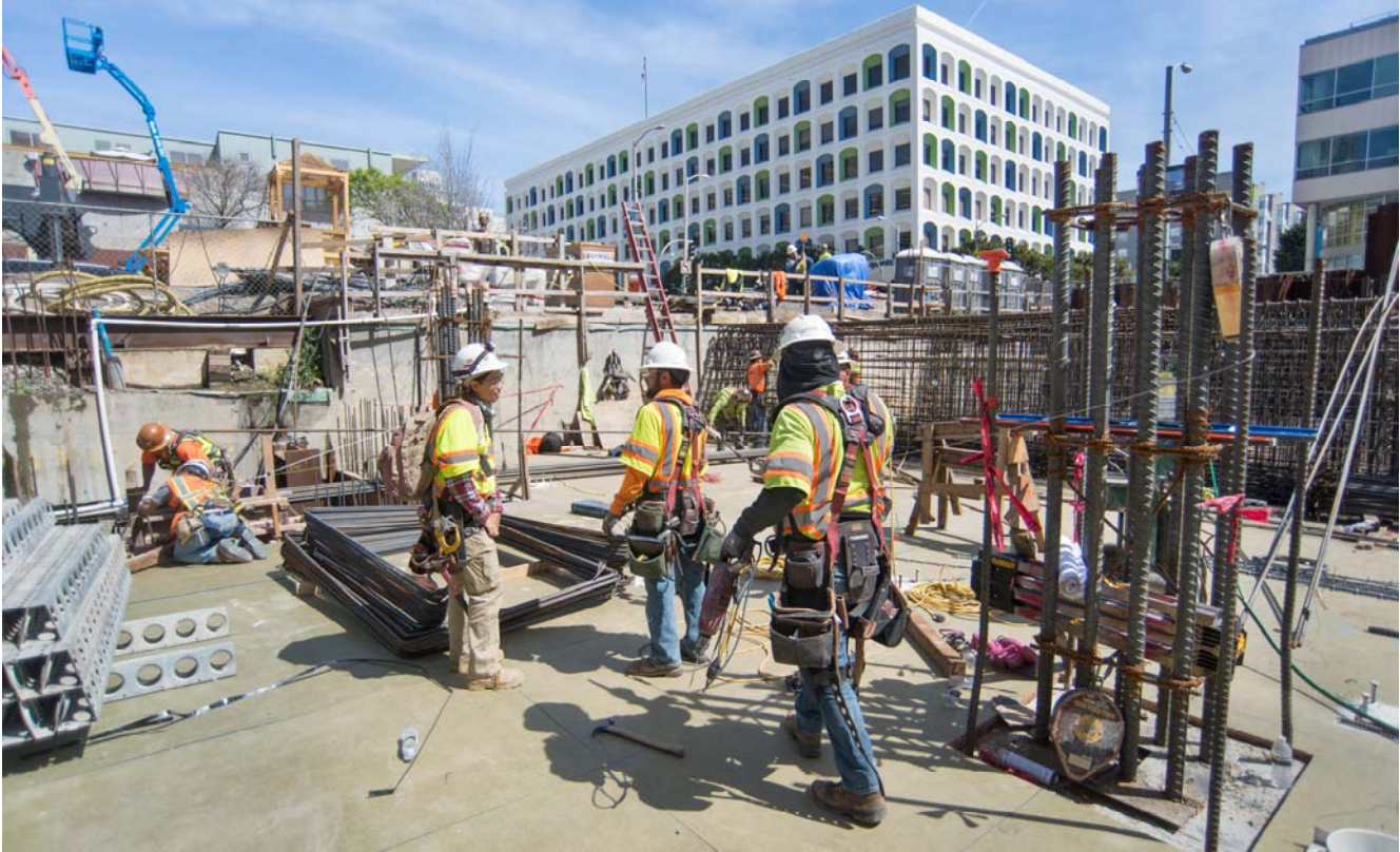
Large gauge rebar extends skyward from inside the future roof deck of the Yerba Buena/Moscone Station headhouse, which may be used as a structural foundation for future transit-oriented development.
