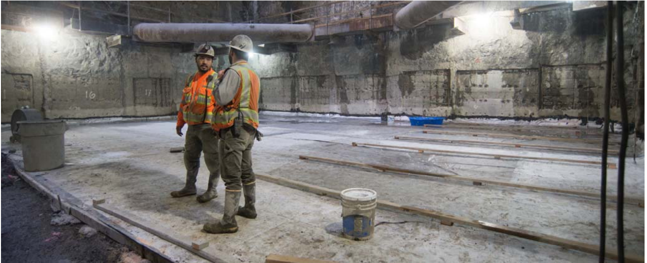
Vinyl sheeting, part of the waterproofing system used throughout station construction, has been laid atop an initial concrete slab at the south end of the Chinatown Station headhouse.
