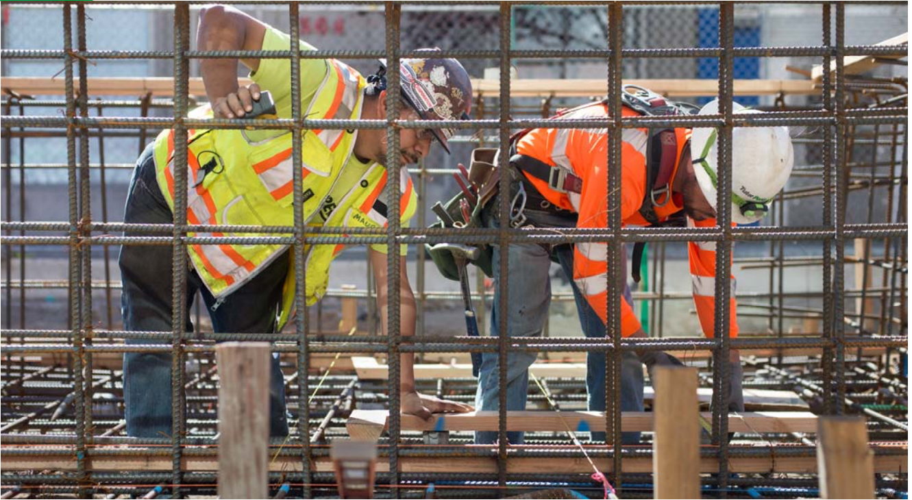
Carpenters install formwork and utility conduits inside the 4th and Brannan surface station's platform foundation rebar cage.
