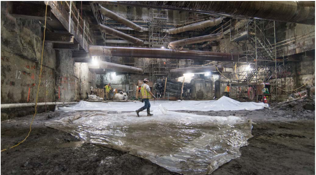
A crew lays out huge sheets of plastic sheeting during a rainstorm to reduce mud at the bottom of the Chinatown Station headhouse.
