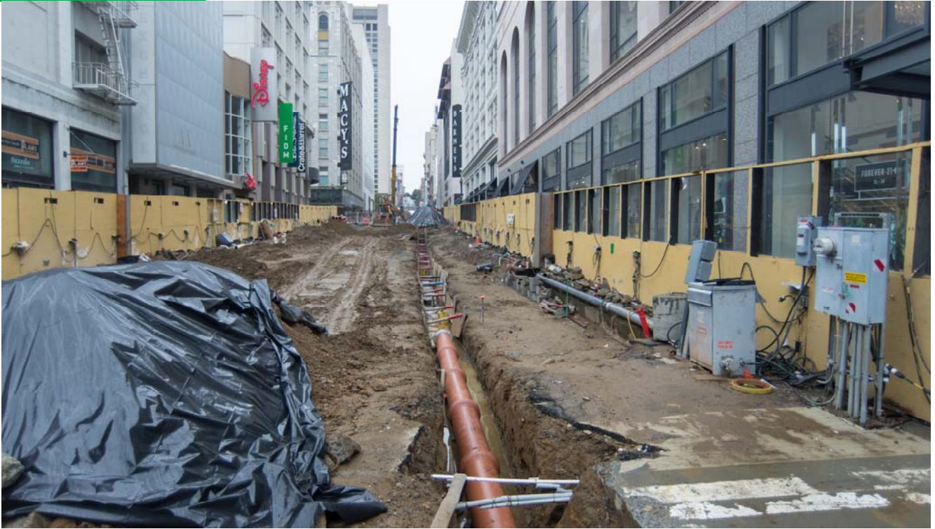
New sections of sewer pipe have been placed in a trench along the east side of Stockton between Ellis and O'Farrell as part of the initial stages of street restoration work.
