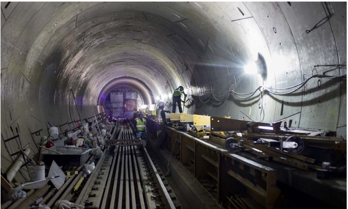
Reinforced concrete walkways along the inner sides of the twin subway tunnels are being constructed one section at a time going north.
