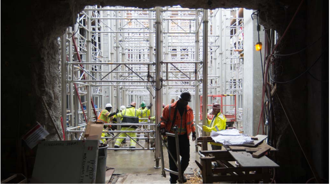
Large, complex sections of scaffolding are carefully positioned into place atop the concourse level floor slab inside the station headhouse.
