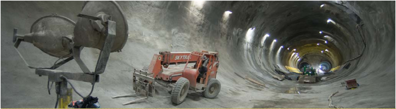
Looking south from just south of Washington Street, the Chinatown Station platform cavern has been fully excavated, and work to install waterproofing has begun.
