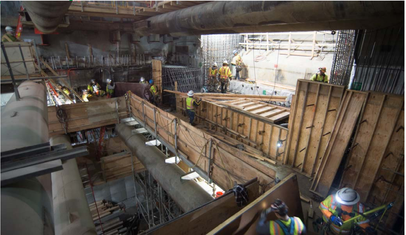
Huge concrete forms are assembled at the south headwall of the Union Square/Market Street Station, as part of interior wall and escalator footing construction.
