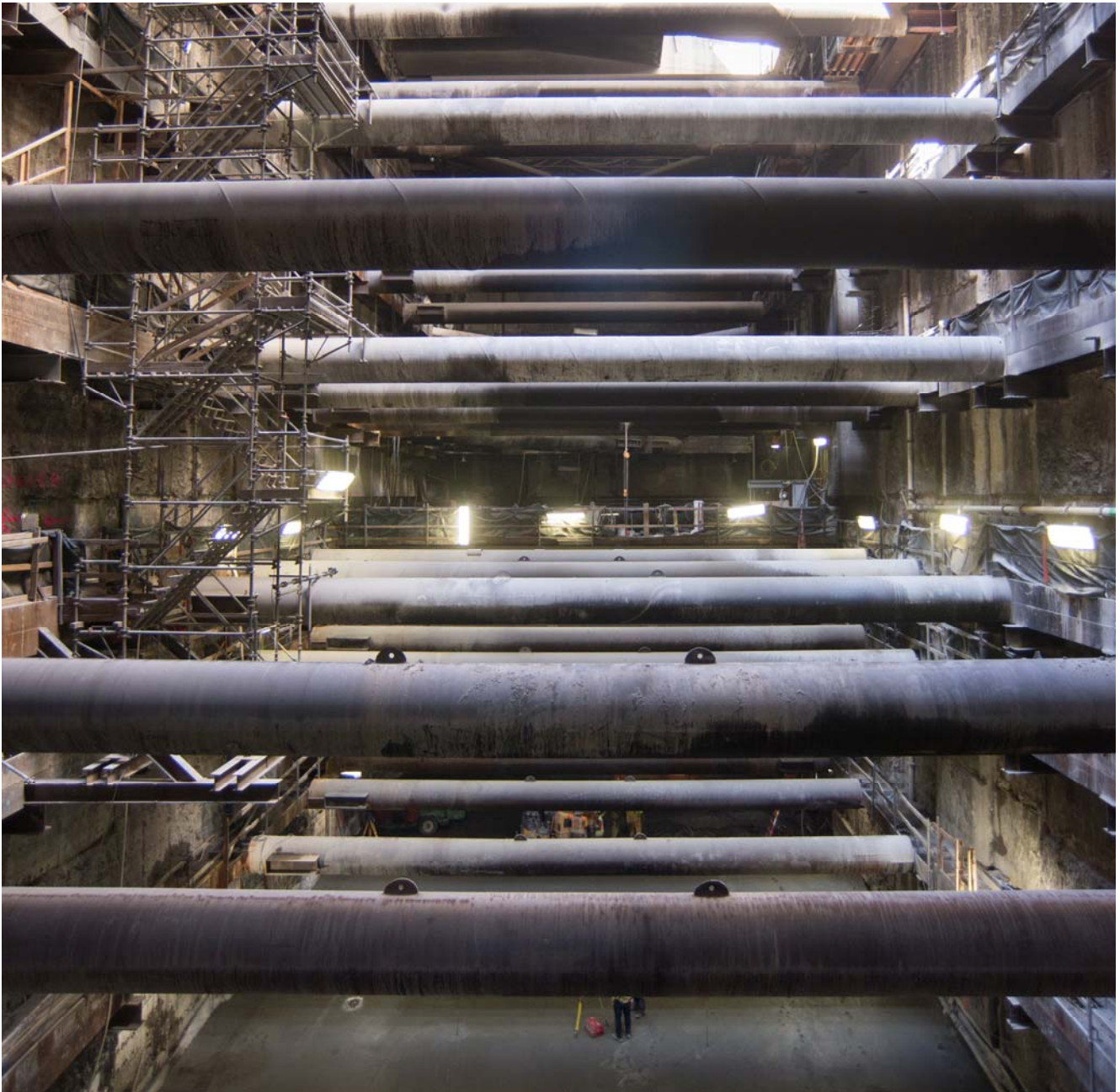
Seemingly endless levels of struts span the width of the Chinatown Station headhouse, looking north from a third of the way up the access staircase.
