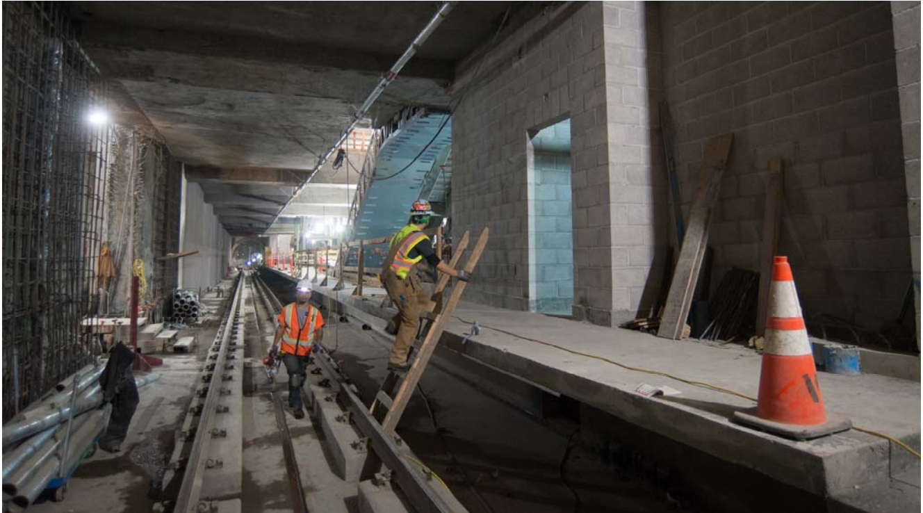
Two men climb up to the station platform from the southbound track area at the south end of the station box. Interior walls and utilities are being installed in the portions of the station already built.
