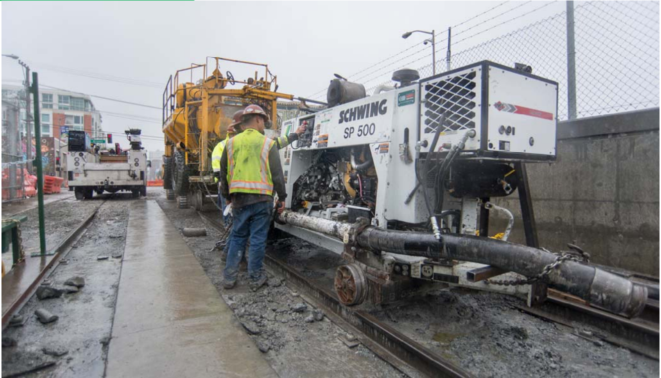
Workers tend to a concrete pump at the top of the tunnel portal at Bryant Street during a heavy rain.
