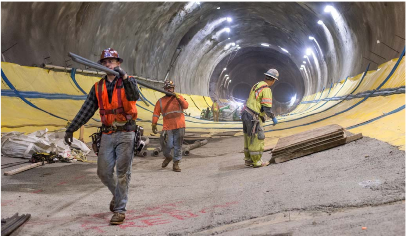
Workers pass back and forth up and down the station cavern, carrying strands of rebar from their delivery area a hundred yards to the north.
