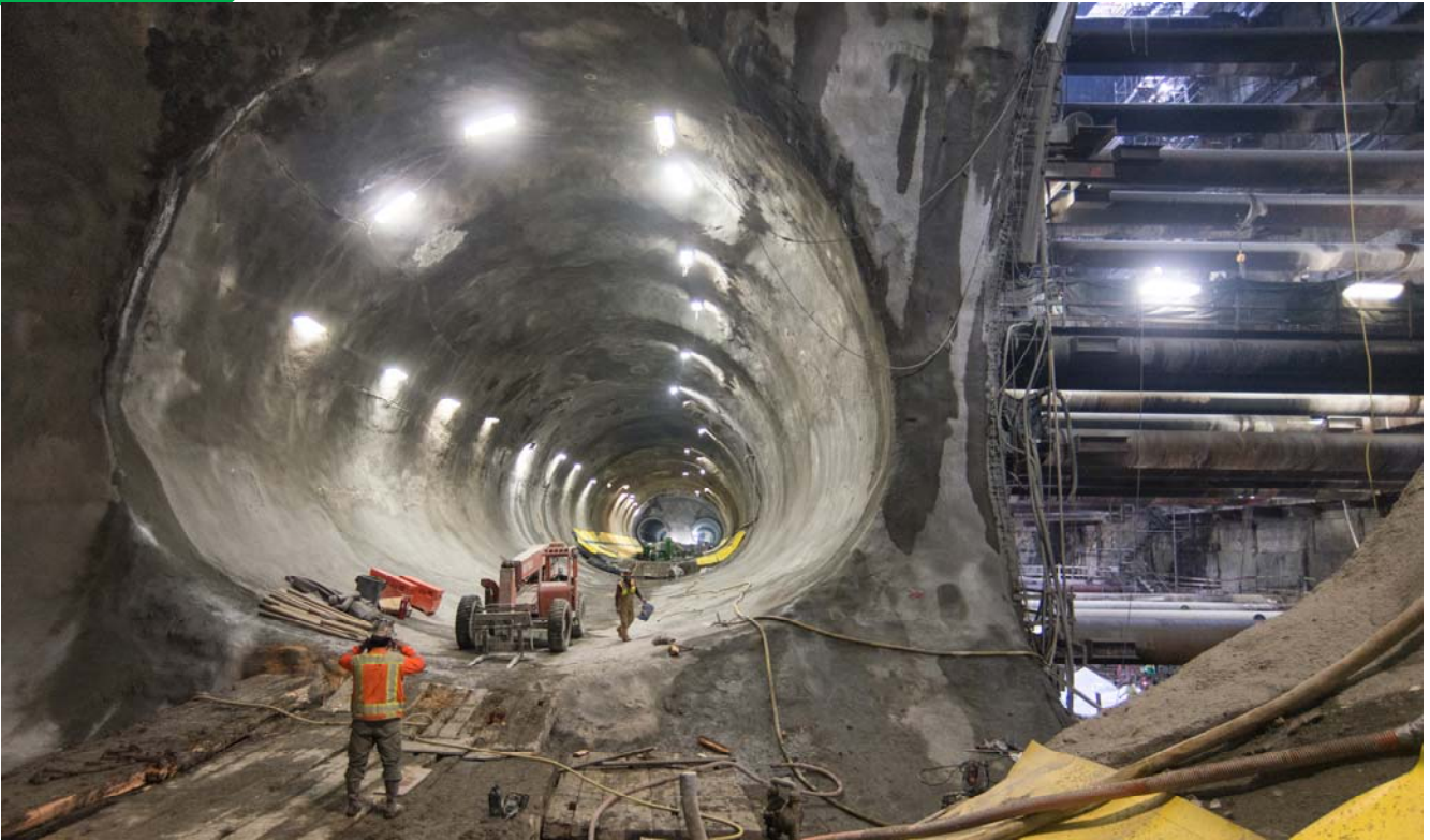
The massive shell of the Chinatown Station platform cavern and part of the curved cross-cut cavern entrance from the headhouse can be seen looking south from the edge of the north cavern.
