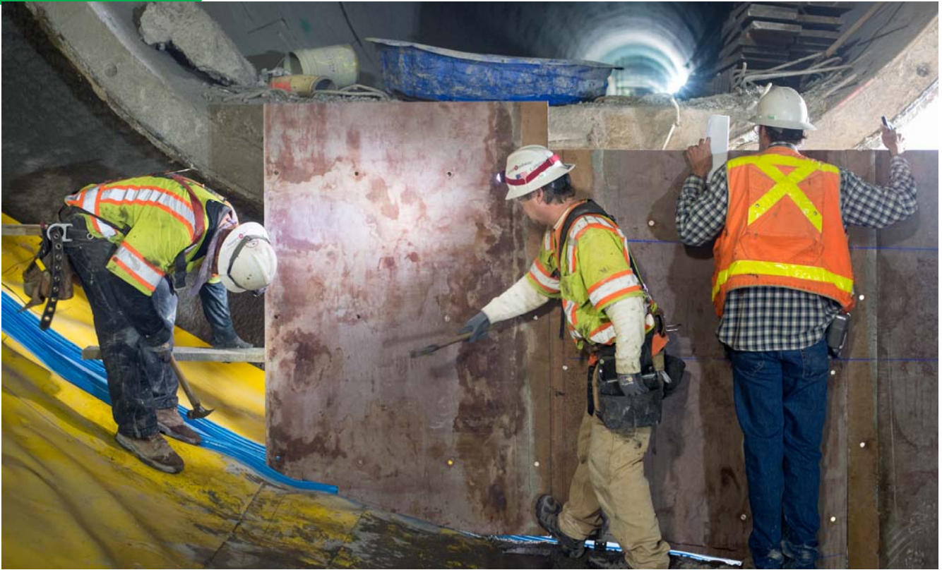
Carpenters assemble portions of framing for concrete forms at the south end of the Chintown Station track crossover cavern.
