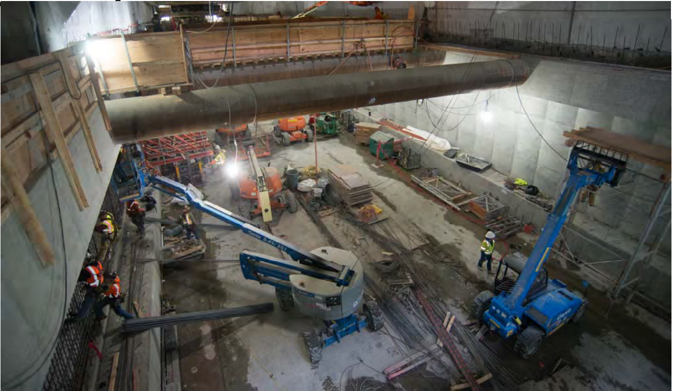
Looking south, workers continue constructing scalloped finish walls on the platform level of the station box, while vinyl sheeting is installed as part of waterproofing work above.
