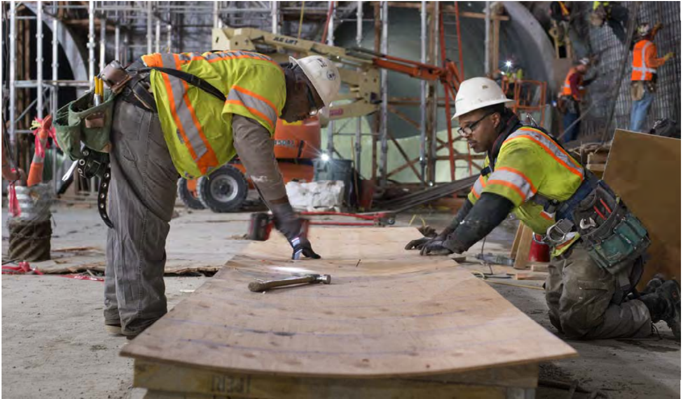
Carpenters build a concrete form near the south headwall as part of construction for scalloped wall texturing down the length of the station platform.
