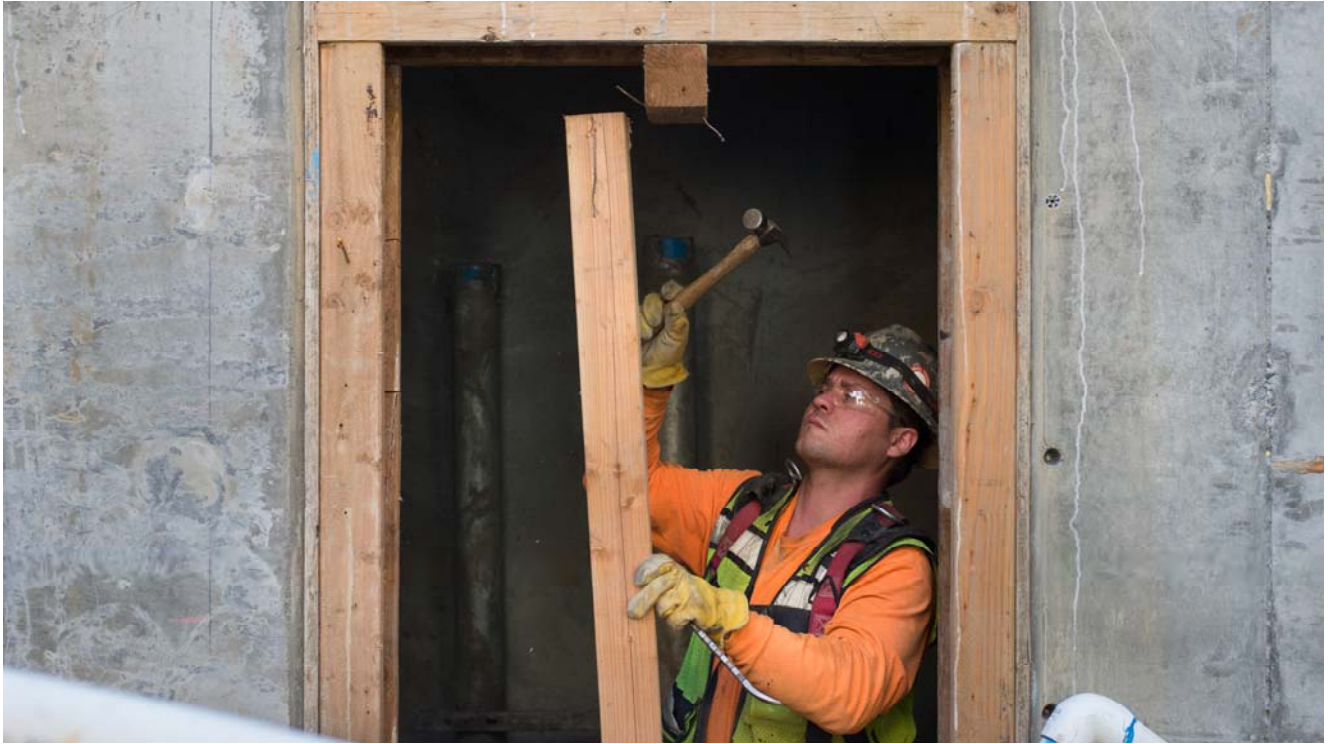
A carpenter removes pieces of concrete formwork for a doorway on the west side of the Yerba Buena/Moscone Station's headhouse, concourse level.
