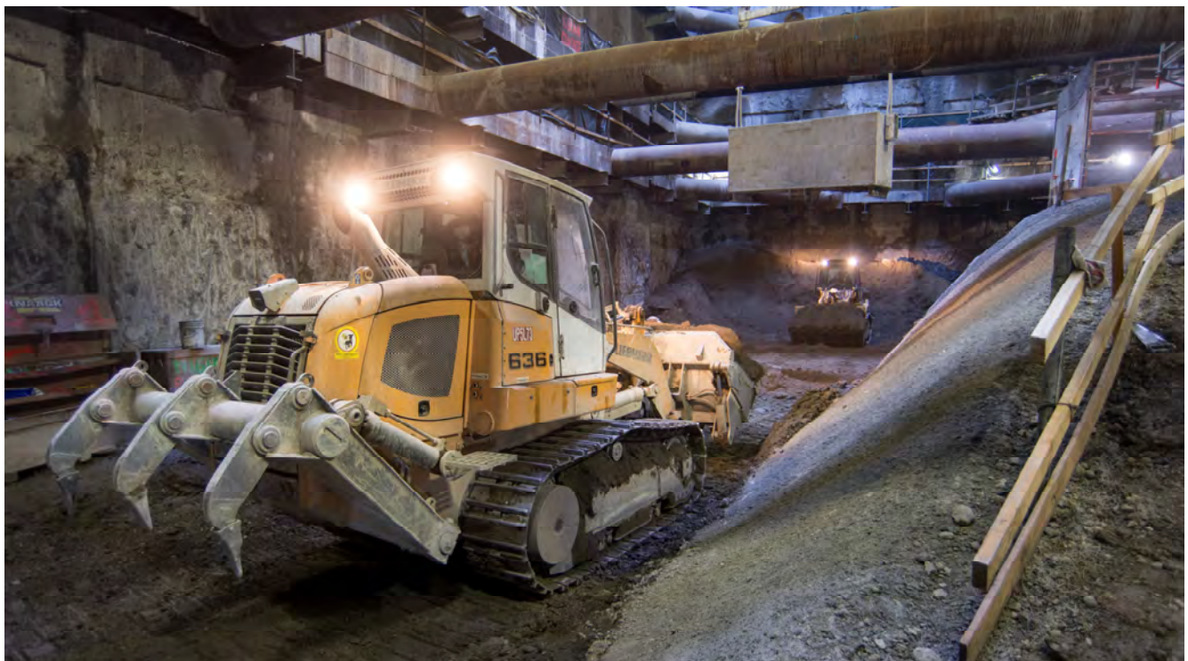
Bulldozers wait patiently as the large steel bucket used to haul excavated material to the surface is lowered into place inside the station headhouse.
