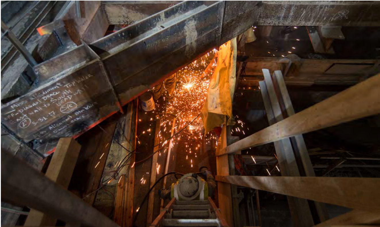
Sparks fly as a welder makes alterations to temporary bracing at the south headwall of the Union Square/Market Street Station, while an associate stands ready to periodically spray water with a hose to keep the heat down.
