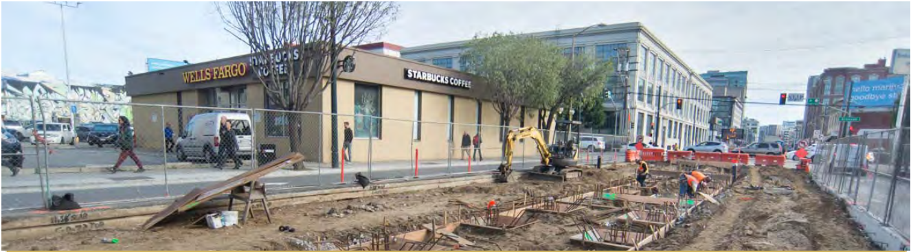
Surface station pile tie-in work continues, as workers install rebar and concrete forms for the next phase of 4th and Brannan Station construction.
