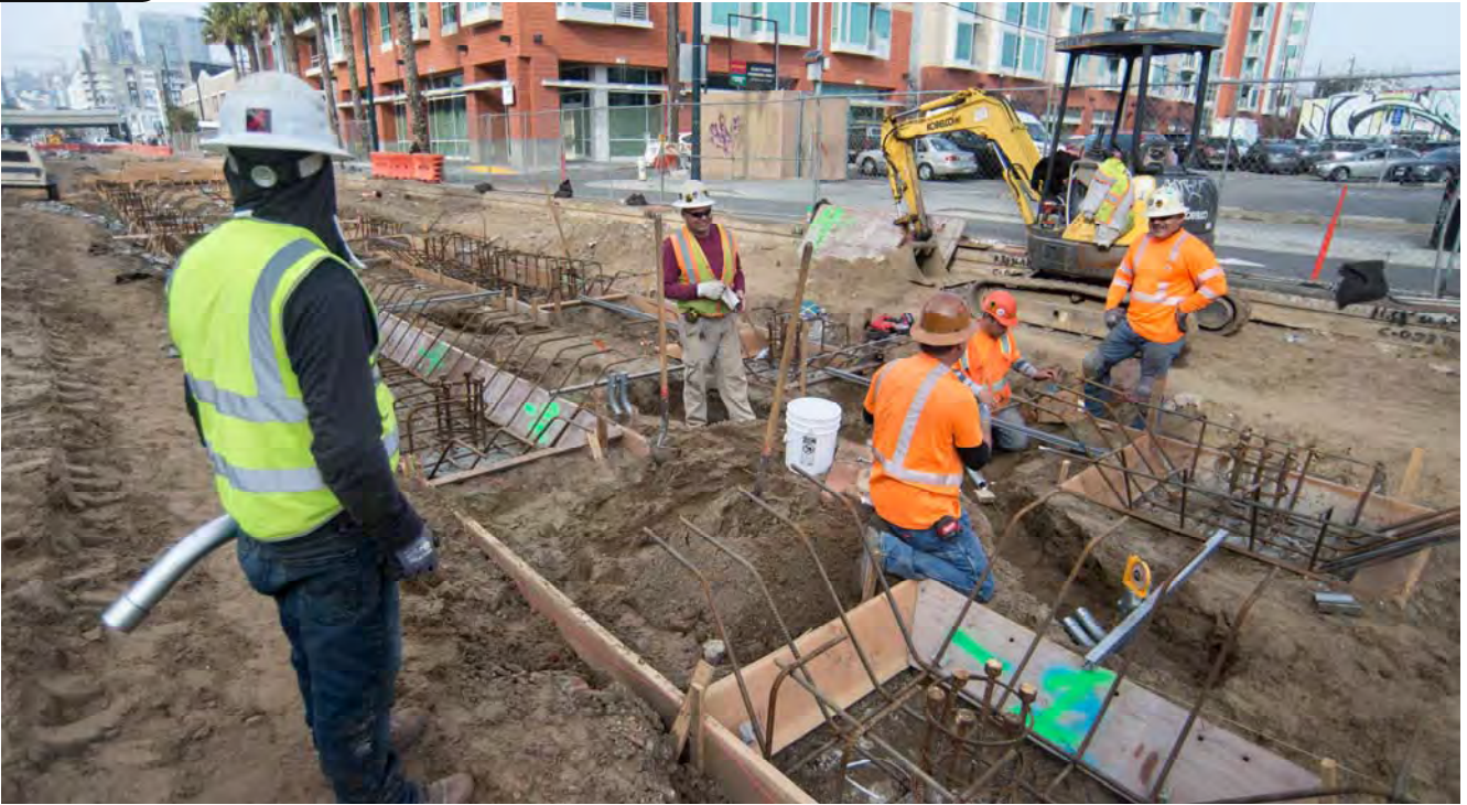
A crew attaches rebar to existing foundation piles as part of pile cap construction work for the 4th and Brannan Station platform.
