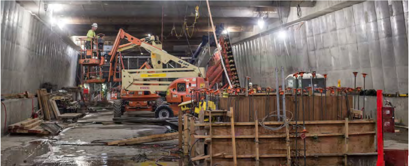
Looking south inside the Union Square/Market Street station box, crews are constructing concrete forms for internal structures, such as the north elevator shaft base in the foreground.
