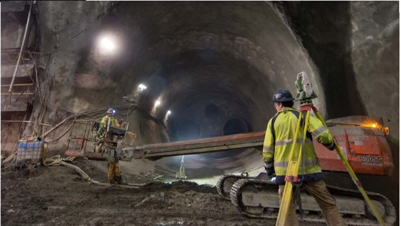
Looking north, a surveyor pauses while two men move a boom lift into position inside the cross-cut cavern, the where the station headhouse enters into the future station platform cavern, currently being excavated.
