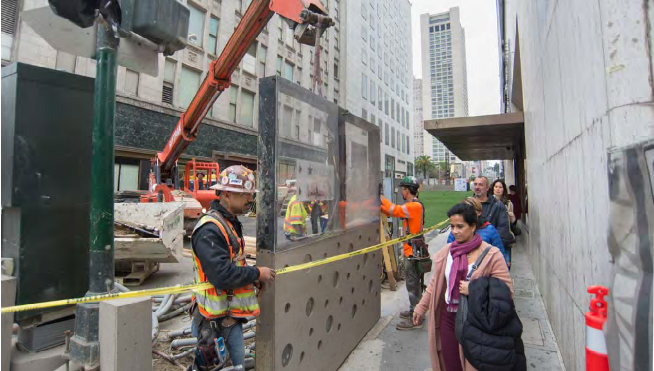
A crew re-installs the first section of pedestrian safety barrier on the east side of Stockton north of O'Farrell, following the end of the 2017 Winter Walk
