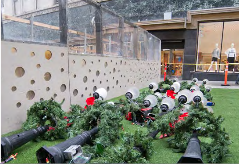
1 Decorative elements, as well as the green turf, are removed and stored
