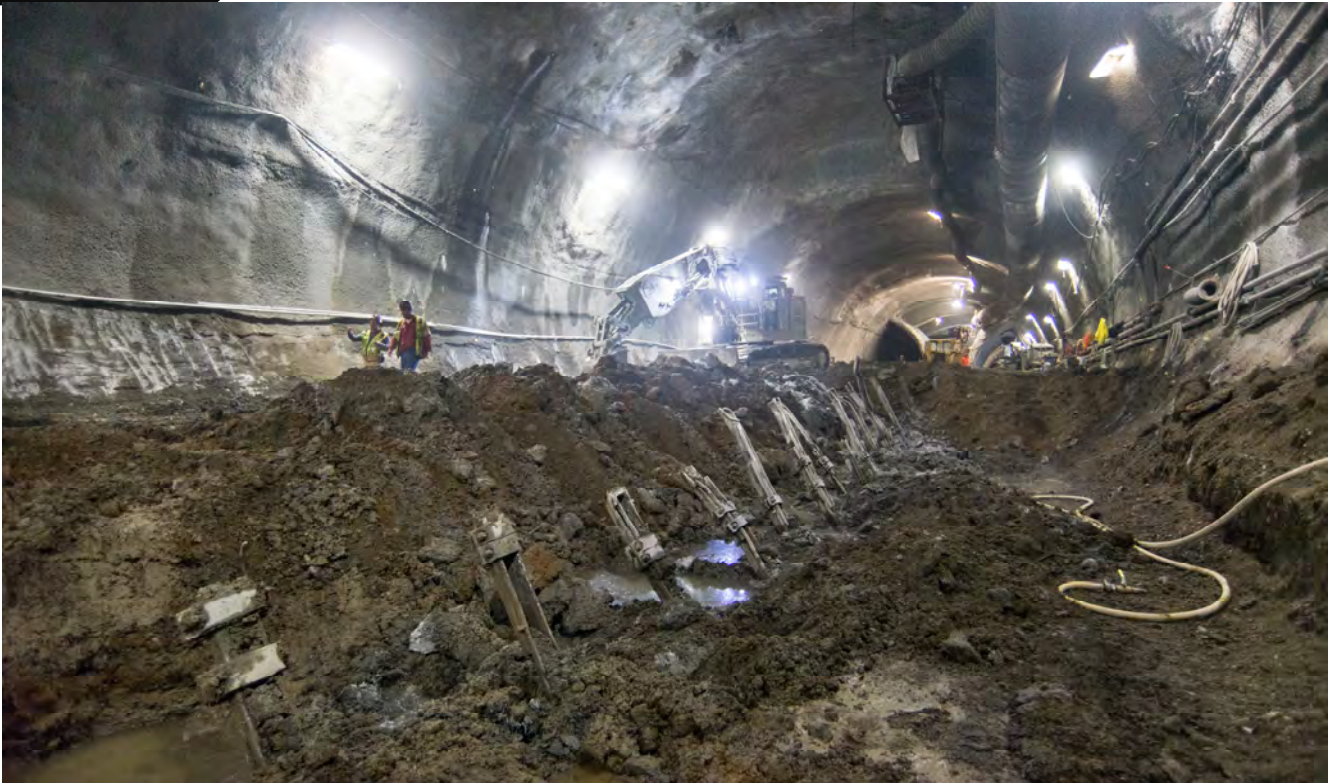
Looking south, steel support ribs which formerly reinforced a wall constructed as part of sequential mining work jut from the soil being excavated inside the Chinatown Station.
