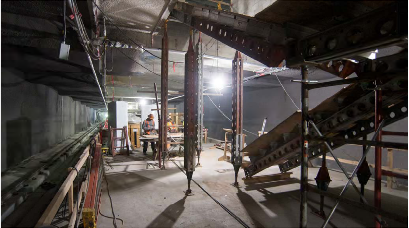
Carpenters build concrete forms toward the north end of the Yerba Buena/Moscone Station platform, where internal walls and other structural elements are being constructed.
