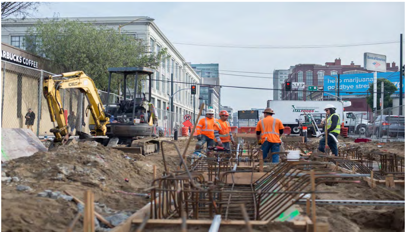
Looking south from 4th and Freelon, crews are installing conduit for utilities as part of 4th and Brannan surface station foundation work.
