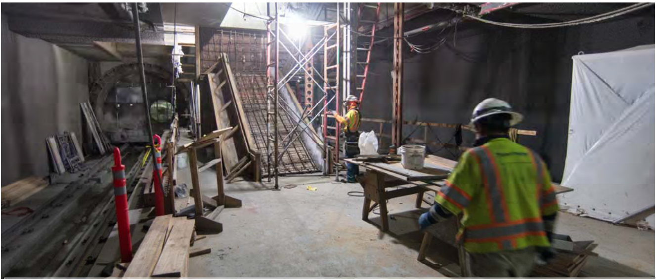
Scaffolding and concrete forms are being installed to construct a passenger staircase at the north end of the Yerba Buena/Moscone Station platform.
