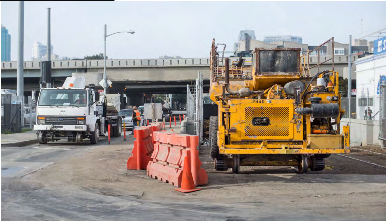
A utility vehicle fitted with rail wheels is moved from staging lot west of the tunnel portal, into the tunnel portal for support work.
