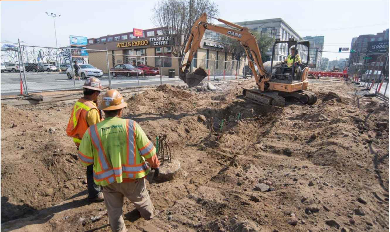
Workers are uncovering the tops of foundation piles as part of 4th and Brannan station platform work.
