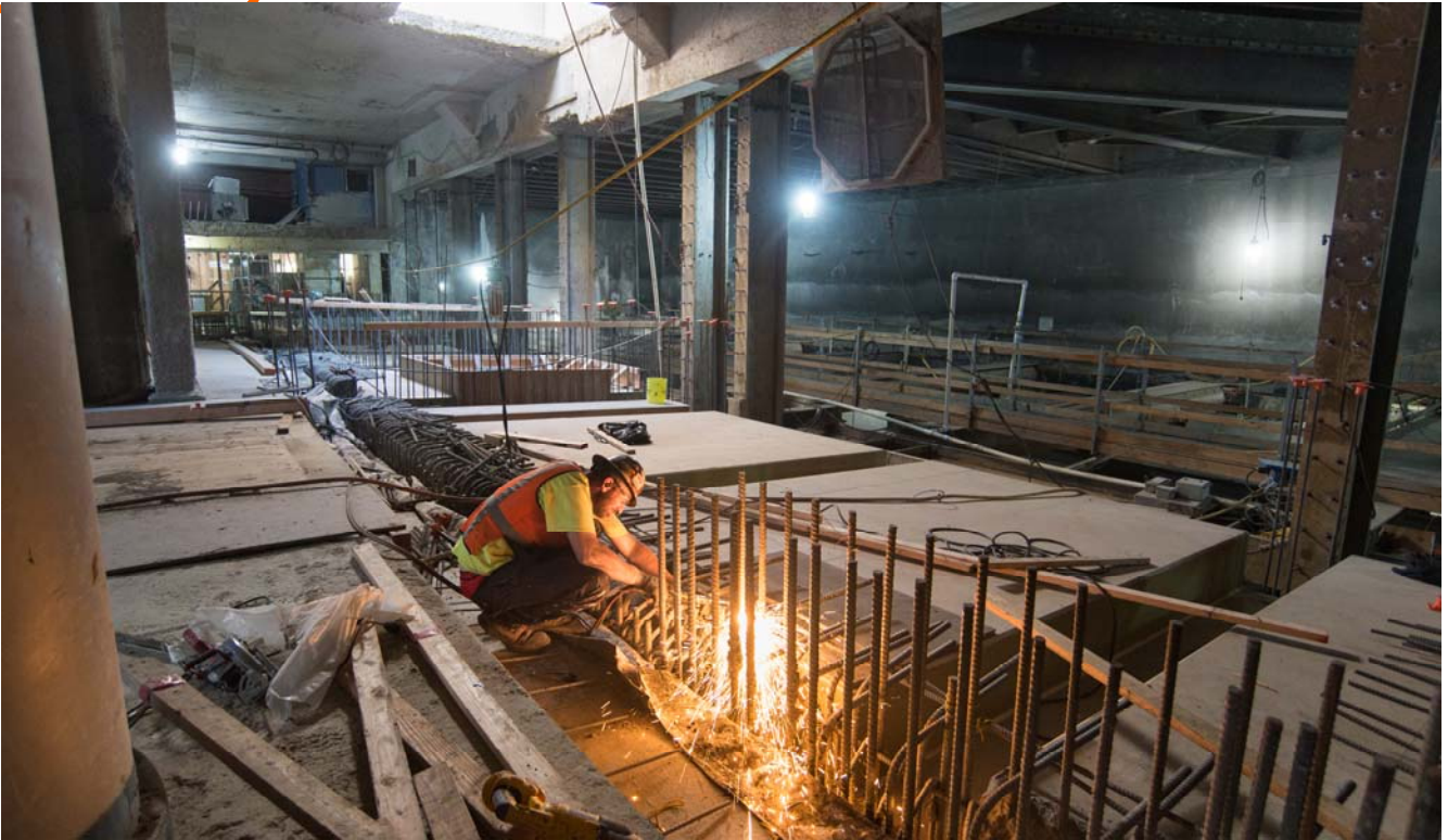
A welder cuts specific lengths of rebar to length inside the north concourse, where form-work for a two-level interior structure is being built.
