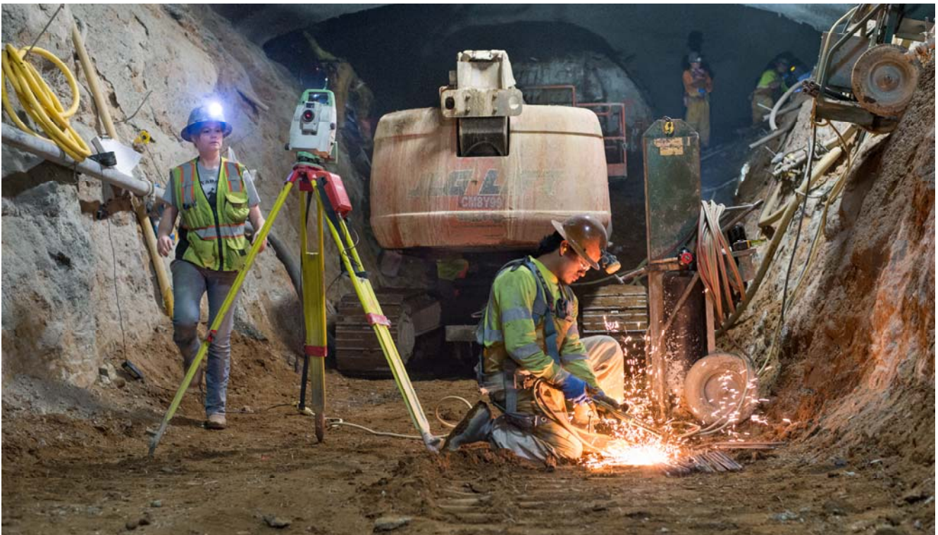
Pieces of rebar are cut to length inside the top heading of the north platform cavern as part of wall and ceiling reinforcing.
