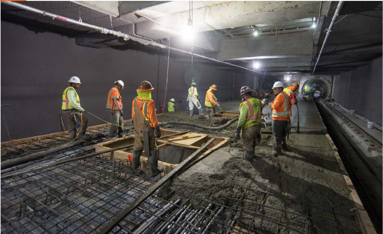
A crew pours concrete around future elevator footings inside the station box, as part of construction for the station platform.
