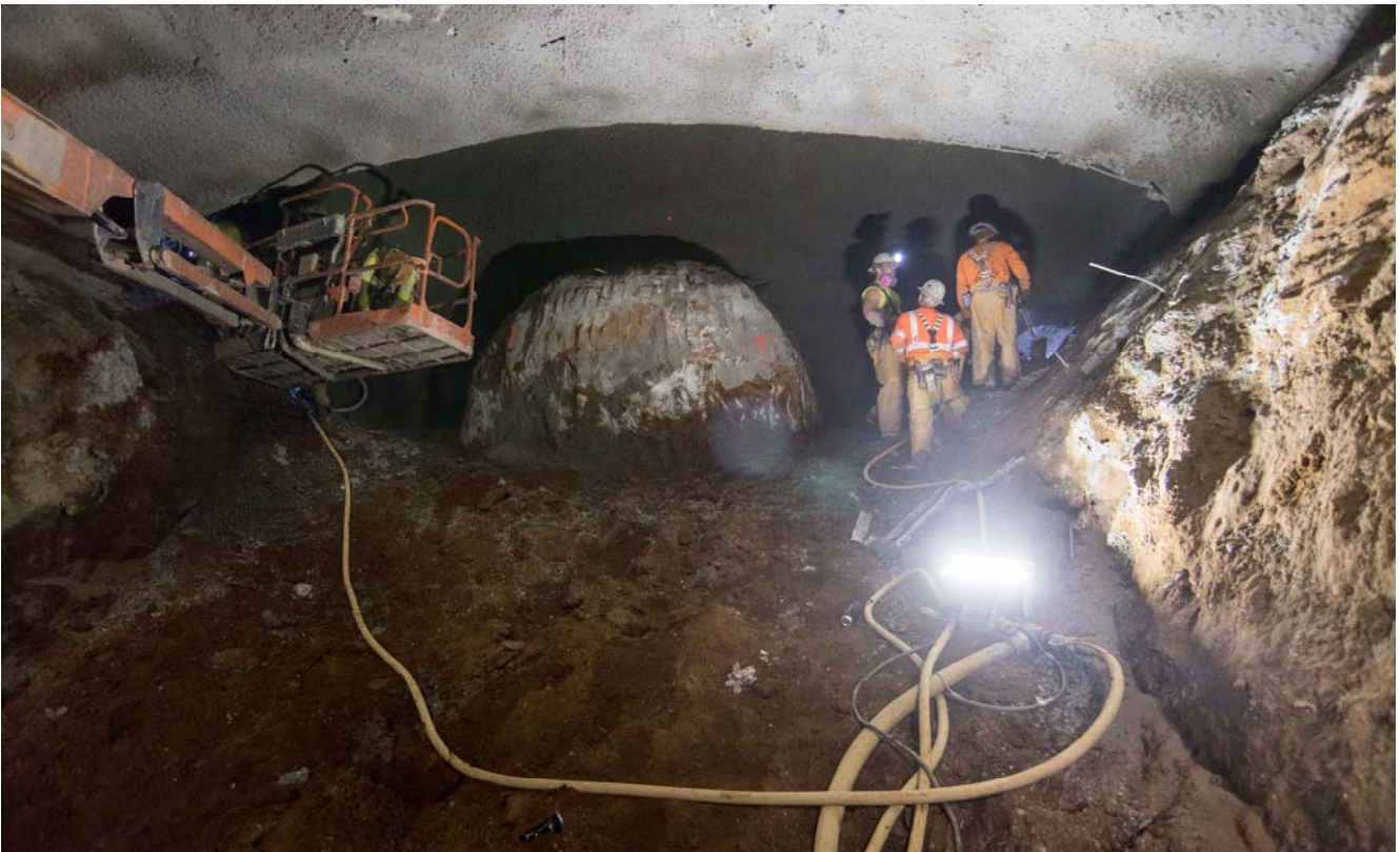
Crews excavating the top heading of the north platform cavern have uncovered (and since broken through) the reinforced shotcrete shell of the north egress shaft.
