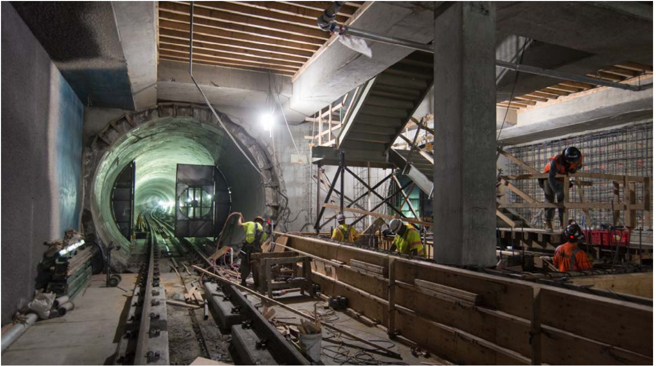
The curve of the northbound track entering the tunnel portal can be seen far in the distance, while workers construct final elements of the platform foundation rebar cage.
