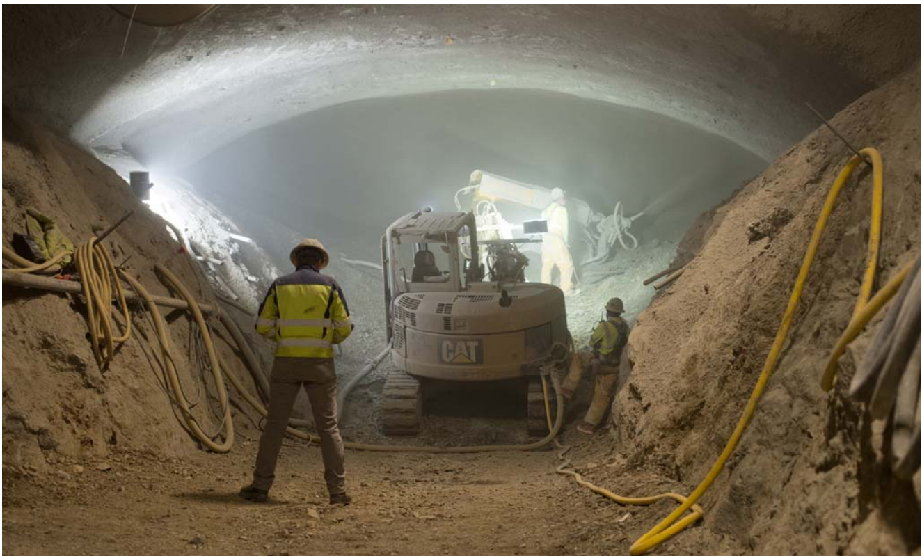
A tunneling engineer observes shotcrete spraying in the top heading for Chinatown Station's platform cavern.
