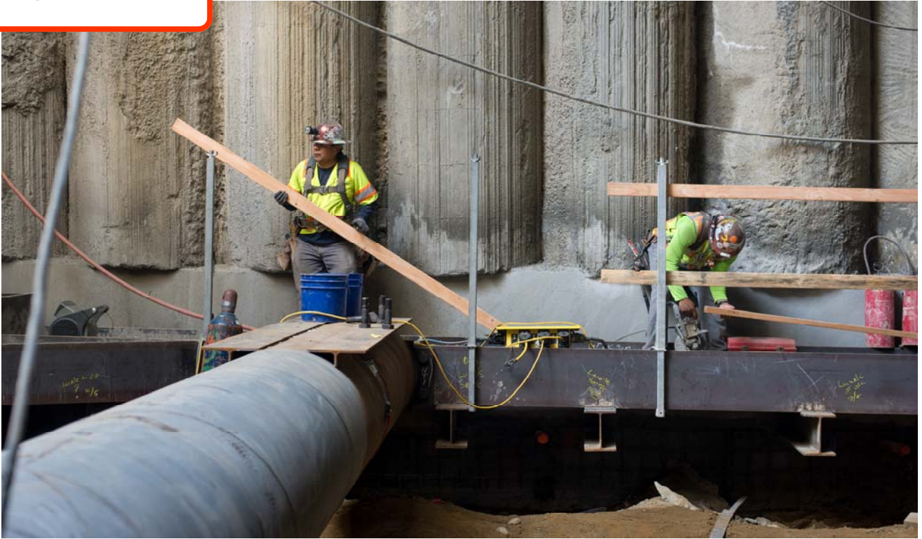
Workers erect safety railings atop large steel beams called walers inside the station box, where excavation is ongoing.
