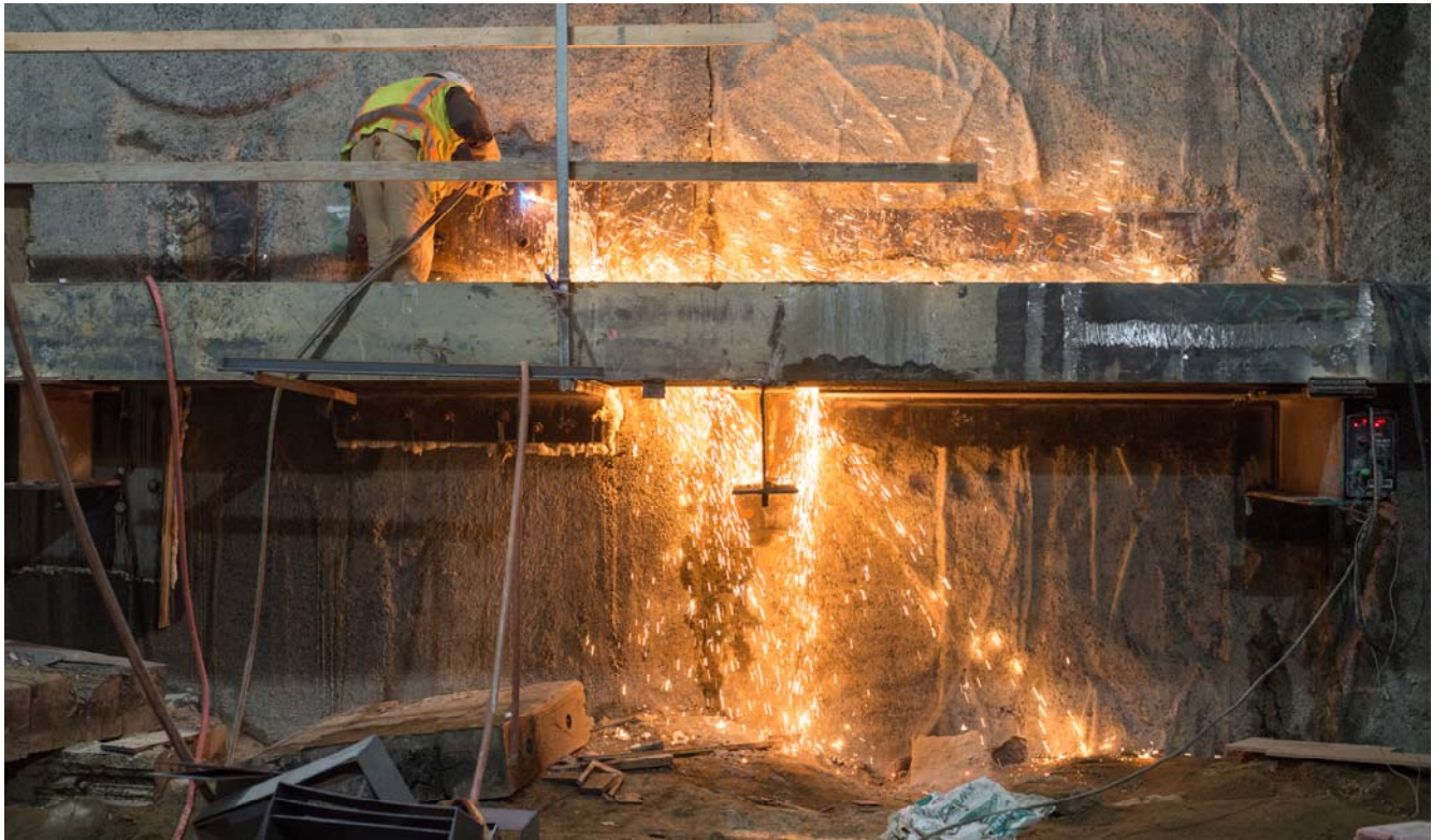
A shower of sparks fly as a worker adjusts the length of bolts holding steel brackets used to temporarily reinforce the outer station walls during excavation.
