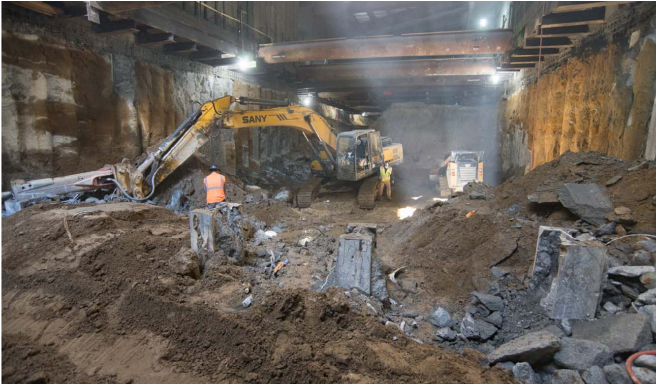
Light shines in the Geary access shaft, where steel beams used to reinforce the north headwall jut out of the soil like teeth. Crews recently removed the top few feet of the headwall to make room for future escalator footings and floor slab construction.
