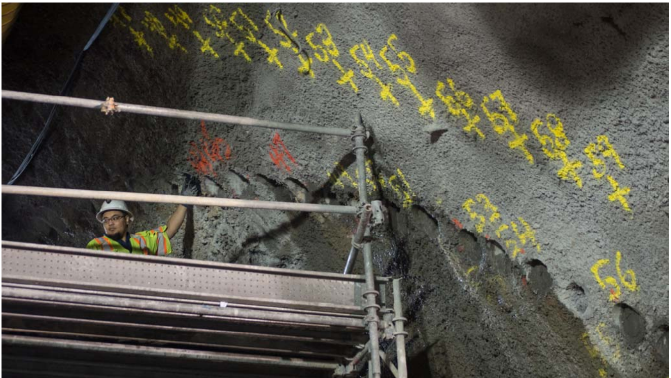
Survey markings on the shotcrete arch roof of the cross-cut cavern mark will aid drilling crews during station cavern roof construction.
