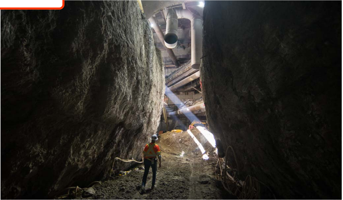
Curved shotcrete walls separating the center drift from the side drifts of the cross-cut cavern loom over workers excavating the invert or bottom of the worksite.
