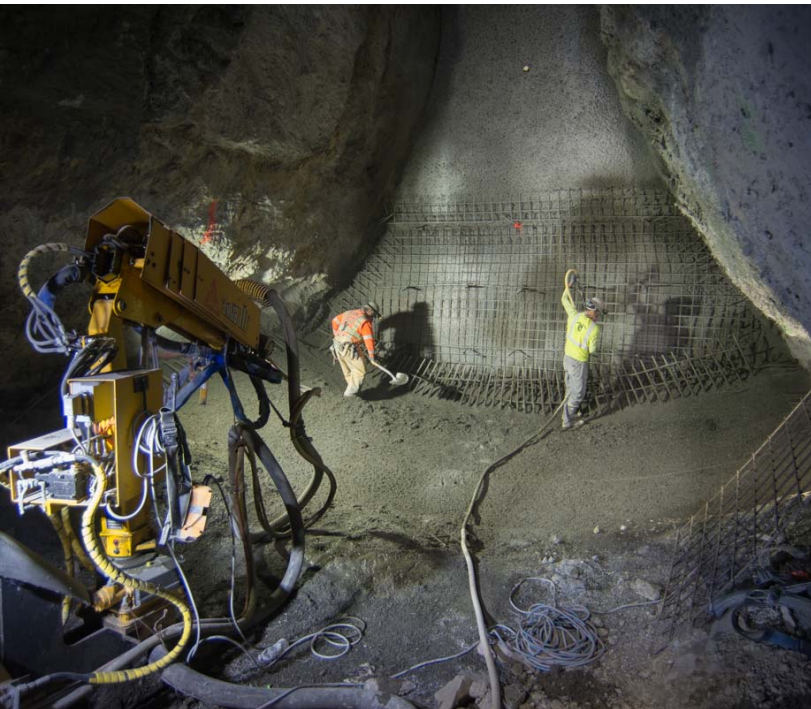
2 Reinforcing steel mesh and shotcrete are applied to the walls and invert
