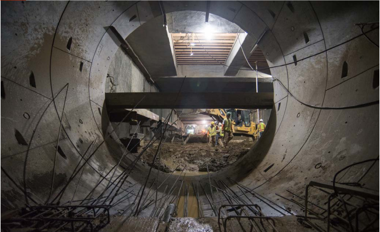
Looking south from just inside the northbound tunnel, workers use a large bulldozer to move steel beams into place before installing them as temporary bracing.
