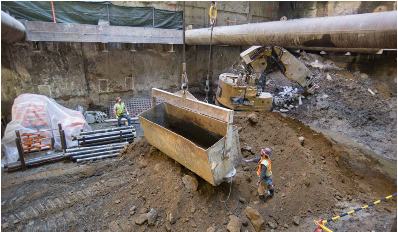
Crews use a large steel container to bring material into the headhouse used to temporarily backfill the approach to the cross-cut cavern, so heavy machinery can more easily move in and out during drilling operations.
