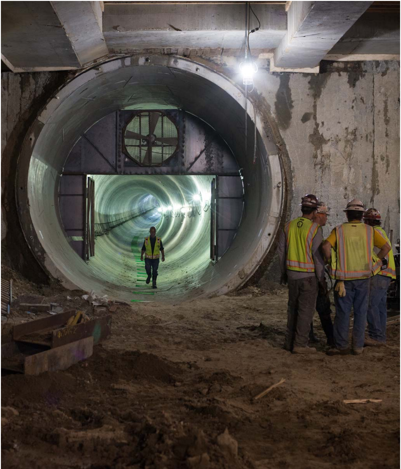
Looking down the northbound tunnel while a crew discusses operations at the southeast corner of the platform level, inside the station box under 4th Street.
