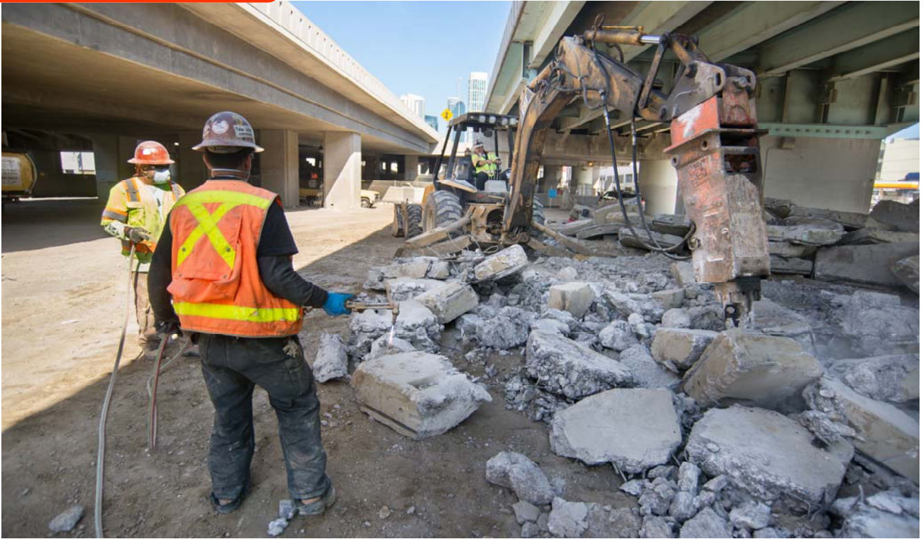
Workers use cutting torches to cut rebar in precast concrete segments removed from unnecessary sections of tunnel inside the YBM station box.
