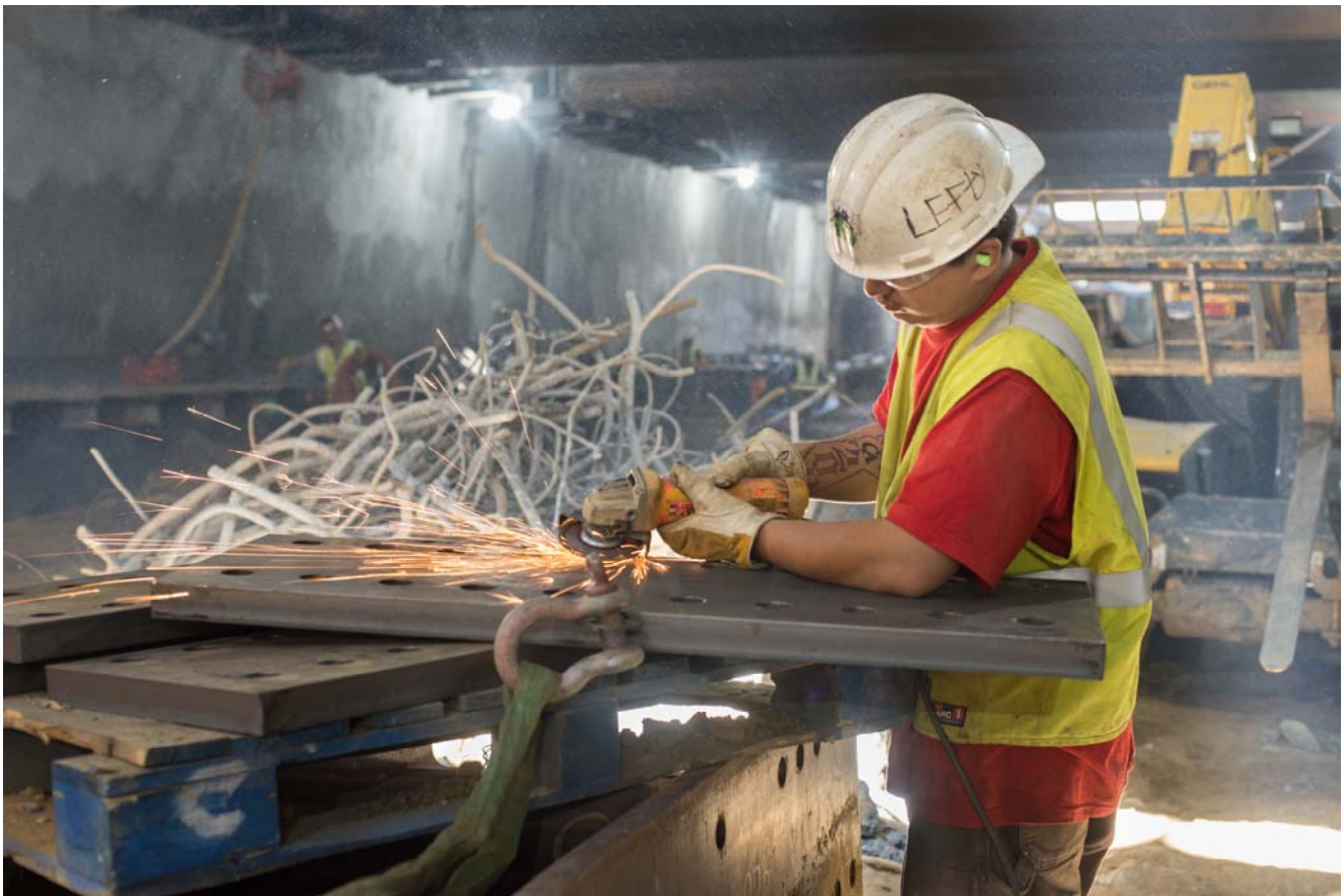
A worker smooths the edges of holes for bolts on a bracket used in temporary bracing inside the station box.
