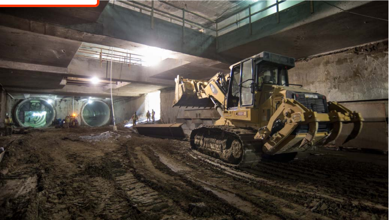
A large bulldozer drags a steel beam called a waler, used to temporarily reinforce the outer walls during excavation.
