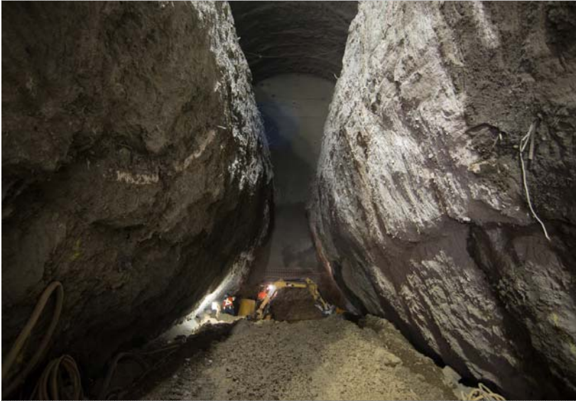
1 Workers use smaller excavation equipment inside the center drift to reach bottom
