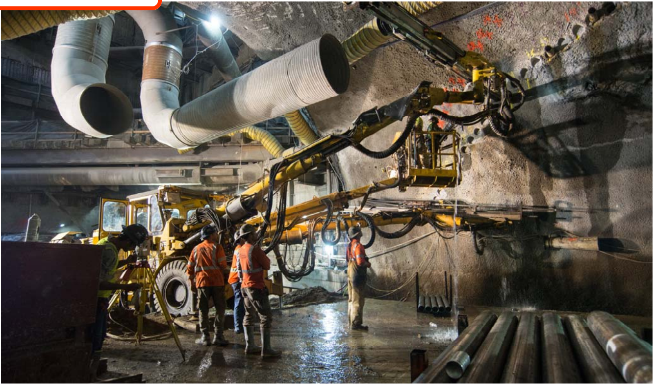
Multiple arms stretch from the drill rig stationed at the cross-cut cavern entrance, where drill casings are ready to be installed during soil grouting.
