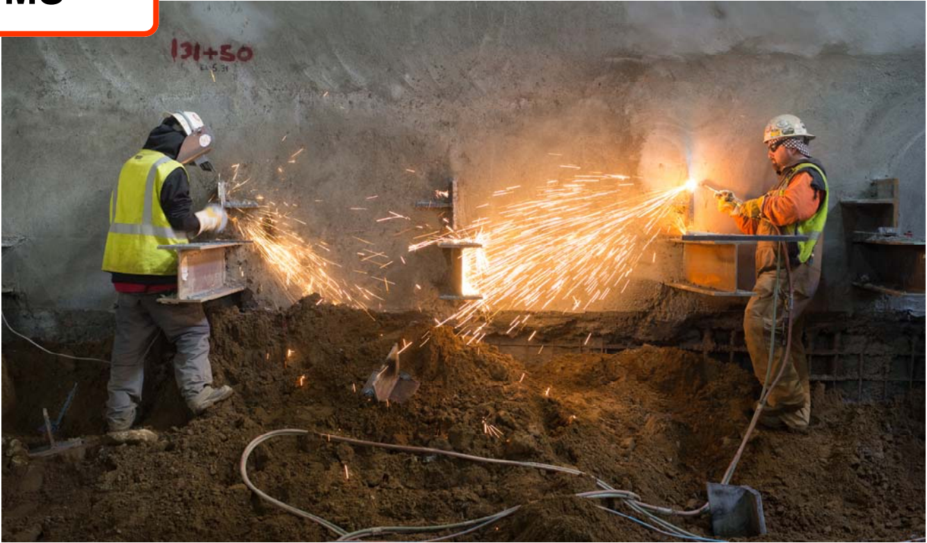
Two ironworkers duel in fire as they adjust the length of brackets for temporarily steel reinforcing on the west side of the station box near Geary.
