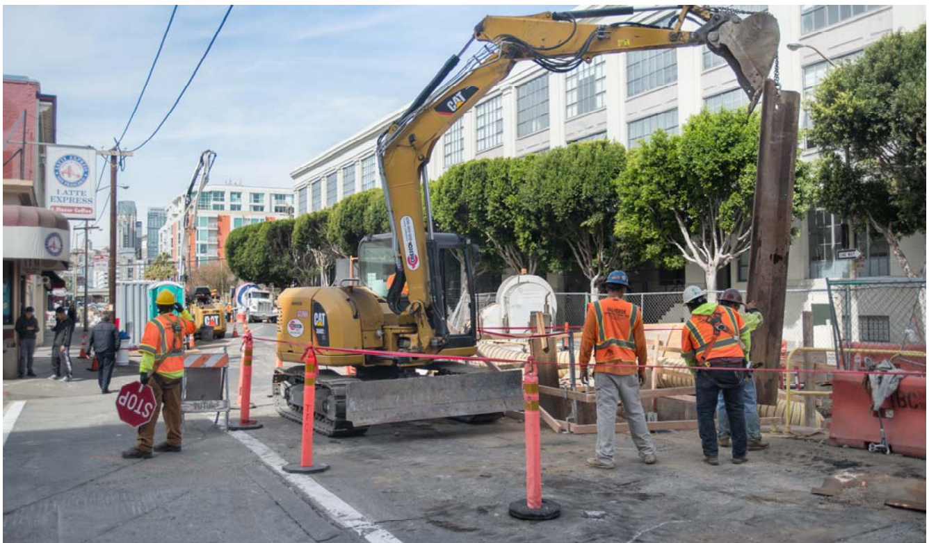
Steel sheet piles are lowered into place to reinforce an excavation site at 4th and Bluxome, where utility upgrade work is underway.
