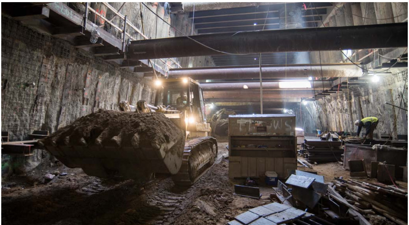
A bulldozer carries a load of soil excavated from the north end of the station box, near the O'Farrell access portal.
