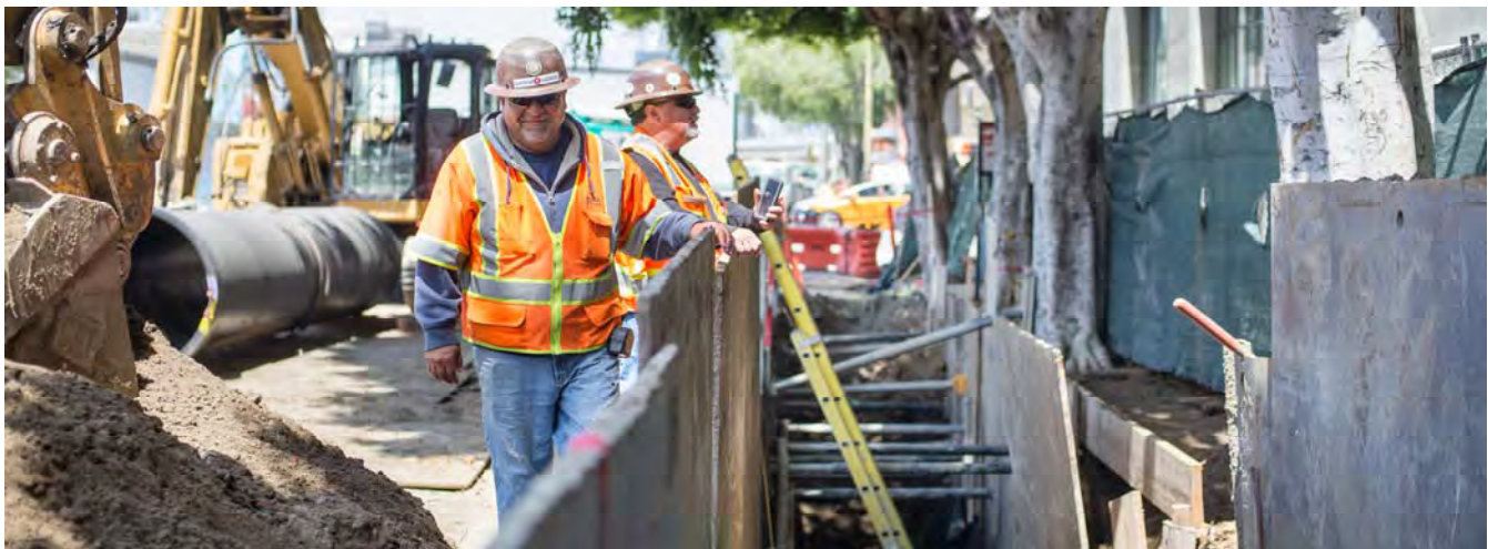
As new sections of sewer pipe are installed in this trench on the east side of 4th, completed sections are backfilled and soil is compacted.
