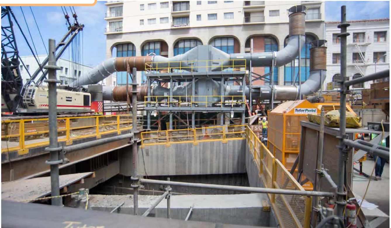
Newly-installed ventilation fans and ductwork on the east side of the Chinatown head-house site.
