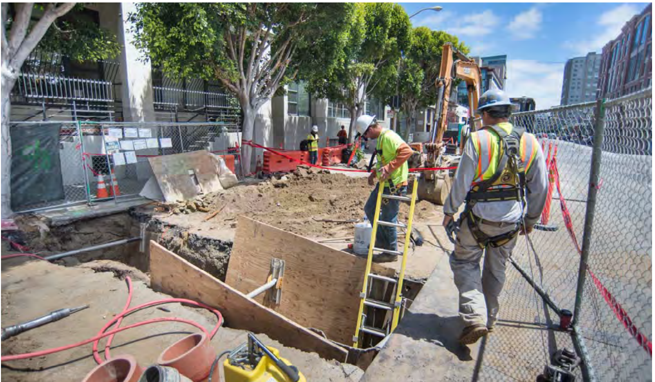
Workers donning safety harnesses prepare to do trench work north of Bluxome alley, where utility laterals are being reinforced and upgraded.
