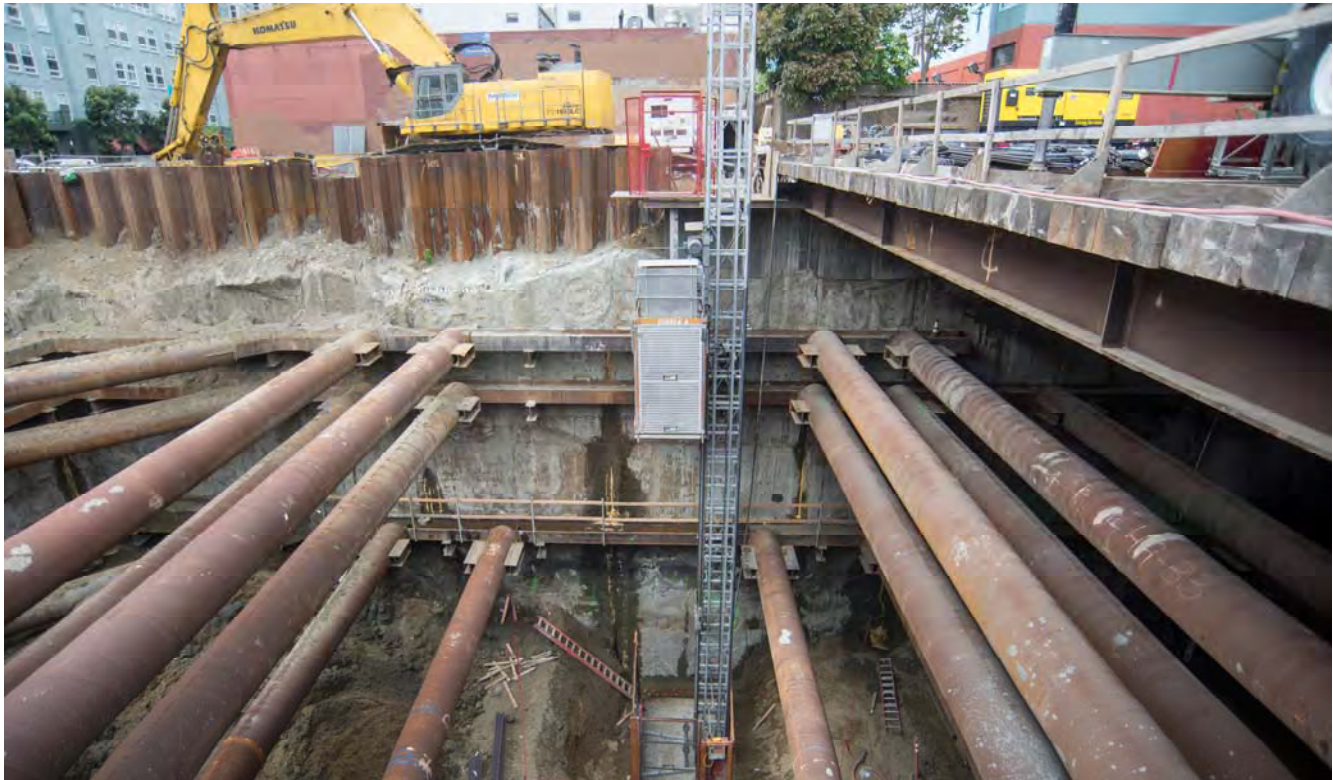
The contractor has installed an elevator to carry workers and equipment to and from the work sites underground.
