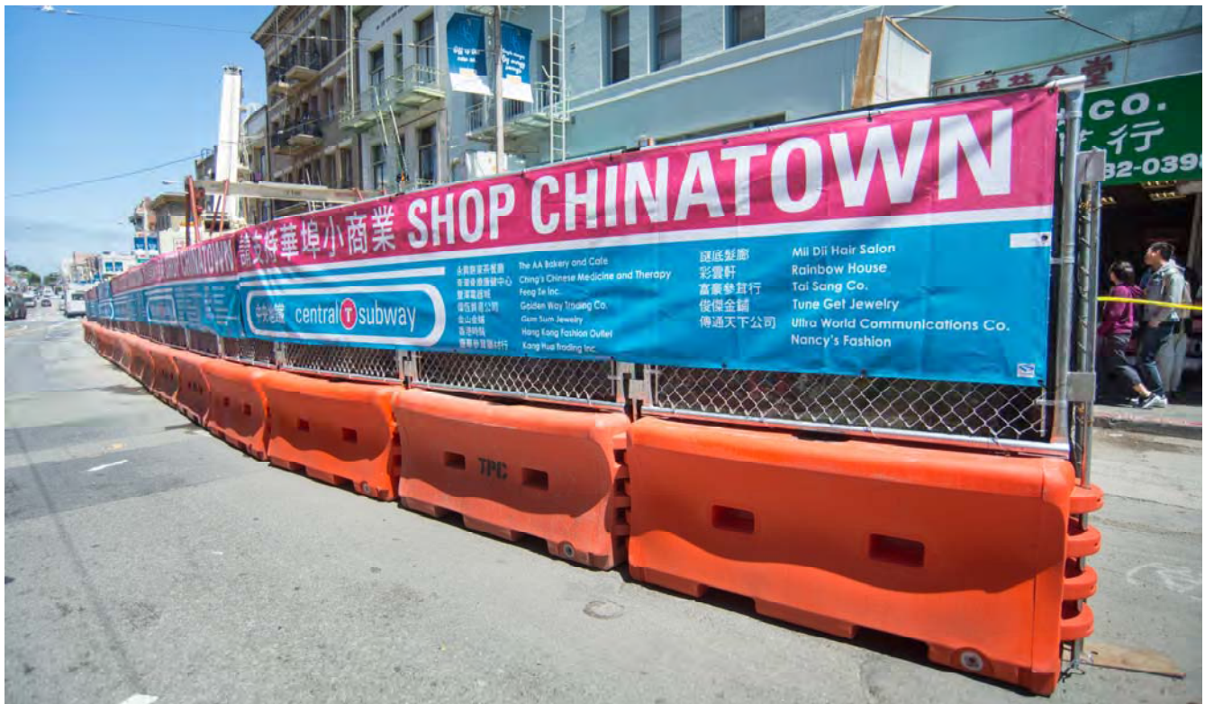
New banners indicating nearby businesses have been installed along the construction fence for the north access shaft between Washington and Jackson on Stockton.
