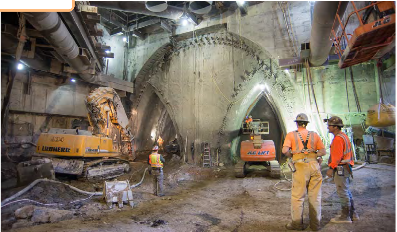
Workers pause before installing steel mesh and spraying shotcrete to reinforce the freshly-excavated walls of the left and right side drifts.
