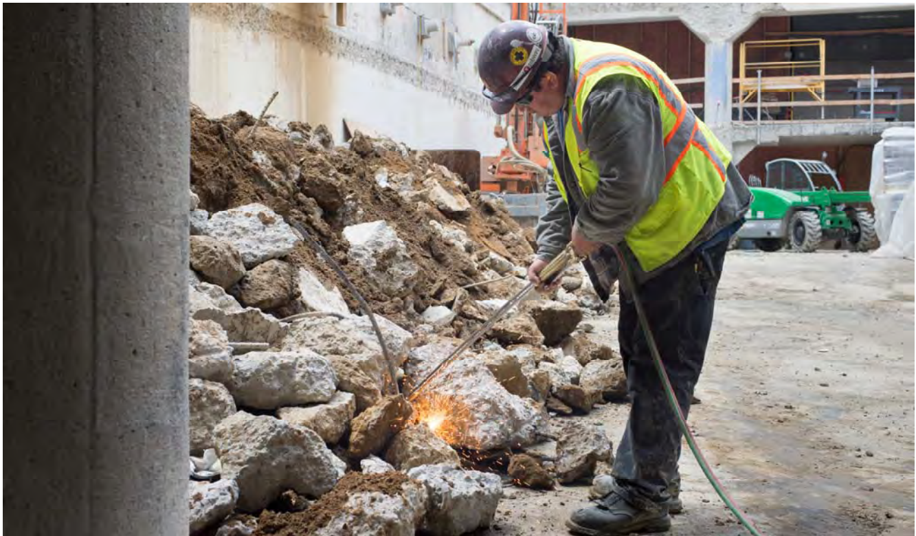
A worker uses a cutting torch to cut sections of rebar away from concrete rubble inside the southeast corner of the Union Square Garage, where the future north station entrance will be located.
