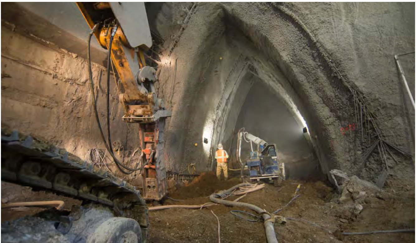
Shotcrete spraying inside the left side drift. These smaller excavation caverns are necessary before creating larger voids, so as to prevent potential ground movement.
