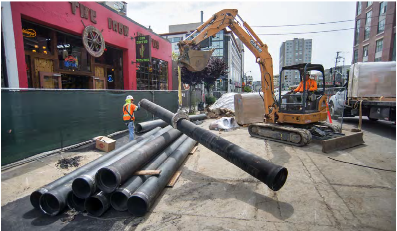
Sections of pipe are unloaded from a truck north of Townsend and stacked for installation.
