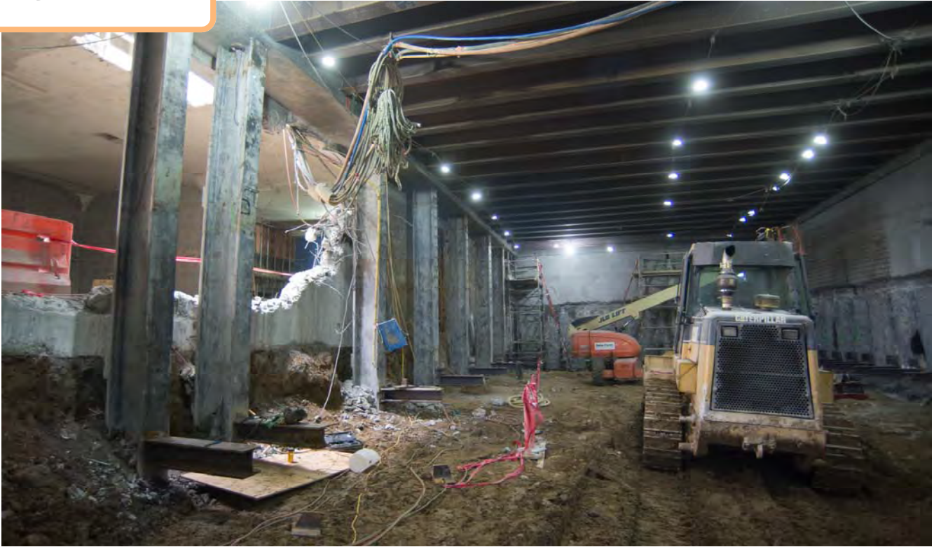
Vertical beams span the west wall inside the north concourse, where demolition work to remove a wall inside the Union Square Garage is ongoing just behind them.
