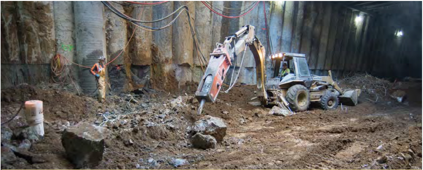
A backhoe fitted with a large jackhammer pulverizes large pieces of concrete removed from the north headwall.
