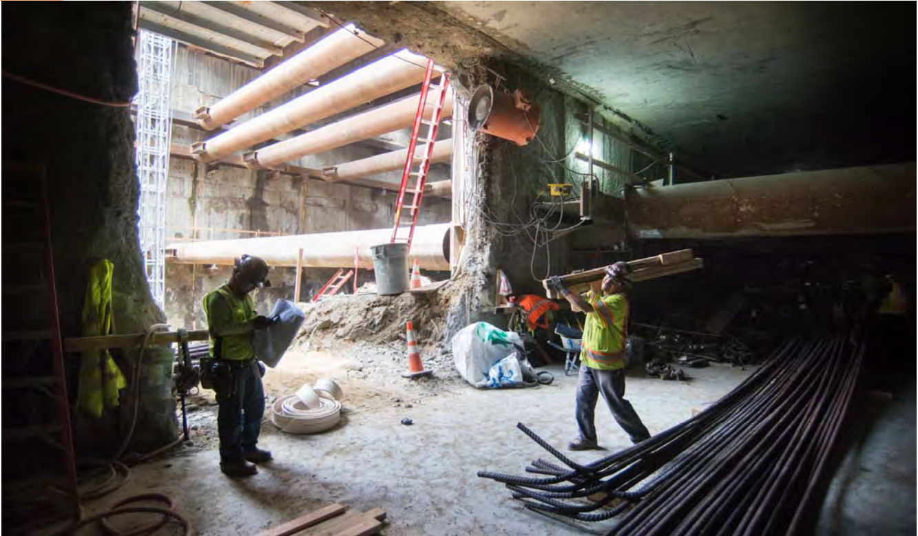
A man checks plans at the access portal from the headhouse into the station box while an associate carries concrete form pieces to be installed precisely where needed.
