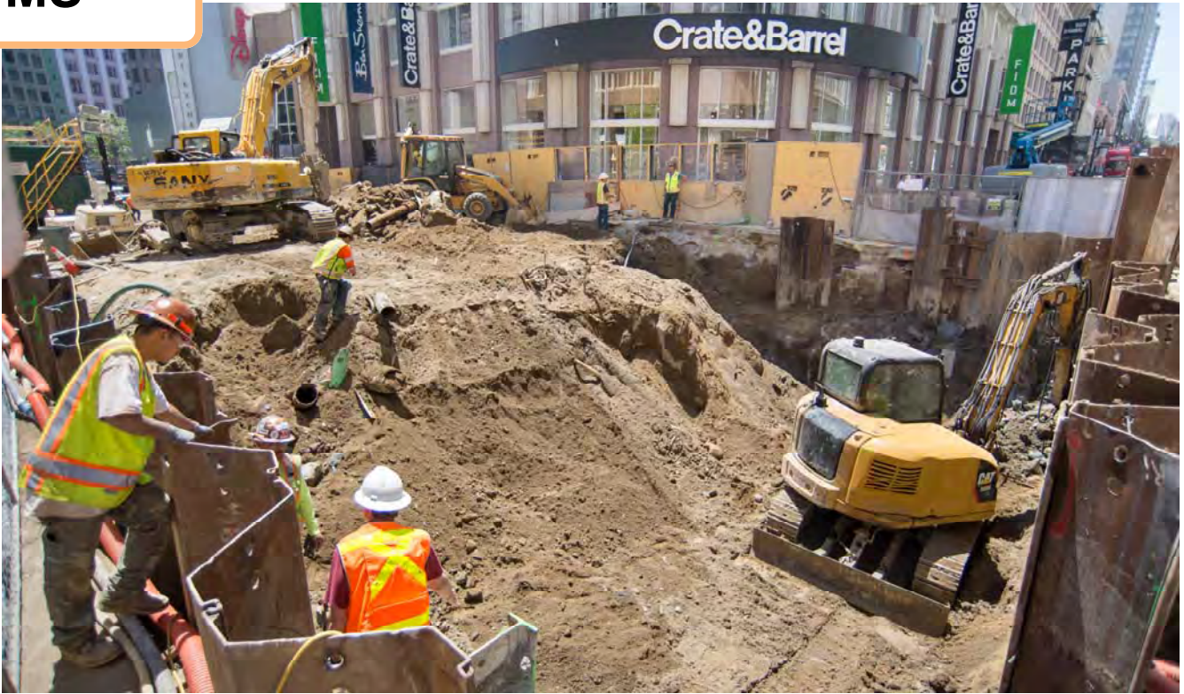
On the south side of the Stockton and O'Farrell intersection work is being done to prepare for the installation of another station roof deck panel.
