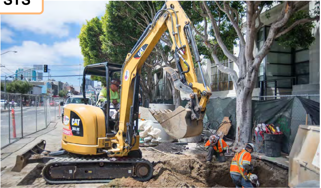
When needed, workers use shovels to carefully unearth utilities which will be upgraded and reinforced. Here, utility laterals are being unearthed following sewer upgrade work.
