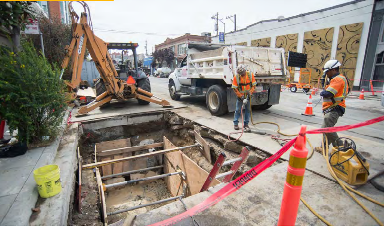
Workers pump out water from an excavation at 4th and Bryant where utilities are being upgraded.
