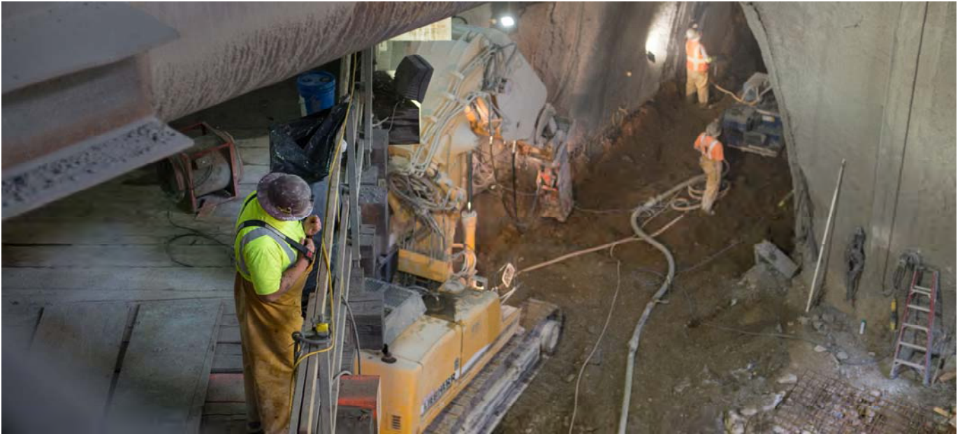
A worker looks down onto shotcrete operations from a platform where shotcrete mixing and pumping equipment is located.
