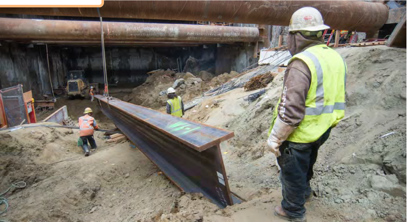
Workers lay down cribbing underneath the large steel beam, as it's lowered into the head-house for installation.
