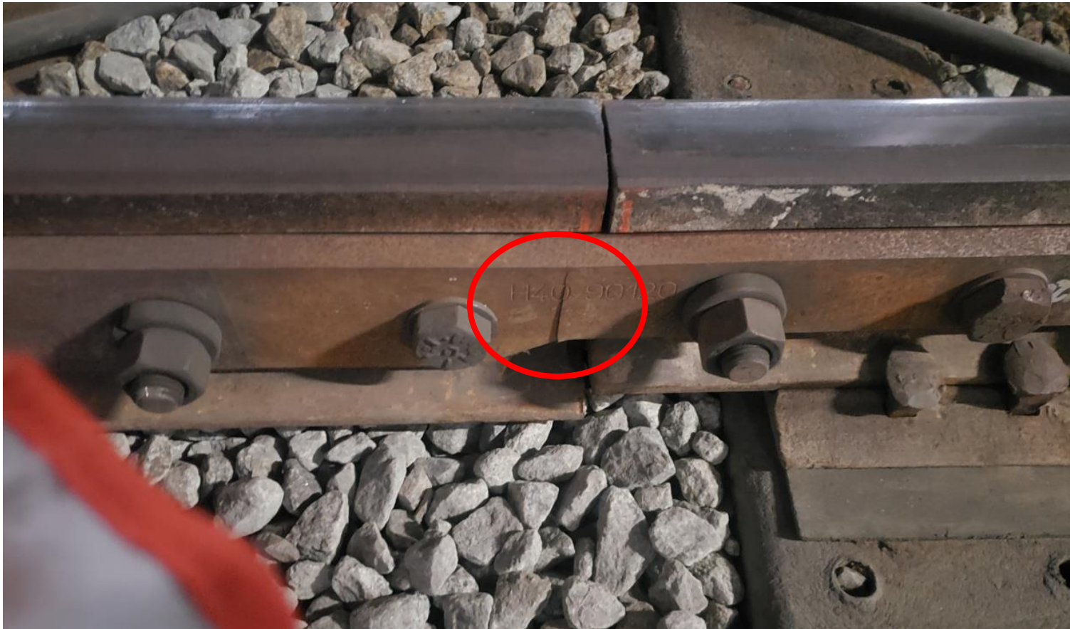
Cracked Compromise Joint
