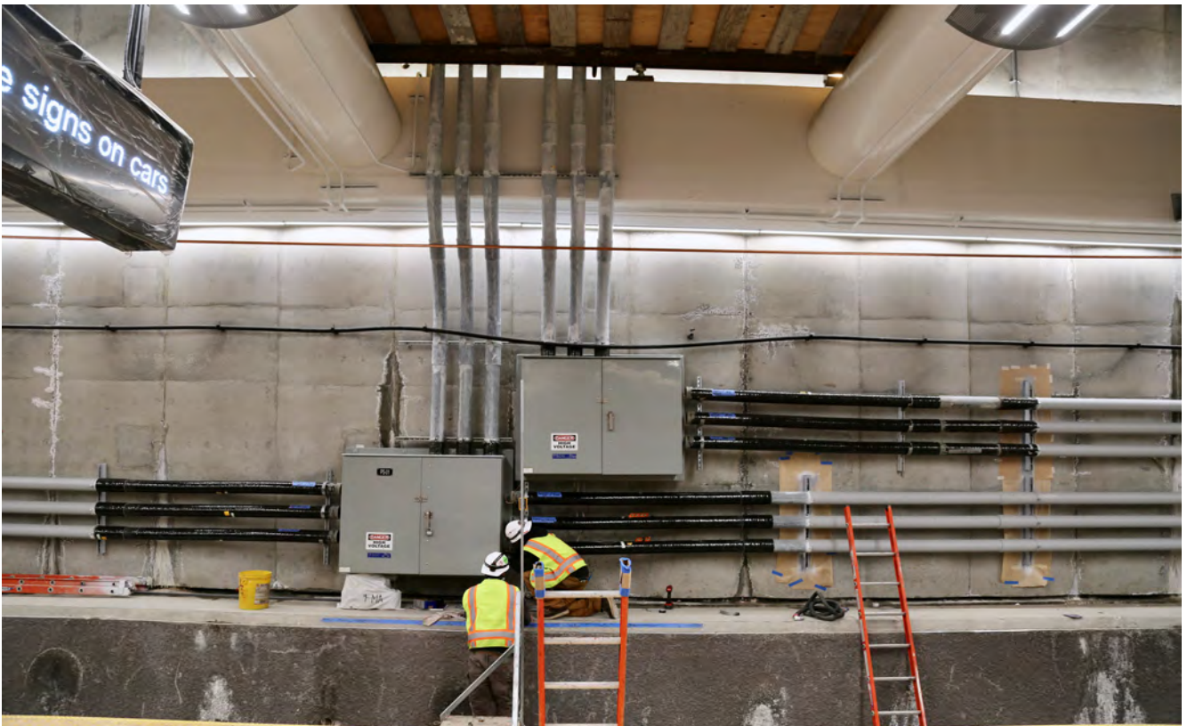
View of the conduit and power boxes at the platform of UMS
