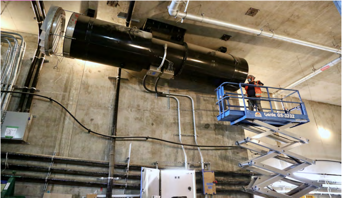
Inside the portal, looking at the conduit on the wall with a fan being worked on
