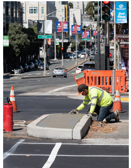
A worker puts the final touches on an improved pedestrian median at Geary and Divisadero. As utility work wraps up, crews are installing new sidewalk extensions (bulbs), curb ramps and medians that will improve safety, accessibility and bus performance along Geary.
