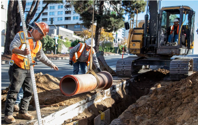
1.5 miles of sewer mains and 2.9 miles of new water mains are over 75% completed
