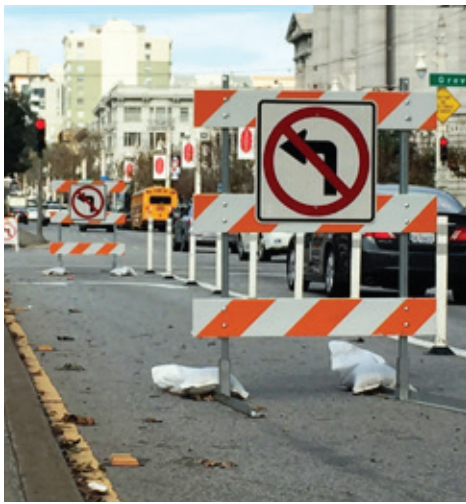
The Van Ness Business Advisory Committee has asked the Van Ness Improvement Project staff to help businesses by providing directions for navigating traffic changes on Van Ness Avenue.
