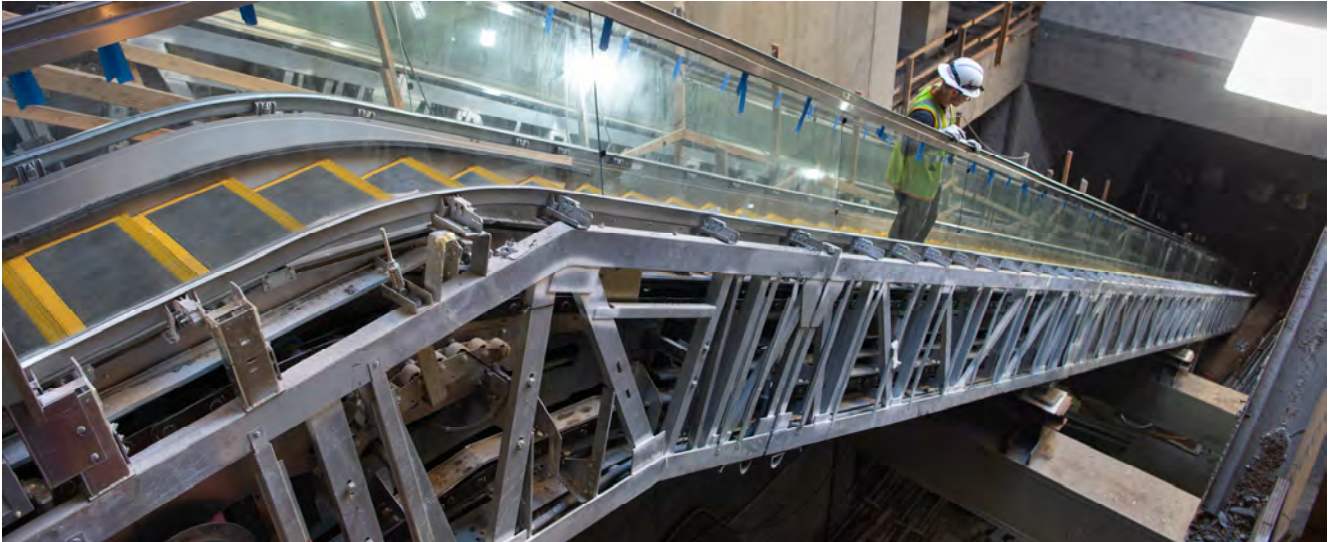
A worker pauses while observing associates nearby along one of the two massive escalators leading to and from Chinatown Station's headhouse lobby and fare gate area from the upper mezzanine.
