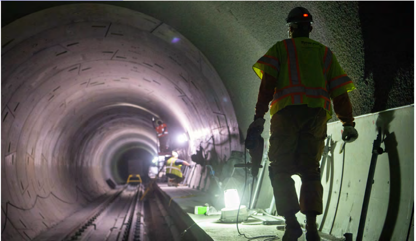
A worker carries an impact drill during installation of future tunnel walkway railing elements inside the southbound tunnel just north of the Chinatown Station platform area.
