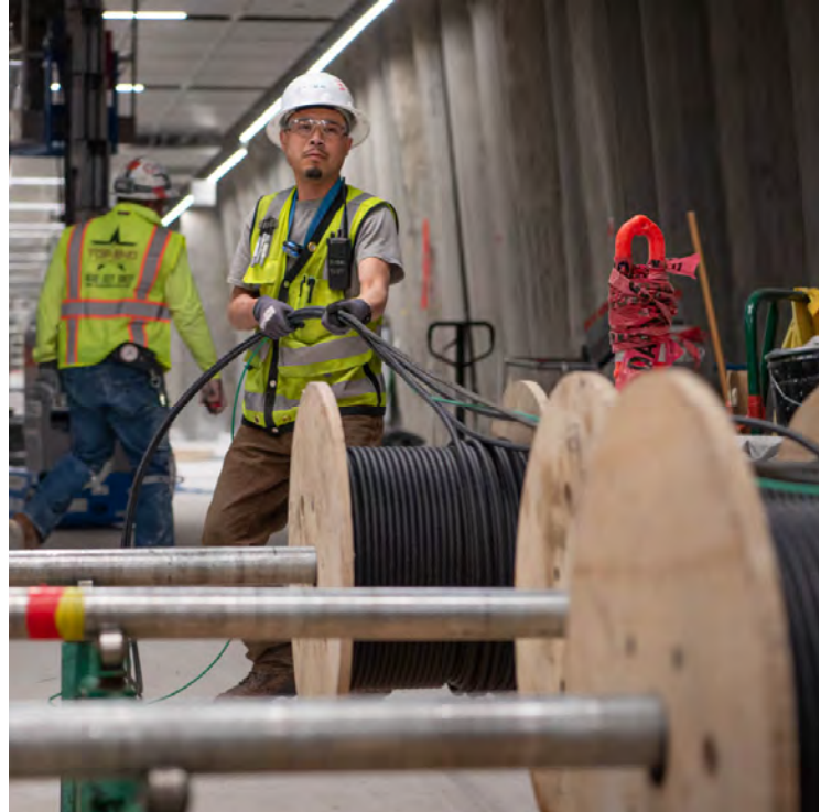
Large cables are pulled and installed in conduits located above ceiling panels inside the station concourse.
