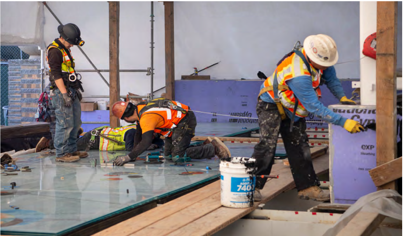
Colorful glass panels are being installed atop the north entrance structure for Union Square/Market Street Station.
