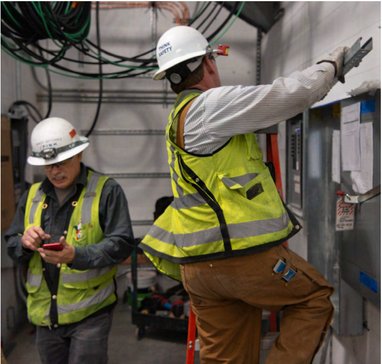
An inspector and a technician check measurements to install steel brackets inside a utility room at the north end of the Union Square/Market Street Station platform.
