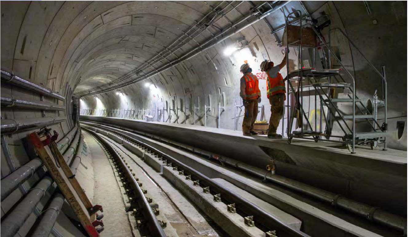
Two men install specially-fashioned utility conduits and mounting brackets inside the northbound tunnel S-curve below the Market Street subway.
