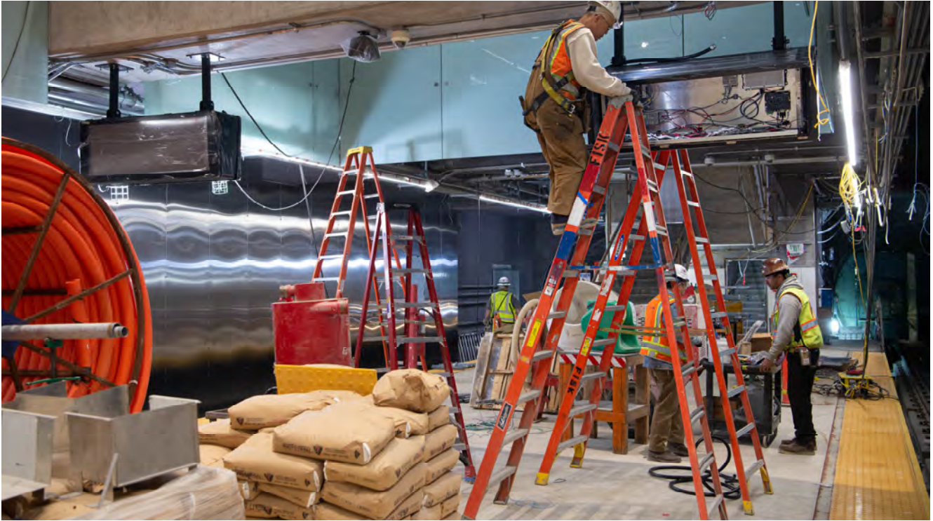
Electronic display boxes are being installed at the north end of Yerba Buena/Moscone Station's platform.
