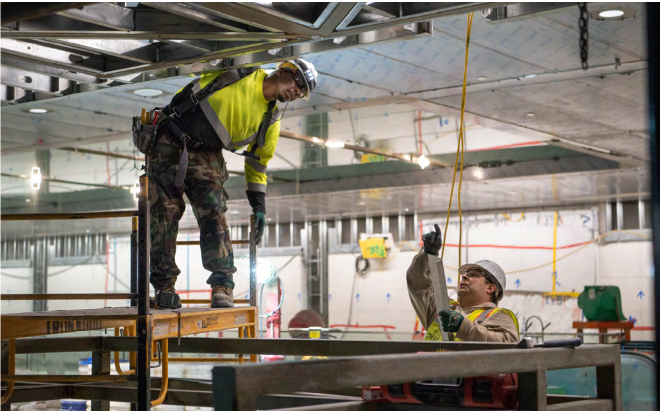
Pieces of steel framing are fabricated and installed piece by piece at the future fare gate entrance area for Yerba Buena/Moscone Station.
