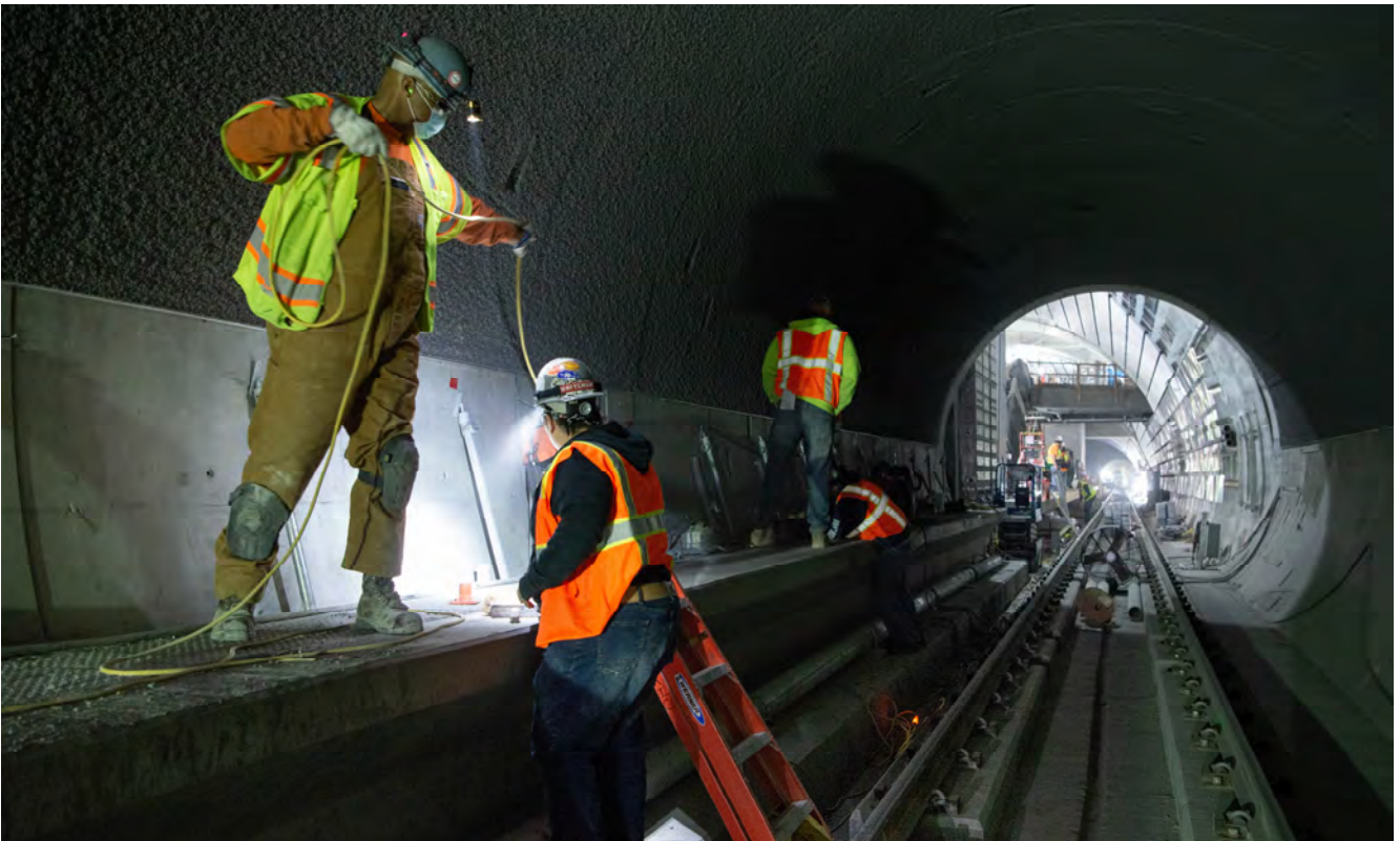
Workers install elements of tunnel walkway railing inside the southbound tunnel, just north of the Chinatown Station platform cavern.
