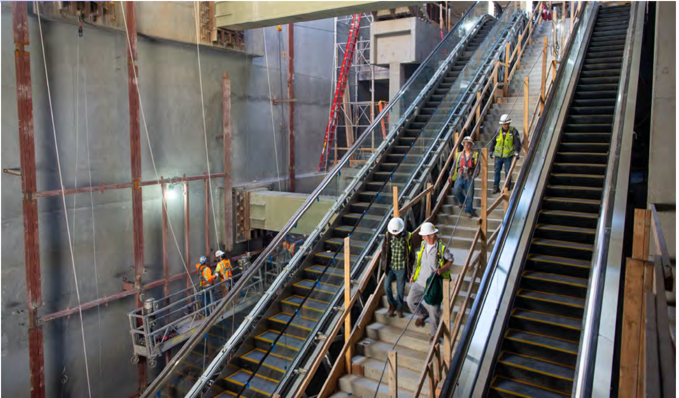
Workers descend the staircase leading from the upper mezzanine into the future Chinatown Station lobby and fare gate area, while steel framing for interior future wall sections is assembled nearby.
