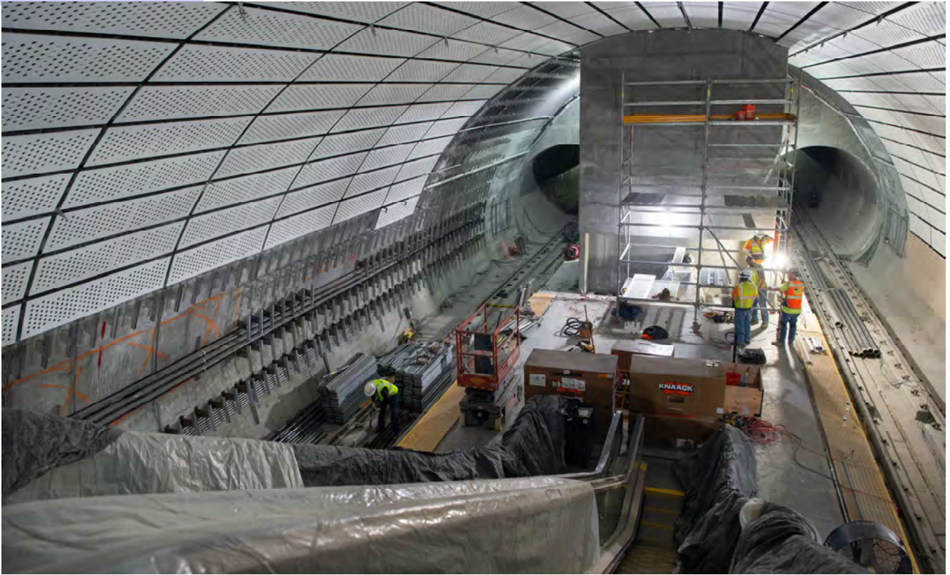
At the north end of the Chinatown Station platform cavern, perforated white panels have been installed with brackets against the arched ceiling and walls.
