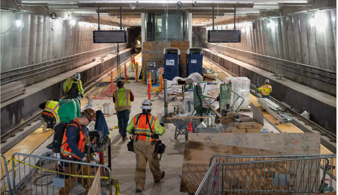
Future message boards and other detailed station elements are being installed on Union Square/Market Street Station's platform level.
