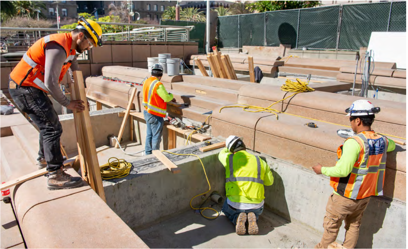
Textured concrete steps and terrace blocks are being placed atop concrete foundation walls in the portion of Union Square surrounding the north entrance for Union
