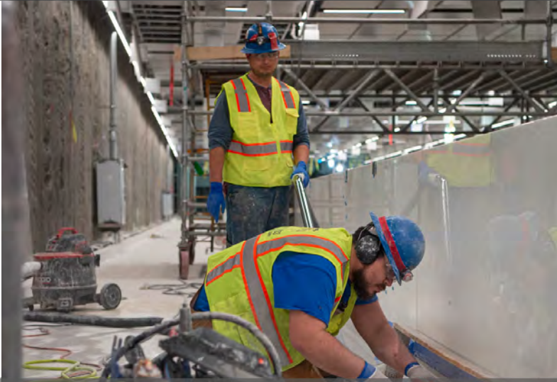
Two men work to keep the area dust-free while smoothing and buffing terrazzo floor transitions.
