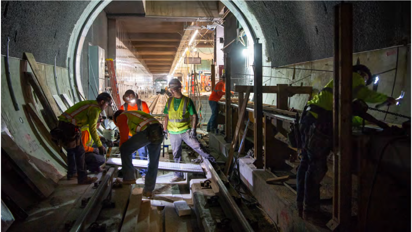
Concrete formwork, rebar cages, and steel panels are being installed to build out one of the last sections of tunnel walkway, seen inside the northbound tunnel as it exits the Yerba Buena/Moscone Station platform area.
