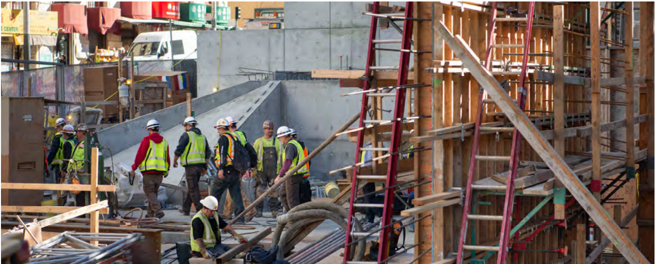
Workers file out of the staff elevator at the end of the day shift, atop the steel-level worksite for Chinatown Station.
