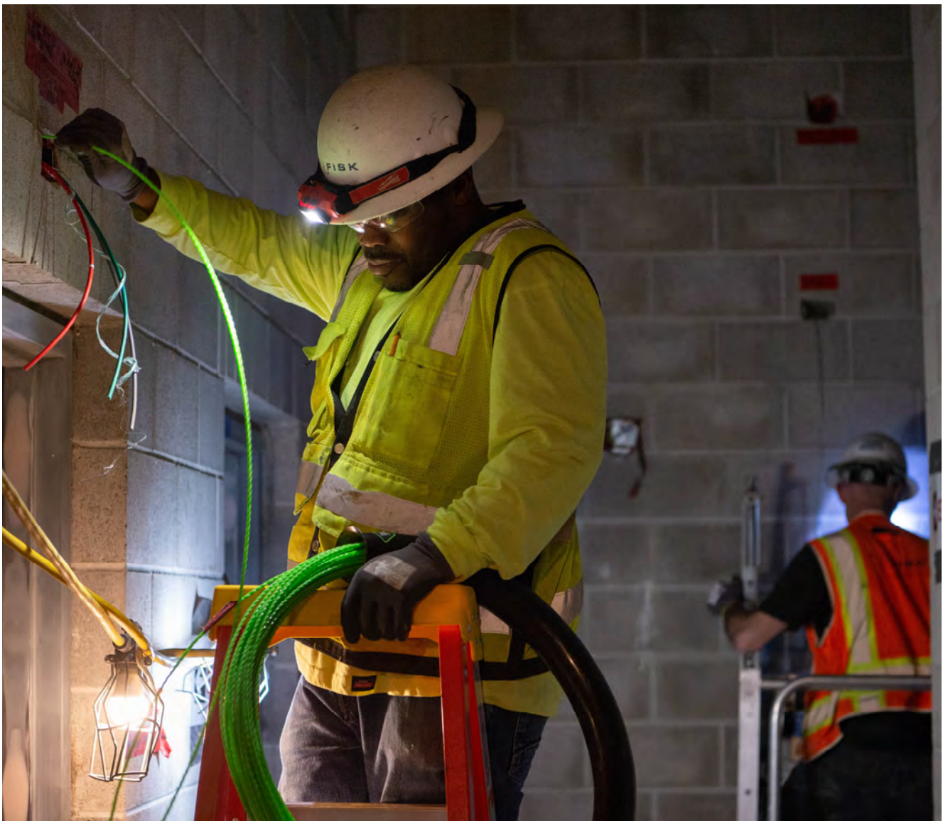
A technician installs electrical and communication wiring on an intermediate floor inside the Chinatown Station headhouse.
