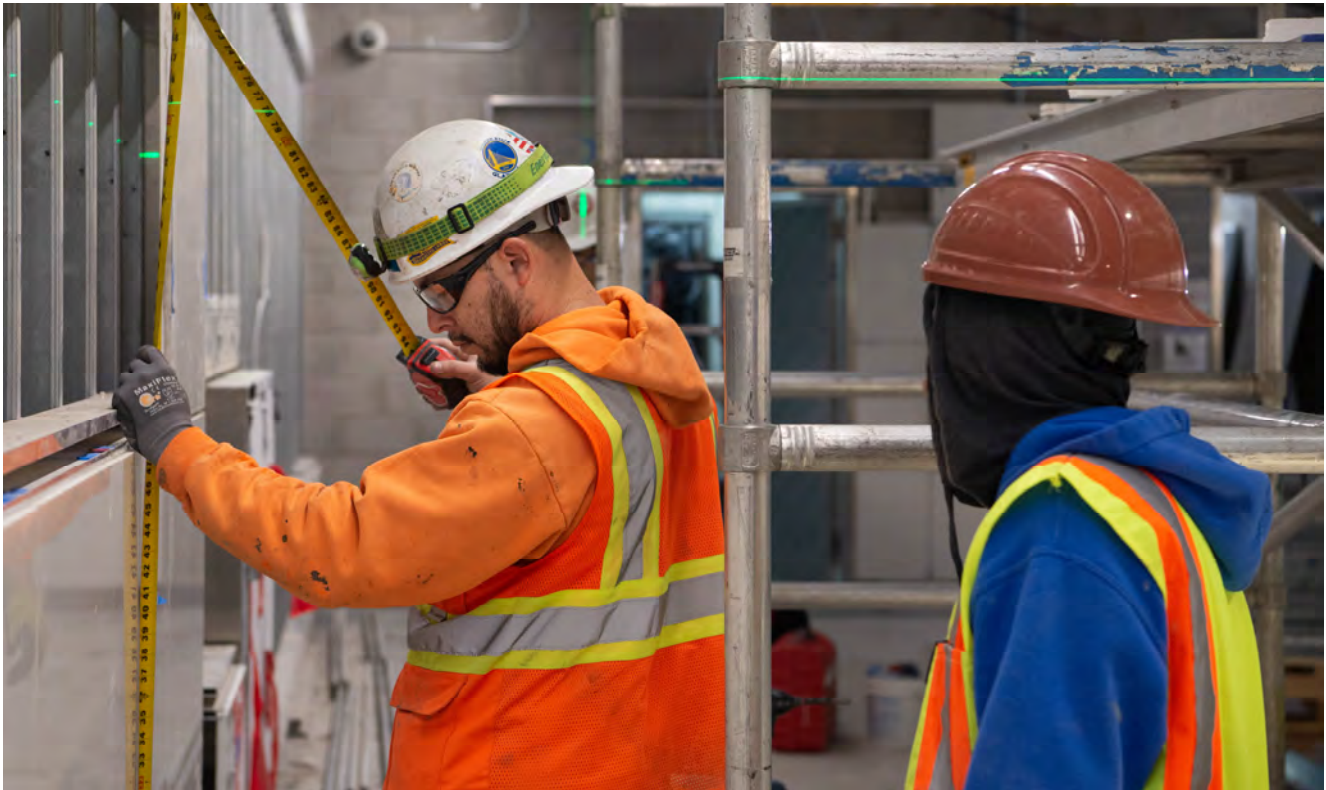
Workers the west side of the Yerba Buena/Moscone Station concourse measure the height of recently-installed wall panel sections.
