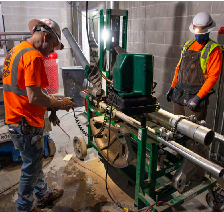
Sections of pipe and conduits are rolled and shaped to fit specifications.
