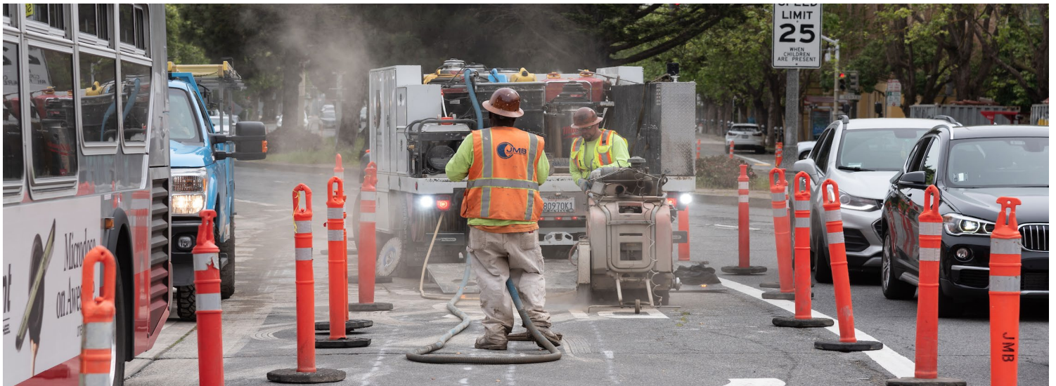
Crews work to replace aging sewer and water lines on Geary Boulevard near Divisadero Street as part of the Geary Rapid Project.
