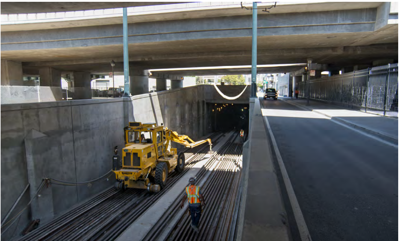
A crew organizes lengths of rail inside the tunnel portal structure under the I-80 Freeway overpasses at 4th street.
