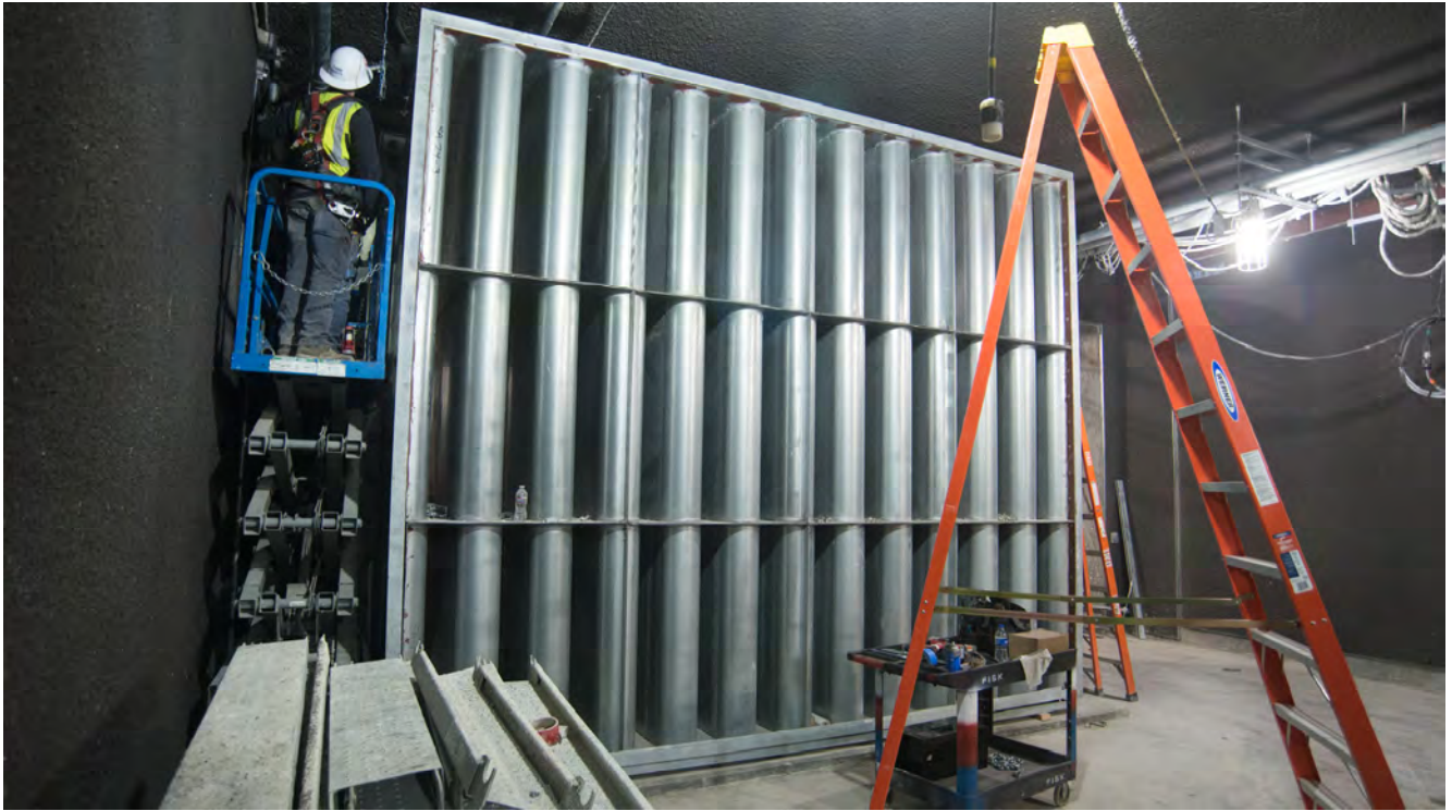
A large radiator system has been installed inside the Yerba Buena/Moscone Station headhouse's mezzanine level.
