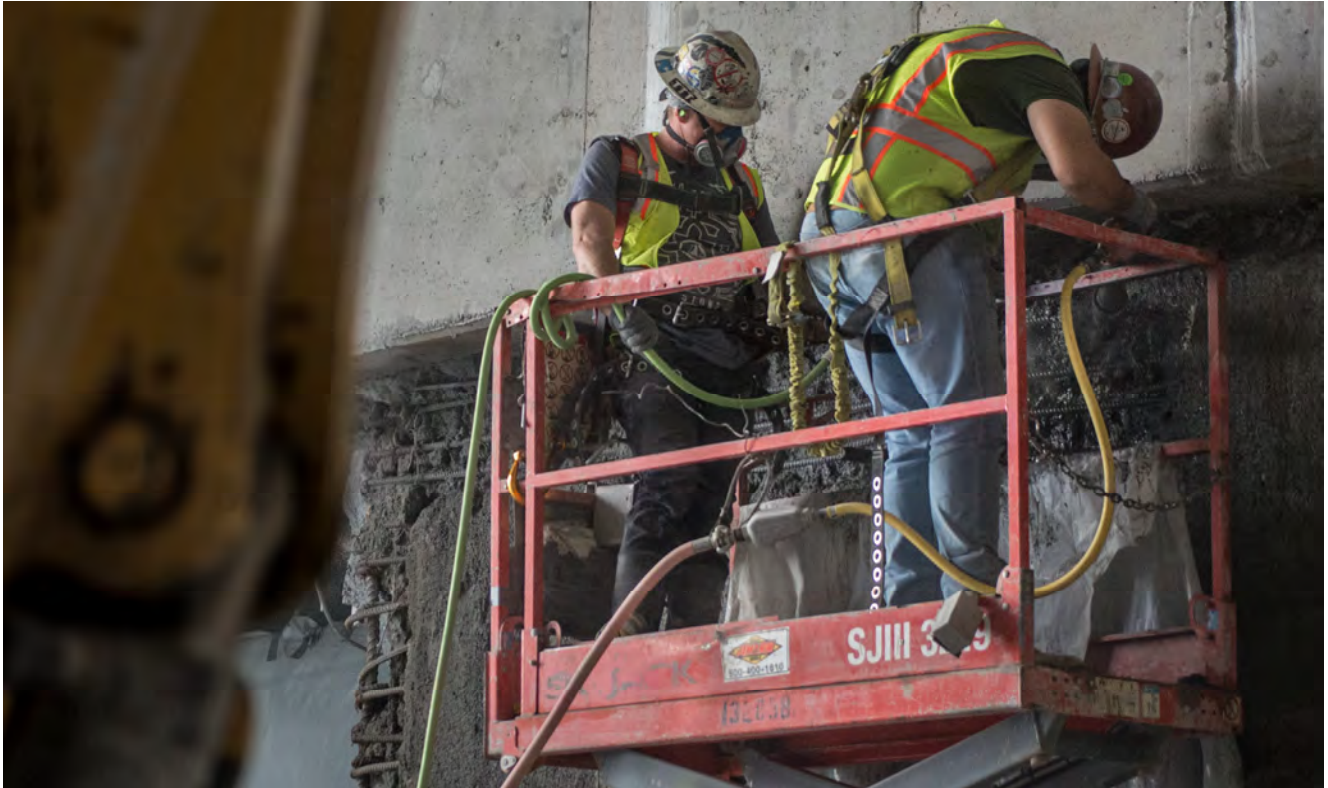
Workers use a jackhammer to remove concrete from a section fo slurry wall slated to be removed to widen the future Yerba Buena/Moscone Station fare gate entrance.
