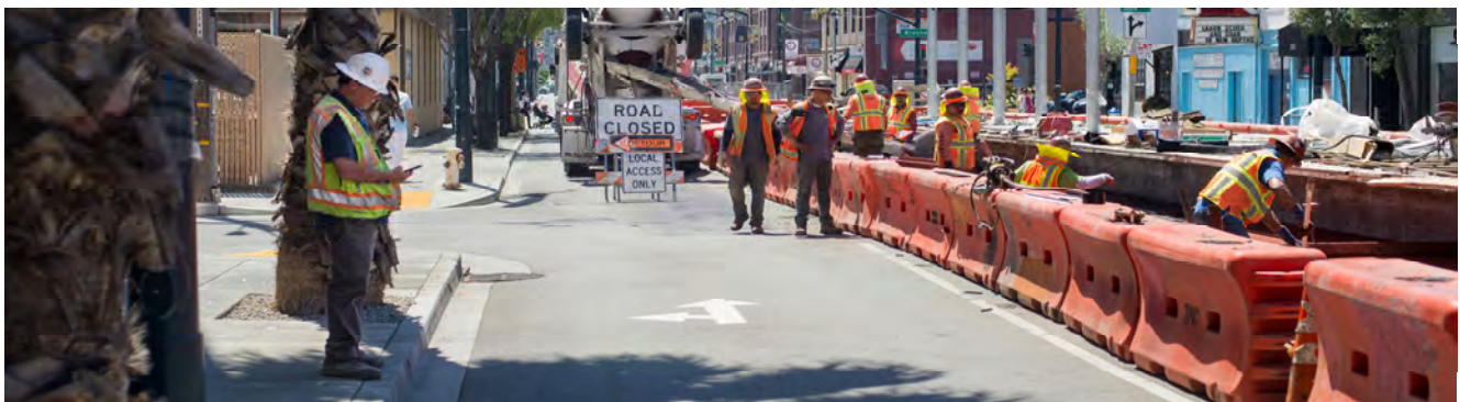
A site inspector records observations during a concrete pour for the alternating red and gray rail slab adjacent to the 4th and Brannan surface station platform.
