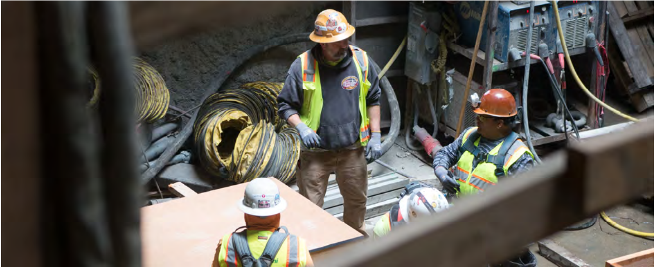
Carpenters discuss and prioritize work to build concrete forms along the east side of the Chinatown Station headhouse's concourse level.
