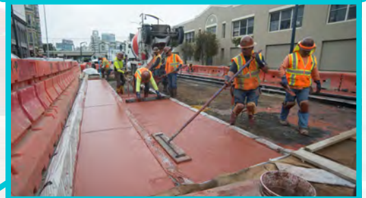
4th St. Surface Track, Systems (STS)
