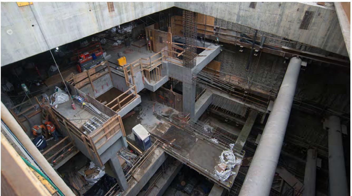
Multiple levels of interior structures can be seen looking down into the main shaft of the Chinatown Station headhouse.
