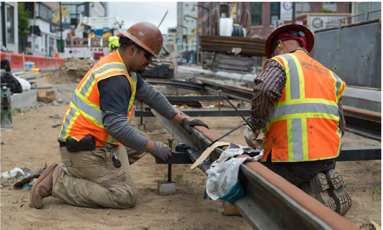
Two workers make adjustments to temporary spacers used to level the rails along the southbound track side of the surface alignment south of Brannan.
