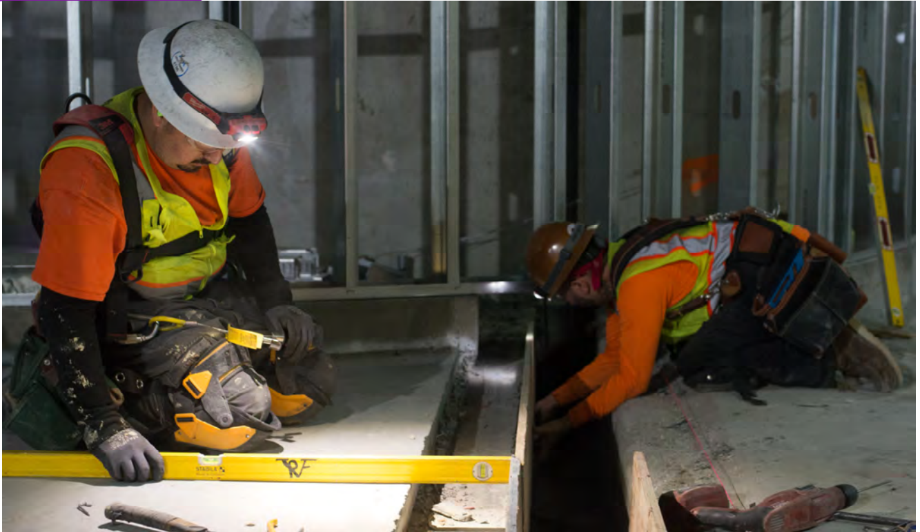
Workers make preparations to install a section of expansion joint in the floor slab where the south concourse of Union Square/Market Street Station meets the entrance to the Powell Station concourse.
