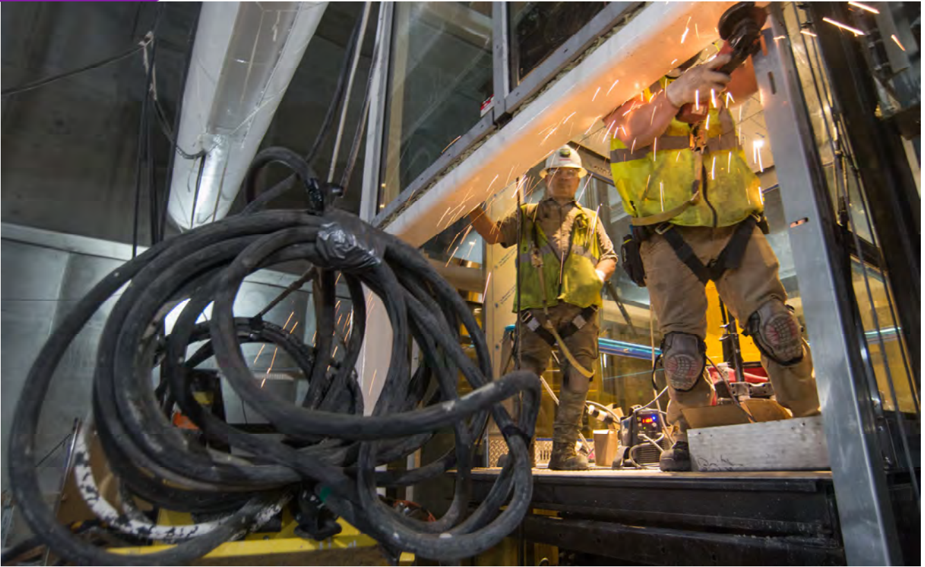
Sparks fly as a worker cuts notches in a L-shaped piece of steel at one of the platform-to-concourse elevators for Union Square/Market Street Station.
