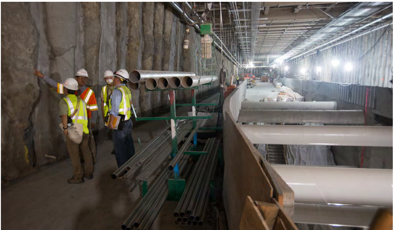
A group of engineers examines the station's exterior wall tangent piles as it tours the south concourse of Union Square/Market Street Station.
