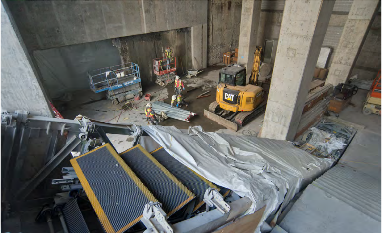
A crew collects sections of pipe on the concourse level of Yerba Buena/Moscone Station's headhouse, with a new escalator peeking out in the foreground.
