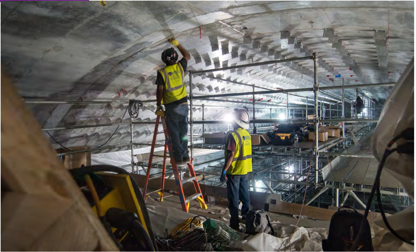
Two men check seams and smooth the surface of the Chinatown Station platform cavern's arched ceiling, ahead of installing another row of steel brackets.
