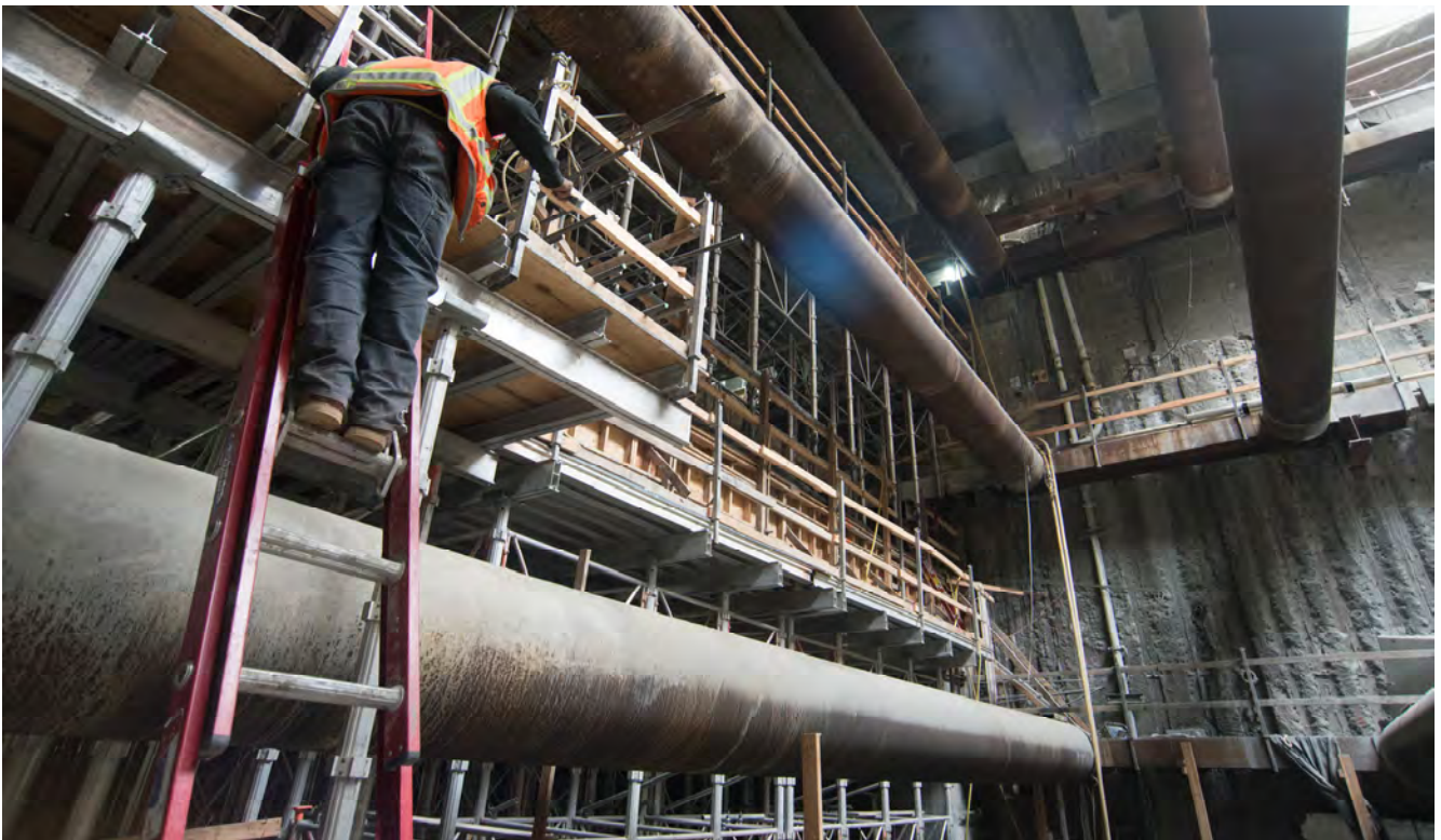
Temporary bracing spans across the width of the work area as a worker descends from an upper level of the Chinatown Station headhouse currently under construction.
