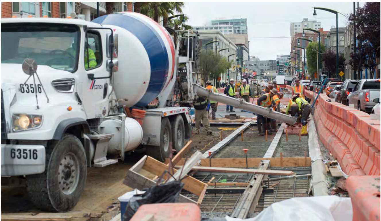
A crew pours another section of rail topping slab along the southbound track side of the surface alignment near Welsh Alley.
