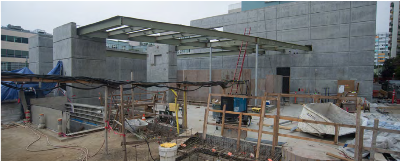
Recently-installed structural steel framing denotes the edges and structure of the future Yerba Buena/Moscone Station entrance structure roof line.
