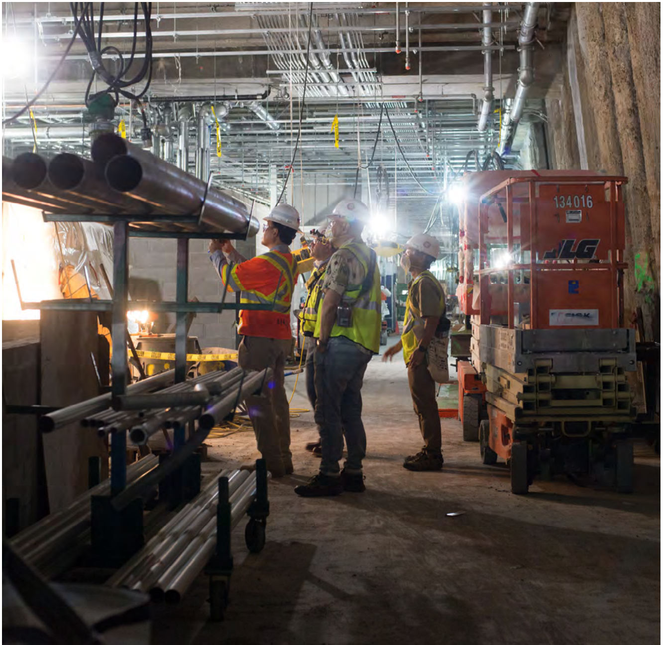
Engineers observe construction on the south concourse for Union Square/Market Street Station.
