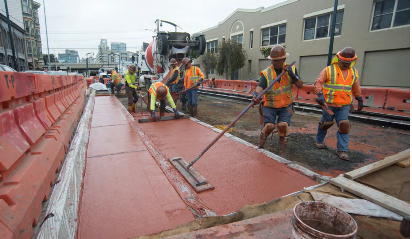
Workers put the finishing touches on a freshly-poured section of the red-tinted topping slab along the southbound track near Welsh Alley.
