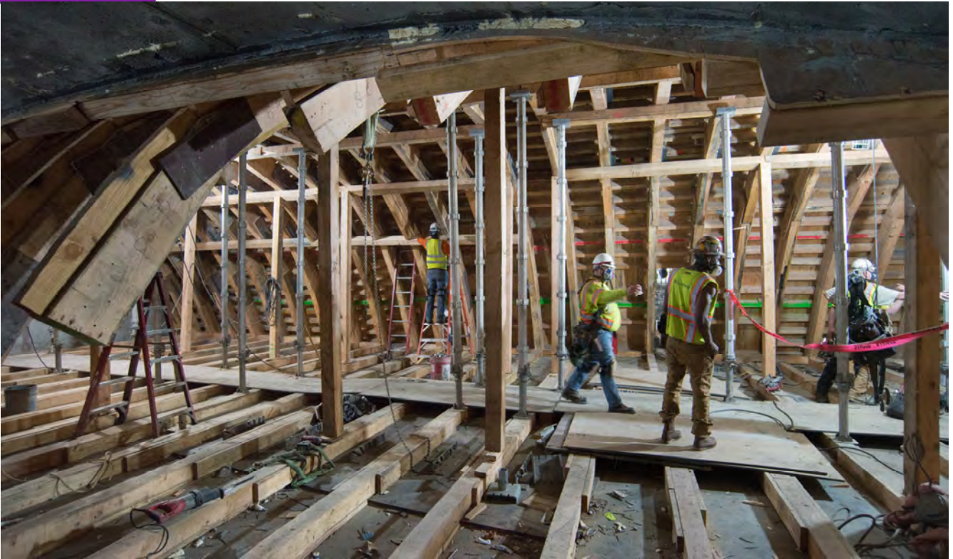
Workers disassemble sections of heavy-duty concrete forms used to create the compound arched ceiling for the entrance into the Chinatown Station cavern.
