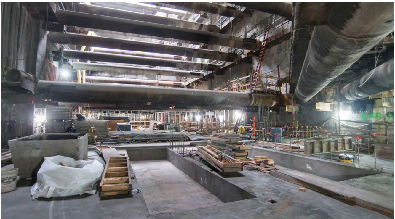
Recesses in the floor slab of the concourse level of the Chinatown Station headhouse mark the eventual landing spots for escalators which will carry passengers to and from the street level high above.
