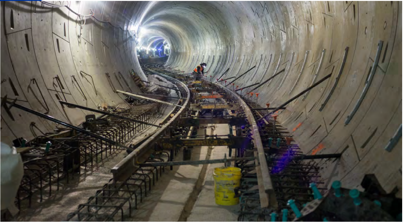
Rebar for future track foundations continues to be installed in the southbound tunnel, as seen just south of the Union Square/Market Street Station platform, inside the S-curve under the Market Street subway.
