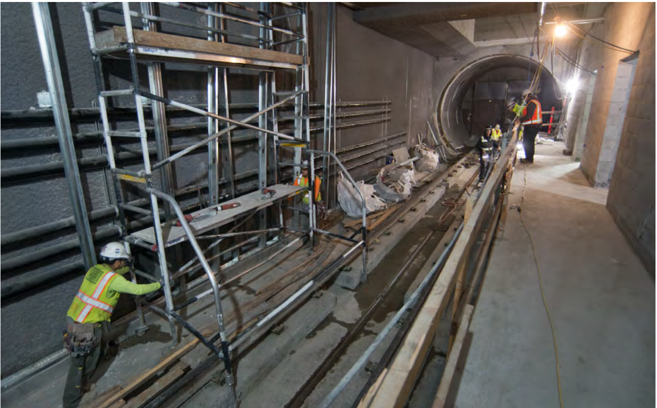
A large section of rolling scaffolding is rolled into place for the installation of metal studs to build a furring wall to hide utility conduits against the northbound side of the Yerba Buena/Moscone Station platform.
