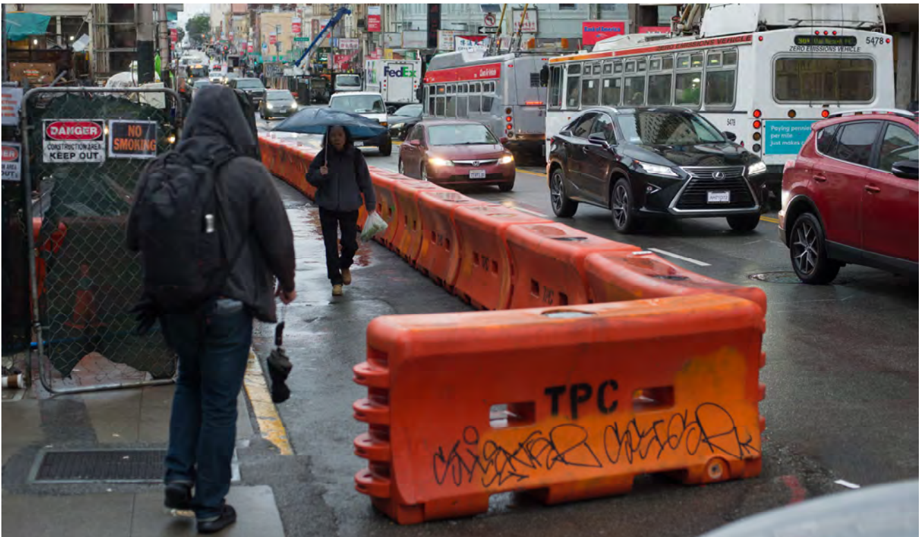
Pedestrians walk the temporary sidewalk adjacent to the Chinatown Station surface work area. This walkway will be temporarily closed again in the coming weeks to facilitate utility upgrades.
