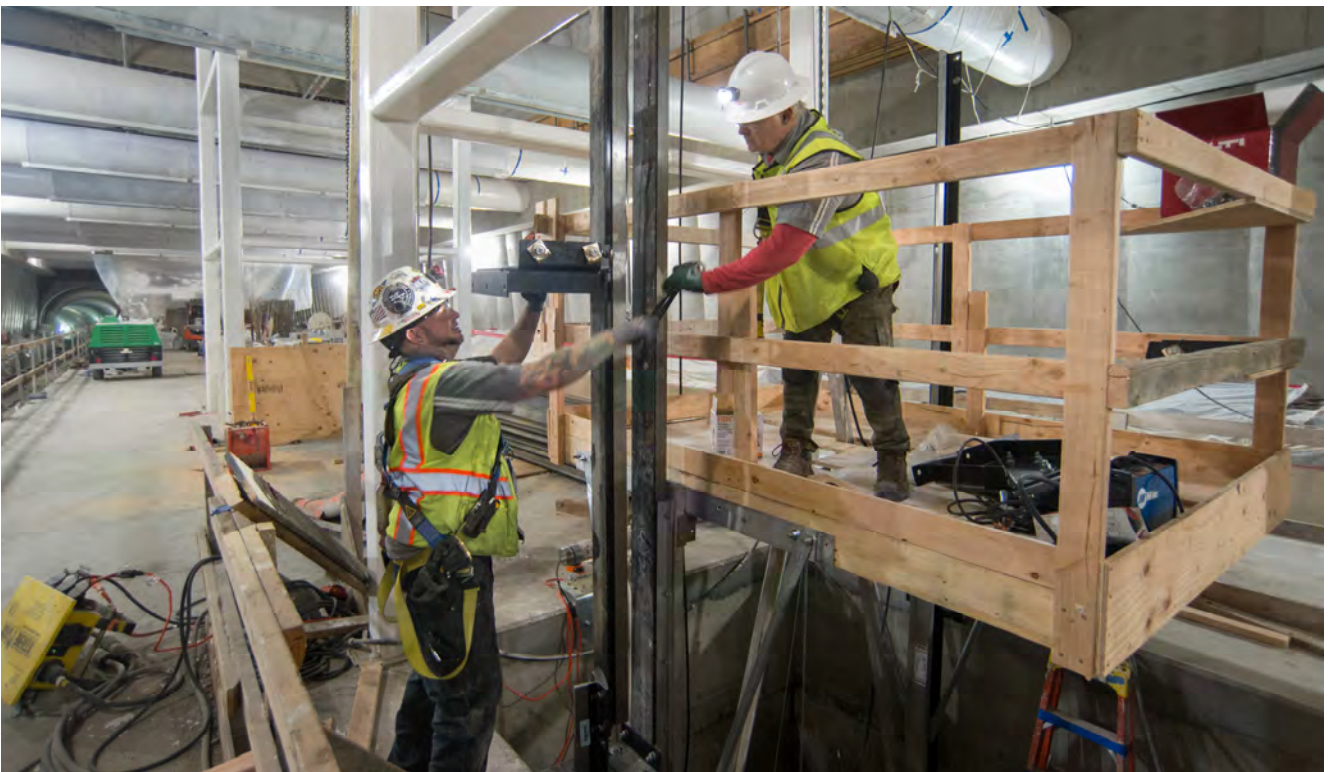
On the platform level of Union Square/Market Street Station, two men pass tools to each other while installing portions of a future elevator mechanism.
