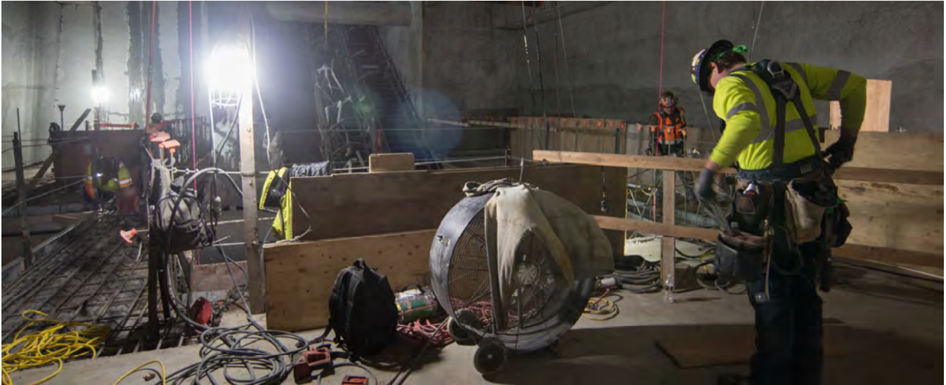
A carpenter on the Mezzanine level pauses near the cut in the south headwall for the Union Square/ Market Street Station where escalators and stairs will carry passengers to and from the platform below.
