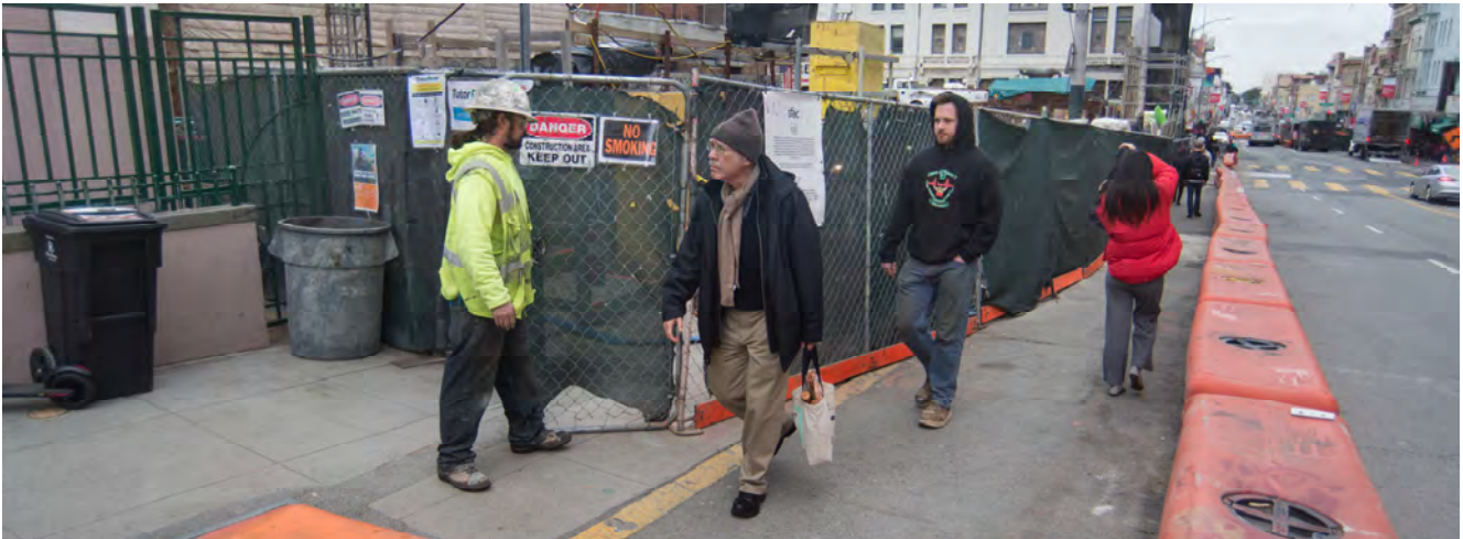
Pedestrians walk down the temporary walkway along the edge of the Chinatown Station headhouse worksite. This walkway may be closed again in the coming weeks following the Chinese New Year to facilitate utility installation.
