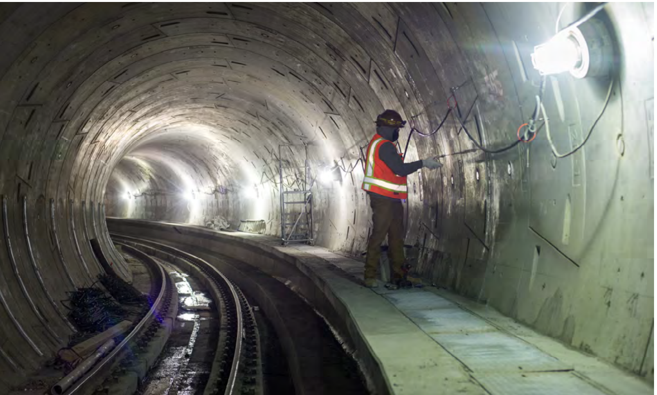
A worker inside the S-curve of the northbound tunnel prepares sections of tunnel wall prior to installing curved brackets to mount utility pipes.
