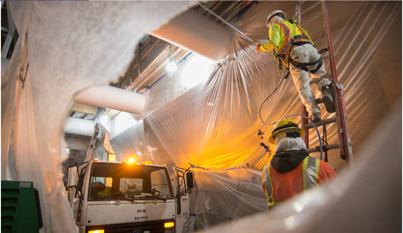
Two crewmembers on the northbound side of the Union Square/Market Street Station platform can be seen painting struts and other interior structural elements, masked off with huge sections of plastic sheeting.
