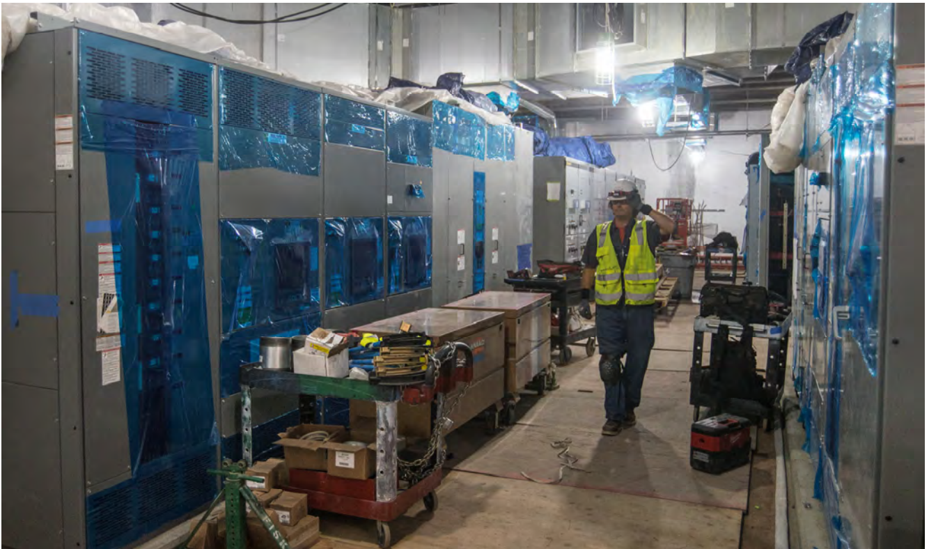
A technician walks the aisles where systems and electrical equipment are being installed inside the north concourse of the Union Square/Market Street Station, just north of Geary under Stockton Street.
