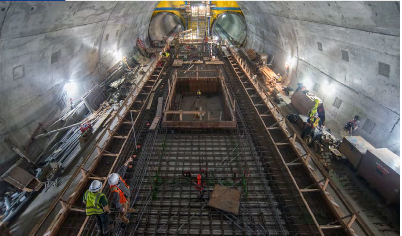
Rebar and formwork are being placed to construct the northern third of the Chinatown Station platform, looking north from the concourse level inside the cross-cut cavern.
