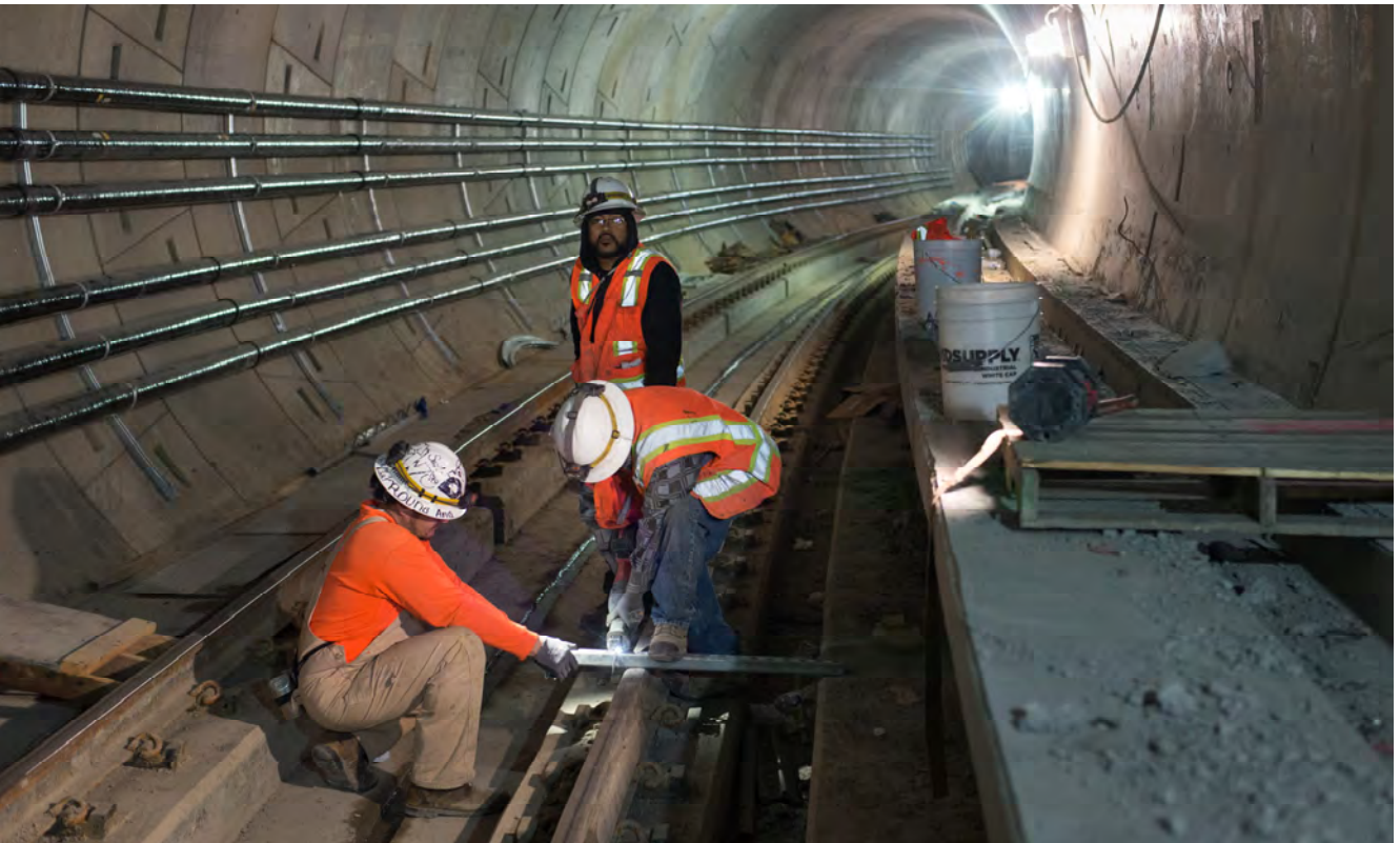
A crew fashions sections of mounting brackets for installation against tunnel walls inside the northbound tunnel as it approaches the Market Street S-curve.
