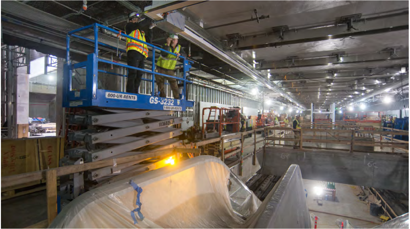
Workers on the concourse level of the Yerba Buena/Moscone Station install a test piece of a section of the finished concourse ceiling design as other crewmembers continue installing utilities and other finishing elements further to the north.
