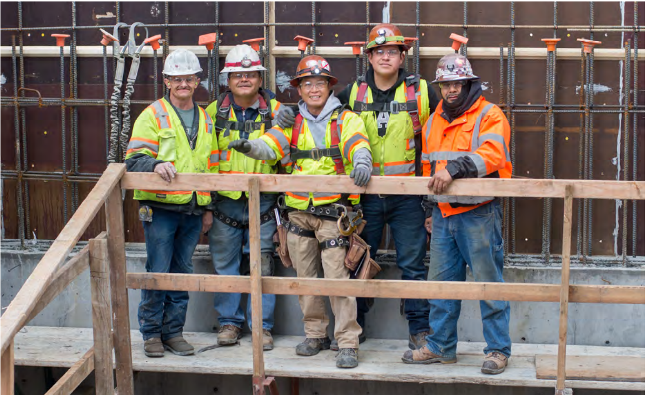
A crew of carpenters stop the Yerba Buena/Moscone Station headhouse poses for the camera against a rebar cage for a surface-level wall being installed at the south edge of the main shaft for escalators and stairs.
