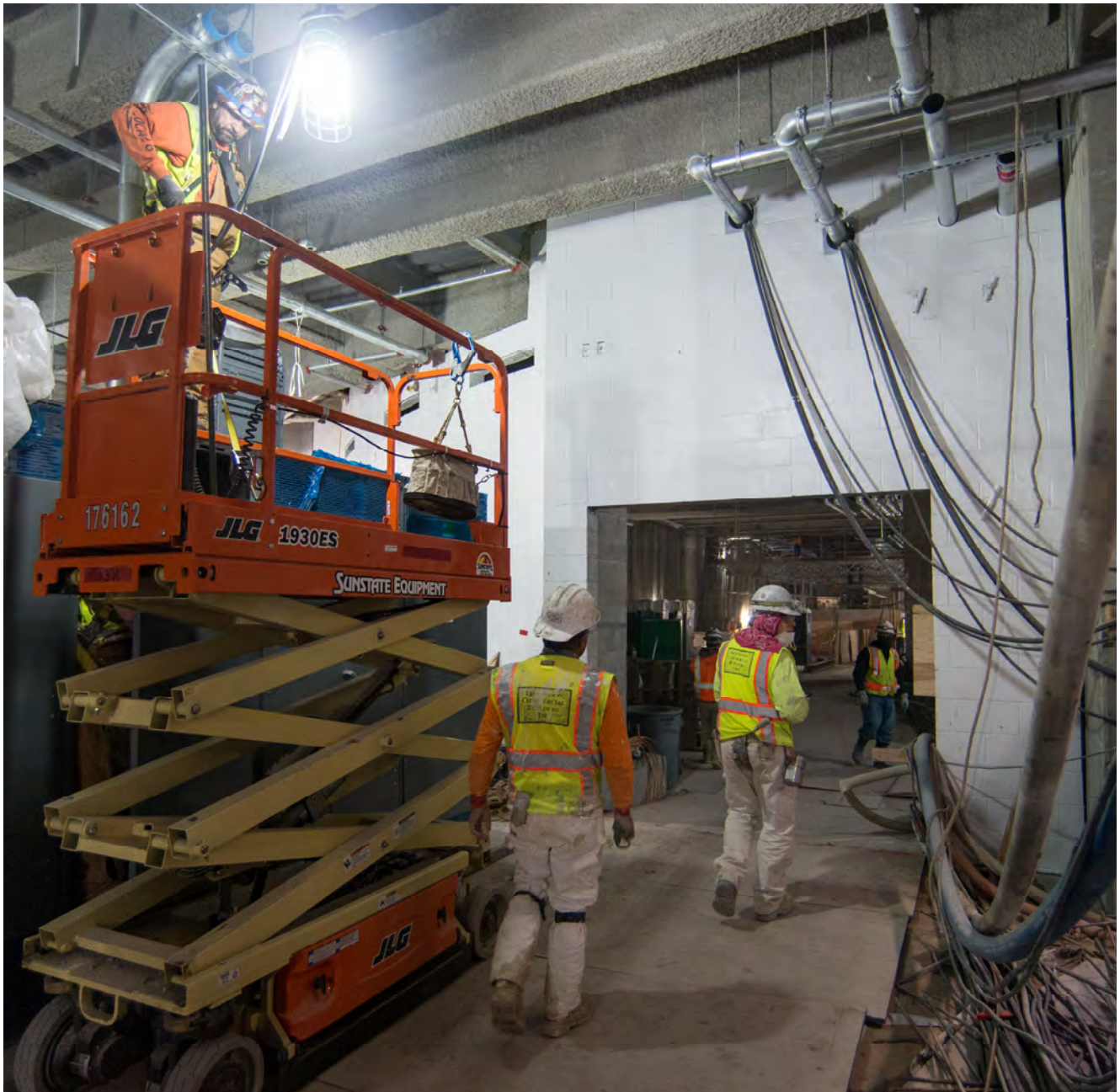
Temporary utilities wind their way around permanent conduits being installed inside the upper level of the north concourse inside Union Square/Market Street Station.
