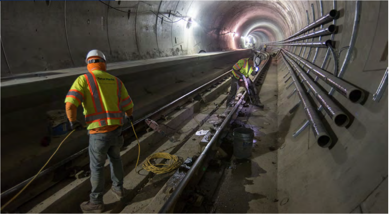
Workers use various air-powered tools to remove debris and clean this section of the northbound tunnel just south of the Market Street S-curve, following the installation of utility pipes along the east wall.
