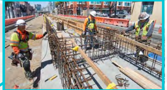
4th St. Surface Track, Systems (STS)
