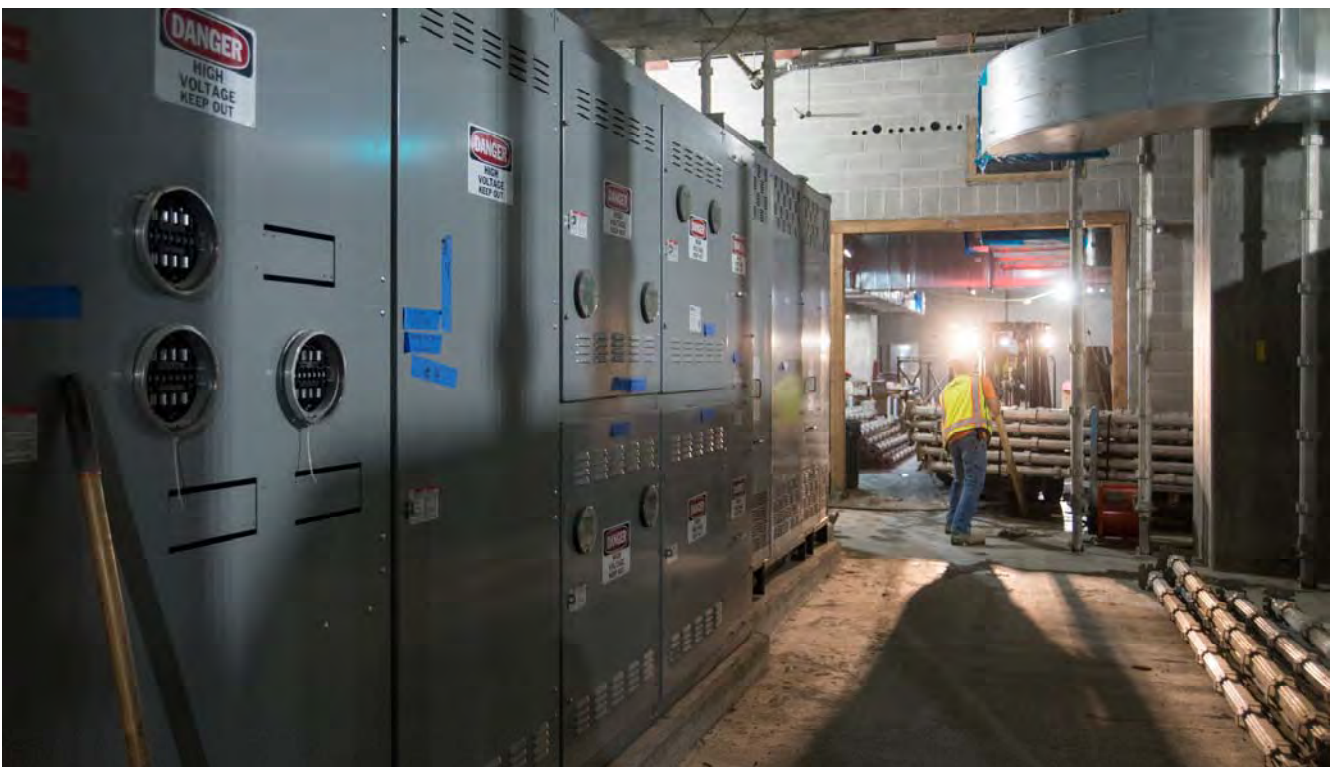
Track control, electrical systems, and other utilities continue to be installed on the lowest level of the Yerba Buena/Moscone Station headhouse.
