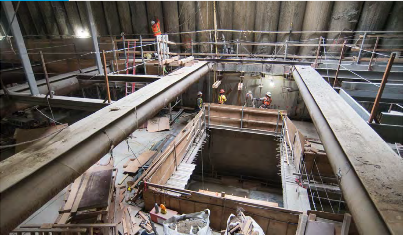
Light pours in the O'Farrell access shaft onto workers constructing supports and formwork for reinforced concrete beams spanning along the outer walls of the station box.
