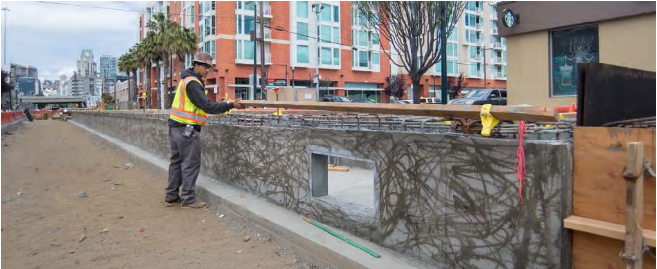
A worker removes temporary formwork atop the platform foundation walls, which have recently been poured. A concrete curing solution sprayed onto the surface left swirled markings.
