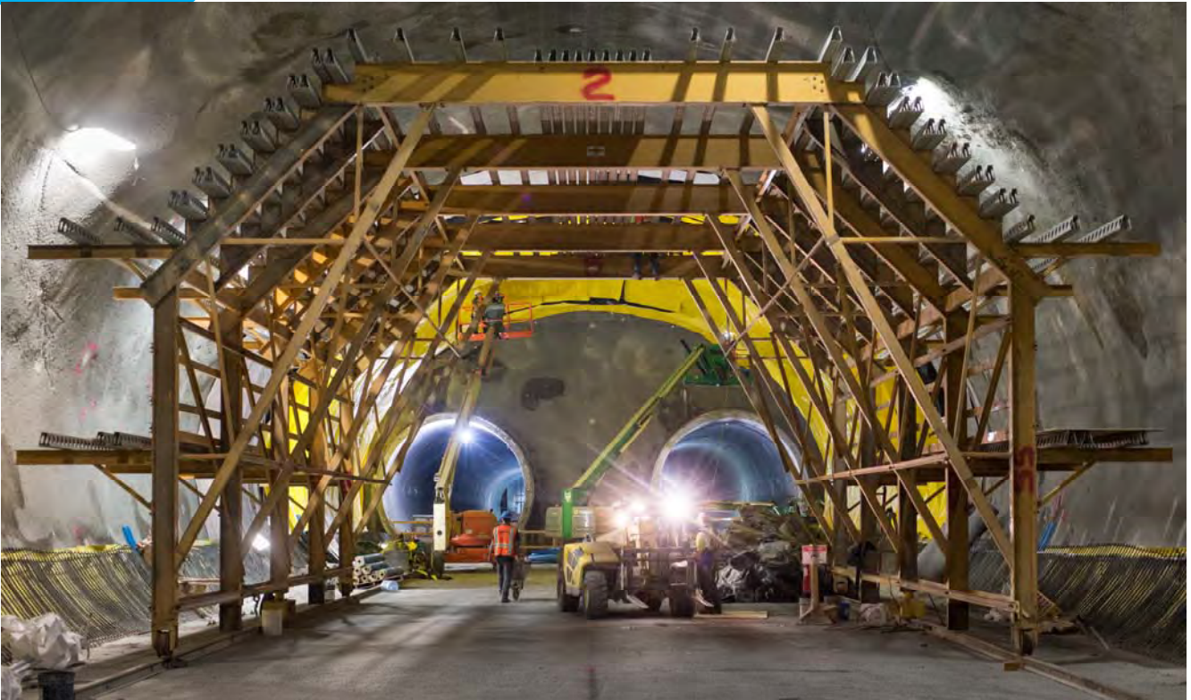
A large, rolling scaffolding structure is being assembled at the south end of the Chinatown track crossover cavern, which will be used to install waterproofing, rebar, and concrete forms against the upper portions of the cavern shell.
