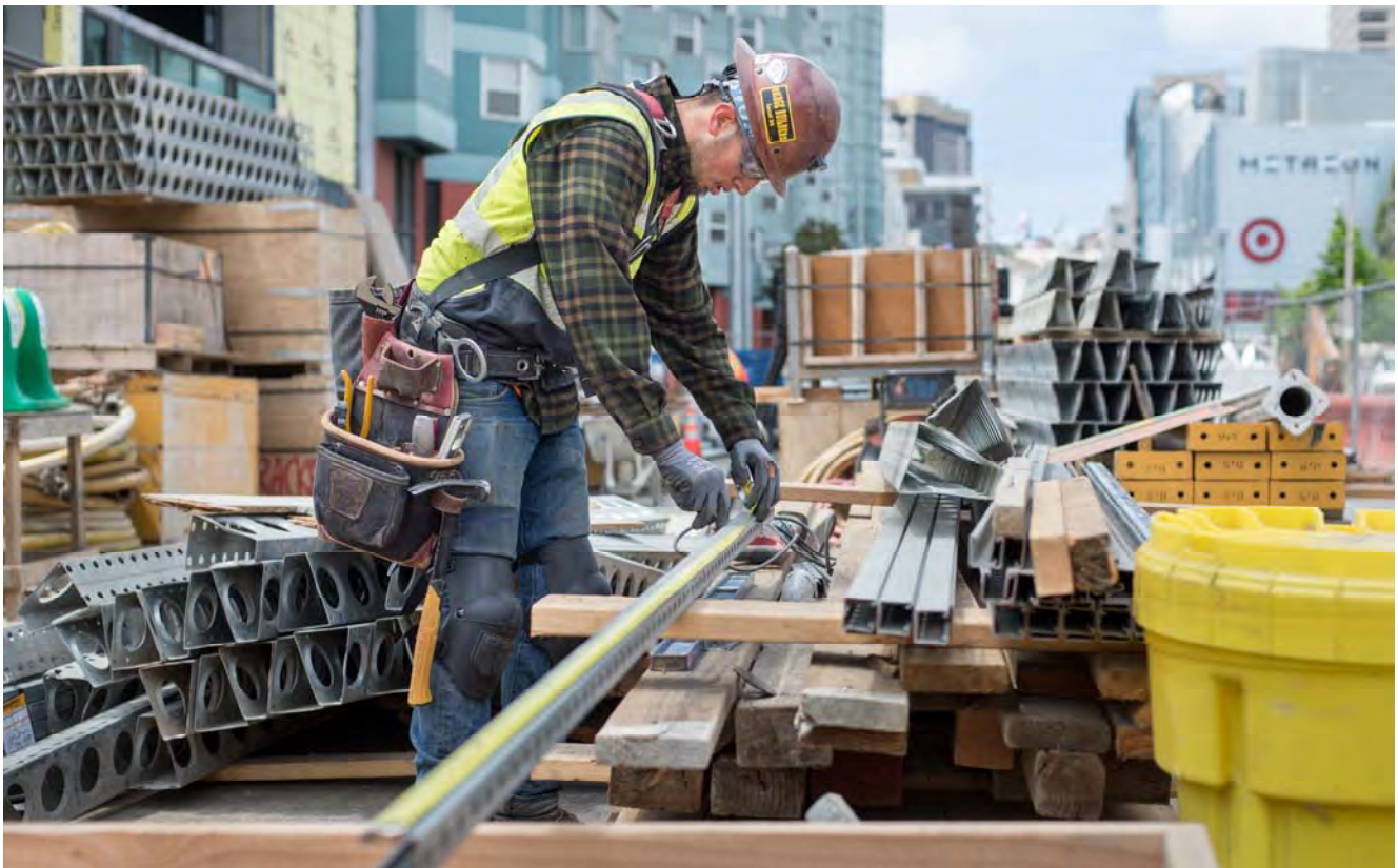
A worker marks out sections of steel brackets used as part of interior utility work for the Yerba Buena/Moscone Station.
