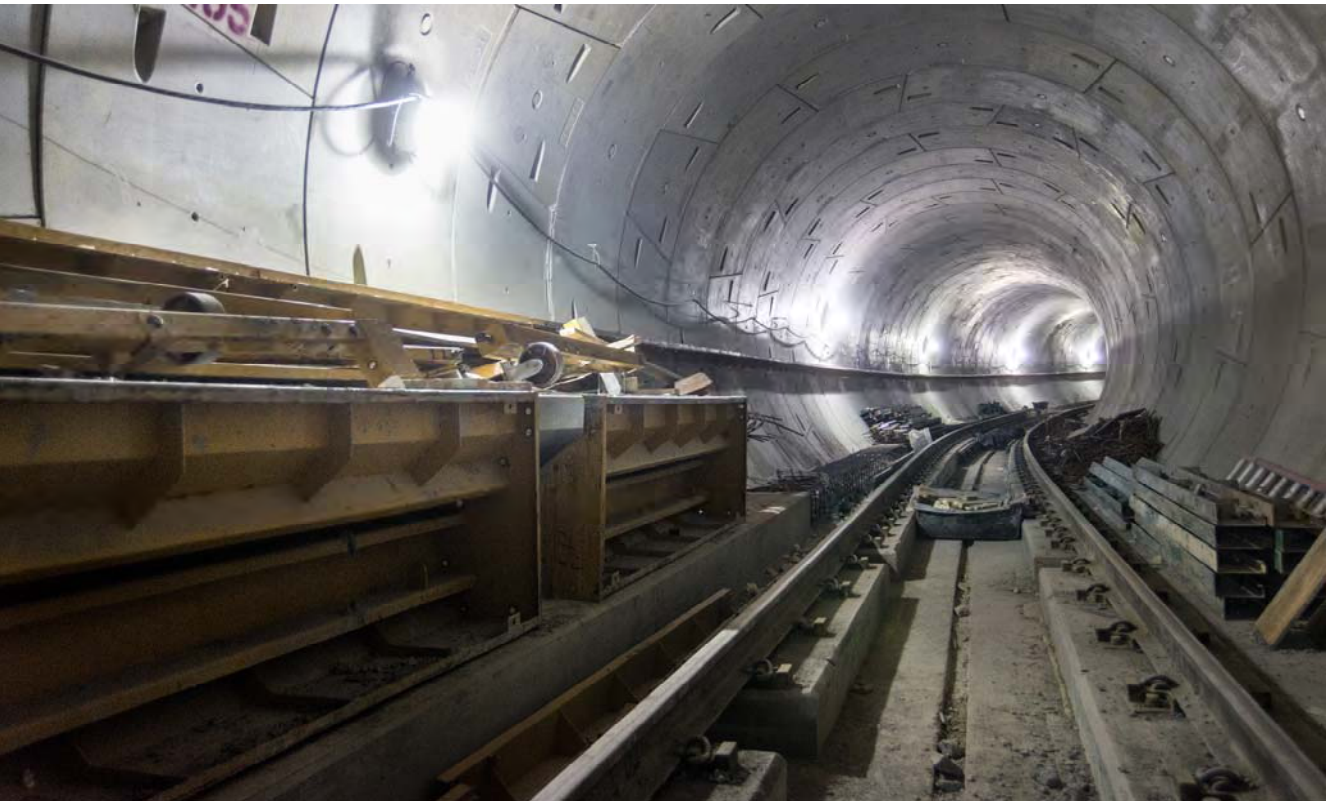
Looking up the northbound tunnel, crews have constructed tunnel walkways up to the S-curve under the Market Street subway.
