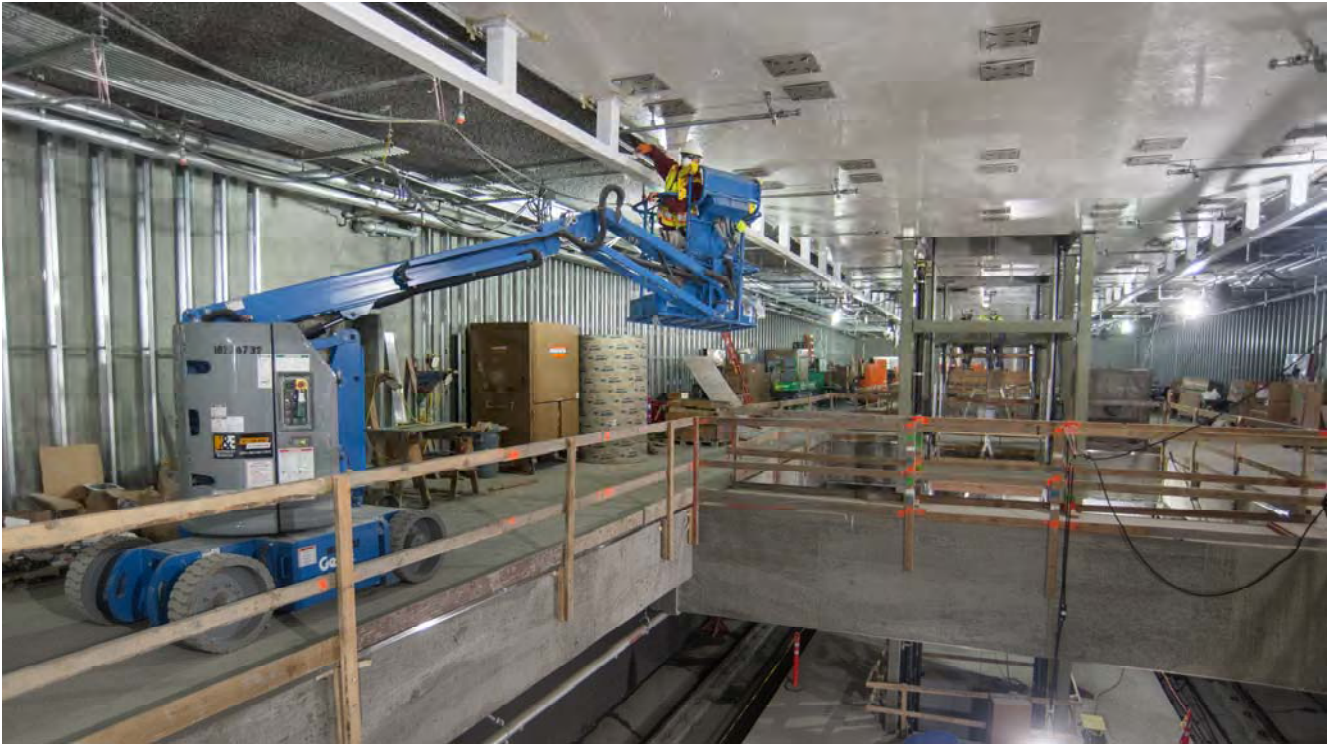
Interior work and utility installation efforts continue inside the Yerba Buena/Moscone Station box, near Clementina and 4th Street.
