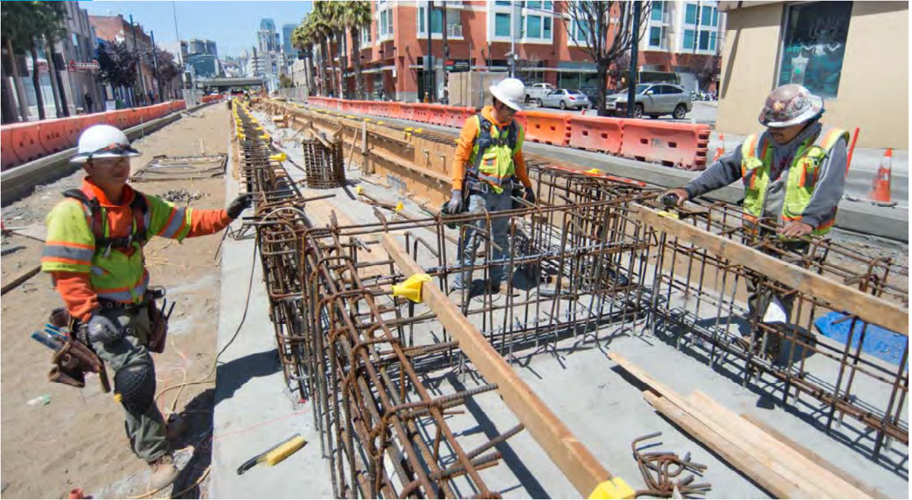
Workers continue to install utility conduits and concrete forms as part of surface platform construction at 4th and Brannan.
