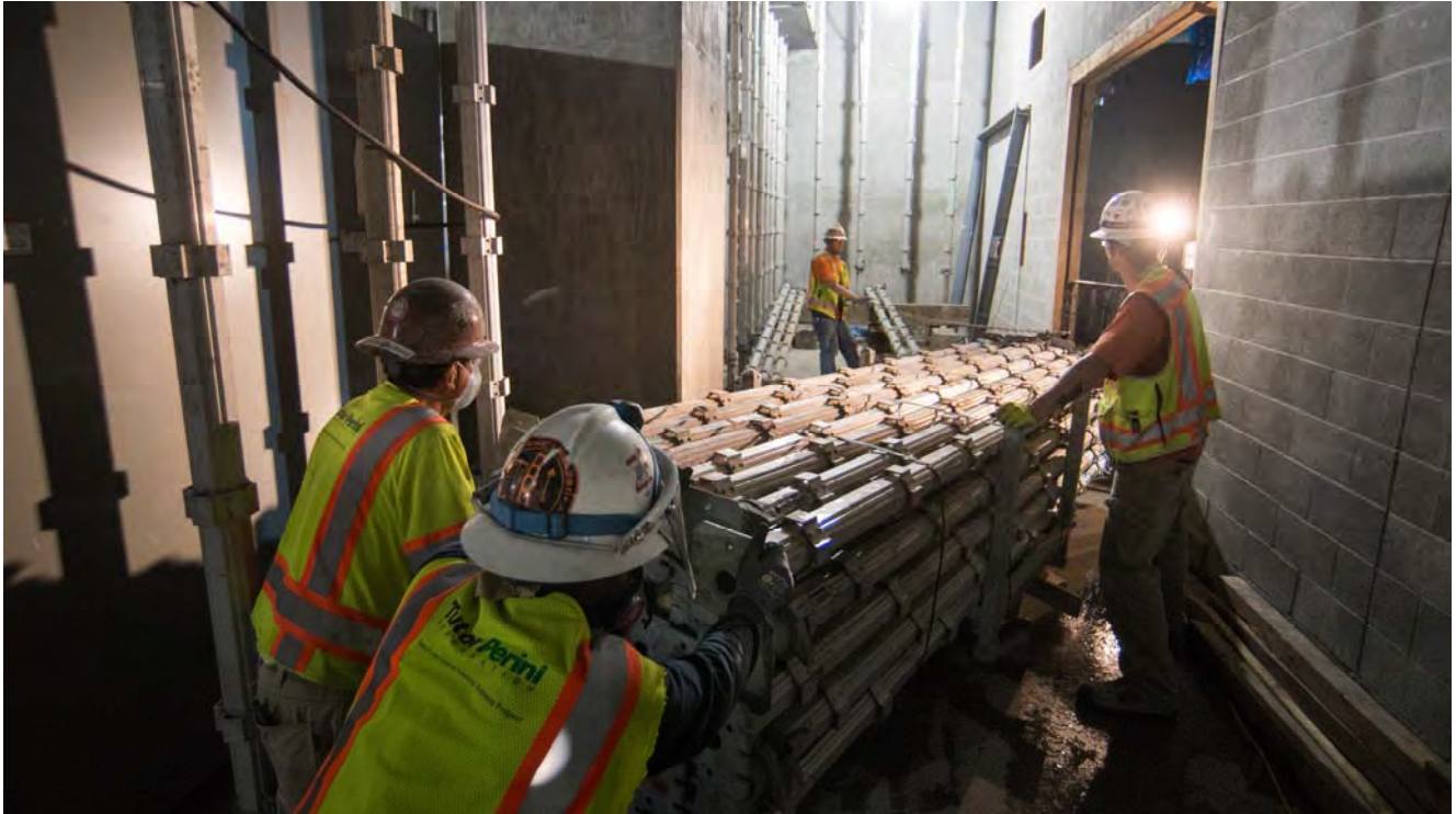
A team carefully maneuvers bundled scaffolding through a narrow walkway at the bottom level of the Yerba Buena/Moscone Station headhouse.
