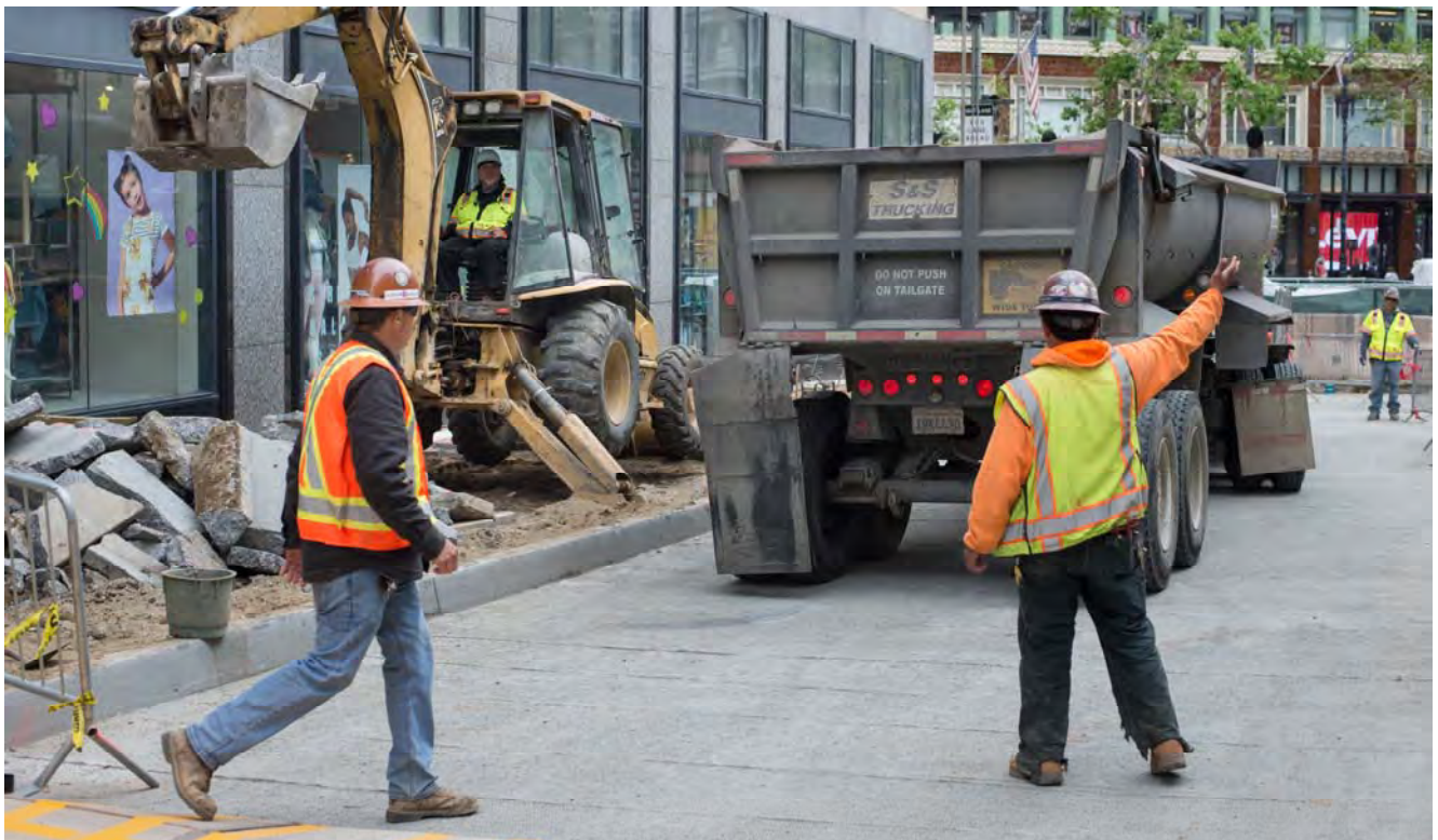
Workers position a truck to be filled with concrete removed from the east sidewalk of Stockton Street north of Ellis, which is slated to be rebuilt as part of roadway restoration work.
