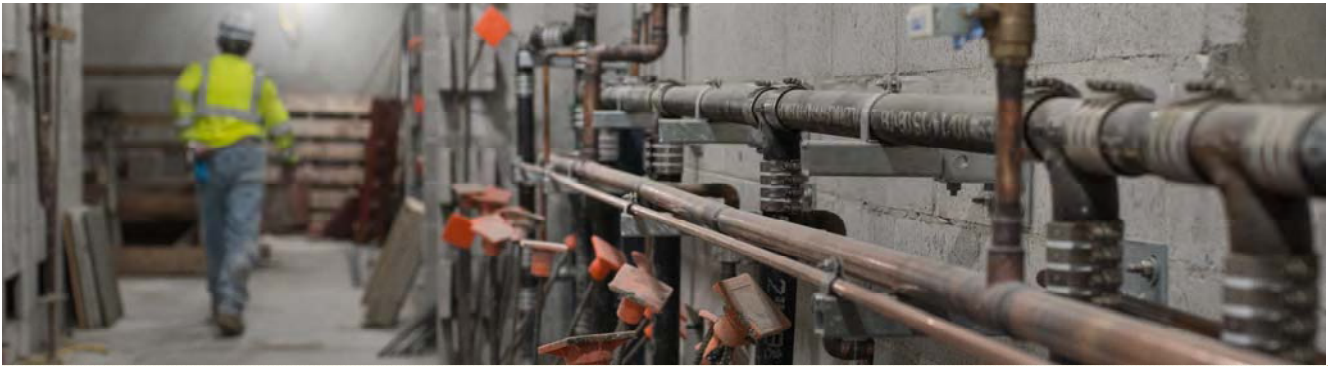
Newly-installed plumbing lines an interior wall on the concourse level near the north end of the Yerba Buena/Moscone Station headhouse.
