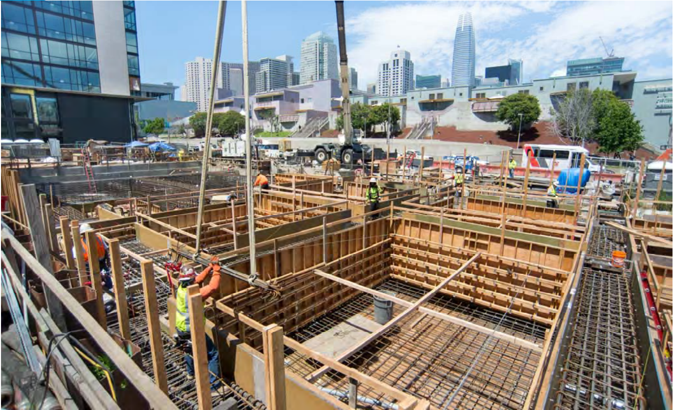
A worker receives a bundle of rebar to be installed on the west side of the massive headhouse roof slab, currently under construction.
