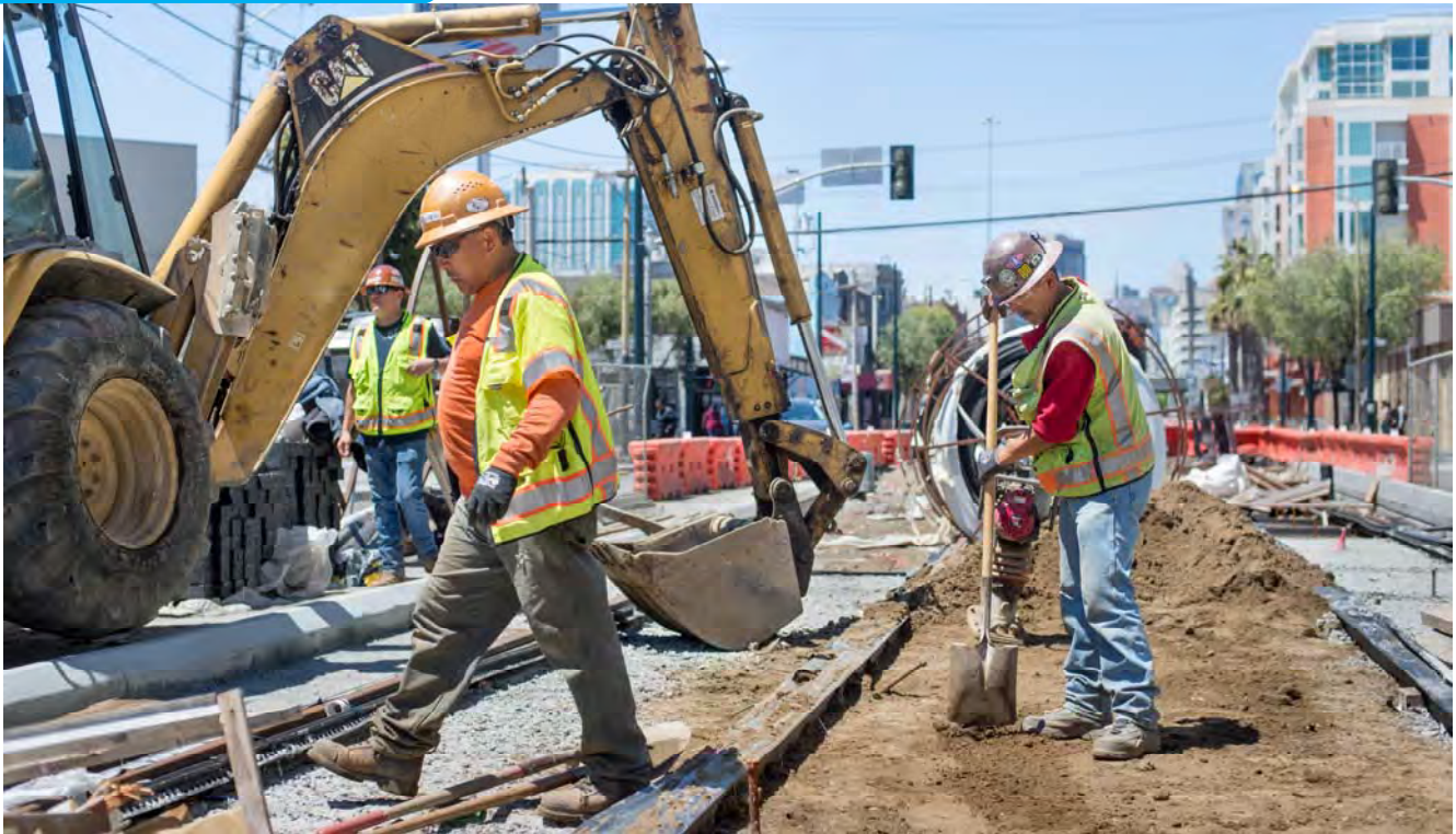
The center of 4th Street between the two trackways is being backfilled with soil to prepare for additional concrete work.
