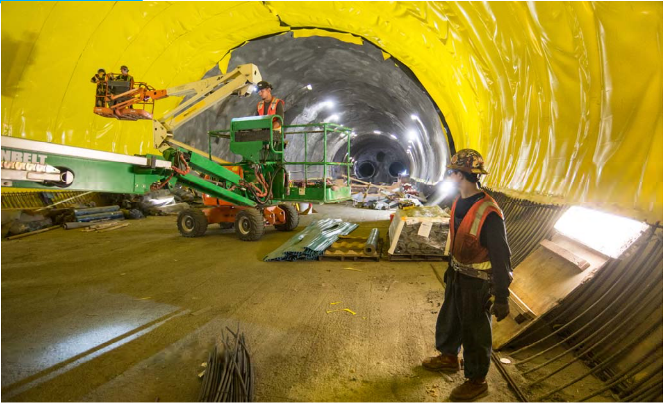
Workers on a variety of boom lifts install and inspect waterproofing against the exterior shell of the Chinatown track crossover cavern.
