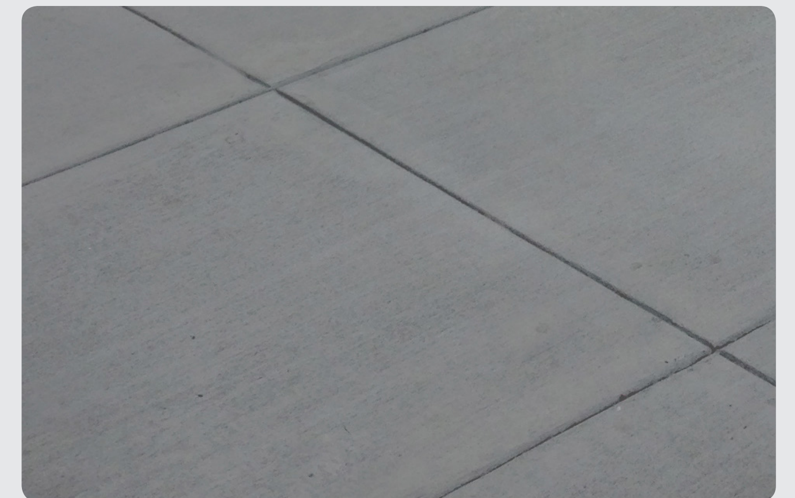
Dark Grey Integral Color Concrete in Path of Travel B without sparkle grain finish
