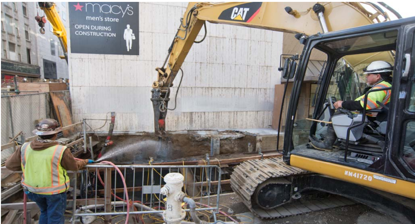
Concrete is removed from around the tops of soldier piles surrounding emergency egress stairs on O'Farrell as part of cleanup work ahead of the 2017 Winter Walk.
