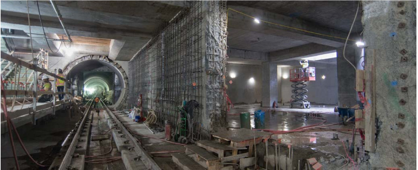
View looking down the southbound track inside the Yerba Buena/Moscone station box, with workers having recently removed scaffolding from the platform level of the headhouse (photo right).
