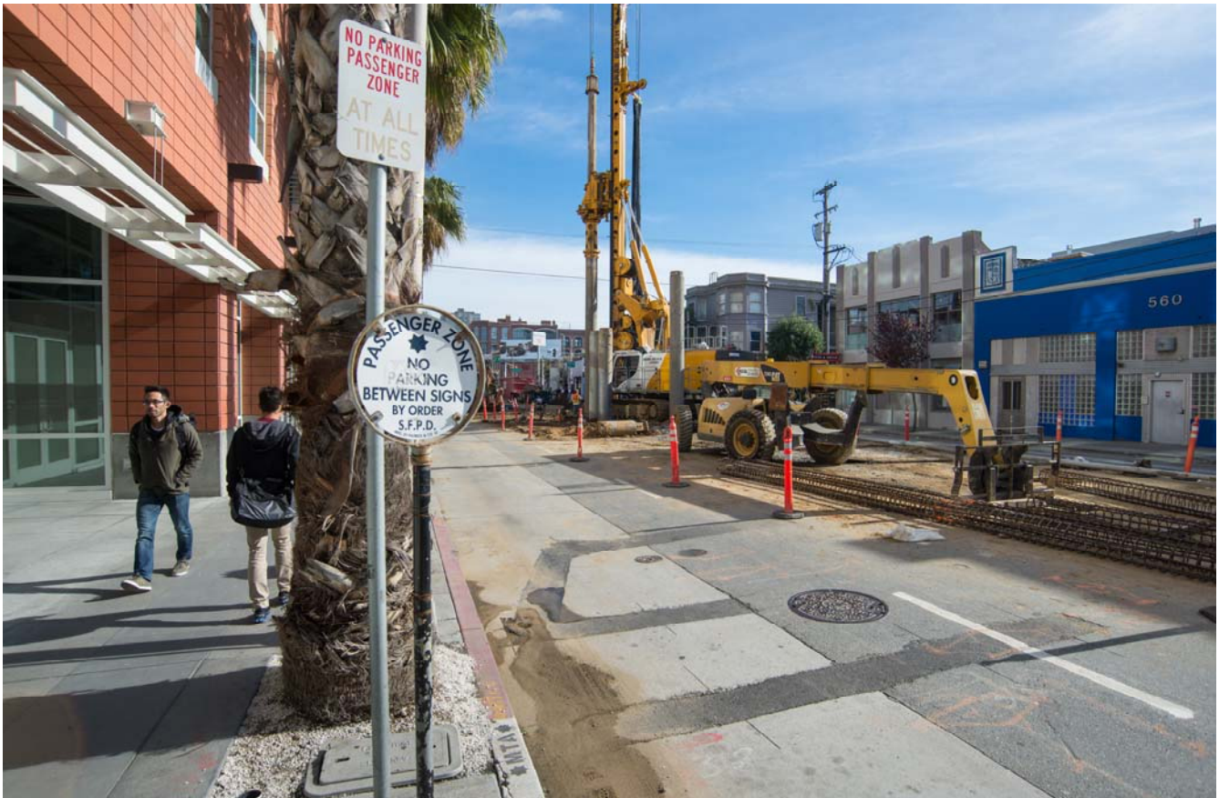
Installation of piles to support the future 4th and Brannan surface station is underway north of Brannan - see 4th Street Surface Station Platform Pile Progress on page 26.
