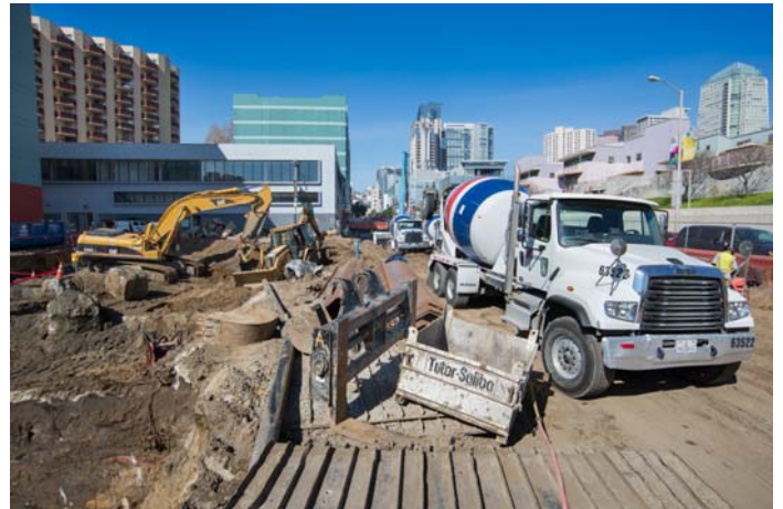
A concrete truck backs into the site, to deliver material used to build part of the roof slab.
