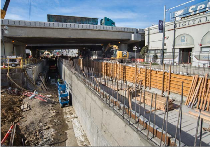
1 Exterior walls and other structural elements of the tunnel portal are constructed
