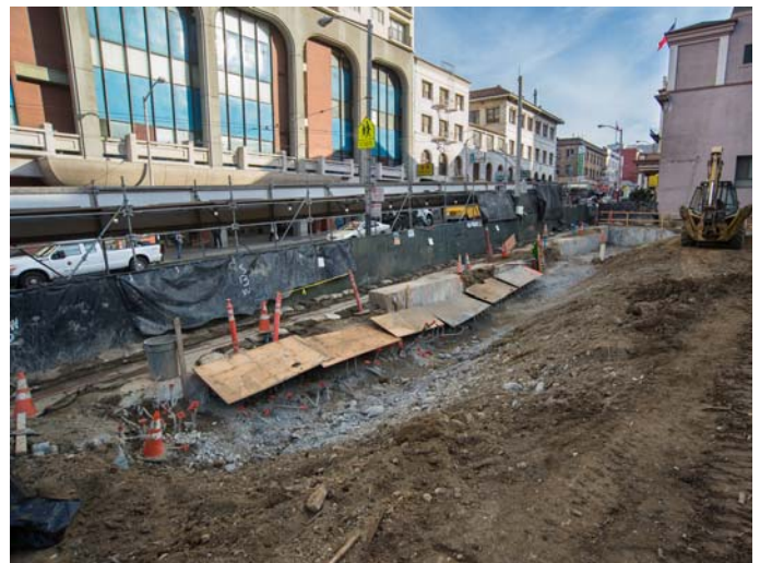
These plywood boards cover exposed rebar, which will be attached to the future roof slab.
