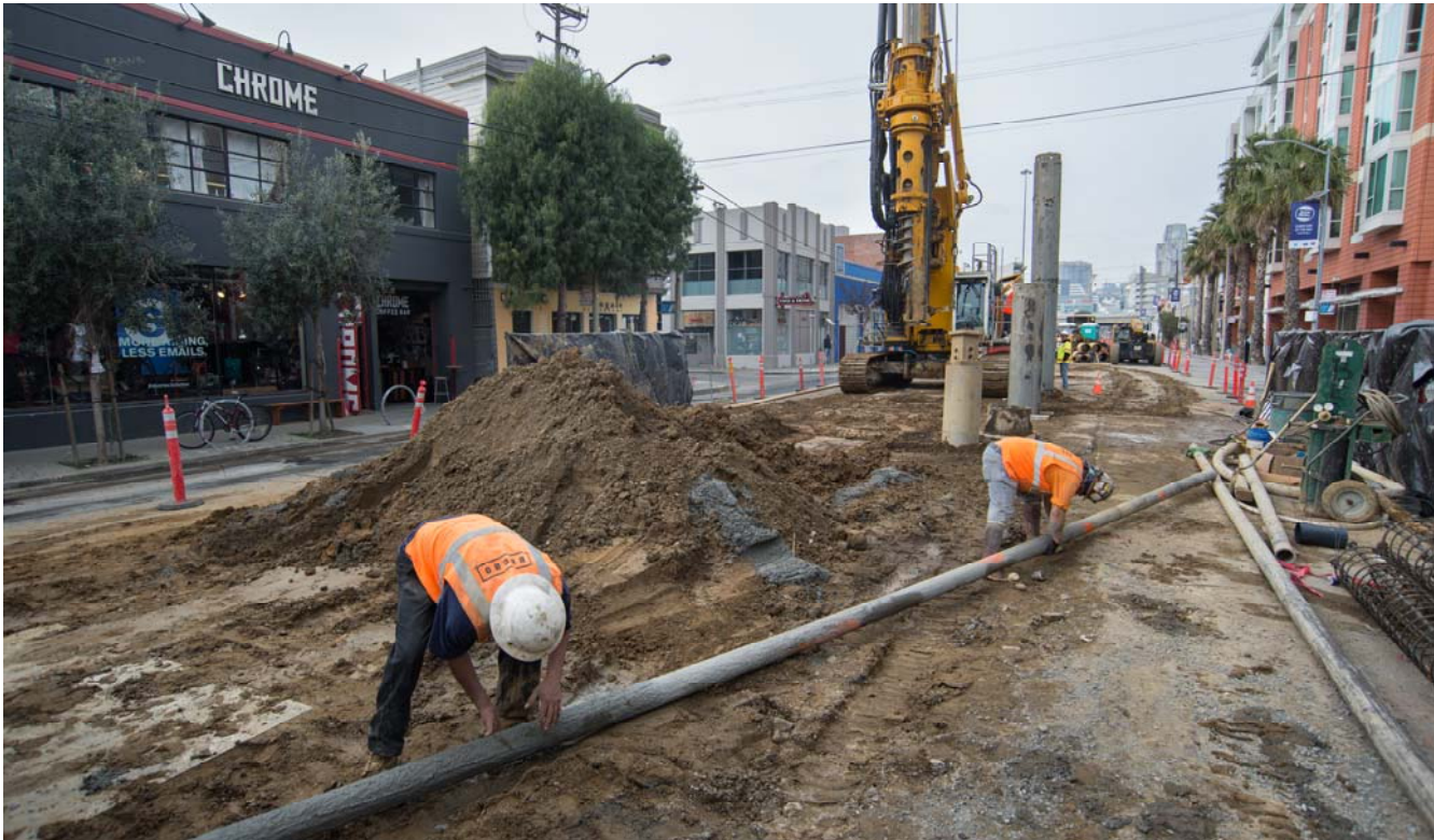
Workers can be seen here moving piping used to pump concrete to the bottom of these foundation pile shafts.
