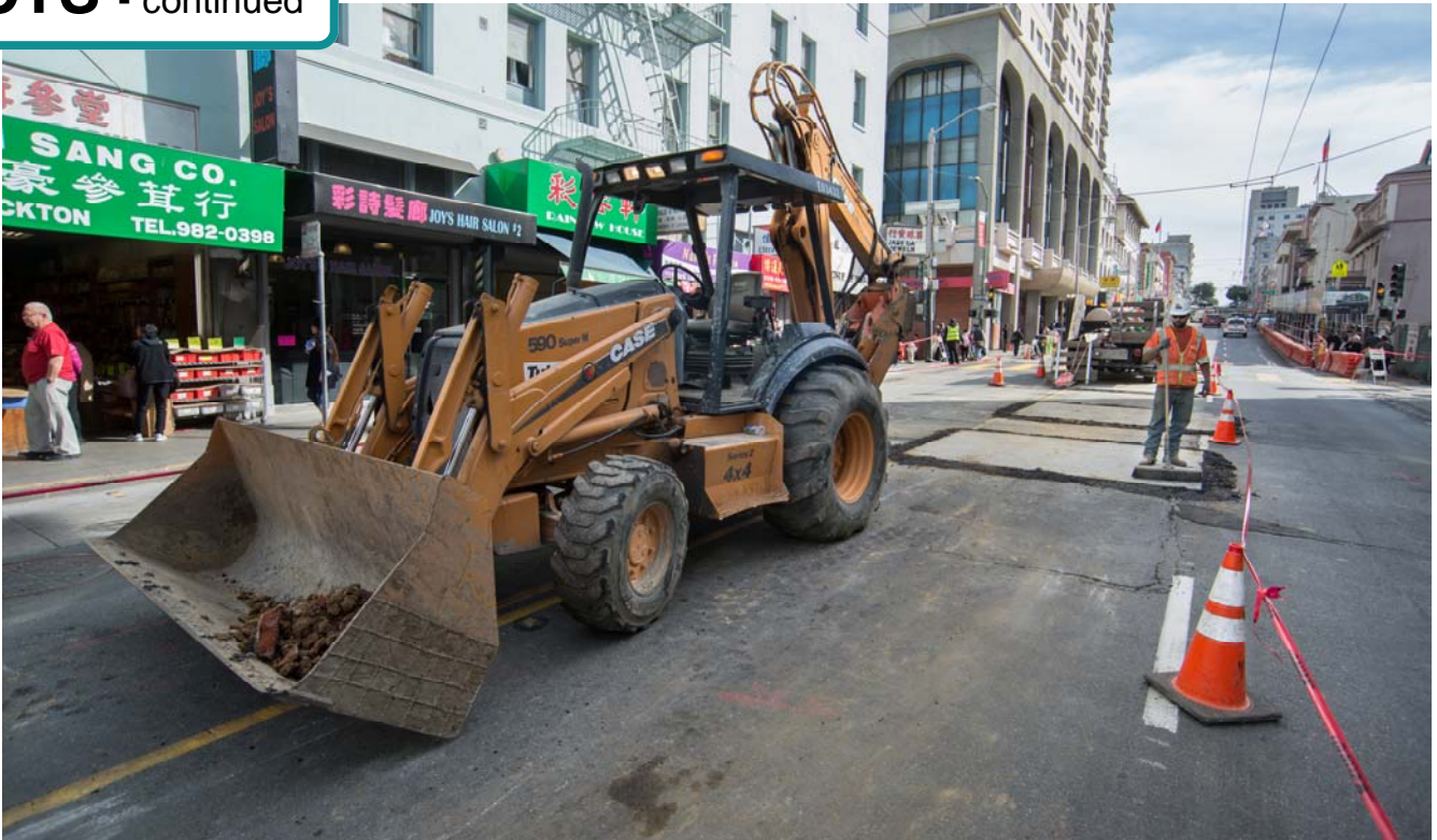
Work to install a new sewer is underway on Stockton between Washington and Jackson.
