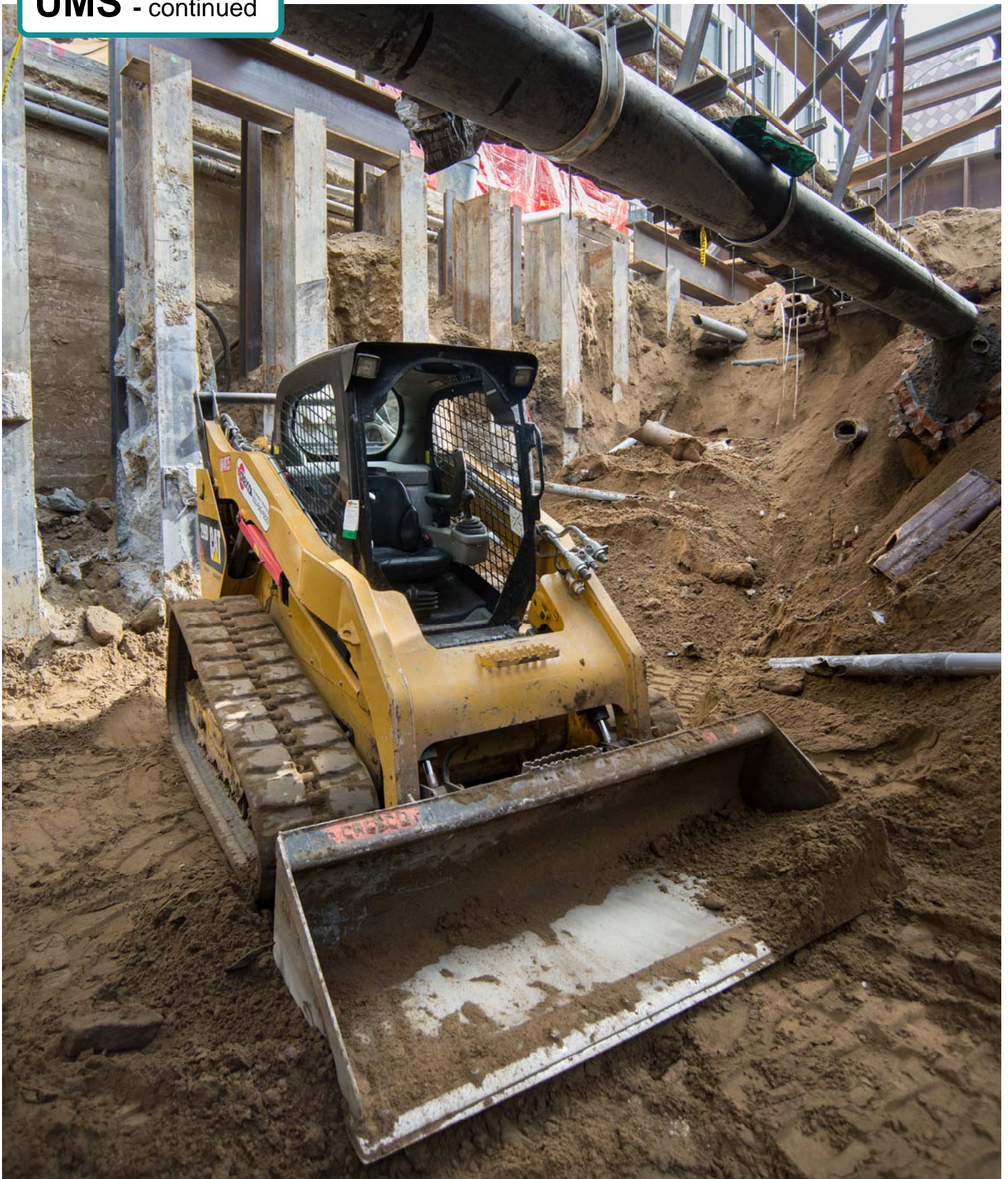
North of Geary on Stockton, workers are methodically reinforcing and hanging active utilities from a truss suspended above the roadway, while excavating soil from below.
