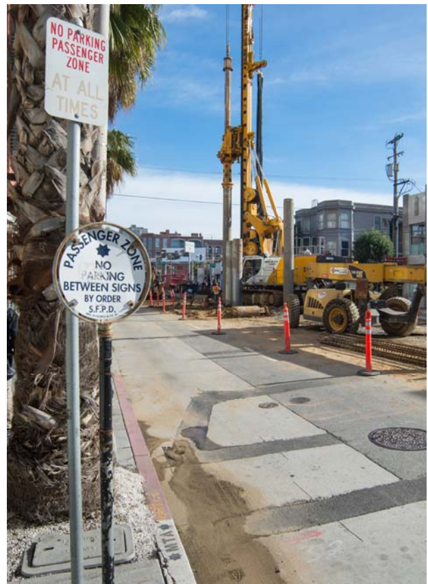
Parking has been removed from 4th Street adjacent to foundation and utility work.
