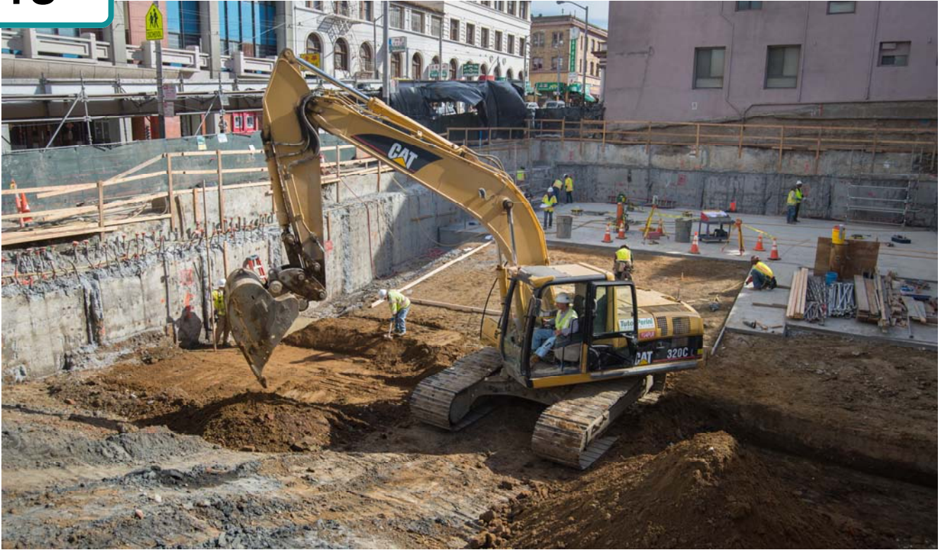
A temporary “rat slab” is being constructed as the bottom of a form which will be used to build the future roof slab of the station.
