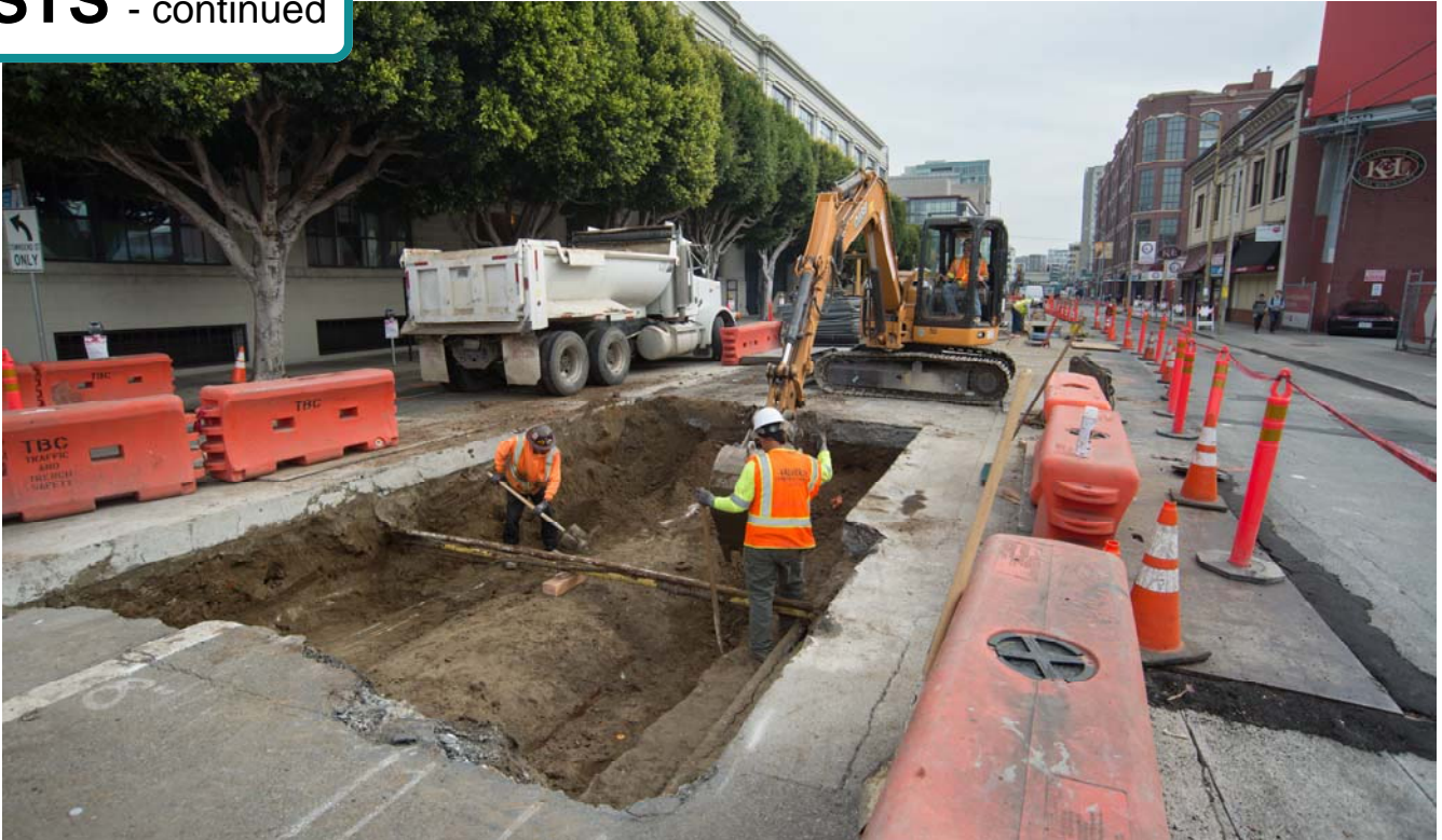
A crew uncovers the arched brick top to a 48-inch sewer just south of Brannan on 4th Street. This sewer will be rebuilt to sustain the weight of trains passing overhead.
