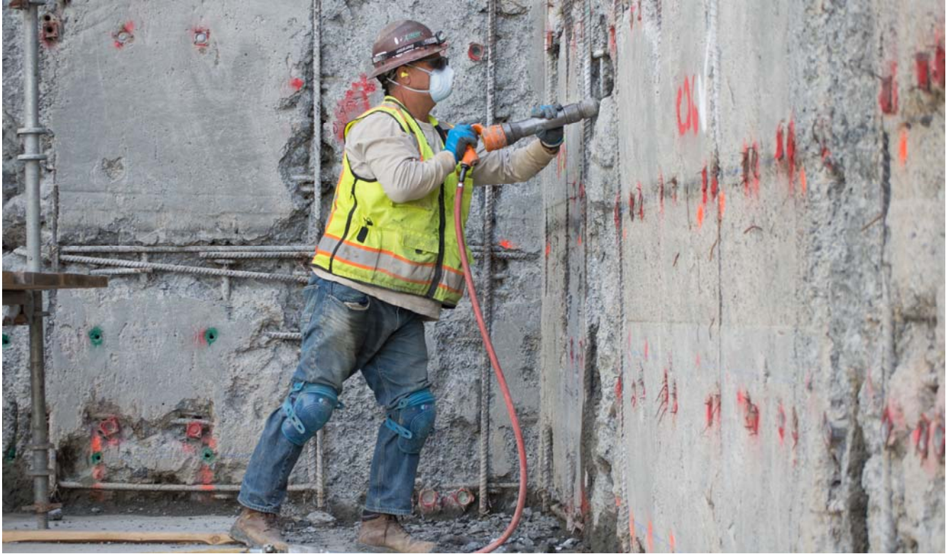
Workers use pneumatic jackhammers to expose rebar, which will be tied in with rebar used in the future roof slab.
