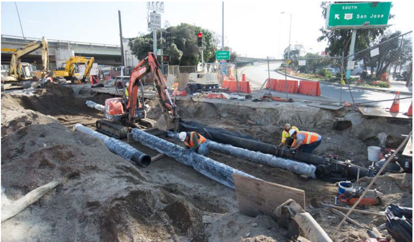
At the northern end of the tunnel portal site, the already-completed roof has been back-filled. New utilities are being installed here, which will eventually extend to Bryant.
