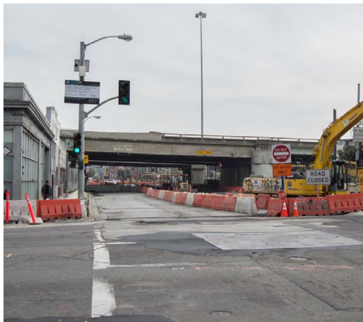
3 The concrete slab is poured and the roadway is reopened in phases
