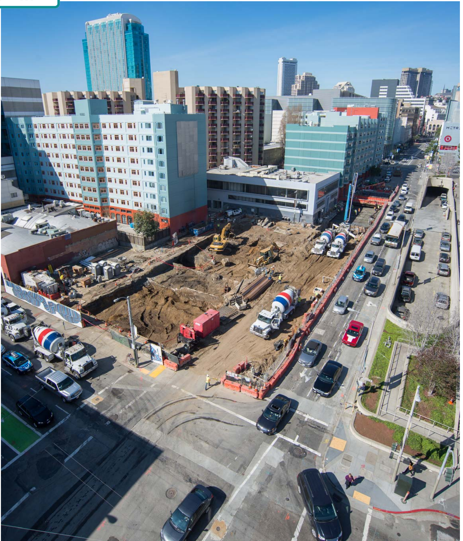
Work to remove underground obstacles to further construction is ongoing at Yerba Buena/ Moscone. Basement walls of former buildings were discovered and removed.
