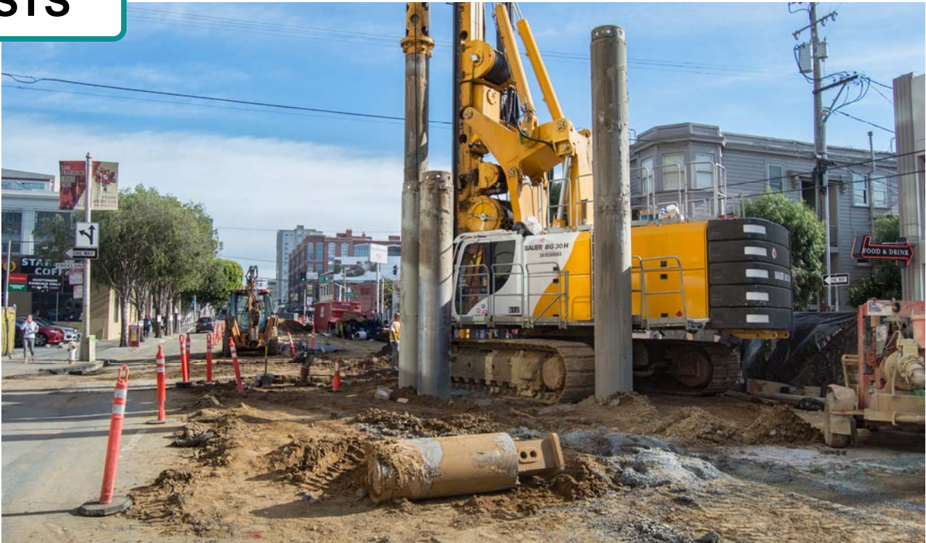
These steel shafts are drilled into the ground and used to hold back soil while an auger removes it inside. Later, rebar is lowered into each shaft and concrete is poured.
