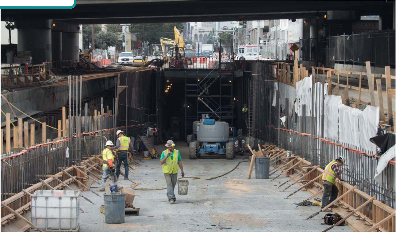
Looking northwest up 4th Street, and into the mouth of the future tunnel portal, workers first install waterproofing barriers before rebar and concrete forms.
