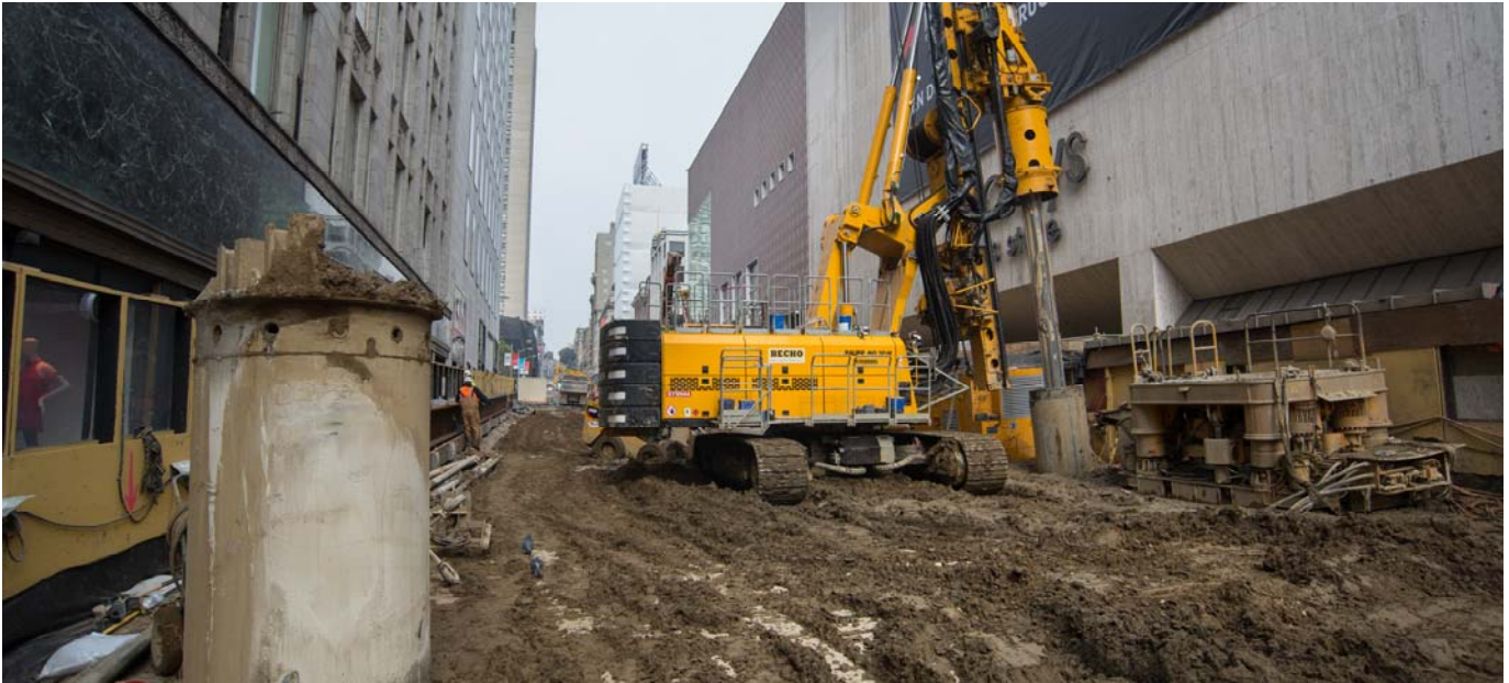
Few exterior wall piles remain to be constructed at the Union Square/Market Street Station site. This work will be wrapped up in the coming weeks.
