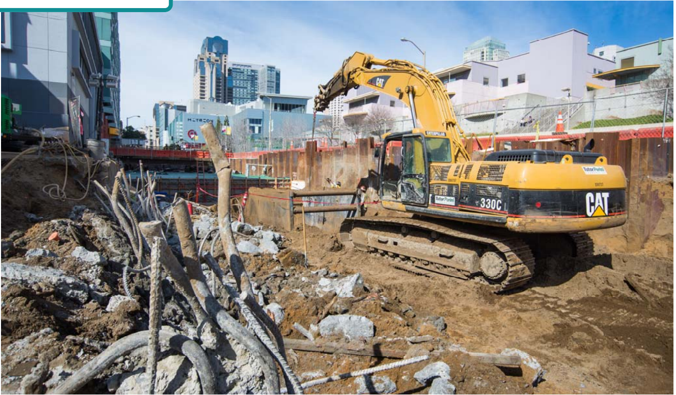
Exposed rebar seen here will be tied into rebar installed for the future roof slab. The roof slab will be constructed in sections, and will be made of reinforced concrete.
