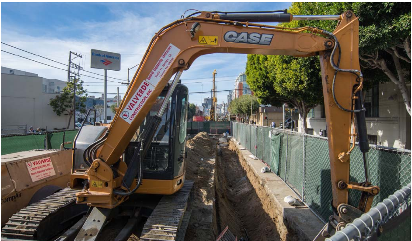
A mini excavator sits waiting to be used for utility excavation the next day.
