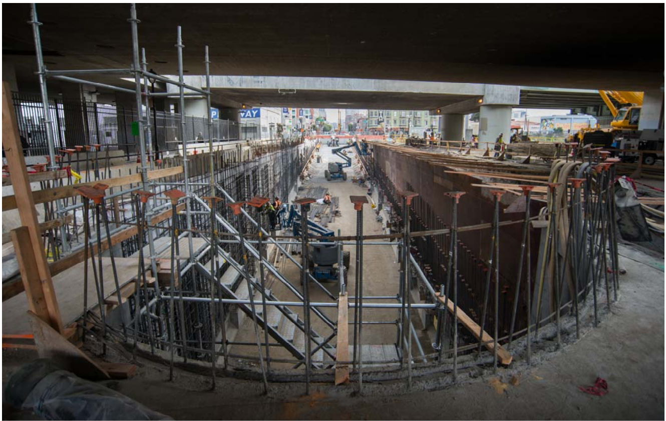
Looking southeast from the crest of the tunnel portal roof, work below to construct the exterior walls is well under way.
