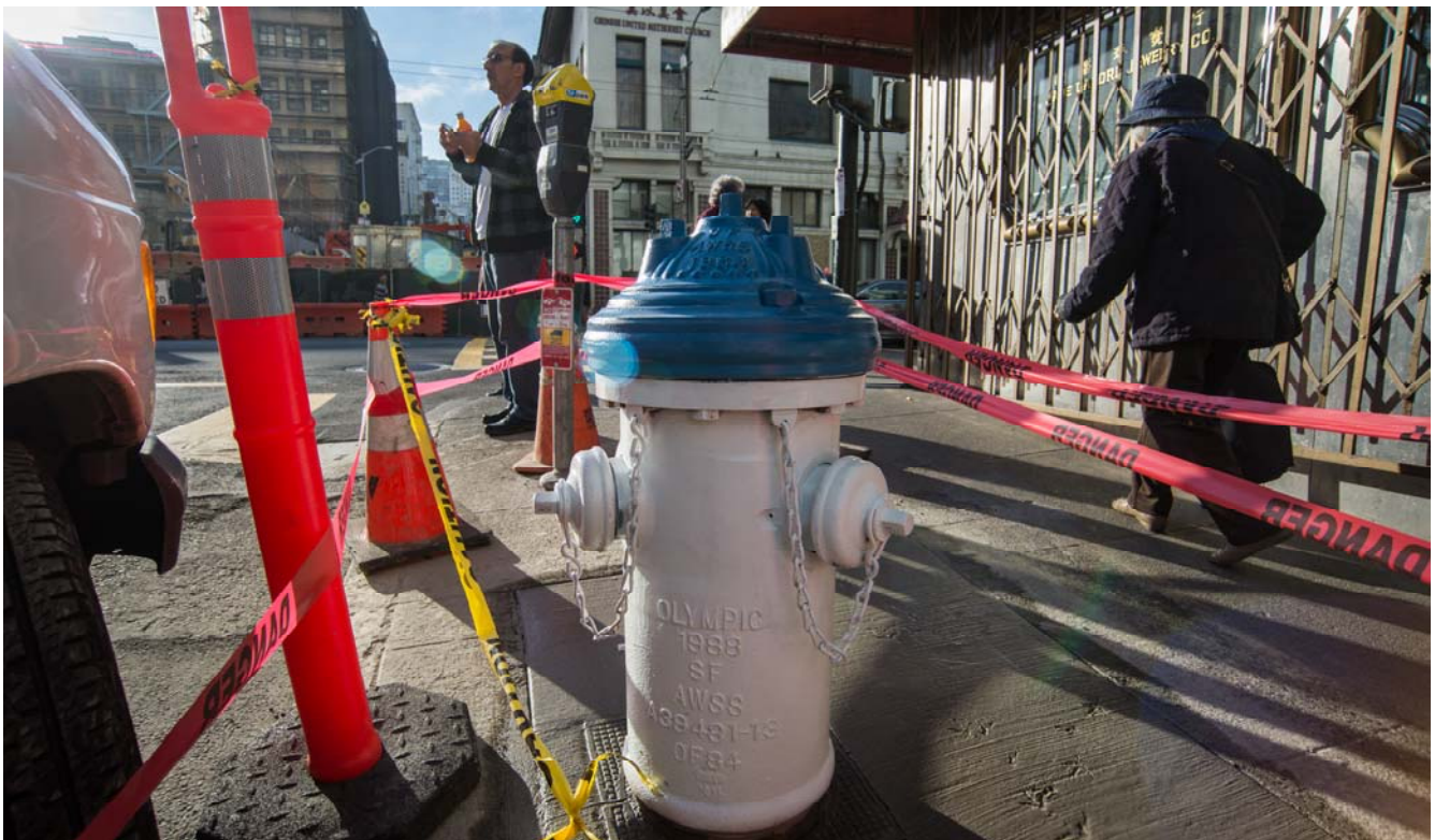
This auxiliary fire hydrant was added to the northeast corner of Stockton and Washington.
