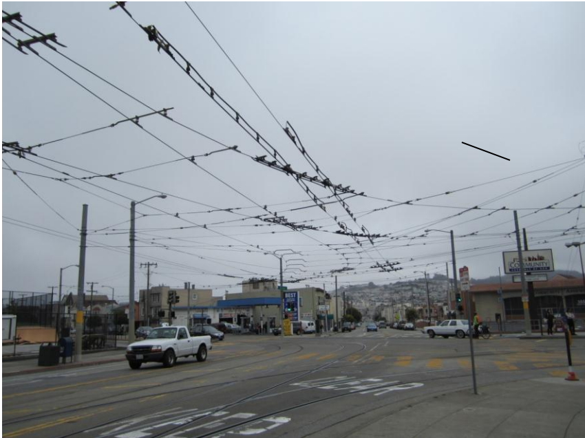
Area 3 Muni Overhead wires
