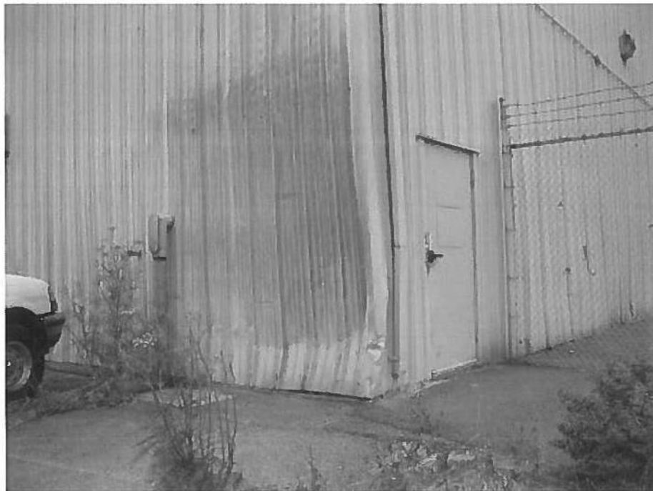
Photograph #9 -View of northwest corner of building, note damage
