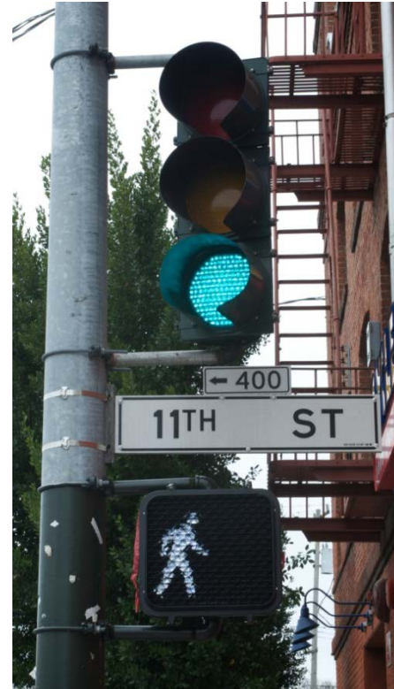
Modern traffic signals
