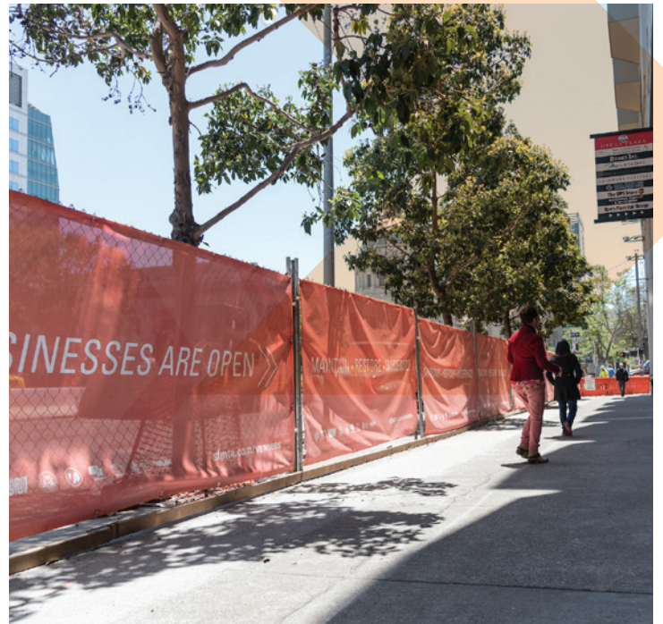
Van Ness Improvement Project mesh has been installed on fences facing the sidewalk all along the corridor.
